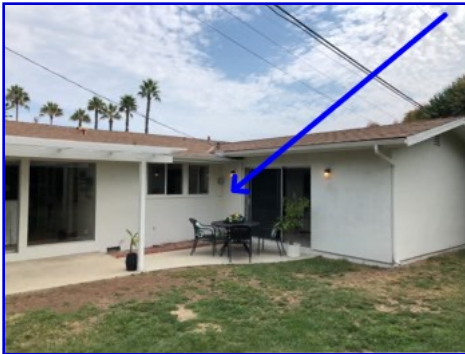
MAIN ELECTRICAL PANEL
