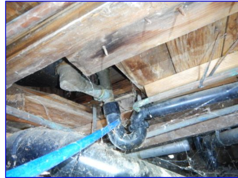
Leaking under tub
