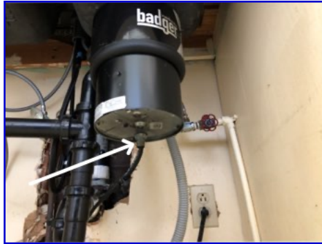
Noisy; Missing wire grommet
