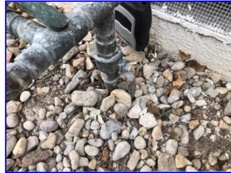
MAIN WATER VALVE
