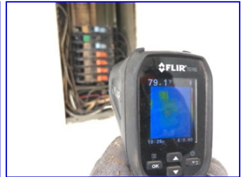
Thermal Image View - Normal temperature readings with no visible signs of overheating at time of inspection
