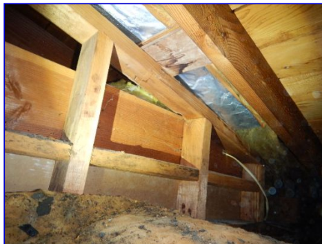
Microbial growth; Stained; Deteriorated wood
