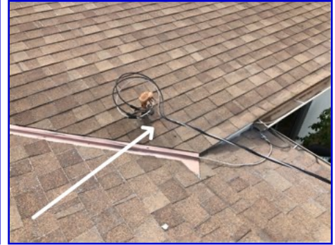
Reroof covers flashing
