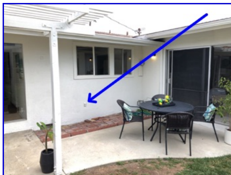
Not GFCI protected
