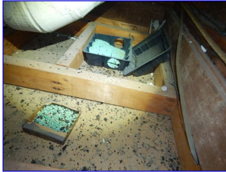
Evidence of rodents
