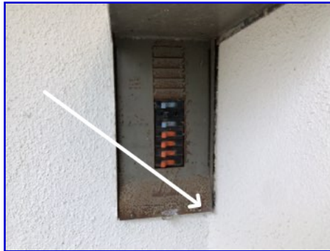
Not labeled; Missing screw; Zinsco
