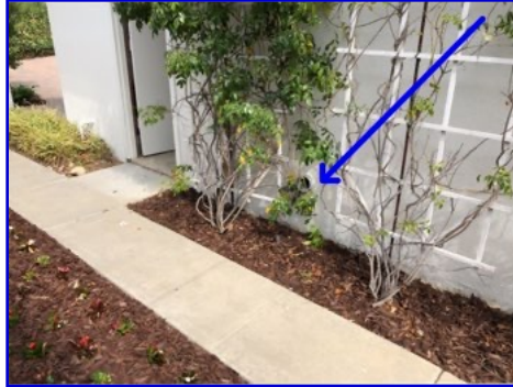
Missing exterior cover
