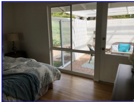
Not tempered glass; Not operating
