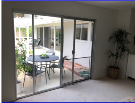
Not latching; Difficult to operate
