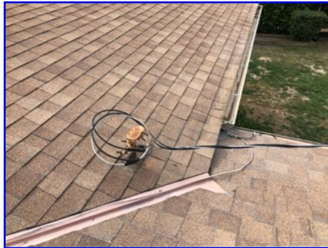
Too close to roof
