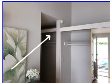
J-box missing cover
