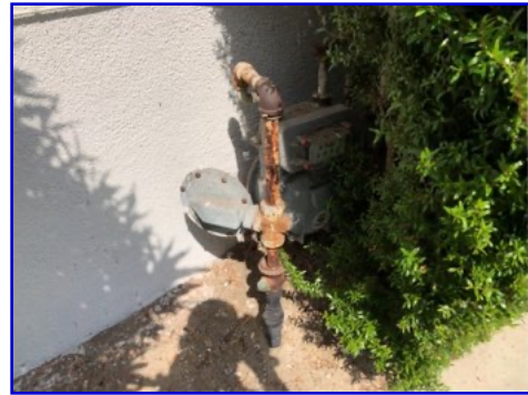
MAIN GAS VALVE; Significant rust
