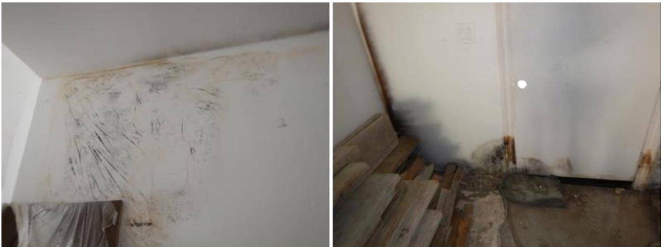
View of mold stains in garage
