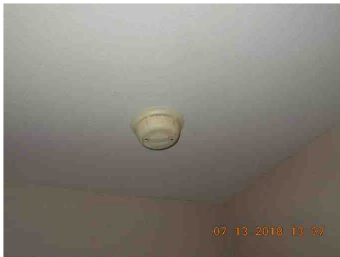
1st floor smoke detector
