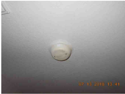
2nd floor Smoke detector
