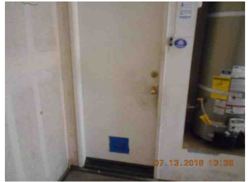
Breached Fire Door
