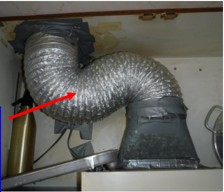
The kitchen exhaust fan may not use a flexible duct
