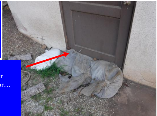
The garage N-sideyard is prone to flooding...
