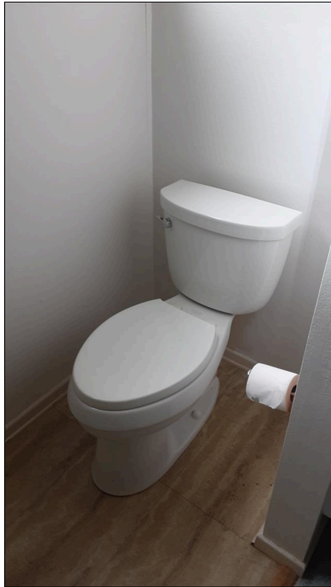
6.5 Item 2(Picture) Loose toilet, master bathroom
