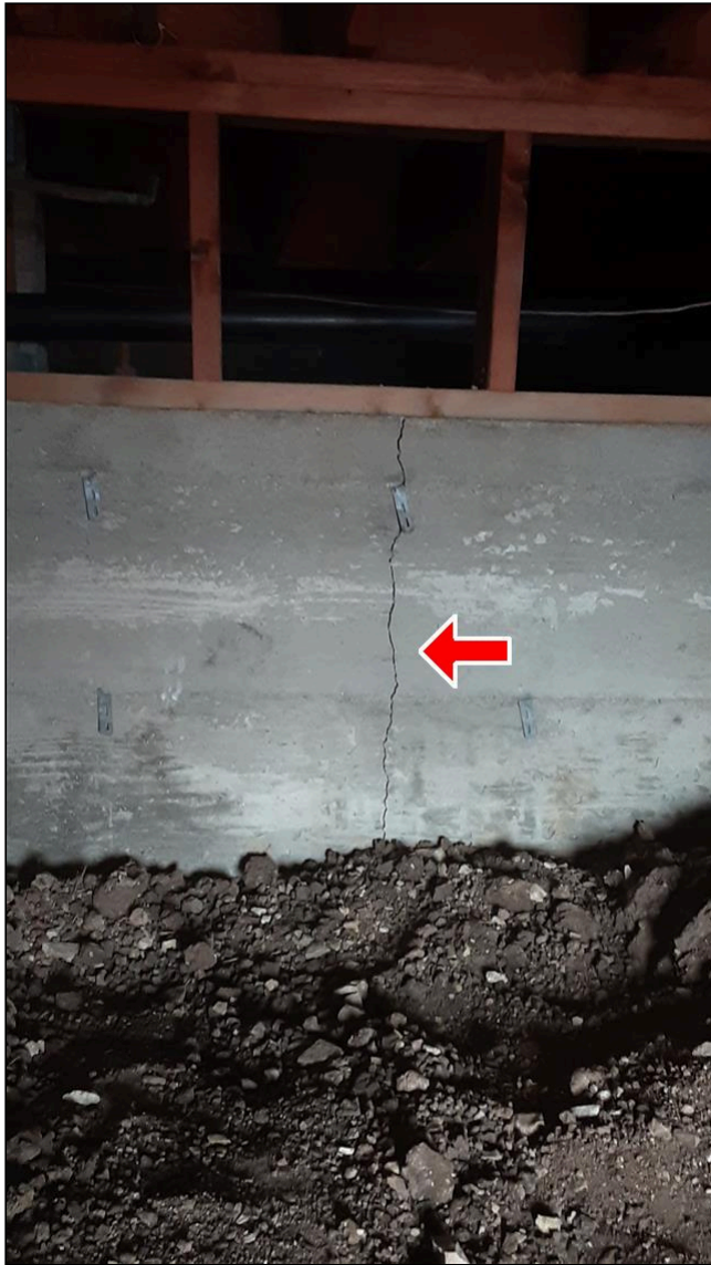
11.0 Item 1(Picture) Minor cracking
