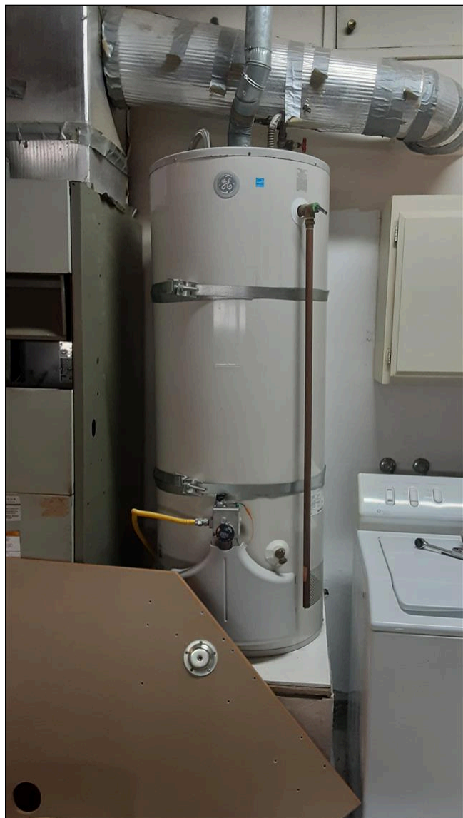
6.2 Item 1(Picture) Water heater
