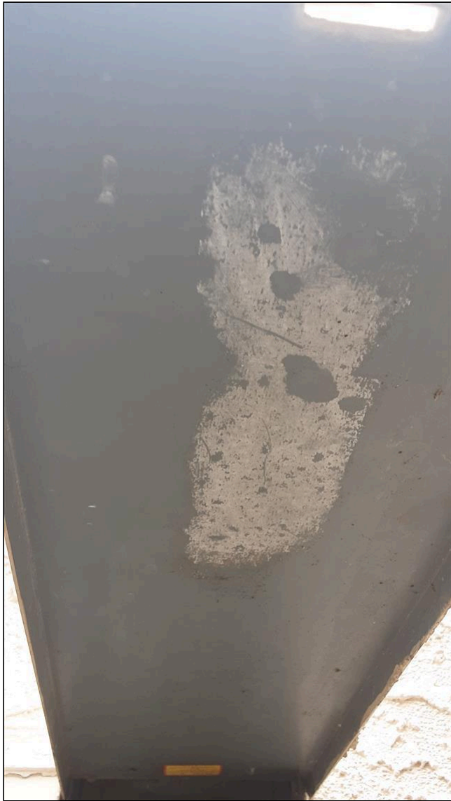
5.2 Item 1(Picture) Missing panel information
