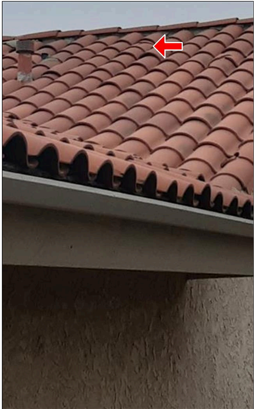
2.0 Item 2(Picture) Cracked roof tile
