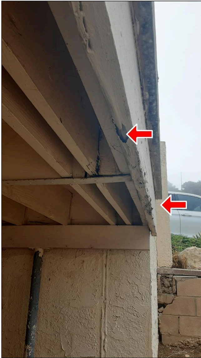
1.5 Item 1(Picture) Wood damage, main entry bridge
