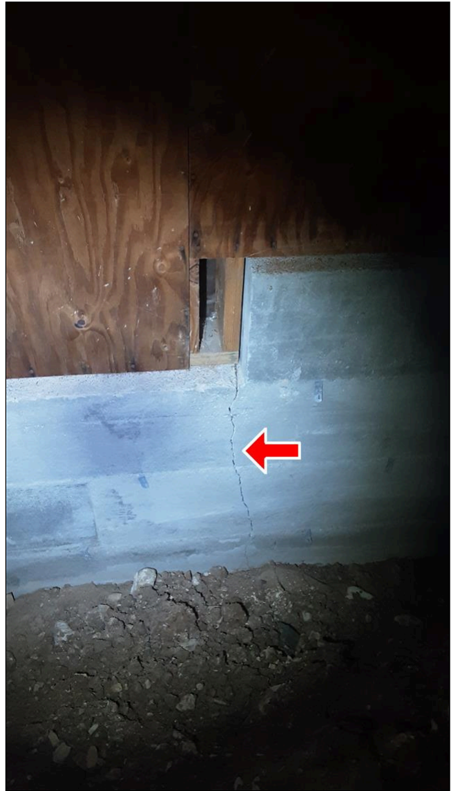
11.0 Item 2(Picture) Minor cracking
