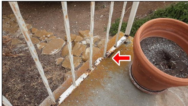
1.7 Item 3(Picture) Damaged railing
