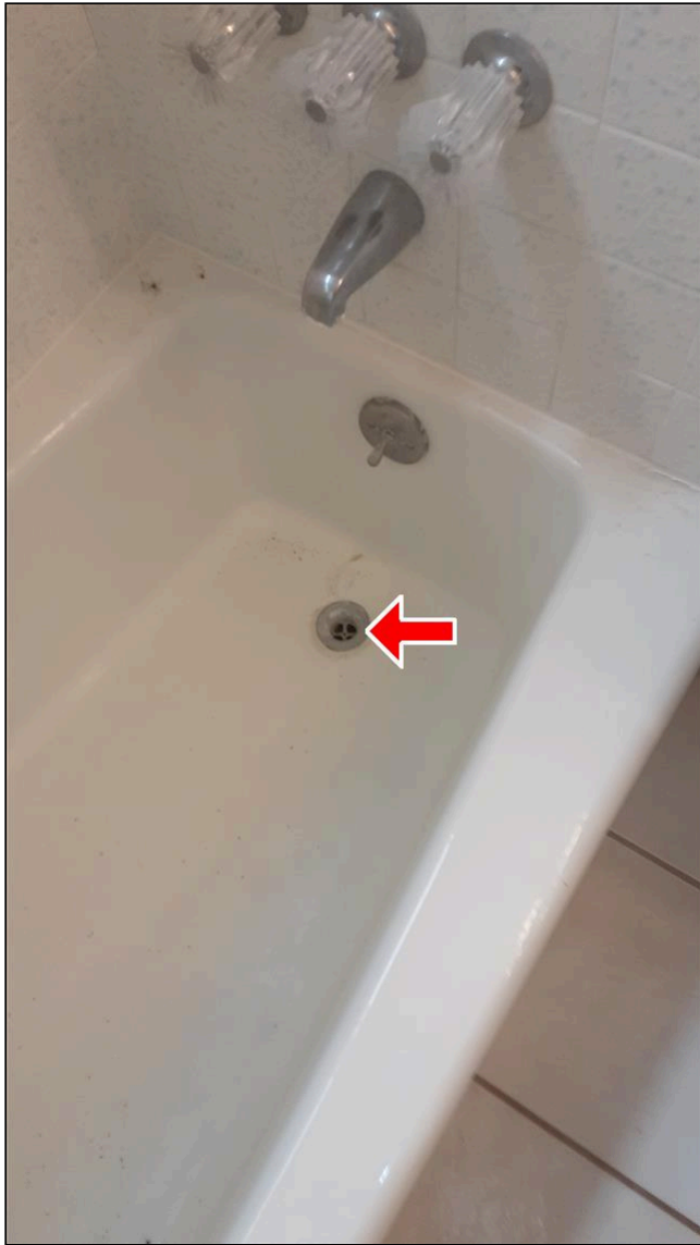
6.5 Item 3(Picture) Missing drain stop
