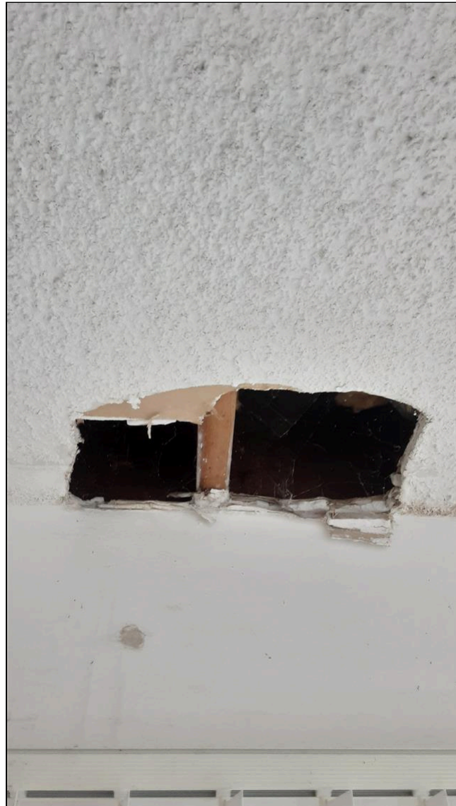
4.0 Item 1(Picture) Ceiling damage, lower level northwest bedroom
