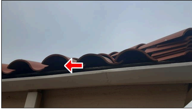
2.0 Item 1(Picture) Missing bird stops
