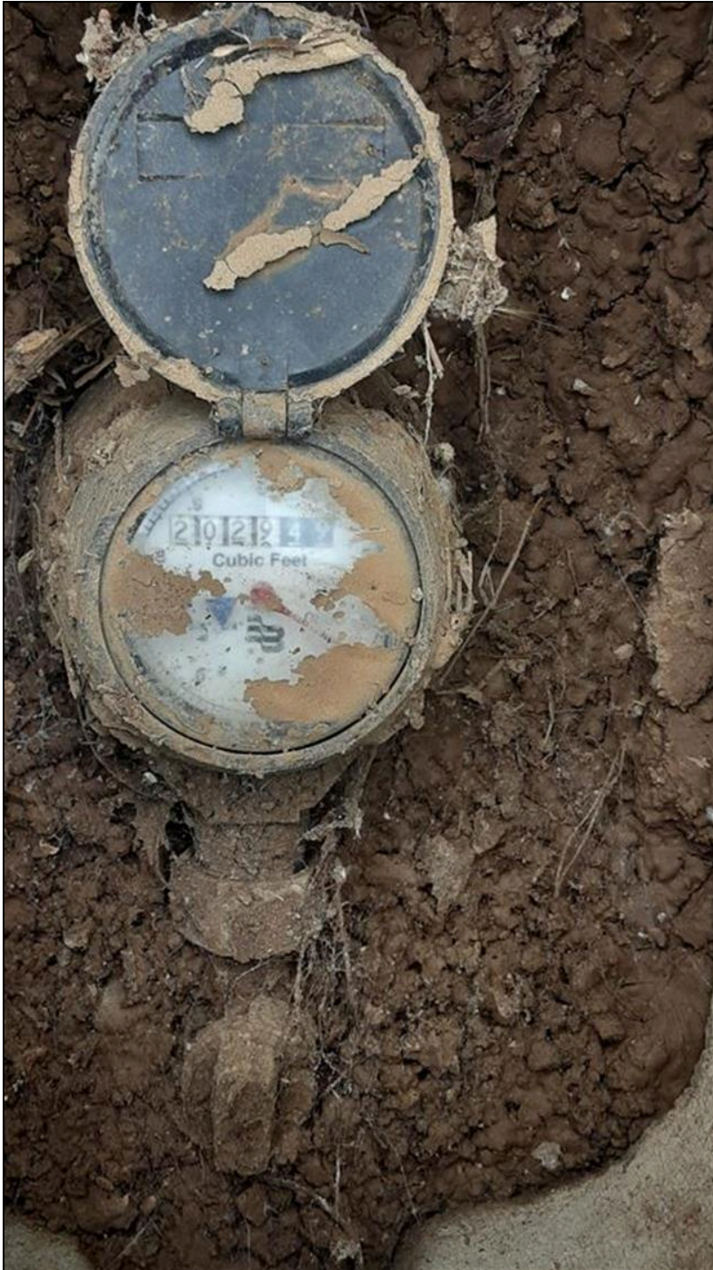
6.0 Item 1(Picture) Water meter
