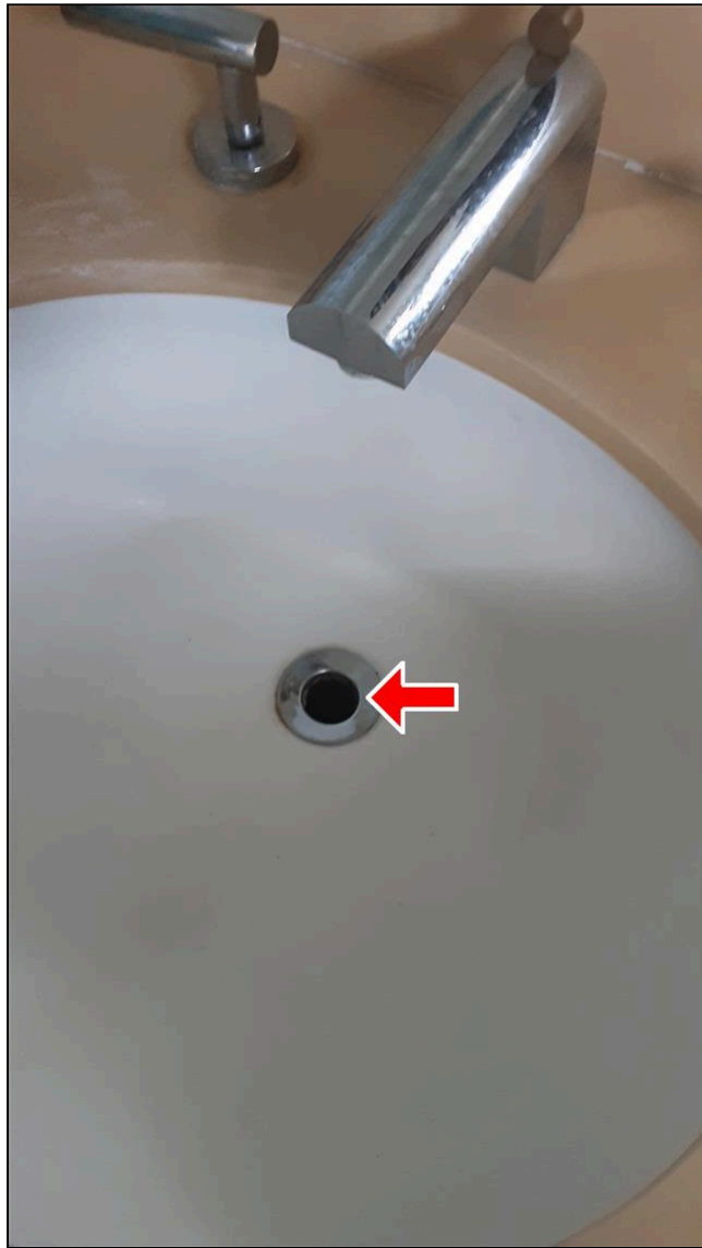
6.5 Item 1(Picture) Drain stop missing, powder room sink
