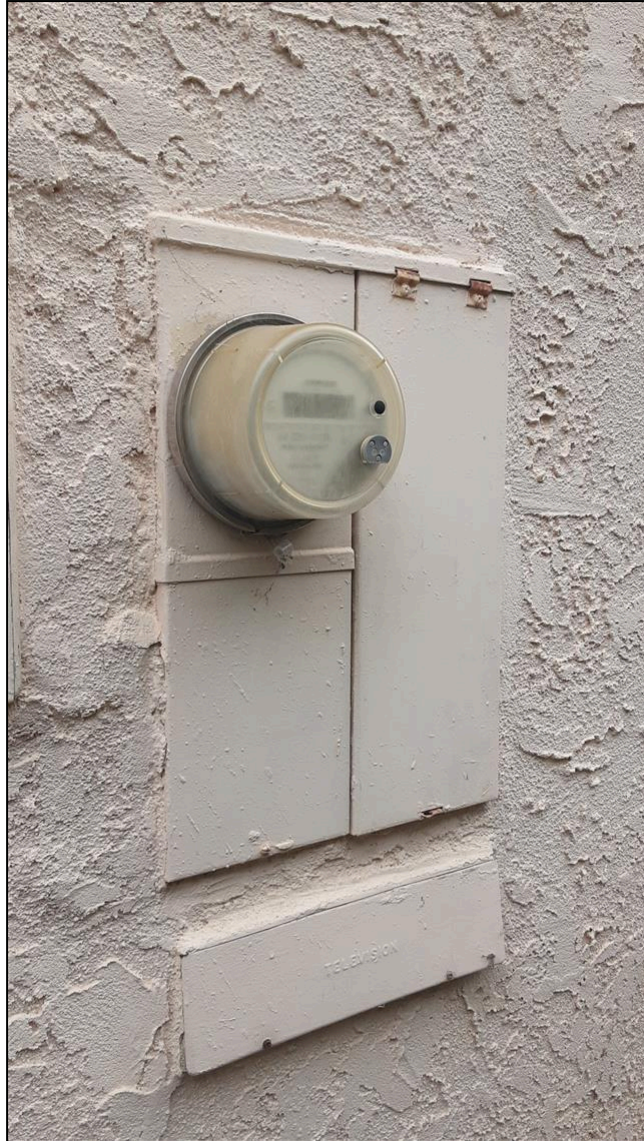
5.1 Item 1(Picture) Electric meter and main distribution panel
