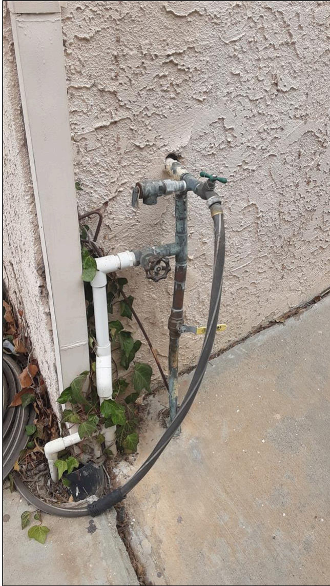
6.0 Item 2(Picture) Main water shut off
