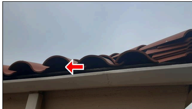
2.0 Item 1(Picture) Missing bird stops
