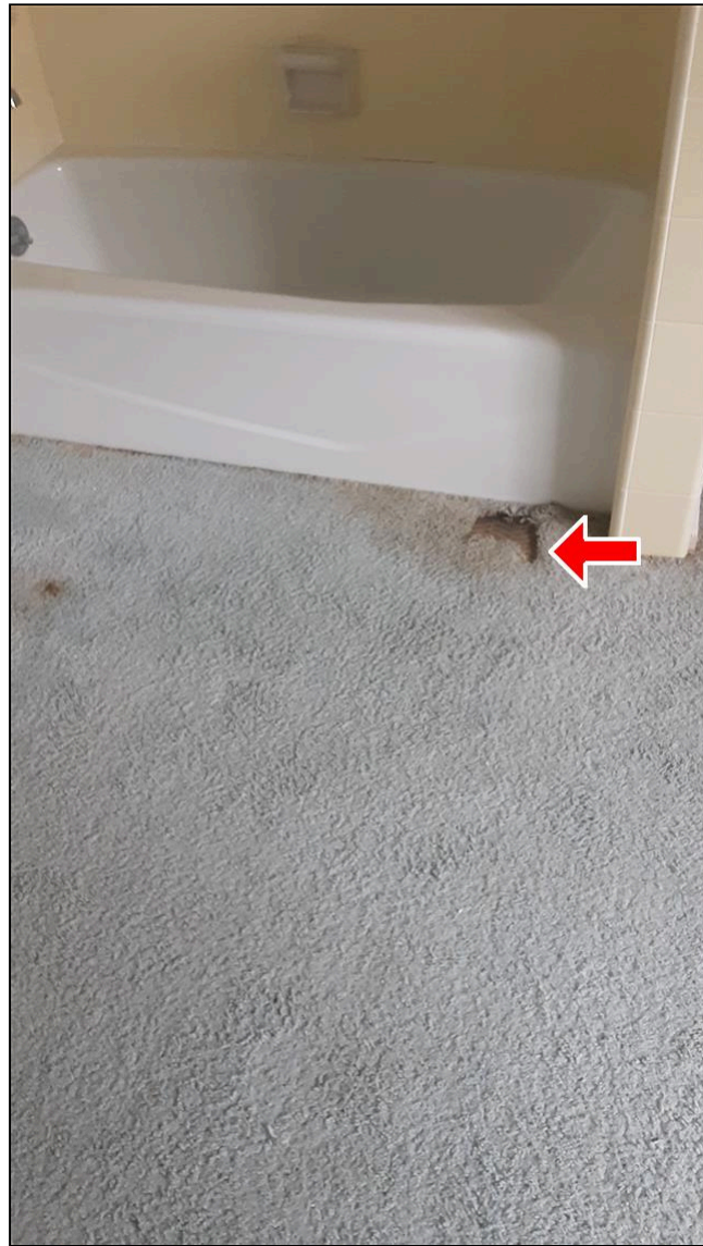
4.2 Item 2(Picture) Damaged carpet
