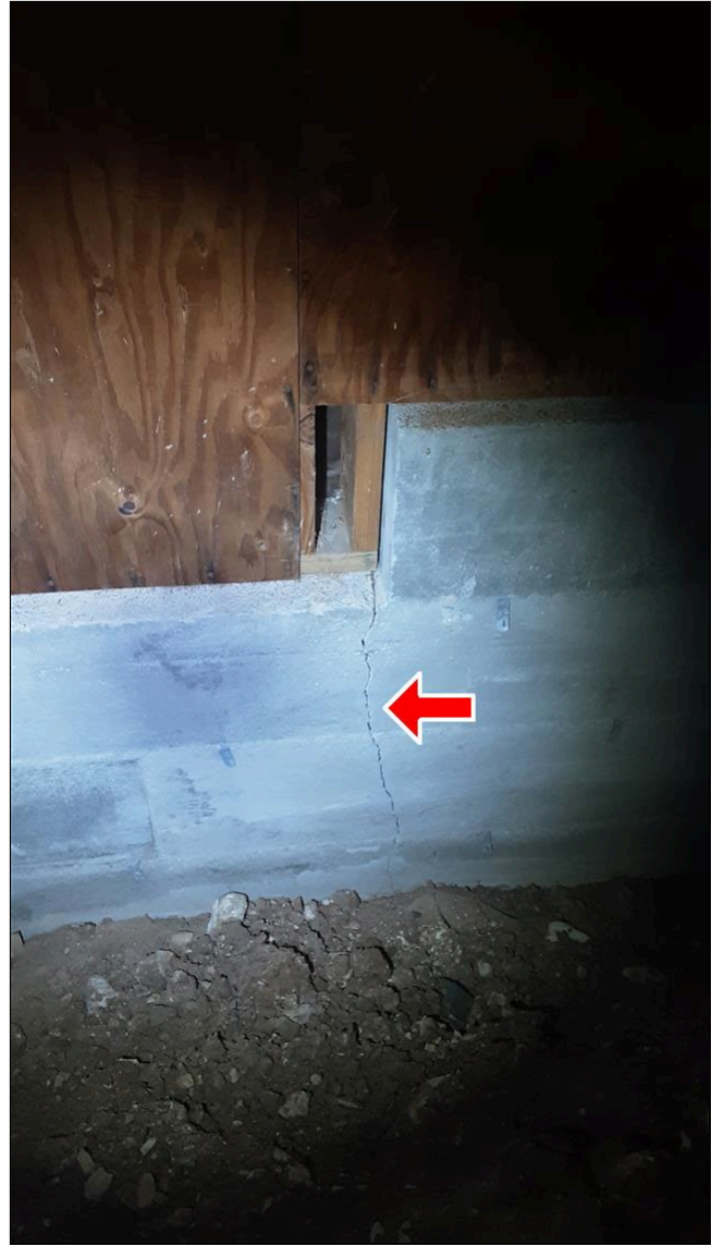
11.0 Item 2(Picture) Minor cracking
