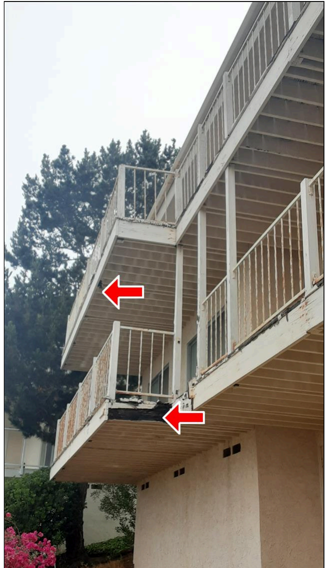
1.8 Item 2(Picture) Wood damage, balcony
