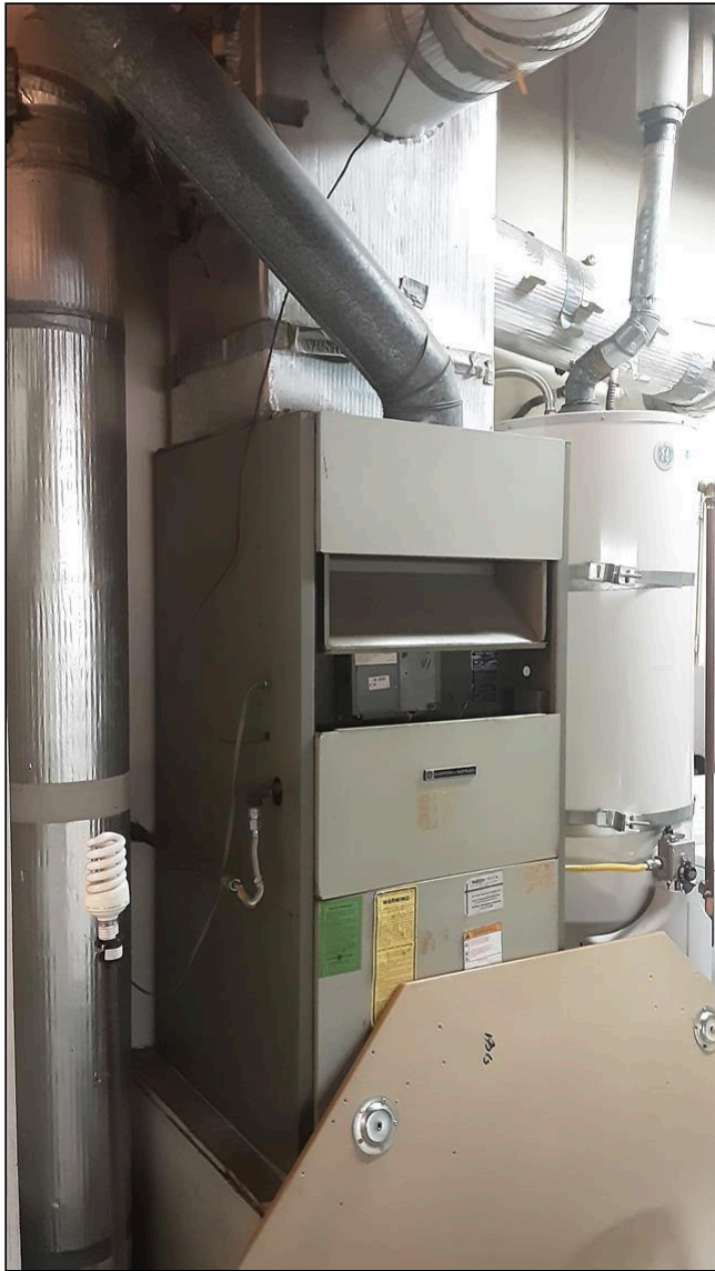
9.0 Item 1(Picture) Heat system
