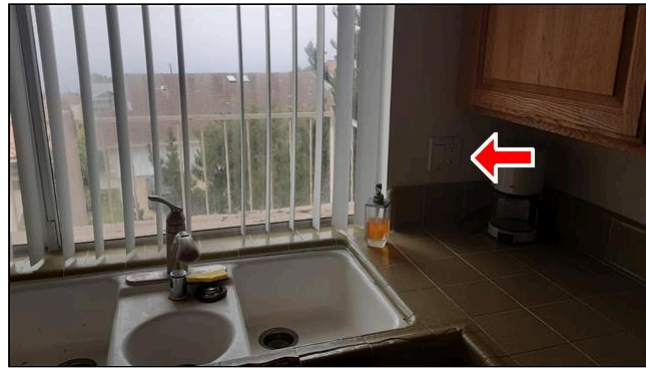
5.5 Item 3(Picture) Kitchen outlet
