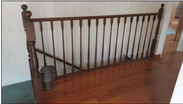
4.4 Item 1(Picture) Baluster on stairwell
