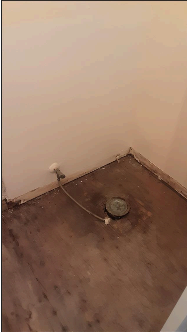
6.4 Item 2(Picture) Missing toilet, lower level hall bathroom
