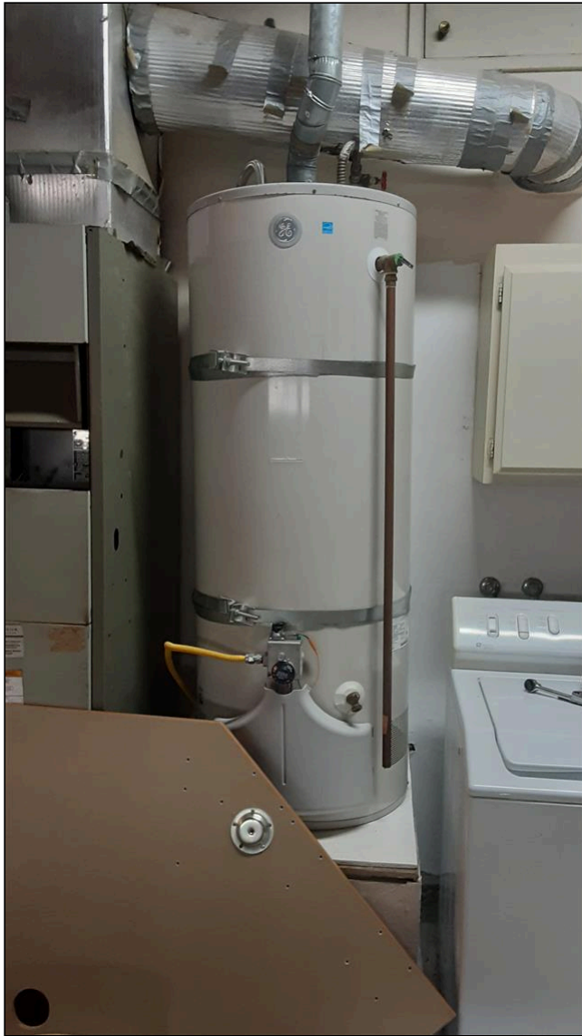
6.2 Item 1(Picture) Water heater
