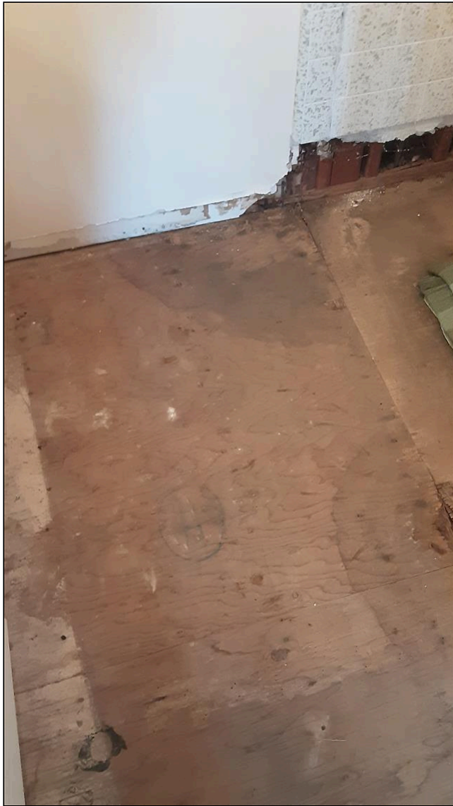
4.2 Item 3(Picture) Missing flooring, lower level hall bathroom
