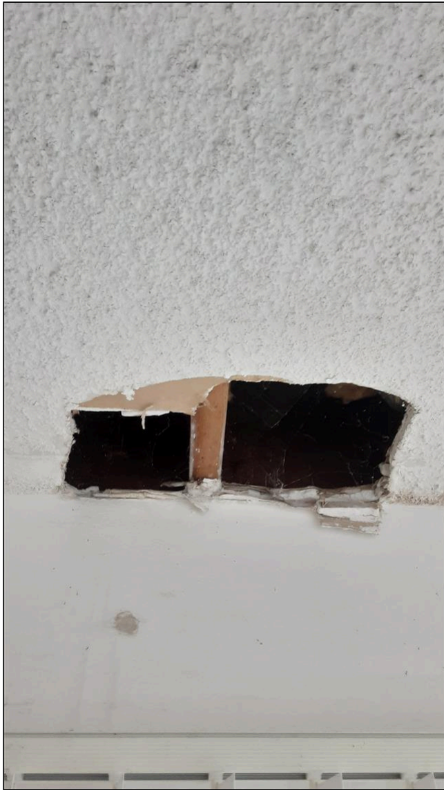
4.0 Item 1(Picture) Ceiling damage, lower level northwest bedroom
