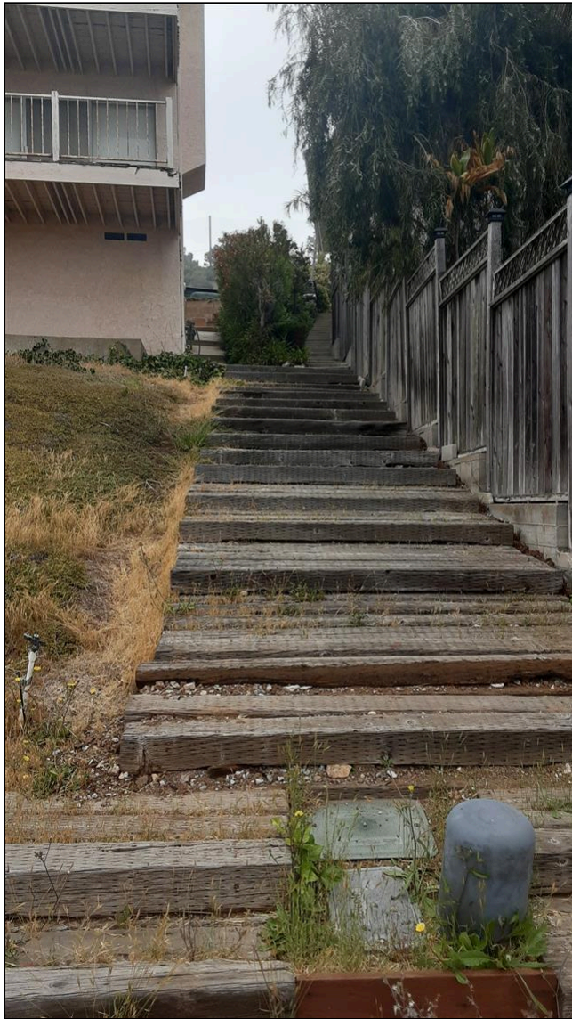
1.7 Item 1(Picture) Missing railing, steps leading to west side
