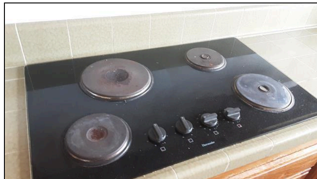
7.1 Item 1(Picture) Kitchen burners
