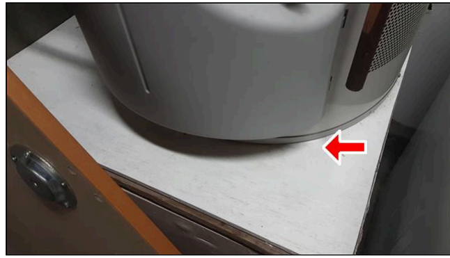
6.2 Item 4(Picture) Missing drip pan
