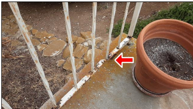
1.7 Item 3(Picture) Damaged railing
