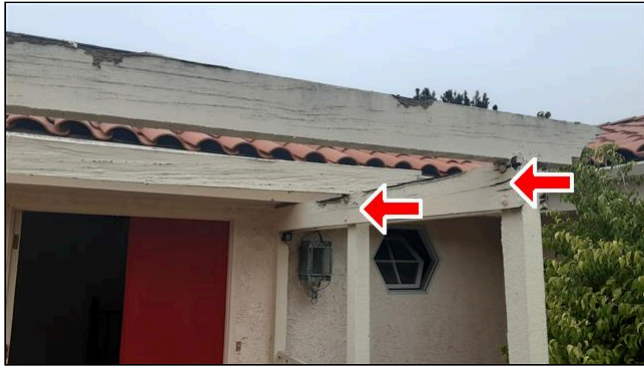
1.8 Item 4(Picture) Wood damage, front entry
