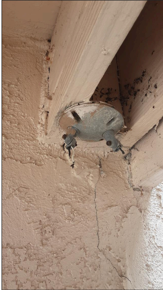
5.5 Item 1(Picture) Damaged fixture/exposed wiring, below main entry bridge
