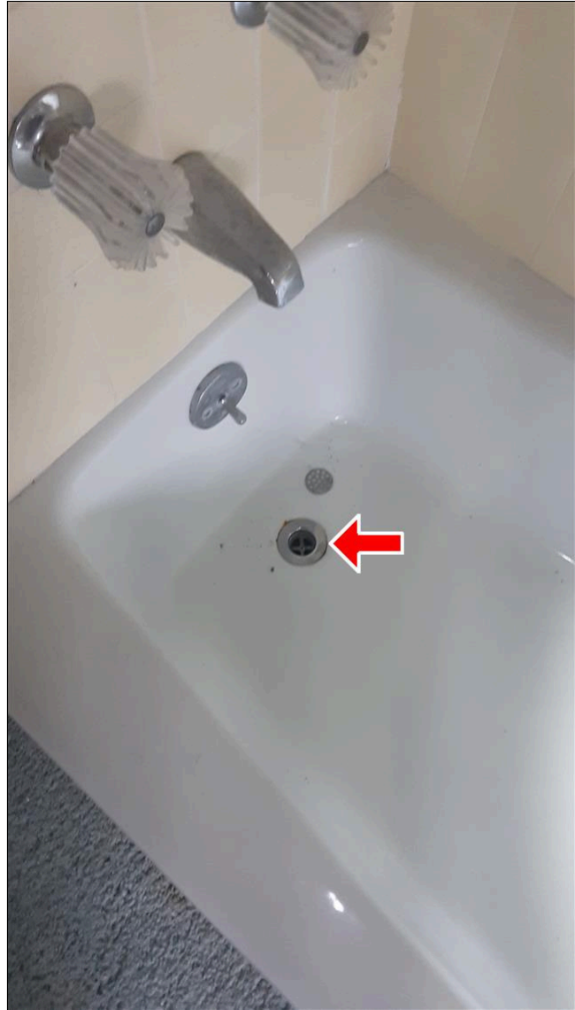
6.5 Item 4(Picture) Missing drain stop
