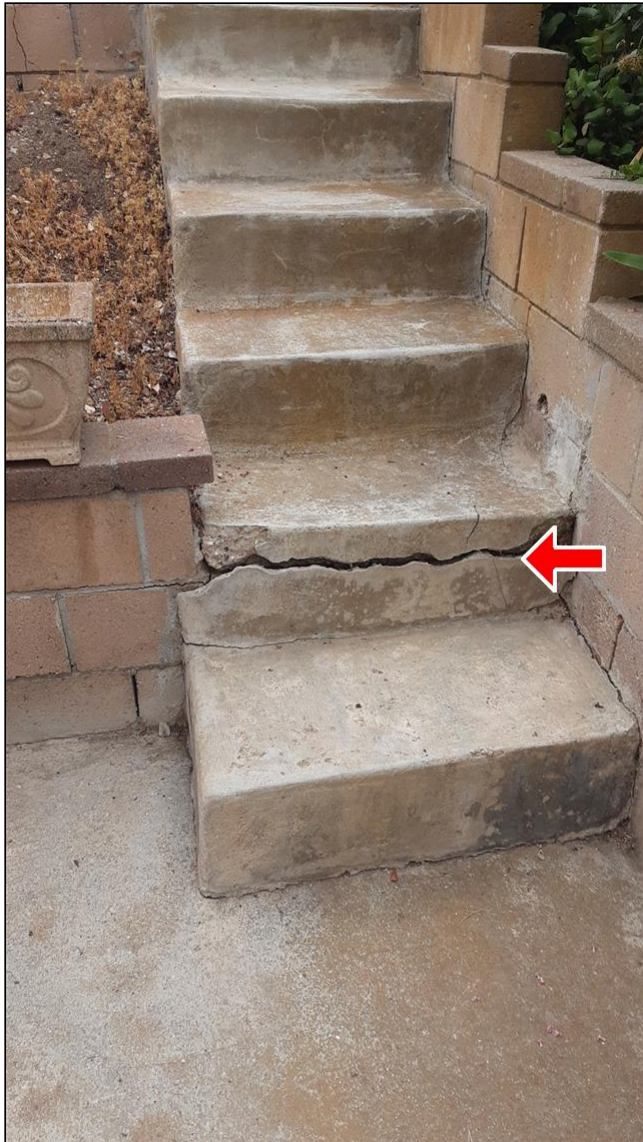
1.6 Item 2(Picture) Cracking steps leading to front patio
