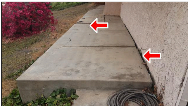
1.8 Item 3(Picture) Concrete damage, west side
