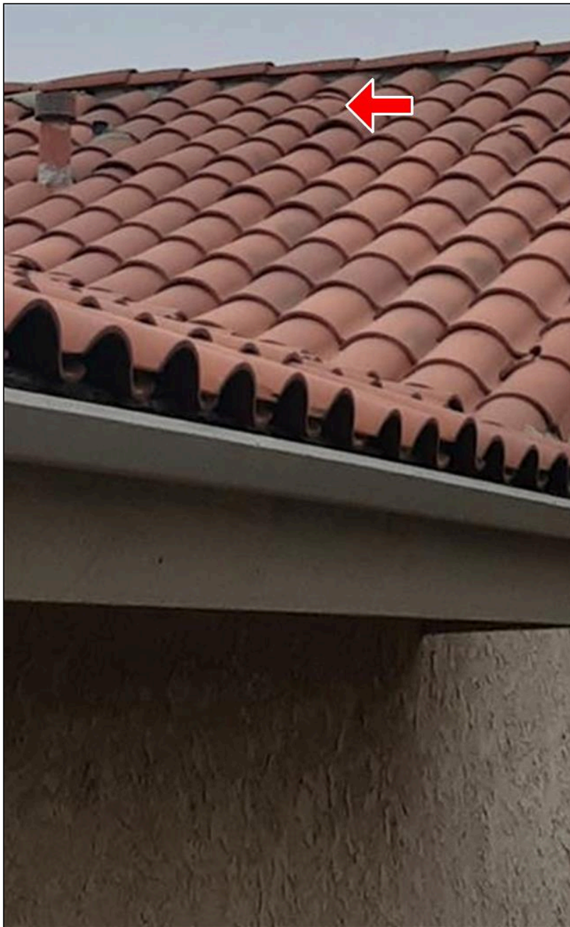
2.0 Item 2(Picture) Cracked roof tile
