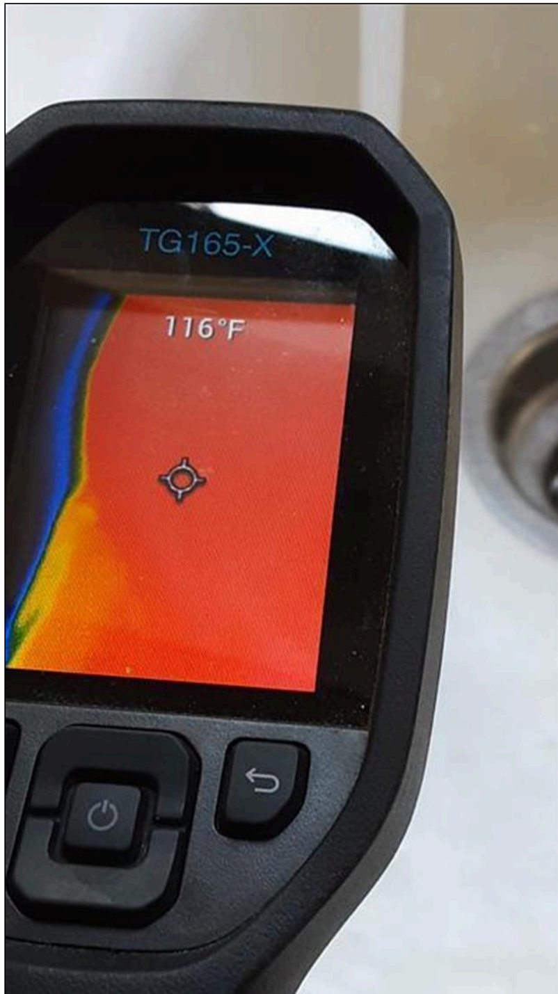
6.2 Item 3(Picture) Hot water temp
