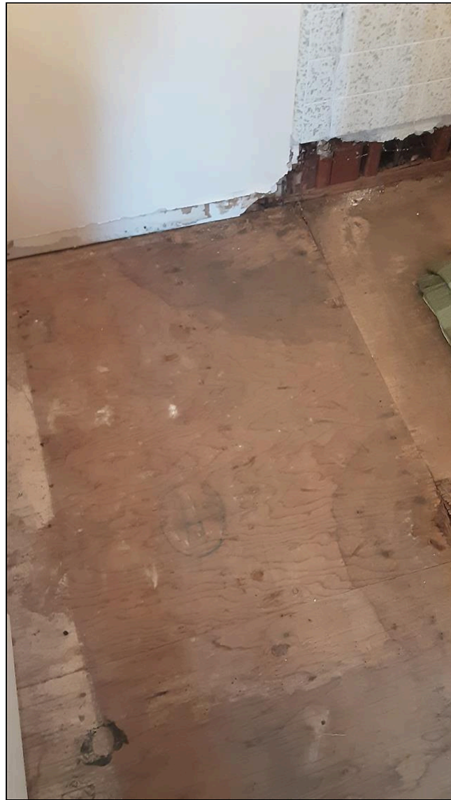
4.2 Item 3(Picture) Missing flooring, lower level hall bathroom
