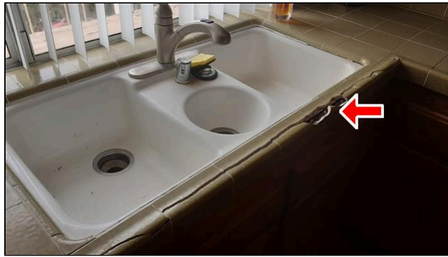
4.5 Item 1(Picture) Kitchen countertop, tile damage
