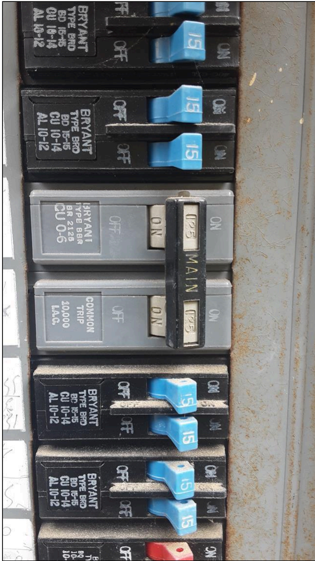
5.3 Item 2(Picture) 125 amp main shut off
