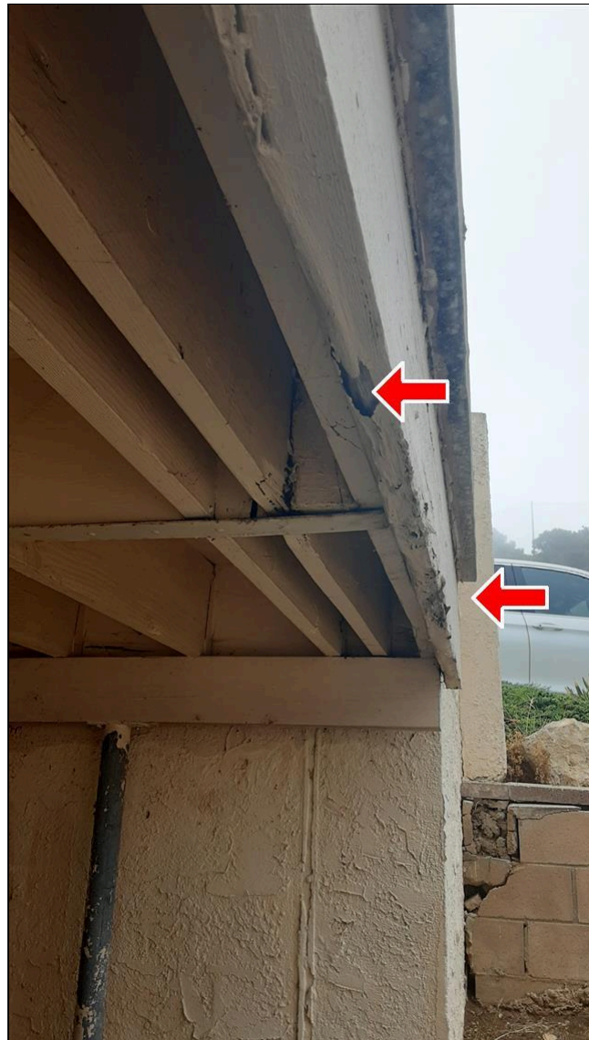
1.5 Item 1(Picture) Wood damage, main entry bridge
