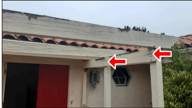
1.8 Item 4(Picture) Wood damage, front entry
