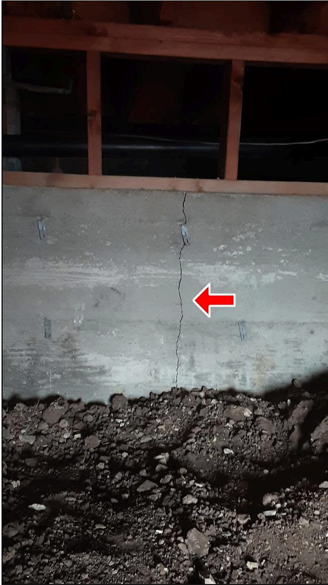
11.0 Item 1(Picture) Minor cracking
