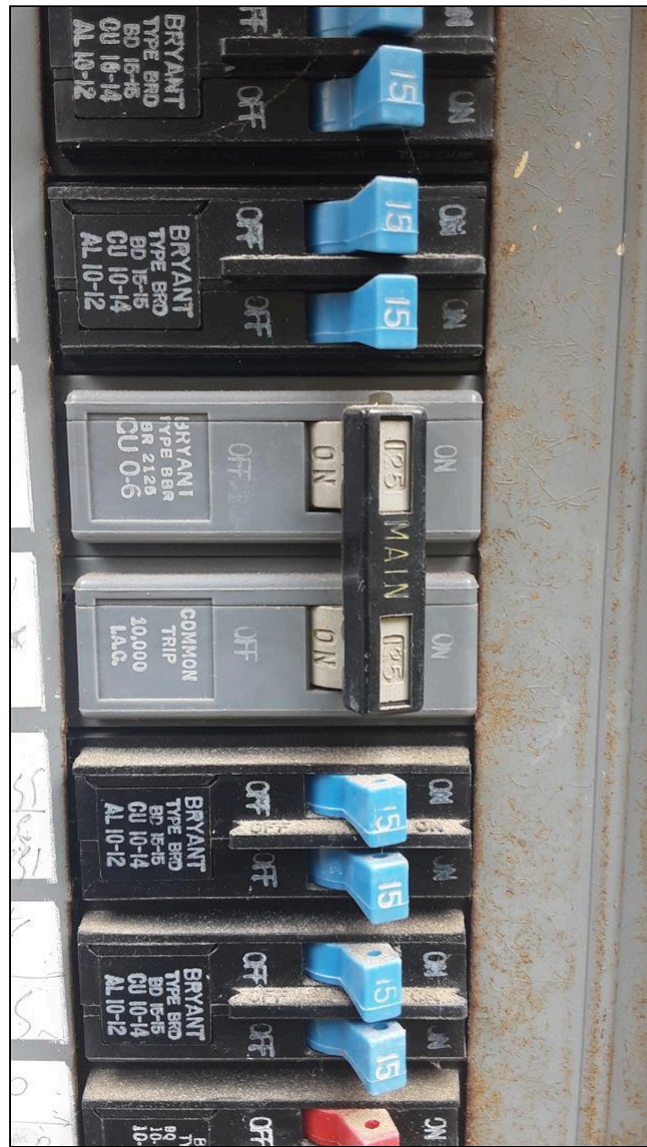
5.3 Item 2(Picture) 125 amp main shut off
