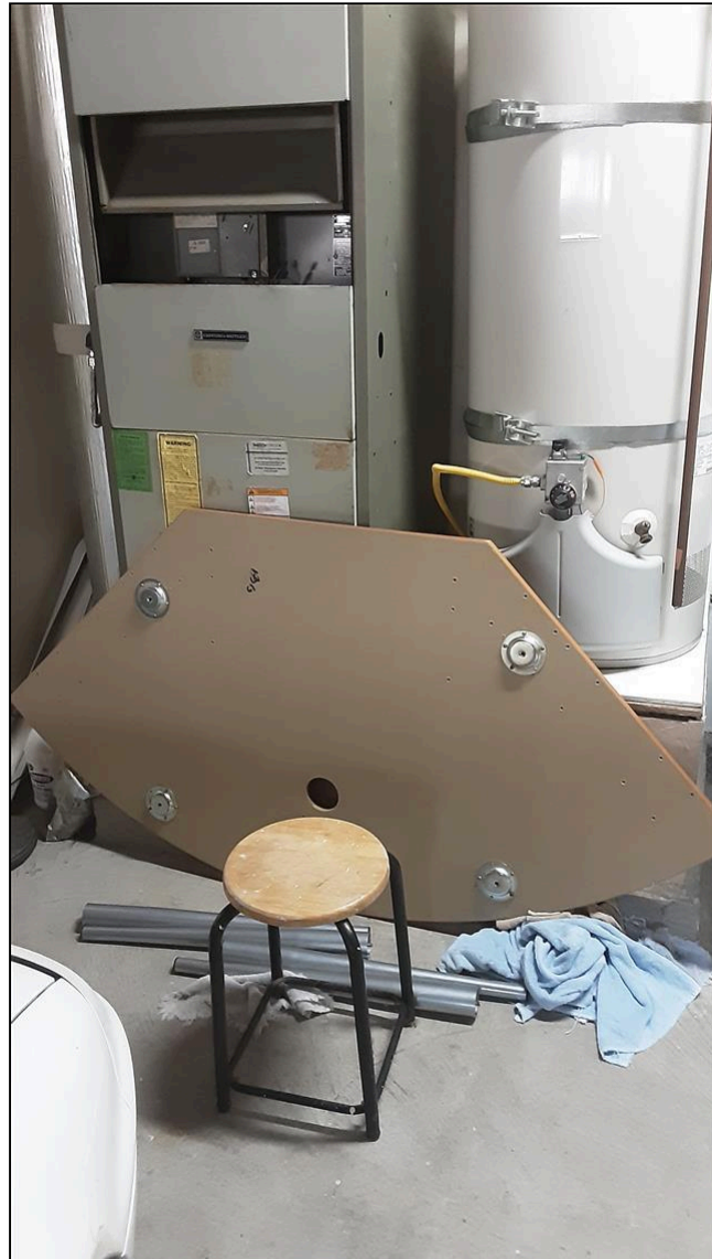
6.2 Item 5(Picture) No protection for appliances in garage
