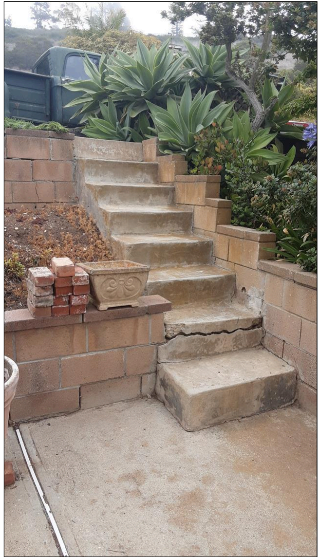
1.7 Item 2(Picture) Missing railing leading to front patio
