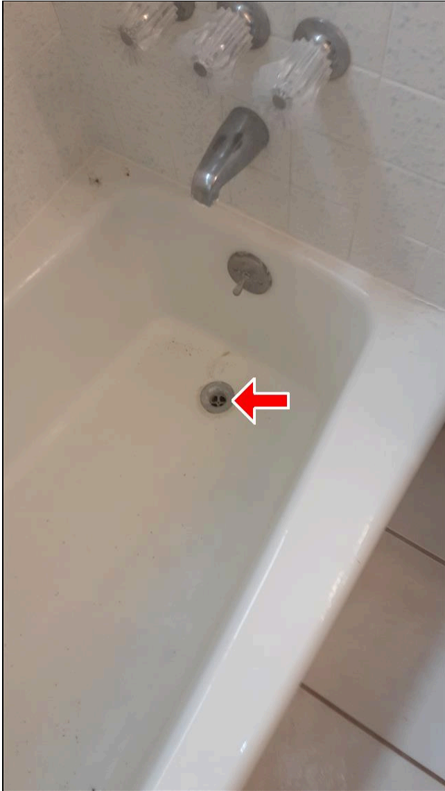
6.5 Item 3(Picture) Missing drain stop
