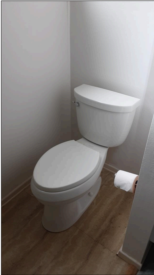
6.5 Item 2(Picture) Loose toilet, master bathroom
