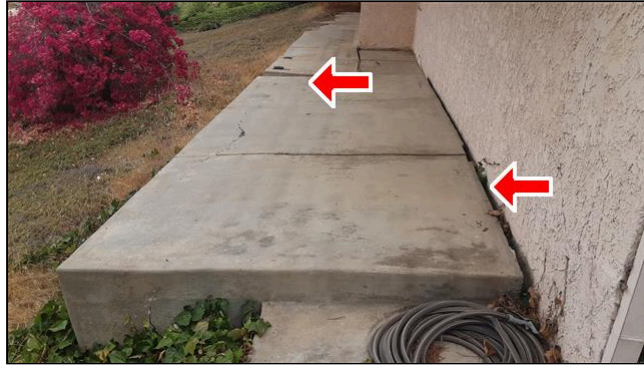
1.8 Item 3(Picture) Concrete damage, west side
