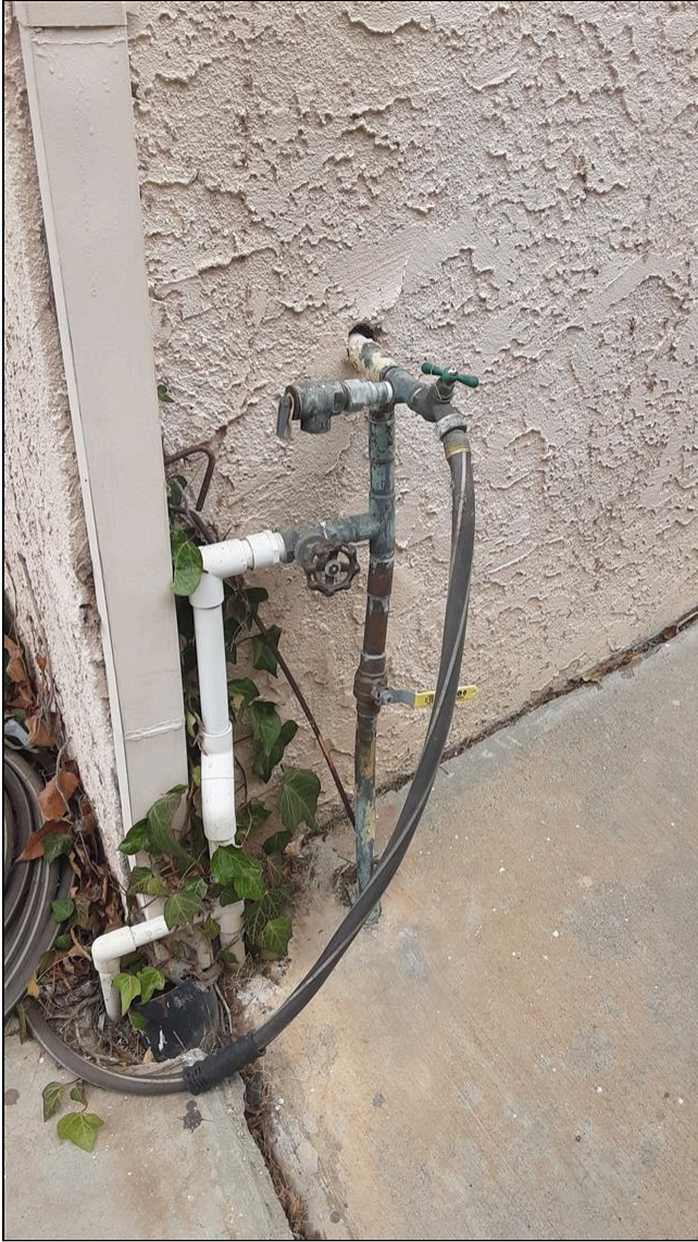
6.0 Item 2(Picture) Main water shut off
