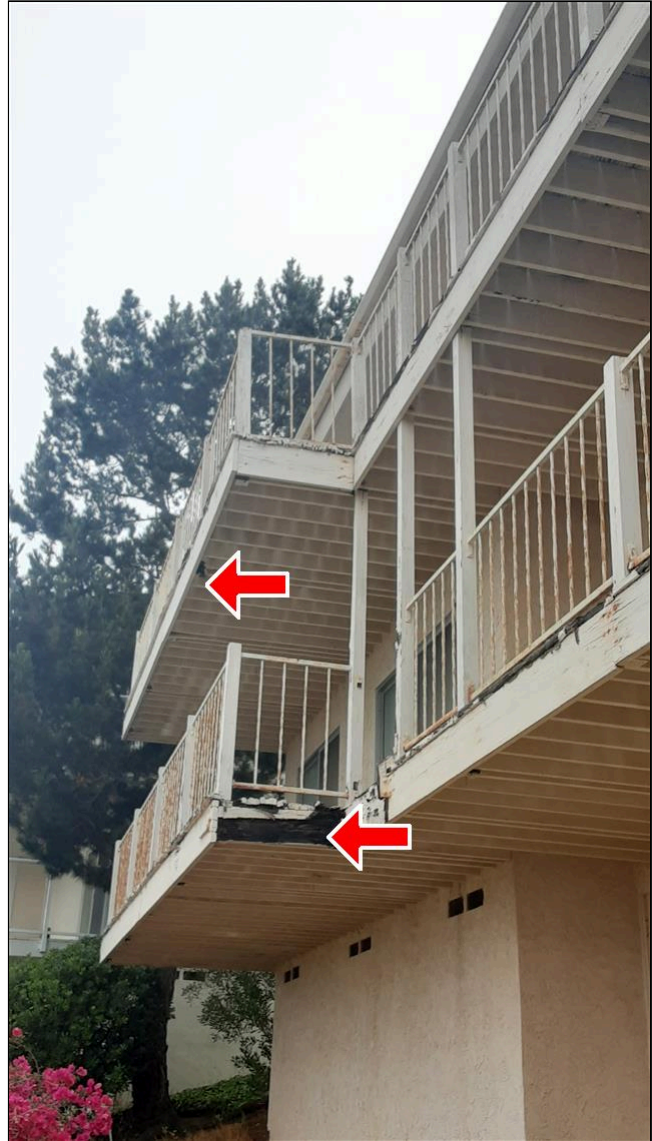
1.8 Item 2(Picture) Wood damage, balcony
