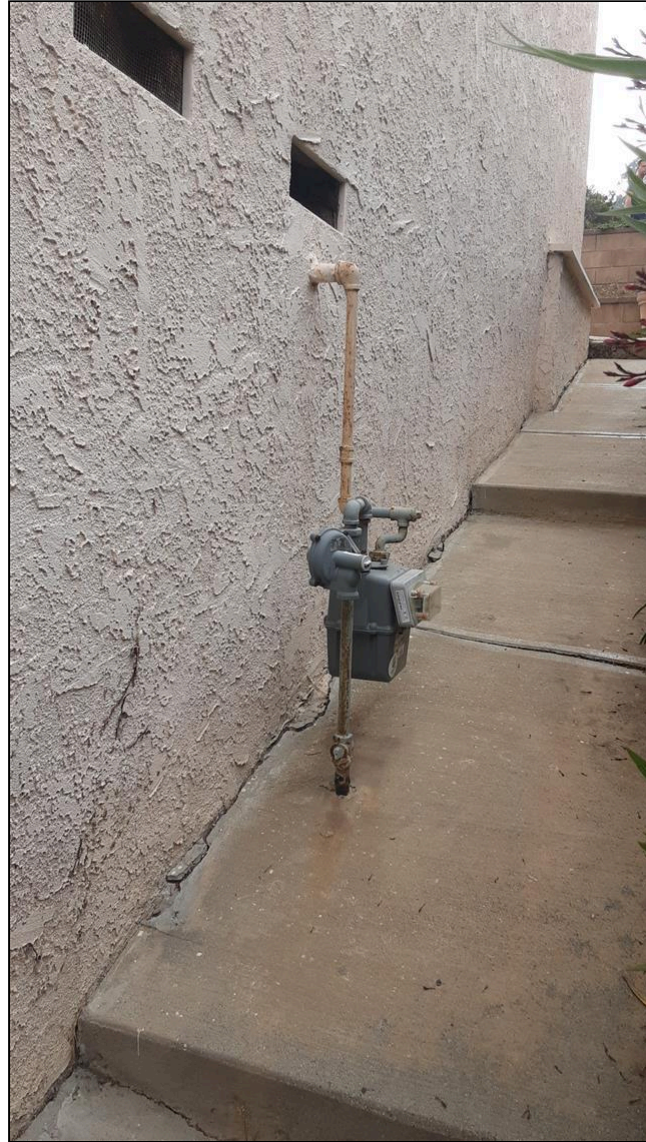
6.1 Item 1(Picture) Gas meter/main shut off
