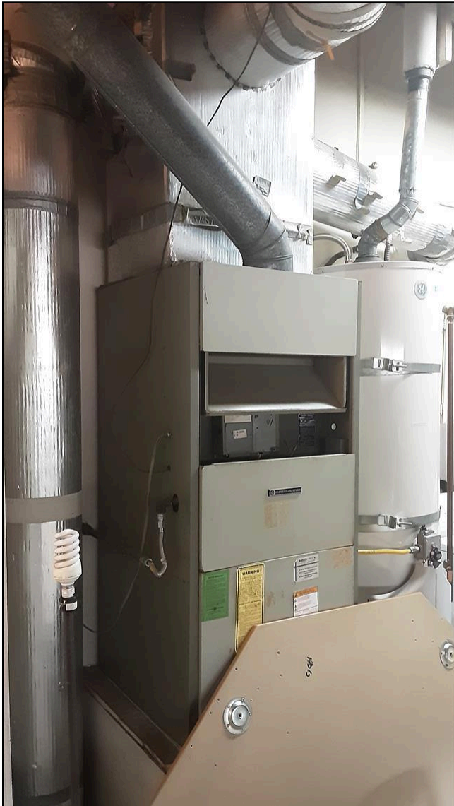
9.0 Item 1(Picture) Heat system
