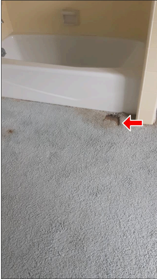
4.2 Item 2(Picture) Damaged carpet
