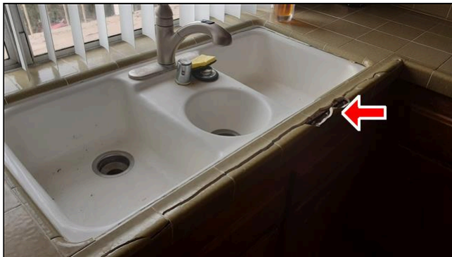
4.5 Item 1(Picture) Kitchen countertop, tile damage
