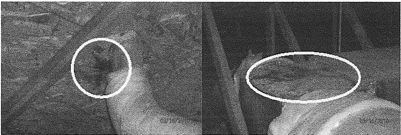
Moisture stains on plenum
