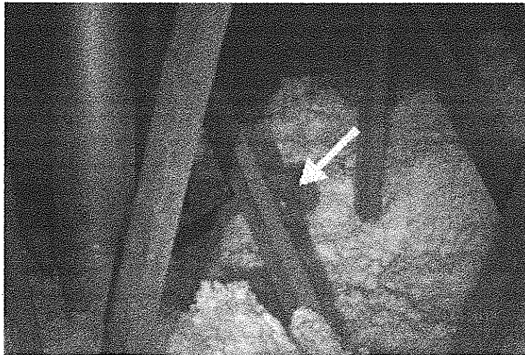
Open junction box
