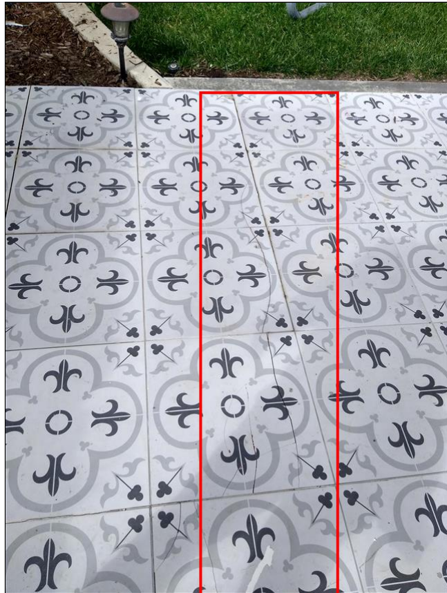
2.3 Item 2(Picture) Cracking noted at tile
