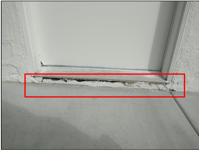
2.0 Item 2(Picture) Wear noted at garage pedestrian door threshold. Recommend repairs to prevent water intrusion.
