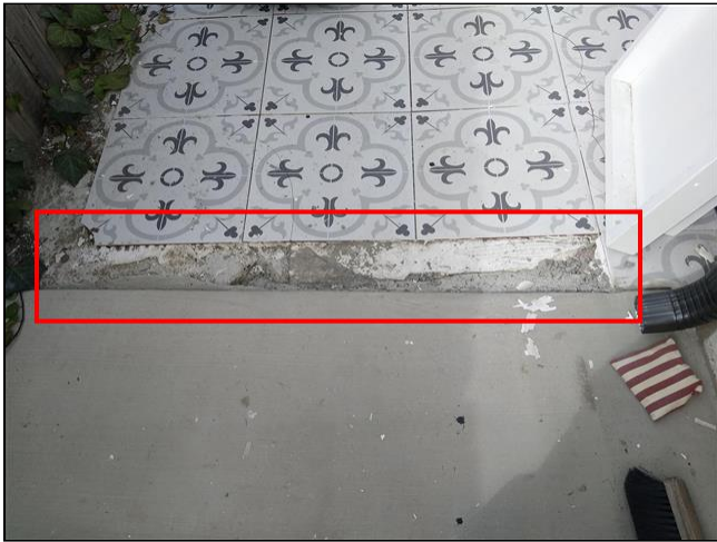
2.3 Item 1(Picture) Wear, uneven areas noted
