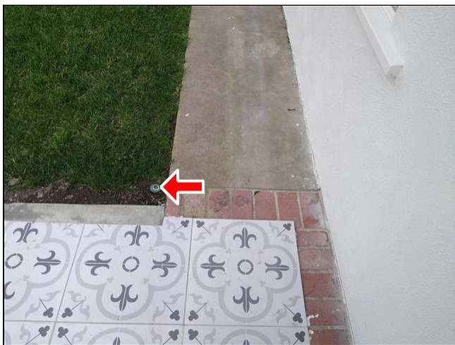
2.7 Item 3(Picture) Sprinkler head noted by pavement
