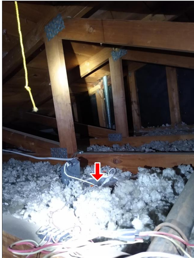
7.4 Item 5(Picture) Open junction box noted, W attic area
