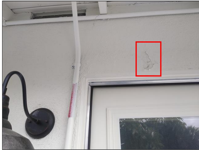
2.0 Item 3(Picture) Wear noted
