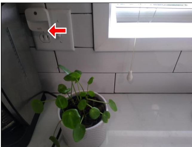
7.3 Item 11(Picture) Kitchen countertop outlets are Two-prong, Not GFCI
