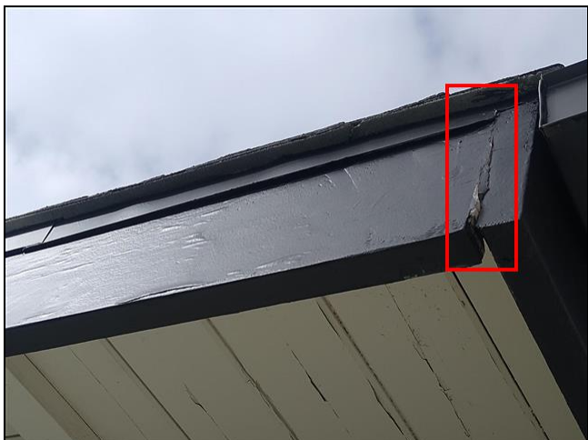
1.6 Item 1(Picture) Wear noted
