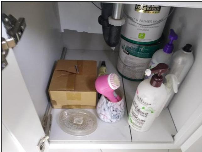
6.0.C Item 3(Picture) NOTE: Inspection under sink is limited due to personal items blocking view and access. Suggest careful evaluation when fully visible and accessible.
