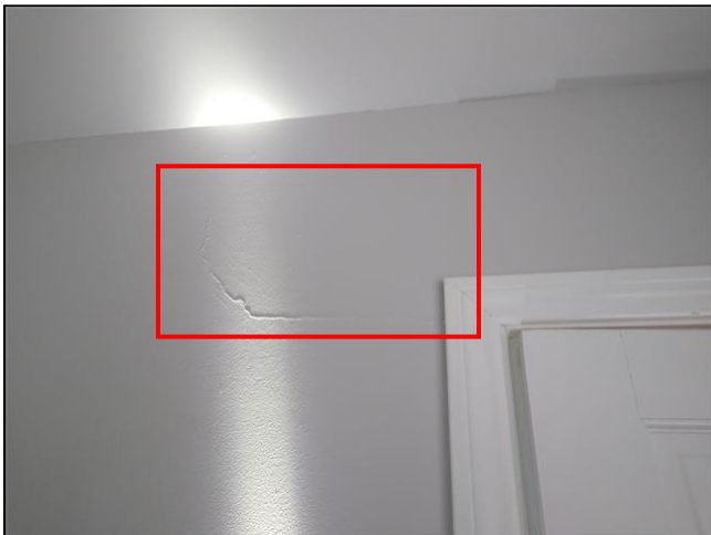
4.0 Item 3(Picture) Cracking noted in Master bedroom at wall by door, possibly due to settlement. Suggest repairs/repainting.
