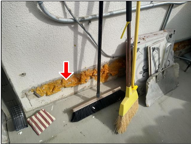
2.0 Item 5(Picture) Unconventional repairs noted (area by electrical panel). Ask seller for history.
