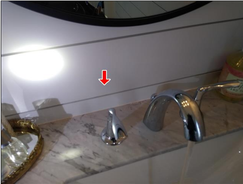
6.0.C Item 2(Picture) NOTE/MAINTENANCE TIP: Material behind bathroom sink is not optimized for wet locations. Recommend monitoring over time and upgrading materials as desired for improved performance.
