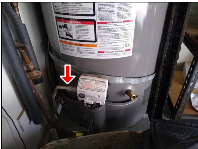
6.8.A Item 1(Picture) No sediment trap noted
