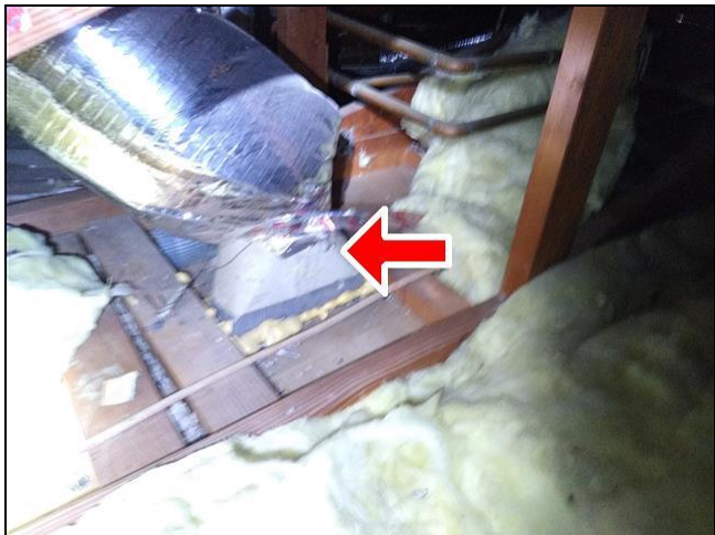
8.4 Item 1(Picture) Possible asbestos-containing material noted at duct boot
