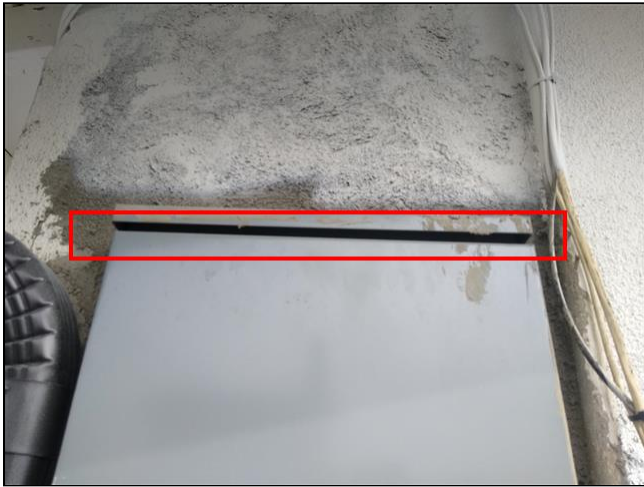
7.1 Item 3(Picture) Gap noted at upper portion of electrical panel enclosure
