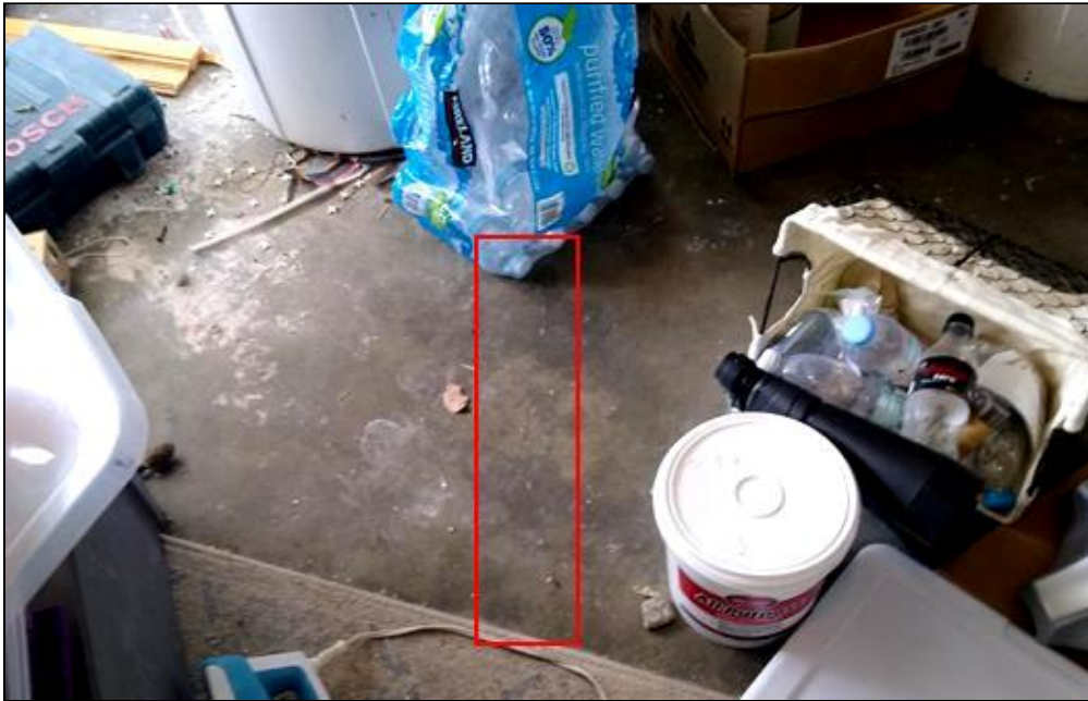
3.1 Item 2(Picture) Crack noted
