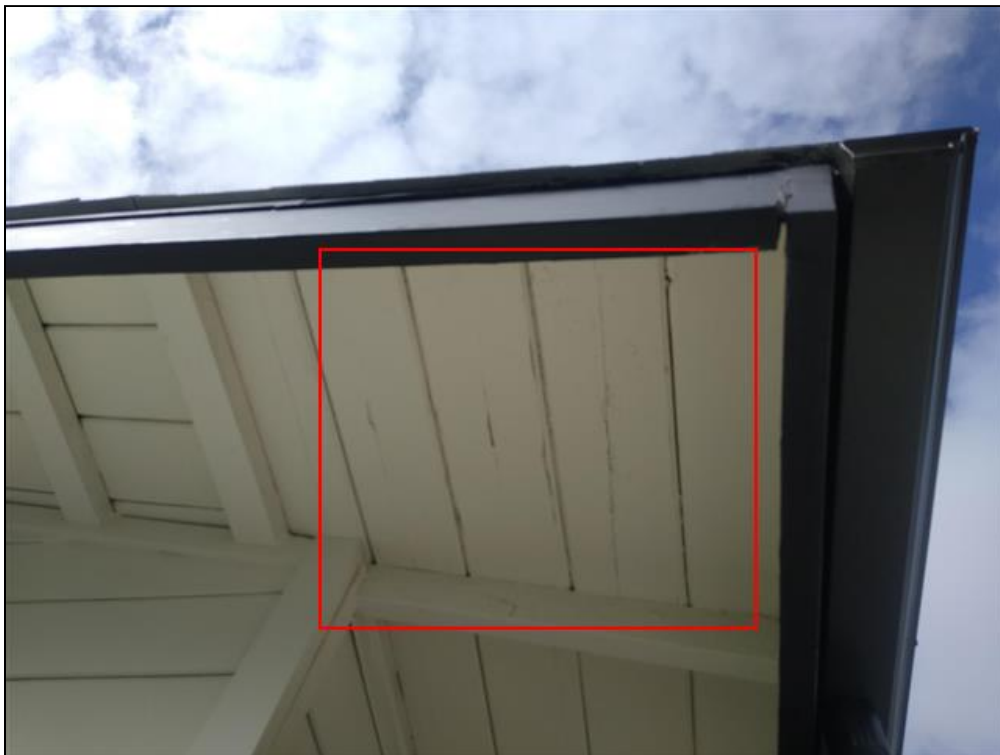
1.6 Item 3(Picture) Wear noted
