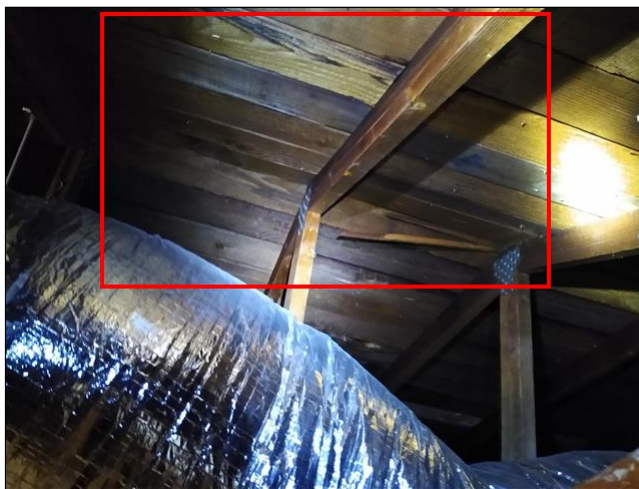
9.1 Item 2(Picture) Staining noted
