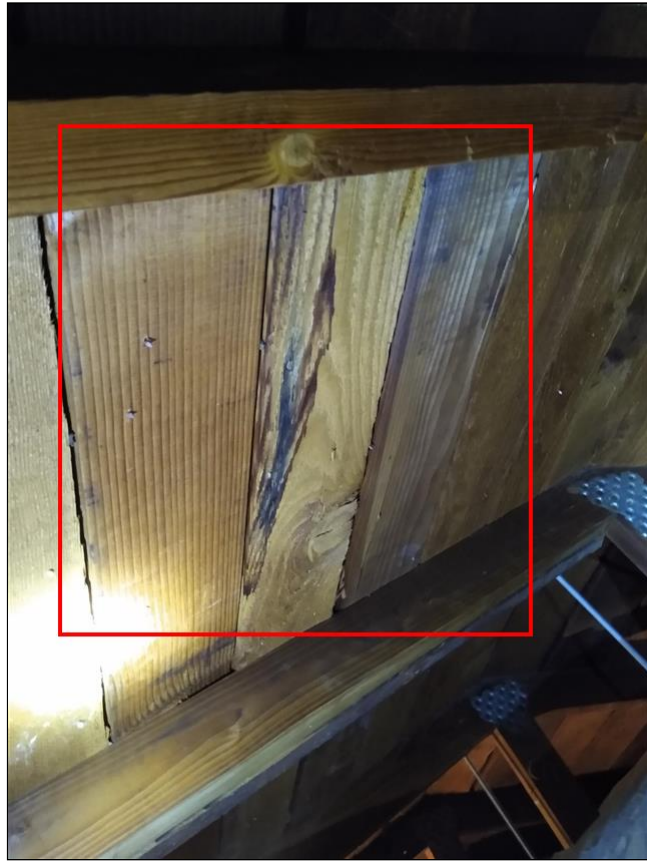
9.1 Item 4(Picture) Staining noted
