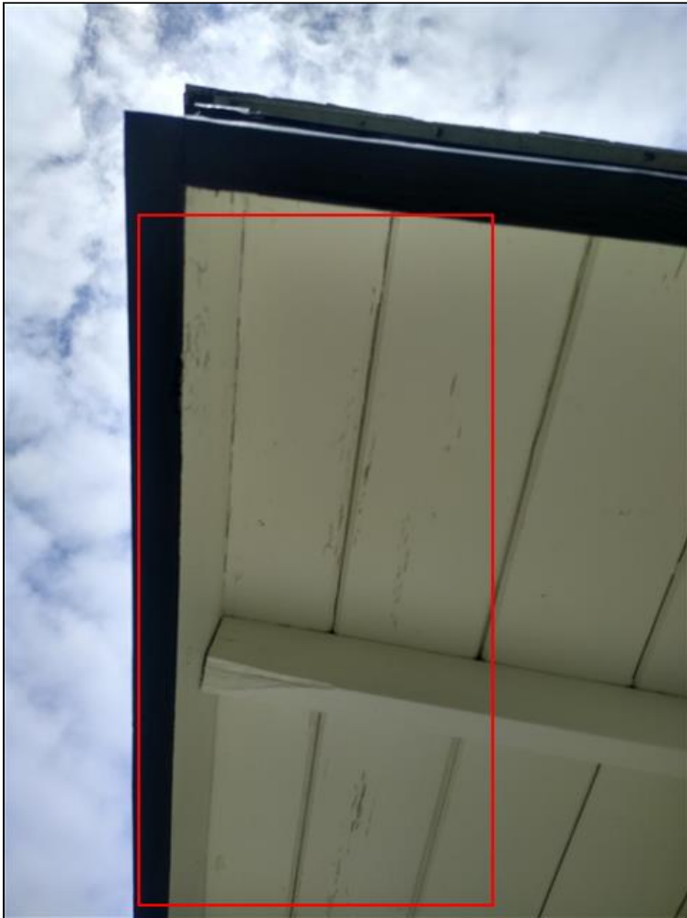
1.6 Item 4(Picture) Wear noted at paint
