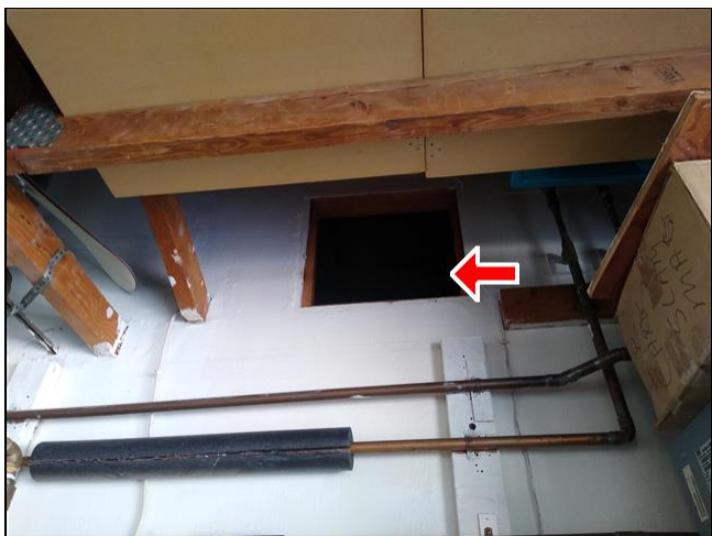
3.2 Item 3(Picture) Attic access opening does not have a fire-rated door assembly.
