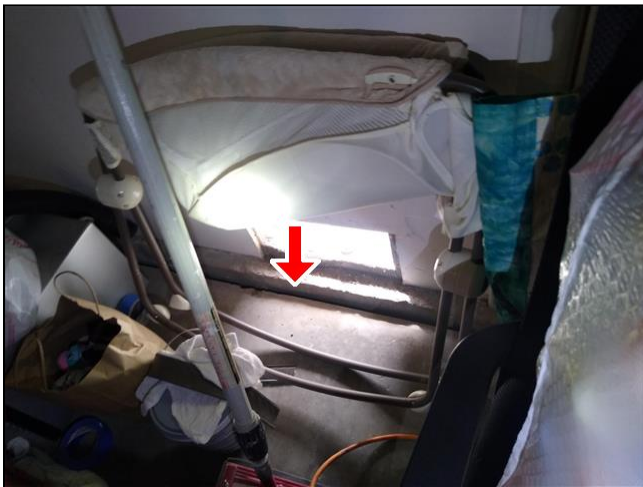
3.1 Item 3(Picture) Gap noted where garage floor slab meets curb
