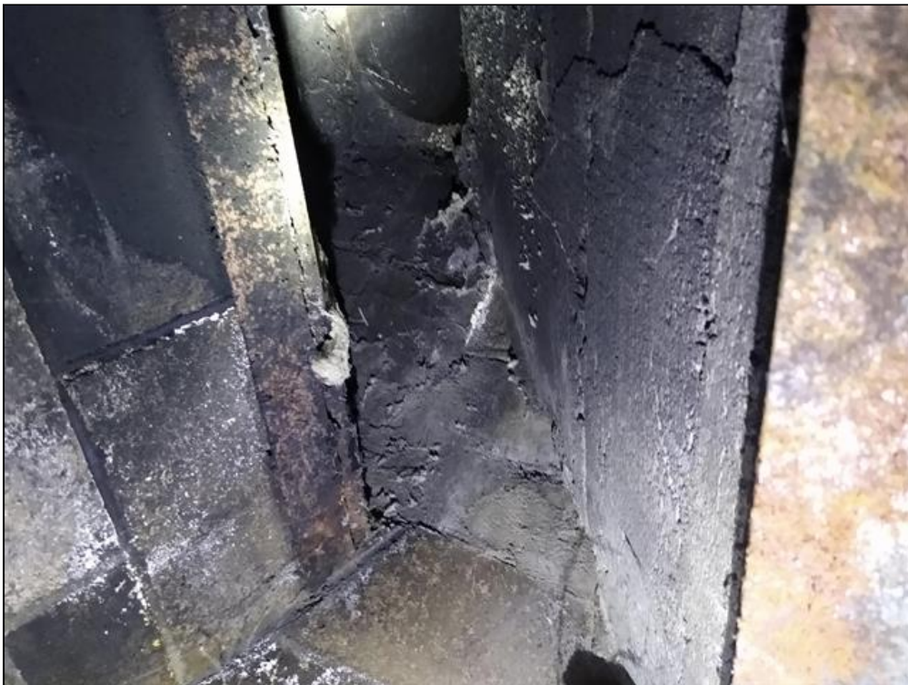
4.6 Item 4(Picture) View into smoke chamber on left side
