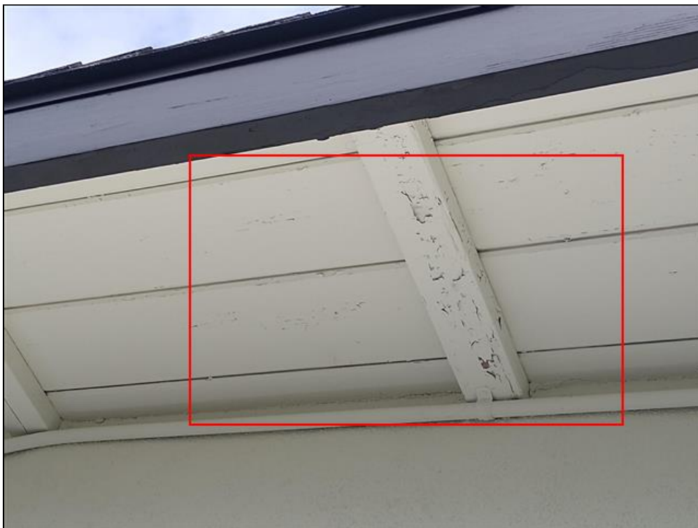
1.6 Item 5(Picture) Peeled paint noted
