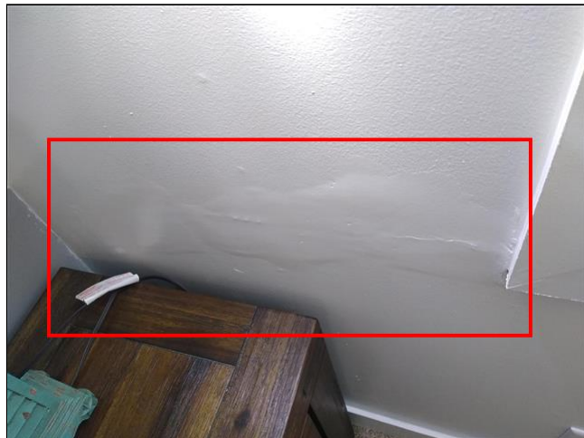
4.0 Item 4(Picture) Patching/repairs noted at front bedroom wall by window
