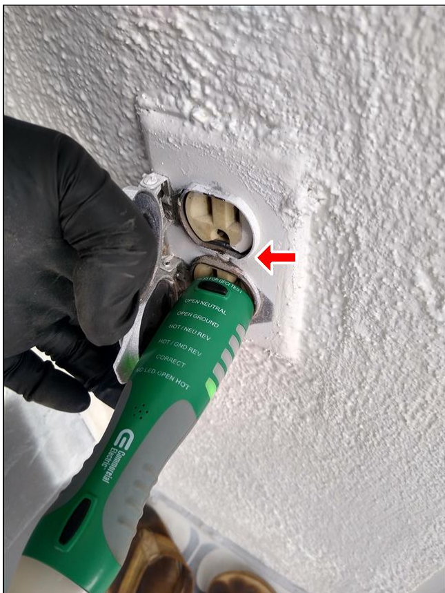
7.3 Item 1(Picture) Exterior outlets, Not GFCI. No weather covering noted (rear area)
