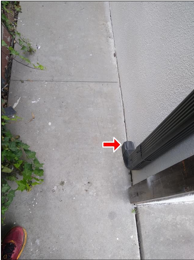
1.5 Item 1(Picture) Downspout terminates by base of structure. Recommend repairs and adding downspout extender/splash block.
