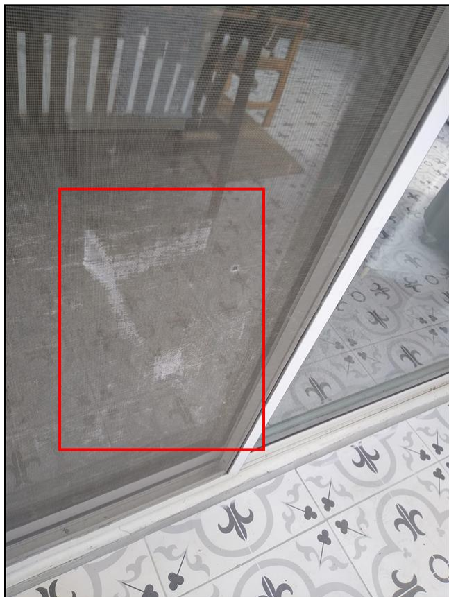
4.4 Item 3(Picture) Wear noted at sliding screen door
