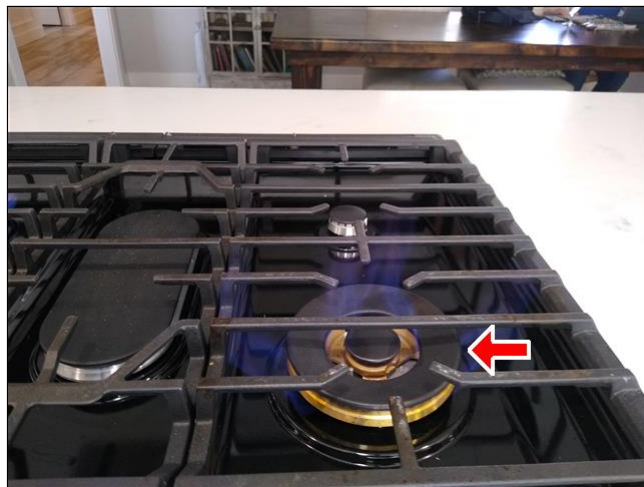
10.2 Item 2(Picture) Front right burner produced uneven flames
