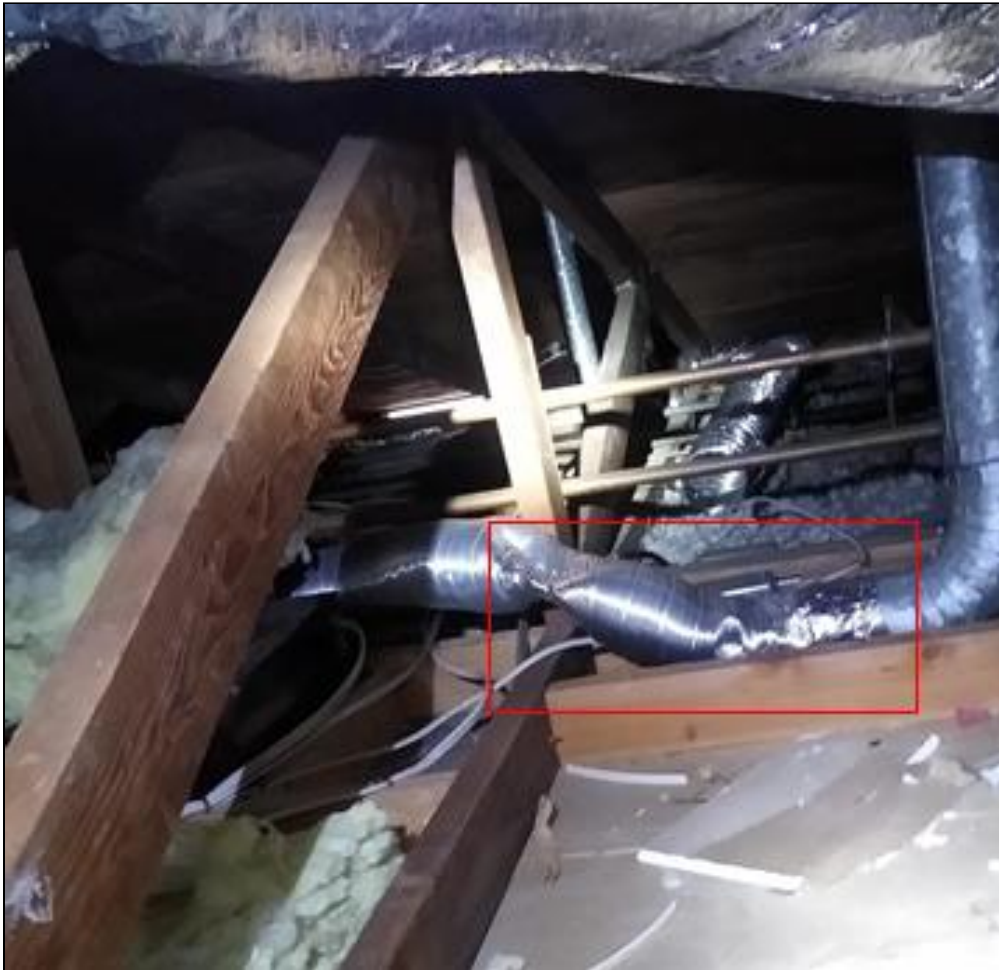
9.2 Item 1(Picture) Bath exhaust ducting is kinked
