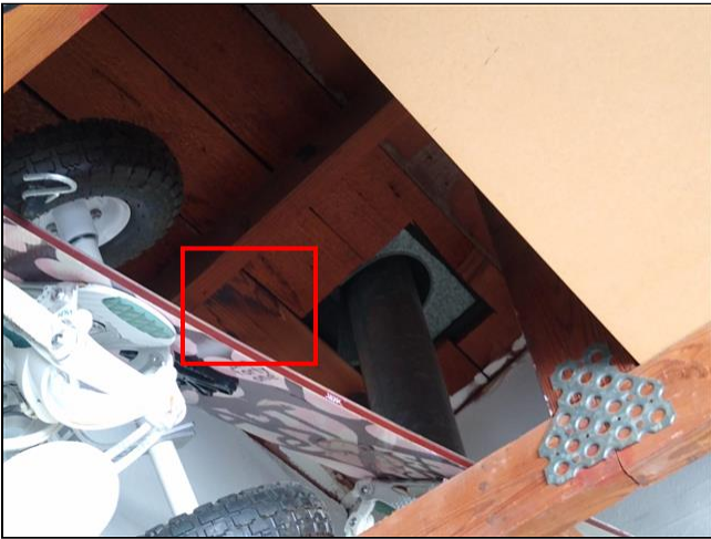
3.0 Item 1(Picture) Staining noted
