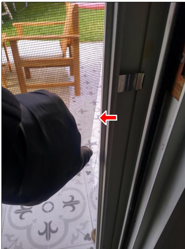
4.4 Item 4(Picture) Wear noted at sliding screen door
