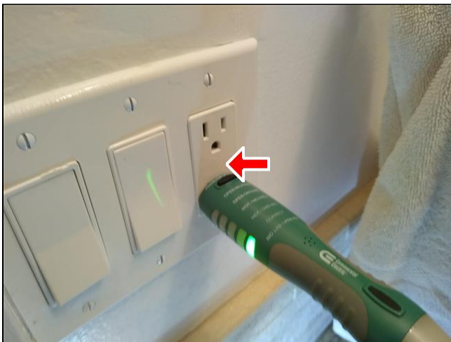
7.3 Item 9(Picture) Shared bathroom outlets, Not GFCI
