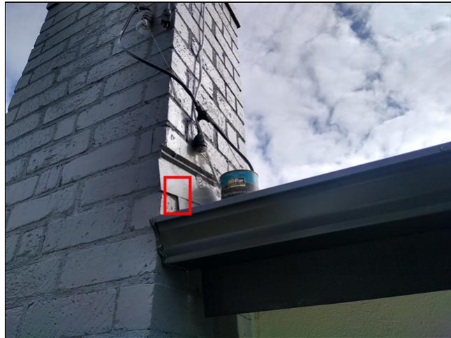
1.1 Item 3(Picture) No kick out flashings noted at both sides of chimney (above rain gutters)
