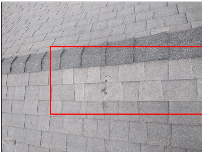
1.0 Item 6(Picture) Wear noted
