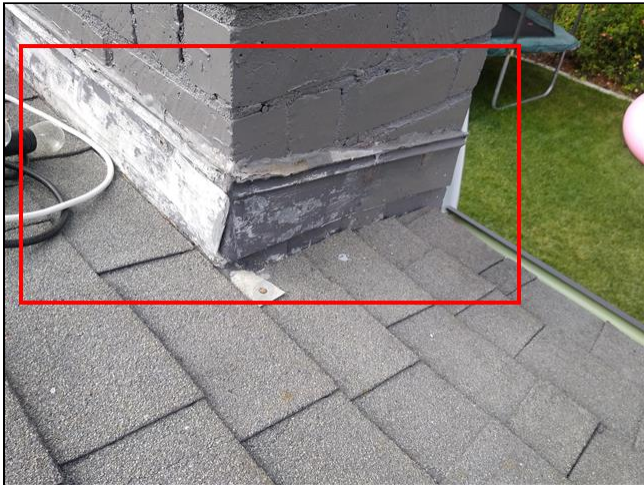
1.1 Item 2(Picture) Older/worn flashings noted
