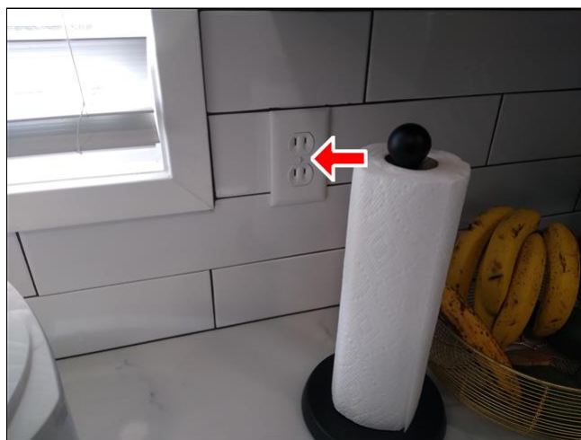
7.3 Item 12(Picture) Kitchen countertop outlets are Two-prong, Not GFCI
