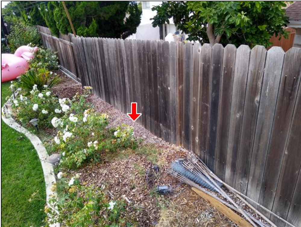
2.6 Item 4(Picture) High soil noted
