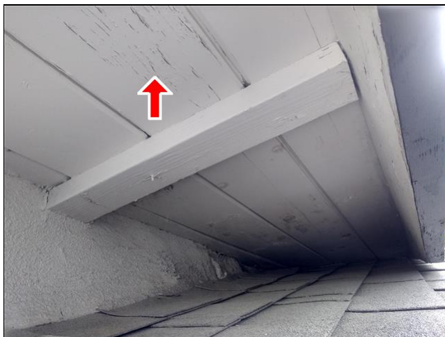
1.6 Item 2(Picture) Wear noted at paint under soffit
