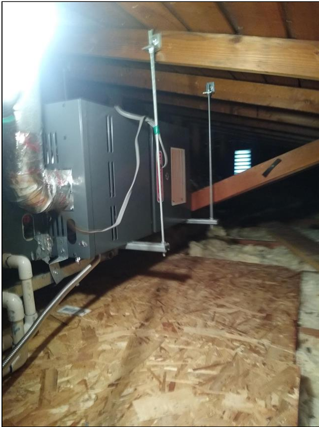
8.5 Item 1(Picture) Goodman gas-fueled furnace
