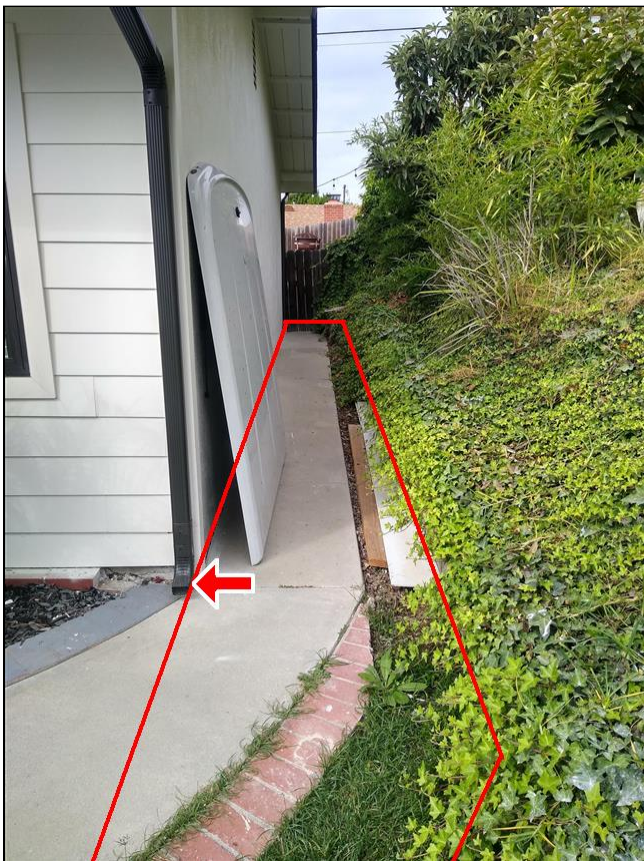
2.7 Item 1(Picture) Area of drainage concern with nearby downspout
