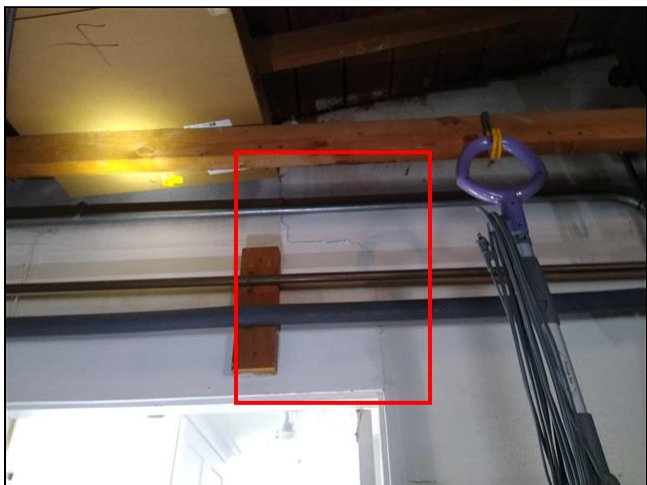
3.2 Item 1(Picture) Cracking noted at wall by garage door, possibly due to settlement.
