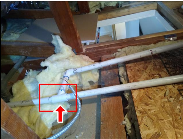
8.3 Item 1(Picture) Primary and secondary condensate lines connect, which is not permitted
