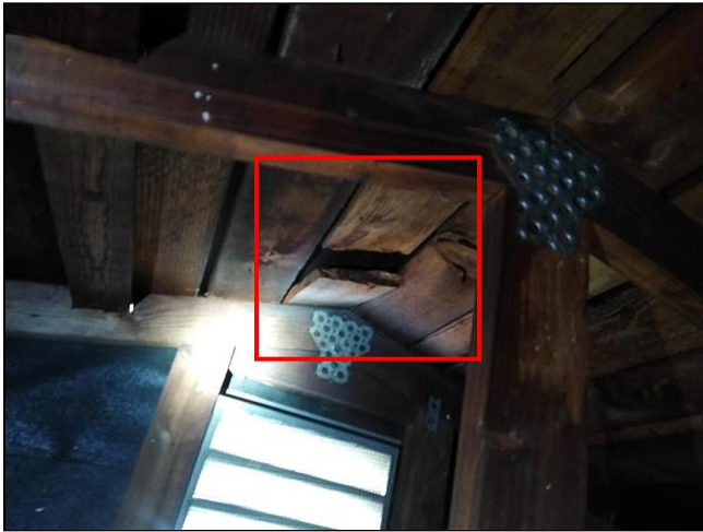
9.0 Item 2(Picture) Broken sheathing noted at ridge area, E
