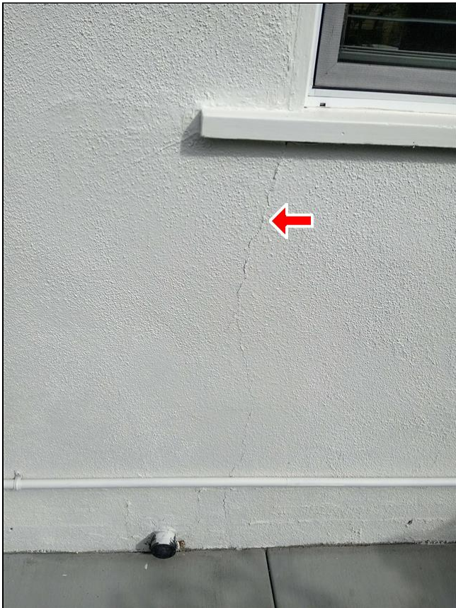
2.0 Item 4(Picture) Cracking noted
