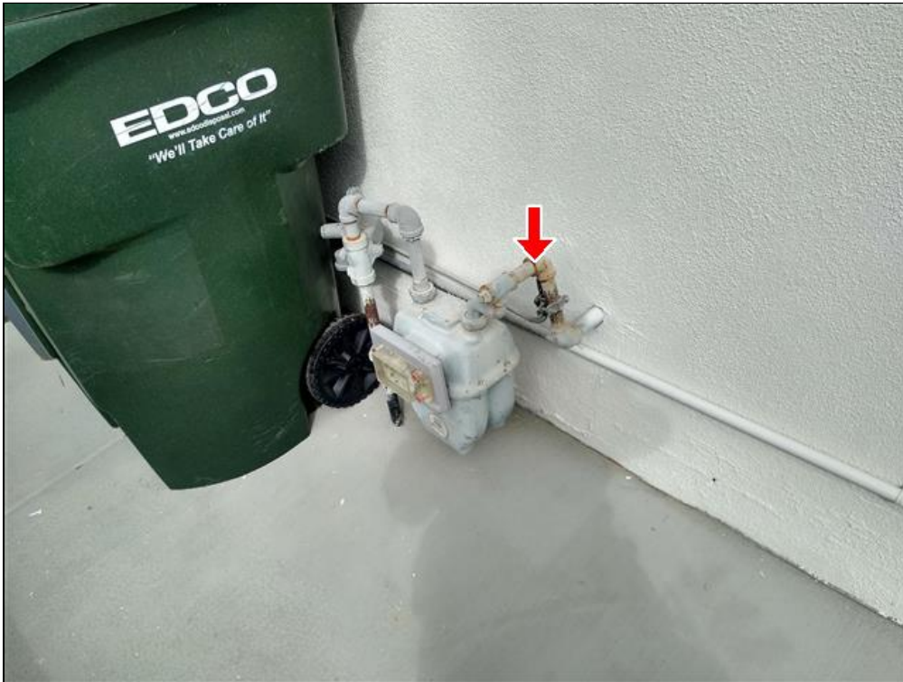
6.5.A Item 1(Picture) No seismic shut-off valve noted
