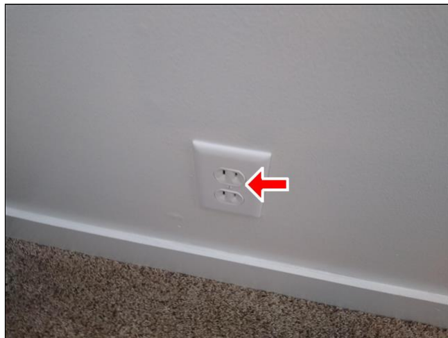
7.3 Item 10(Picture) Two-prong outlets noted, living room
