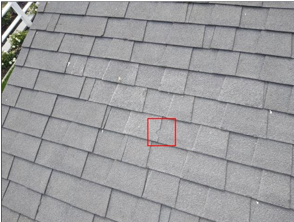
1.0 Item 1(Picture) Wear noted
