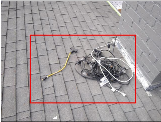
7.4 Item 1(Picture) Extension cord wiring noted behind chimney
