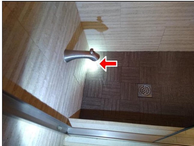
6.2.B Item 2(Picture) Shower diverter does not work properly
