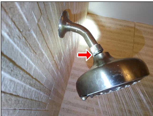
6.2.B Item 3(Picture) Leak noted at shower head
