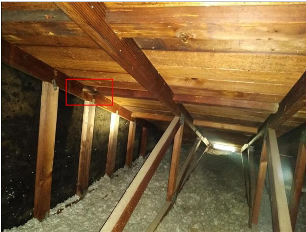
9.1 Item 5(Picture) Staining noted at gable
