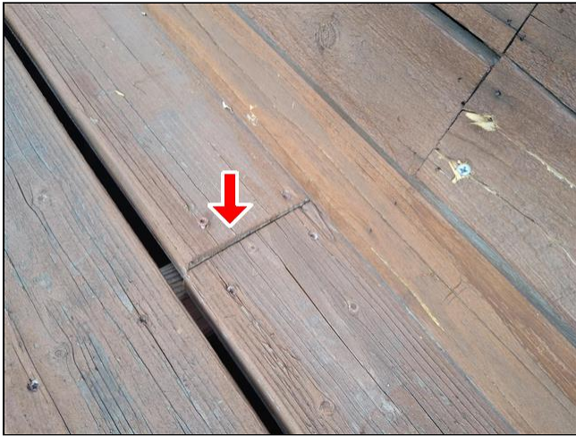
2.2 Item 9(Picture) Warping, loose plank noted with protruding screw, left area of benching
