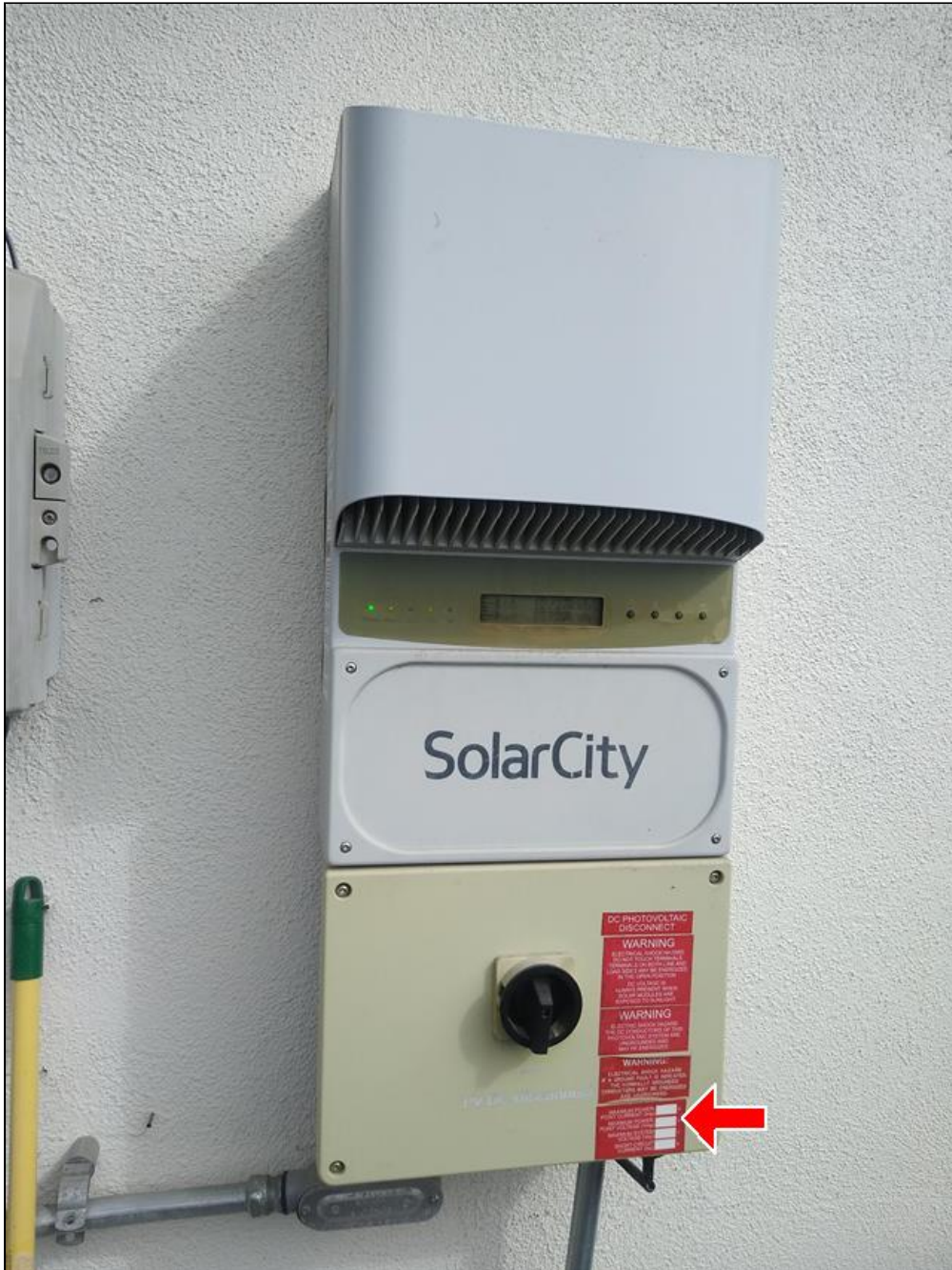
7.1 Item 5(Picture) Voltage and amperage are not on display for emergency services
