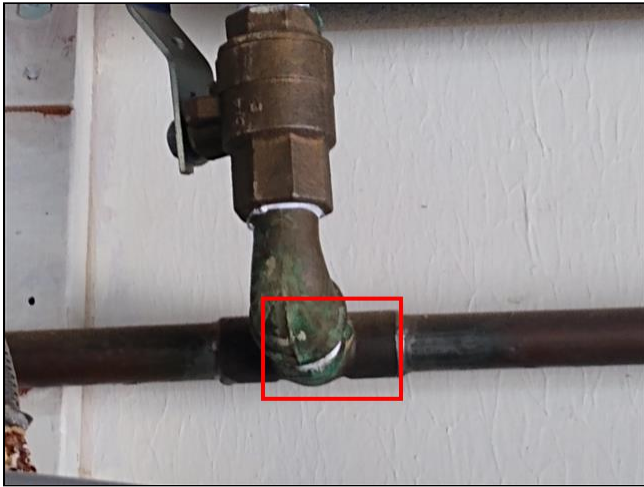
6.6.A Item 5(Picture) Corrosion noted
