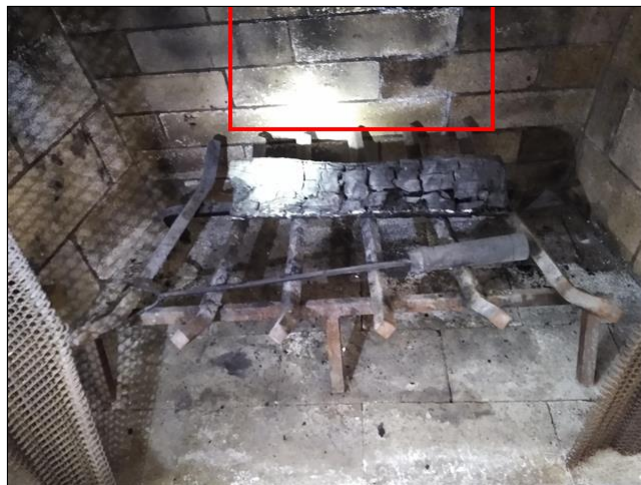
4.6 Item 2(Picture) Efflorescence noted, which may indicate water intrusion from exterior. (See comments under Roofing: Chimney section).
