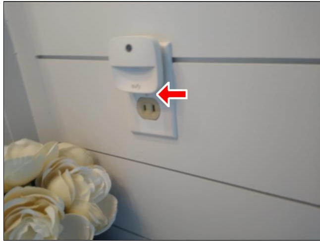
7.3 Item 8(Picture) Master bathroom outlets are Two-prong, Not GFCI
