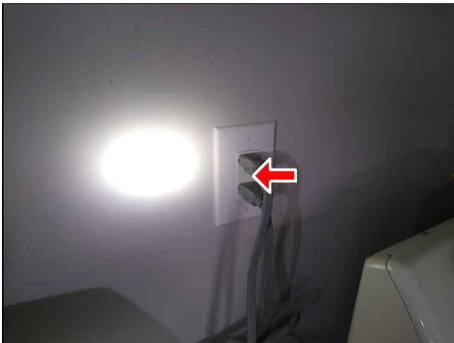
7.3 Item 5(Picture) Laundry area outlets, Not GFCI
