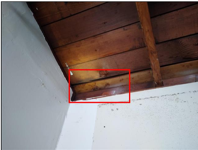
3.0 Item 3(Picture) Staining noted
