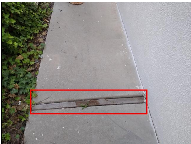
2.5 Item 1(Picture) Uneven surfaces noted, E
