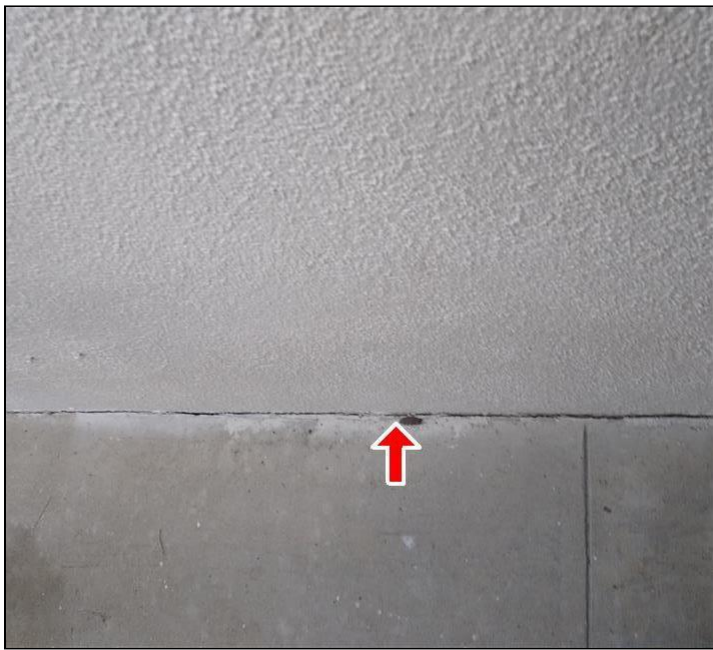
2.0 Item 9(Picture) Recommend sealing where pavement meets siding with elastomeric expansion joint.
