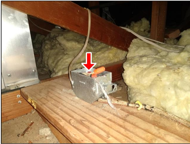
7.4 Item 4(Picture) Open junction box noted near attic access door
