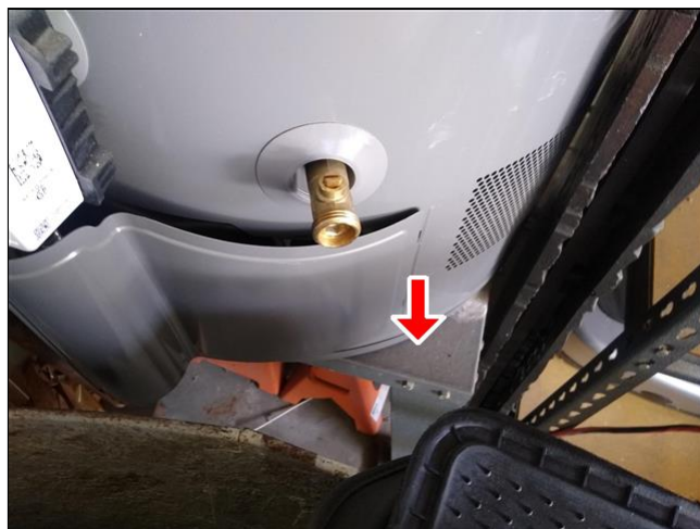
6.6.A Item 2(Picture) No overflow pan noted.
