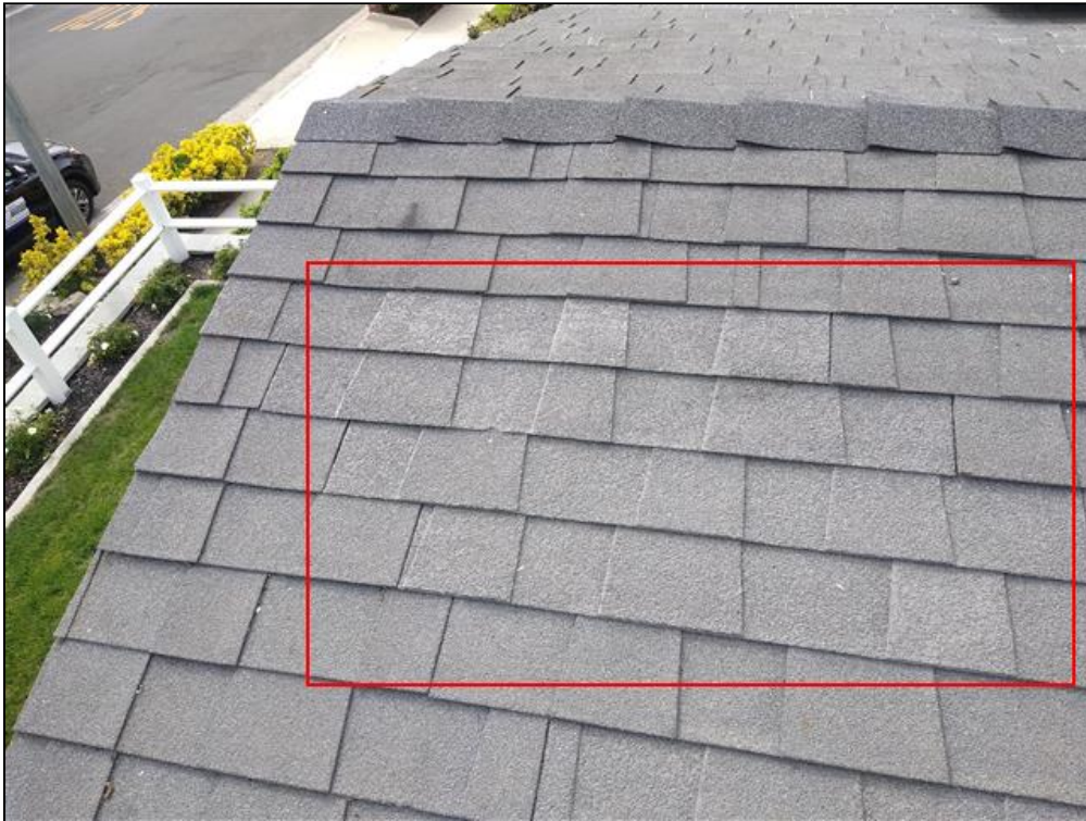
1.0 Item 2(Picture) Wear noted
