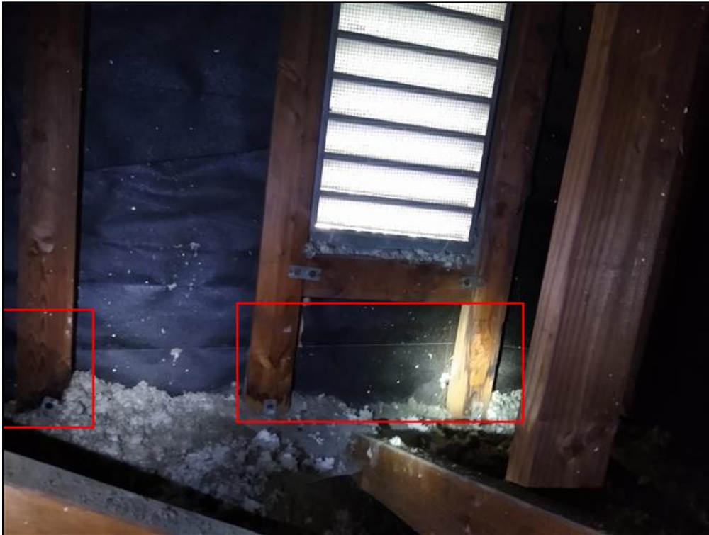
9.1 Item 6(Picture) Staining noted
