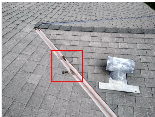
1.0 Item 8(Picture) Debris noted
