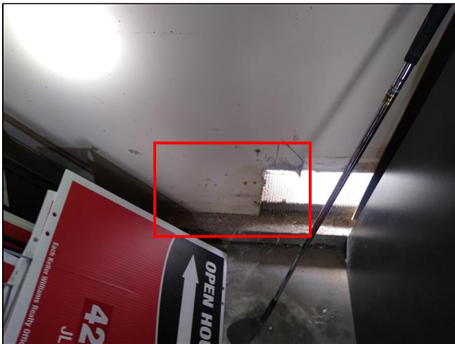
3.2 Item 5(Picture) Staining noted at drywall by garage vent opening.
