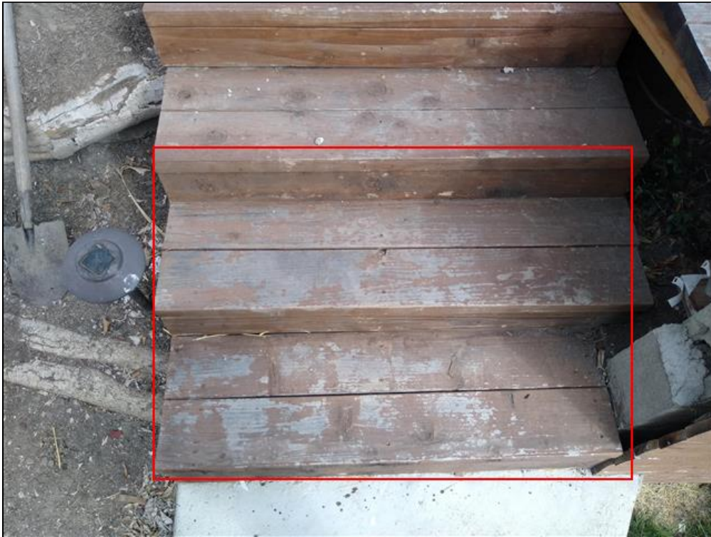
2.2 Item 4(Picture) Wear noted at deck
