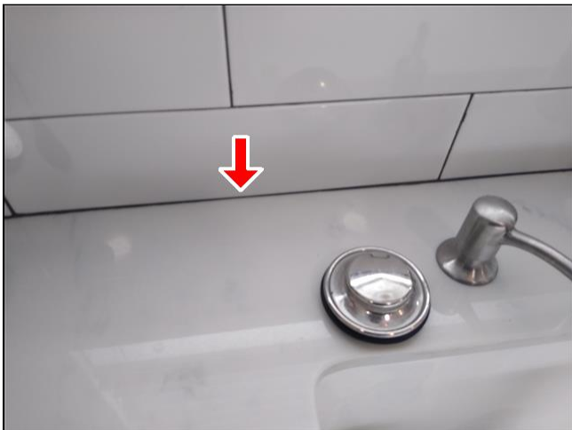
10.9 Item 1(Picture) Recommend caulking where countertop meets backsplash
