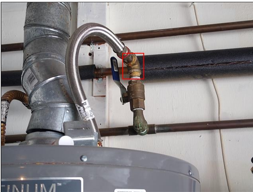
6.6.A Item 6(Picture) Corrosion noted
