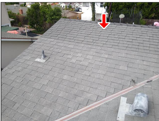
1.0 Item 7(Picture) Repairs noted
