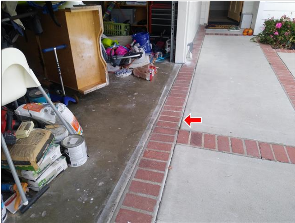
2.4 Item 2(Picture) MAINTENANCE TIP: Suggest repairs/sealing with elastomeric expansion joint to prevent water seepage and subsequent differential settlement/cracking
