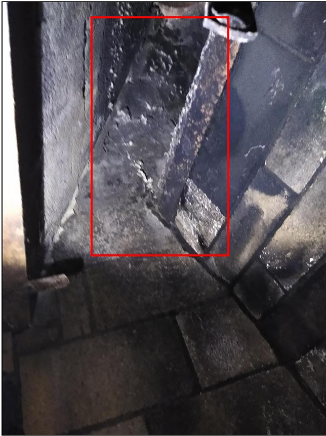
4.6 Item 3(Picture) Uneven surfaces noted in smoke chamber area. Efflorescence also noted.
