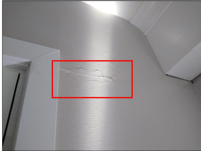
4.0 Item 2(Picture) Patching/repairs noted at wall near laundry area
