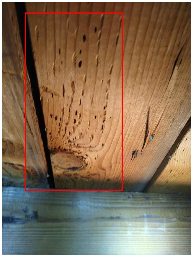
9.1 Item 1(Picture) Wood damage noted
