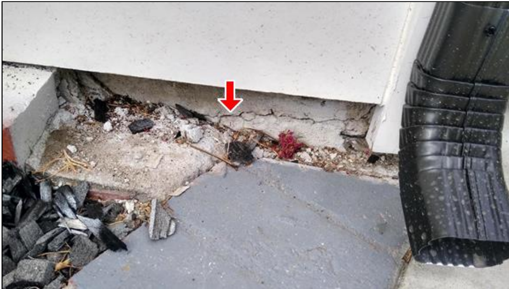
5.1 Item 2(Picture) Close-up of cracking
