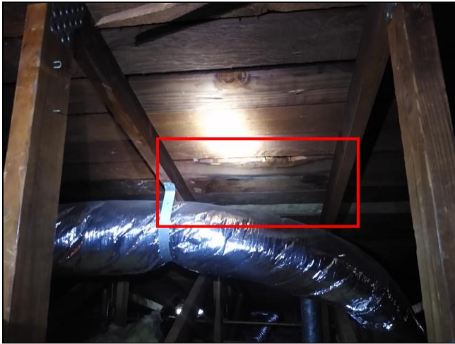
9.1 Item 3(Picture) Staining noted
