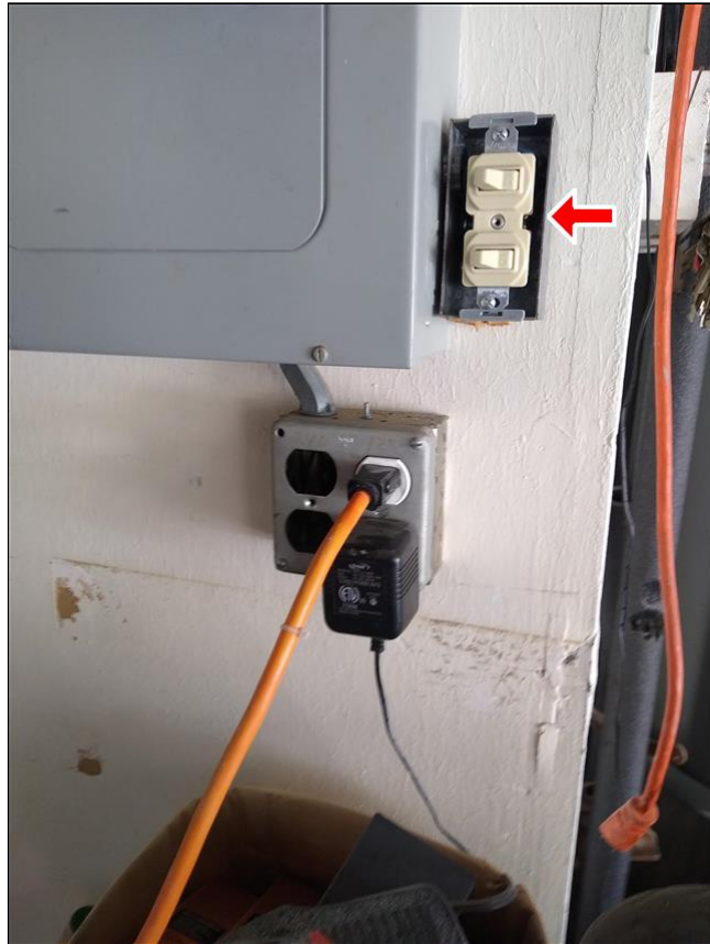
7.3 Item 4(Picture) Missing coverplate noted at garage light switch
