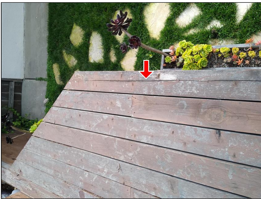
2.2 Item 7(Picture) Splitting noted at plank. Suggest repairs/ replacement.
