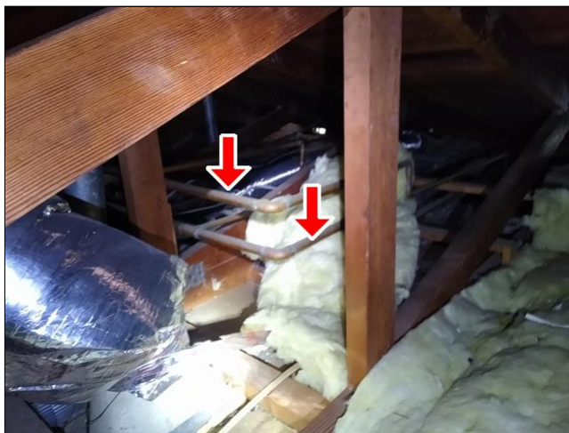
6.0.A Item 2(Picture) OPTION: Insulate copper supply piping in attic area for improved efficiency in retaining temperature
