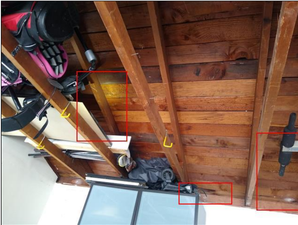
3.0 Item 2(Picture) Staining noted
