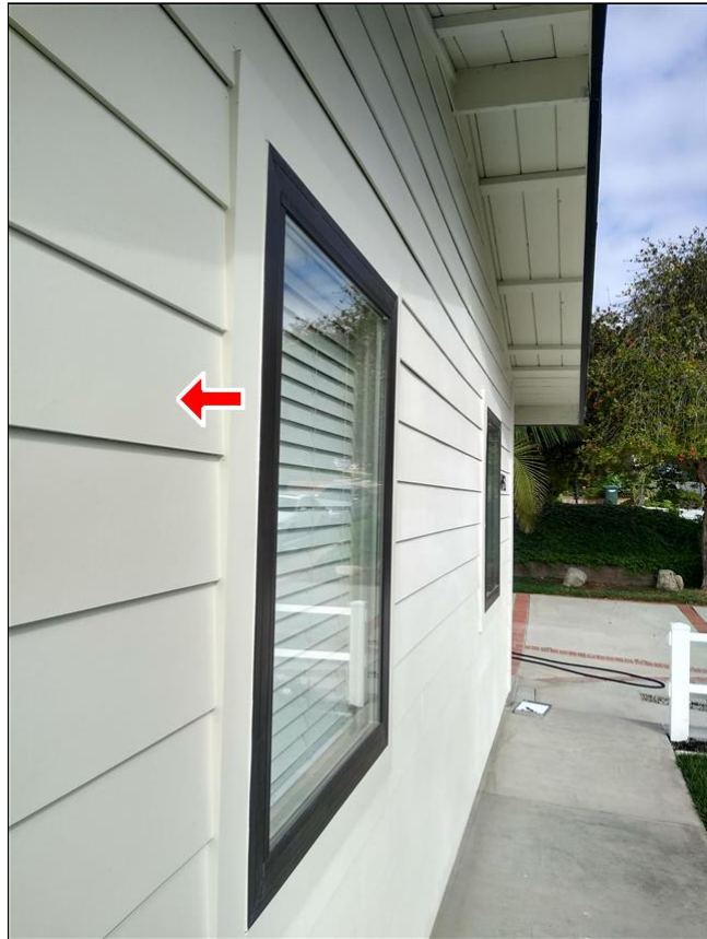
2.0 Item 6(Picture) Composite siding noted
