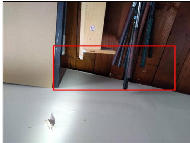
3.0 Item 4(Picture) Staining noted
