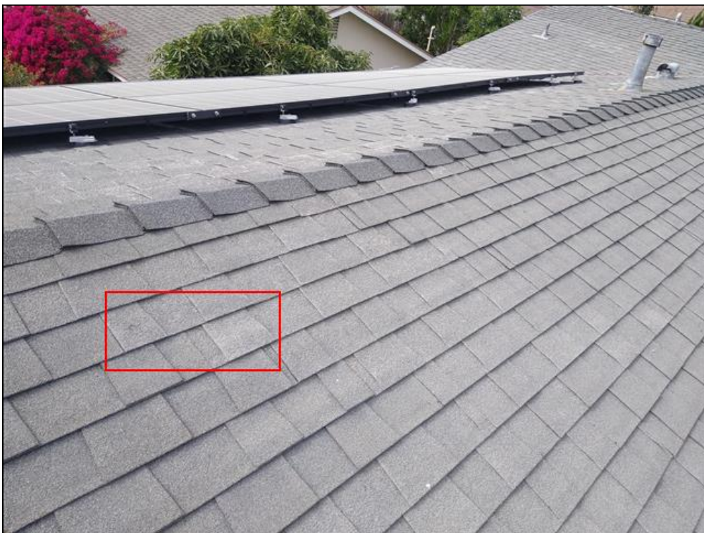
1.0 Item 3(Picture) Wear noted
