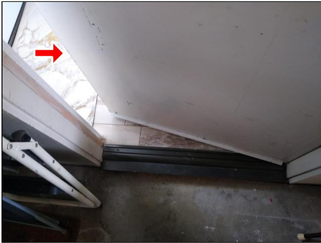
3.2 Item 4(Picture) Door admitting to the garage does not self-close/self-latch
