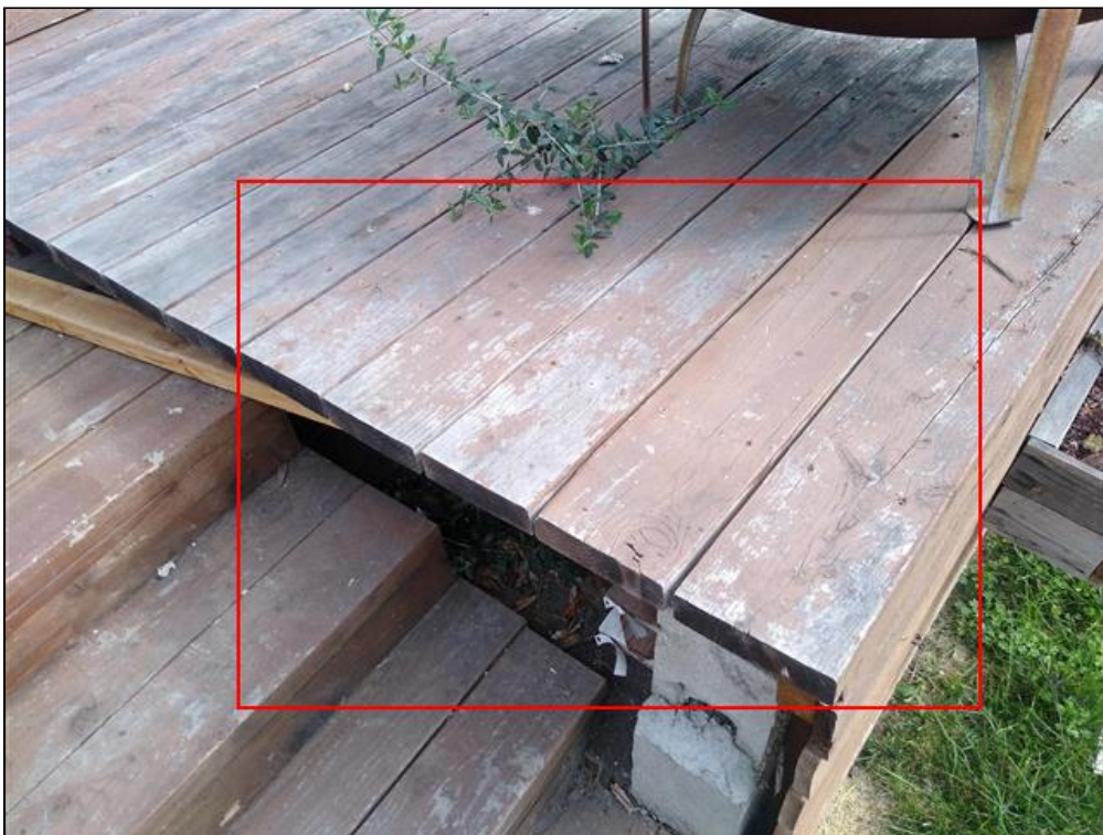
2.2 Item 5(Picture) Wear noted at deck
