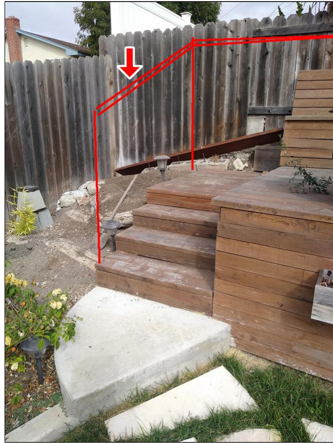
2.2 Item 3(Picture) No handrailing noted
