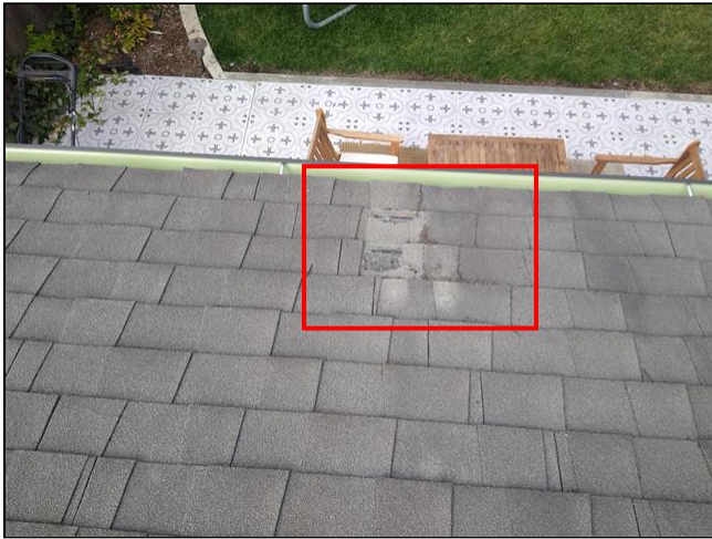
1.0 Item 10(Picture) Wear noted at shingles
