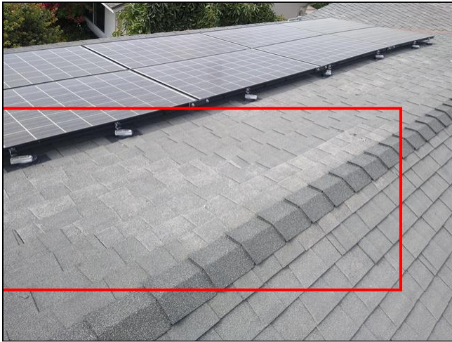
1.0 Item 4(Picture) Wear noted
