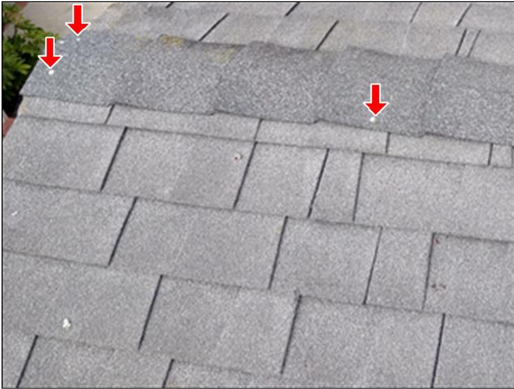
1.0 Item 9(Picture) Exposed fasteners noted
