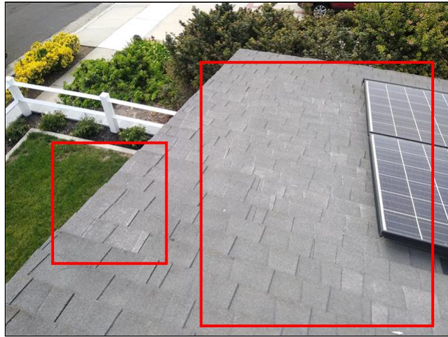
1.0 Item 5(Picture) Wear noted
