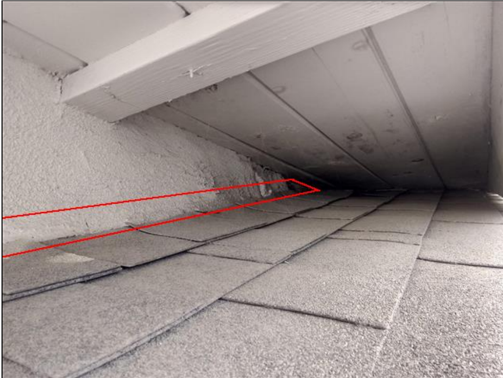
1.2 Item 1(Picture) No flashings noted, central/W
