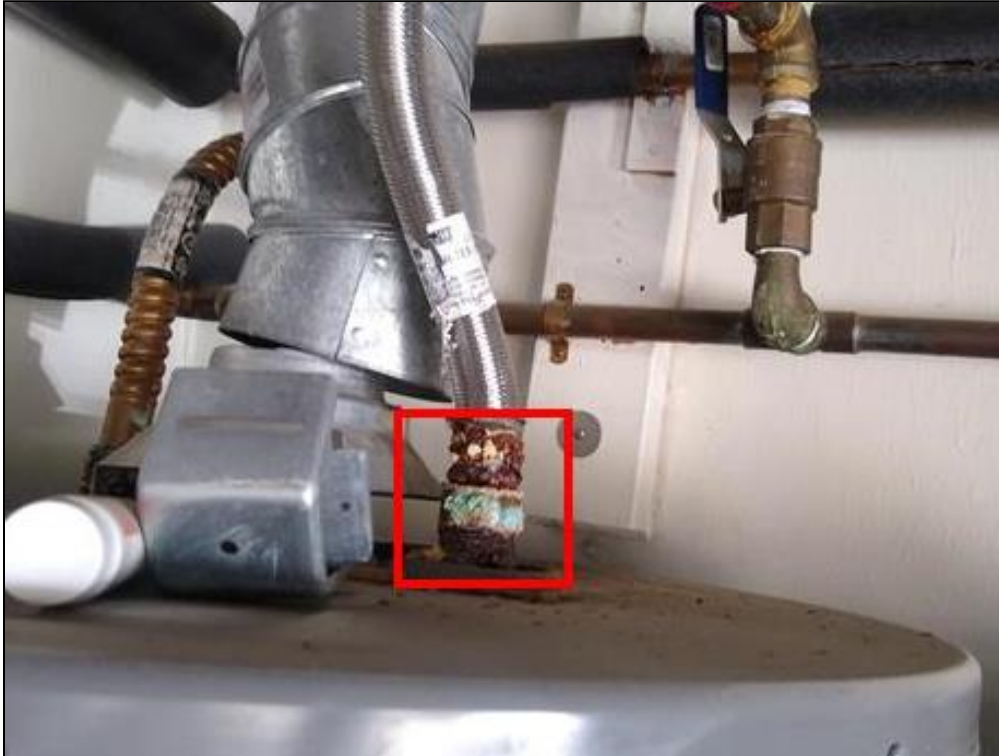
6.6.A Item 4(Picture) Corrosion noted
