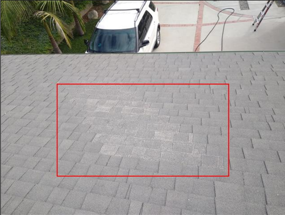
1.0 Item 12(Picture) Wear noted
