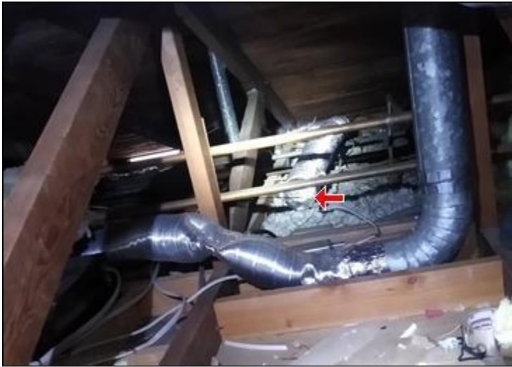
9.2 Item 2(Picture) Exhaust ducting terminates in attic area
