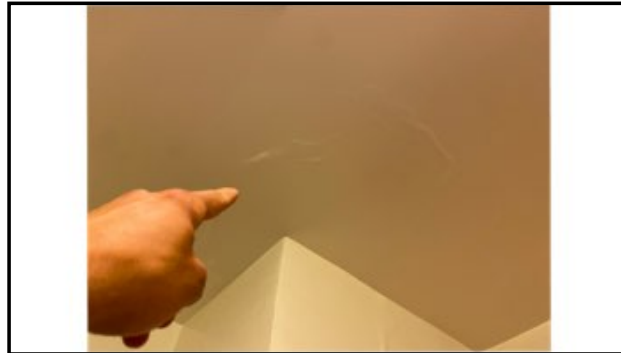
Peeling/blistered/cracking paint in areas
