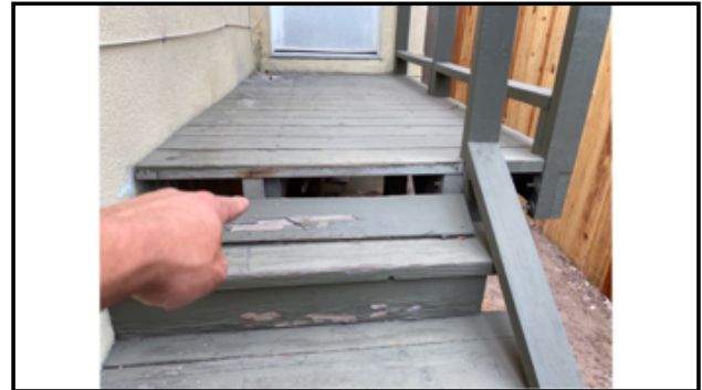
Displaced/lifted/uneven areas trip hazard - needs to be serviced
