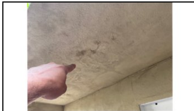
Moisture damage - needs to be serviced
