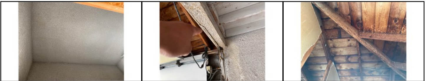
Cracking larger than typical - needs to be evaluated/serviced
