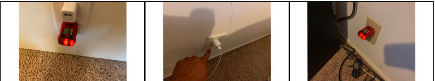
Ungrounded outlets present - typical for the age of the structure - consider upgrading electrical services
