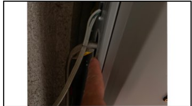
Flexible connector through sheet metal cabinet - needs to be serviced
