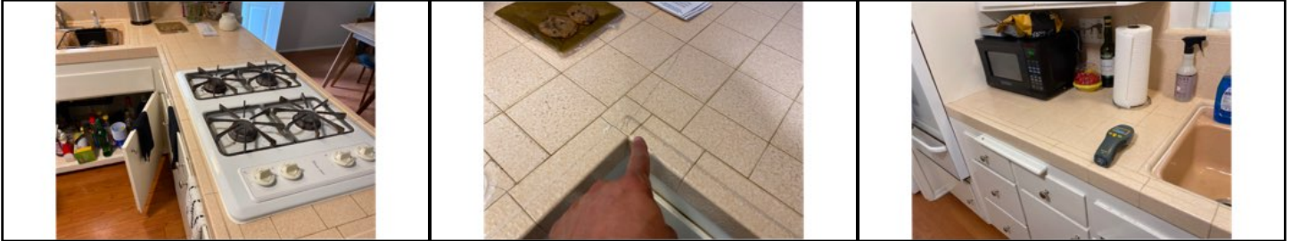
Cracked materials - needs to be serviced
