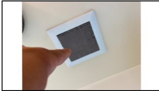
Dirty/dusty unit - recommend cleaning
