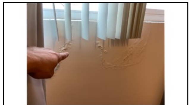
Moisture damaged - needs to be serviced/further evaluated-711
