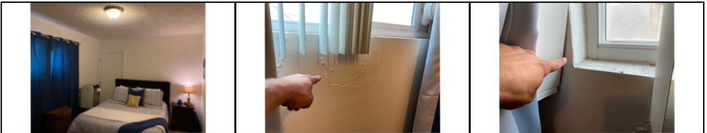
Peeling/blistered/cracking paint in areas
