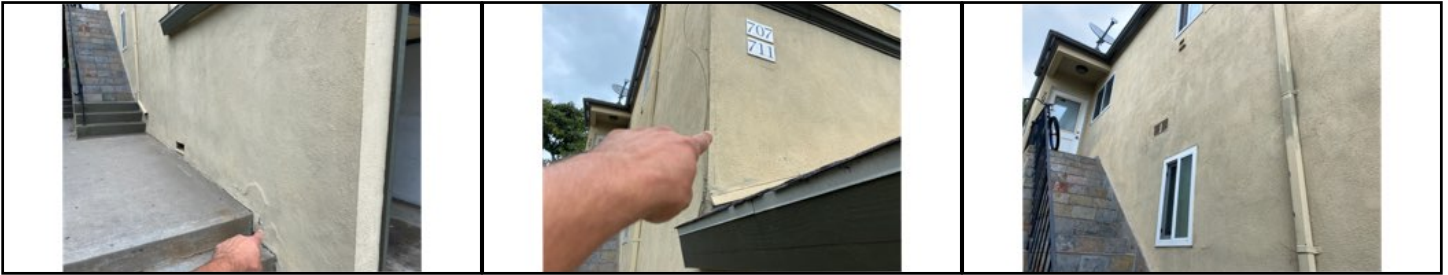
Color coat deteriorated near grade due to moisture - recommend gutters and drainage to help keep moisture away from structure
