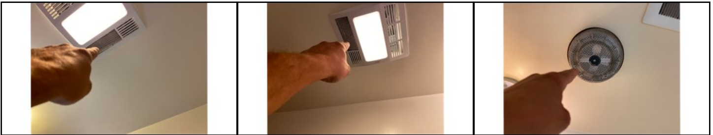
Tested and did not operate - needs to be serviced
