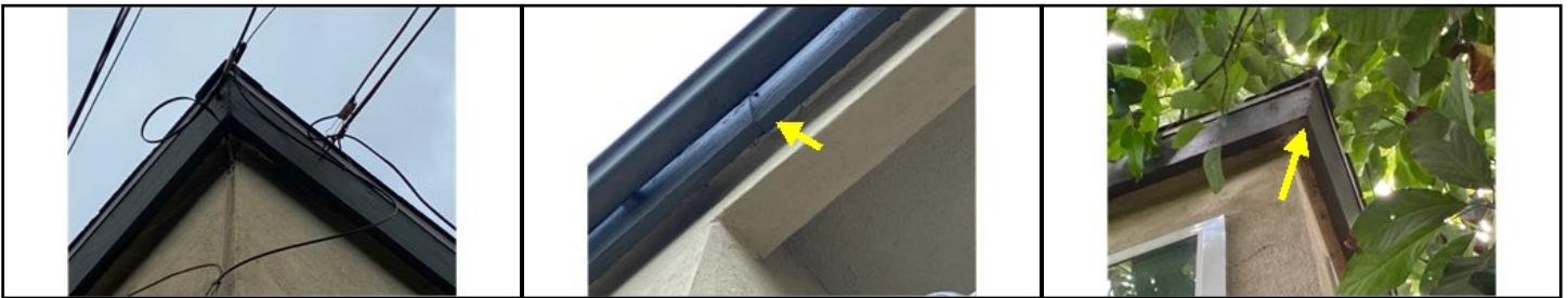
Warped wood / twisted wood - signs of age and wear - needs to be serviced
