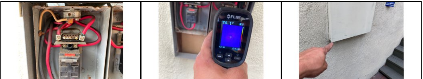
Outer door missing/loose/damaged - needs to be serviced
