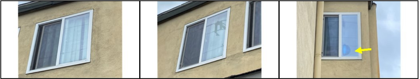
Evidence of internal condensation between glass panes - needs to be serviced - recommend all double-paned glass areas be checked as others may exist
