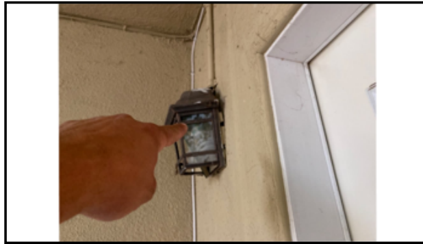
Loose fixture(s) - needs to be serviced
