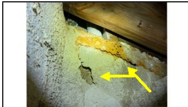
Large holes or cracks observed - needs to be serviced
