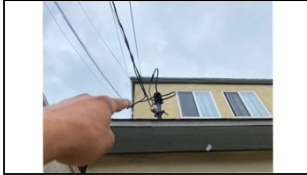
Drip loop not proper configuration - needs to be serviced
