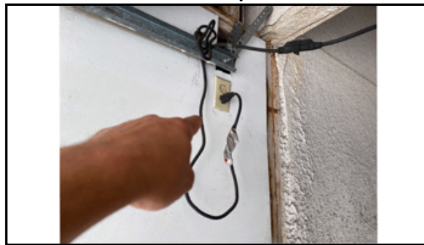
Operates with an extension cord as permanent wiring - recommend contacting a licensed electrical contractor to install a proper outlet near the opener
