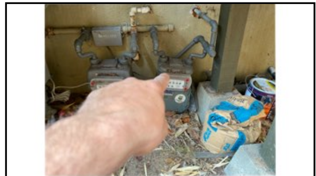
Irregular installation - needs to be serviced- not properly braced
