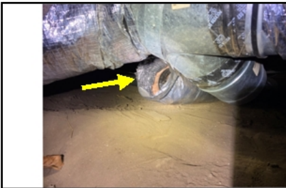
Disconnected - needs to be serviced
