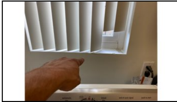
Moisture damaged - needs to be serviced/further evaluated
