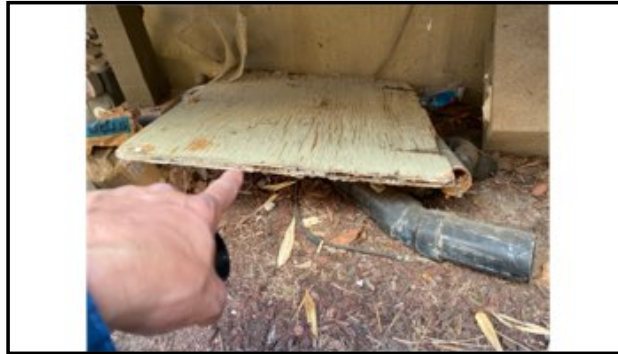
Cover is damaged/cracked/orn - needs to be serviced
