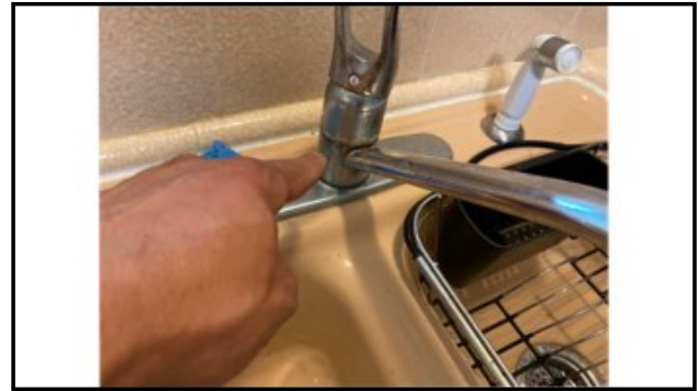
Corrosion present at fixture(s) - signs of wear
