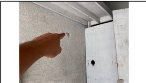
Recommend sealing any holes/gaps/cracks/loose tape – all areas of the firewall should be properly sealed with the correct fire-rated materials
