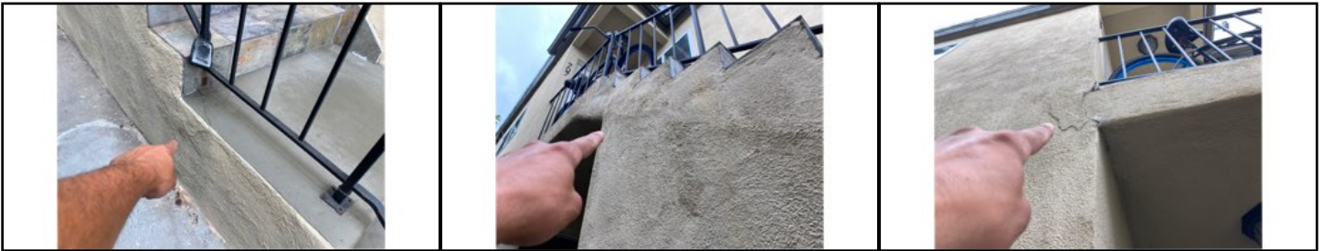
Cracking/chipping/holes more than typical - needs to be serviced
