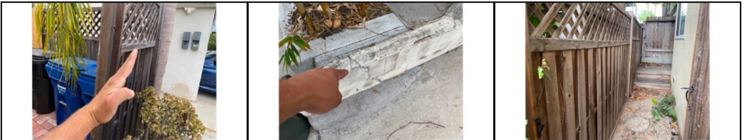
Loose/leaning areas of fencing/walls – needs to be serviced
