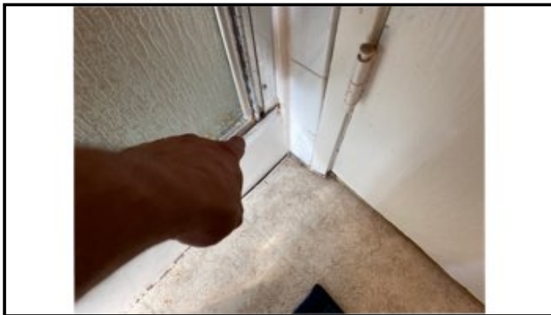
Leakage evident at corners - needs to be serviced- both units
