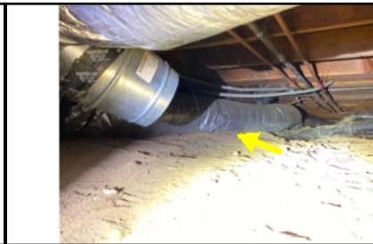
Duct work in contact with soil/lying on ground - needs to be serviced
