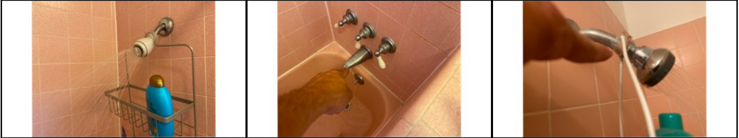
Diverter does not properly divert water to shower head - needs to be serviced-711
