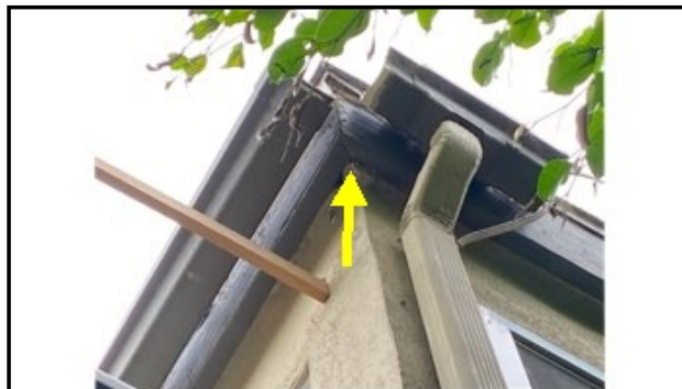
Deteriorated in areas - needs to be serviced - consult the termite report
