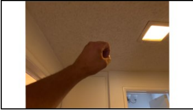
Missing at hall - needs to be installed
