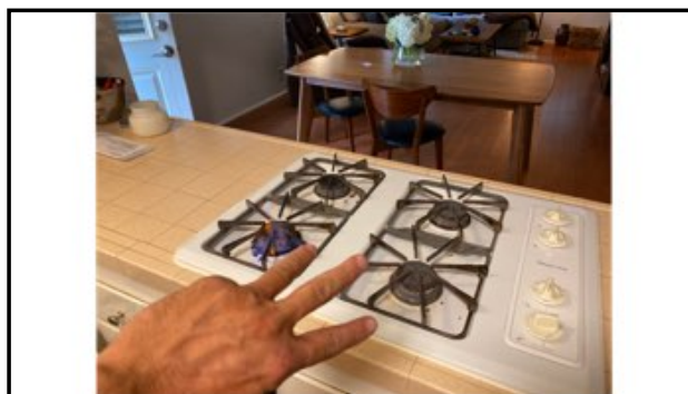
Left rear element/burner not operating - needs to be serviced
