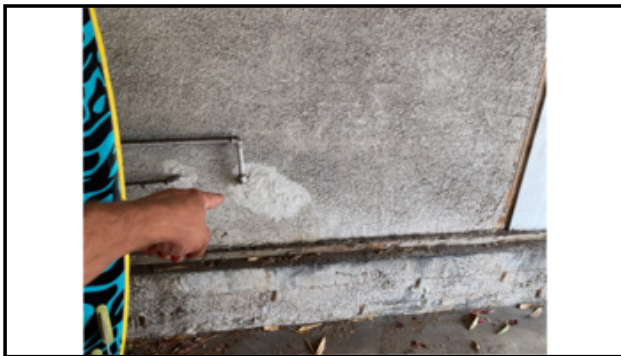
Small holes - recommend patching/painting as needed
