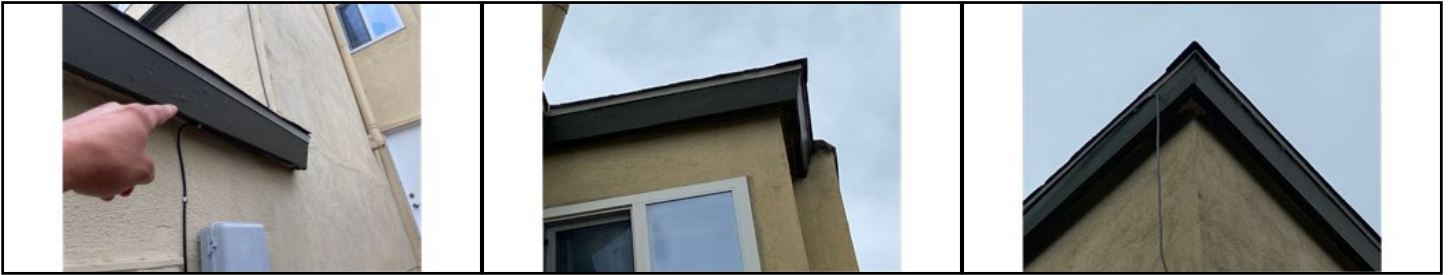
Deteriorated in areas - needs to be serviced - consult the termite report
