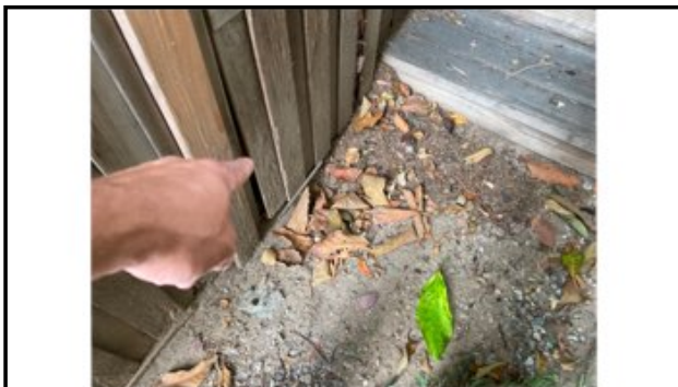
Earth to wood contact present and will reduce the life of wood fencing
