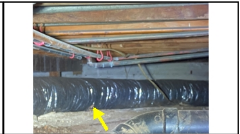
Duct work in contact with soil/lying on ground - needs to be serviced
