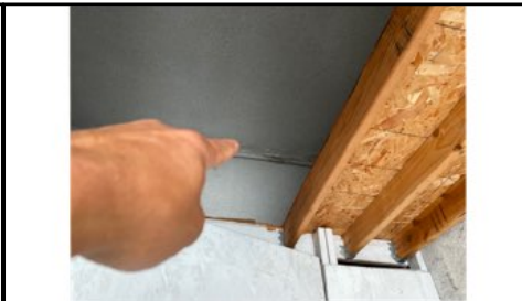
Heavy patched areas - needs to be serviced - condition beneath patches unknown
