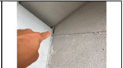
Recommend sealing any holes/gaps/cracks/loose tape – all areas of the firewall should be properly sealed with the correct fire-rated materials
