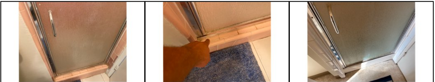
Bottom sweep/seal is missing - needs to be serviced- both units
