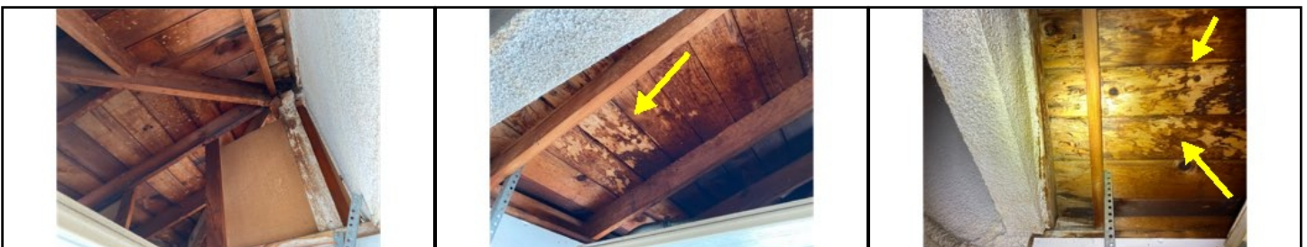
Wood deterioration observed - consult termite report for any wood areas in garage area
