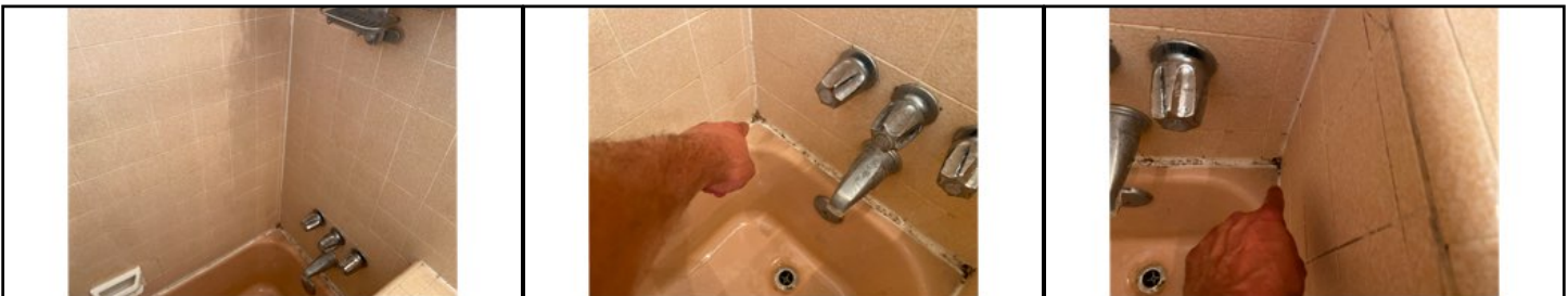
Surface microbial growth/irregular staining is present in areas on nonporous surfaces - recommend cleaning and sealing materials regularly-707 Surface microbial growth/irregular staining is present in areas on nonporous surfaces - recommend cleaning and sealing materials regularly-707
