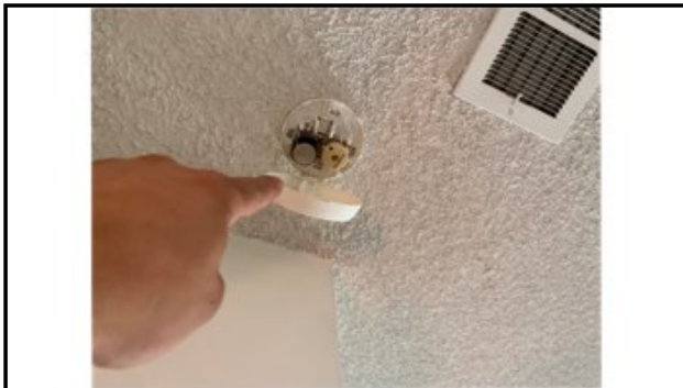
Missing battery - not tested
