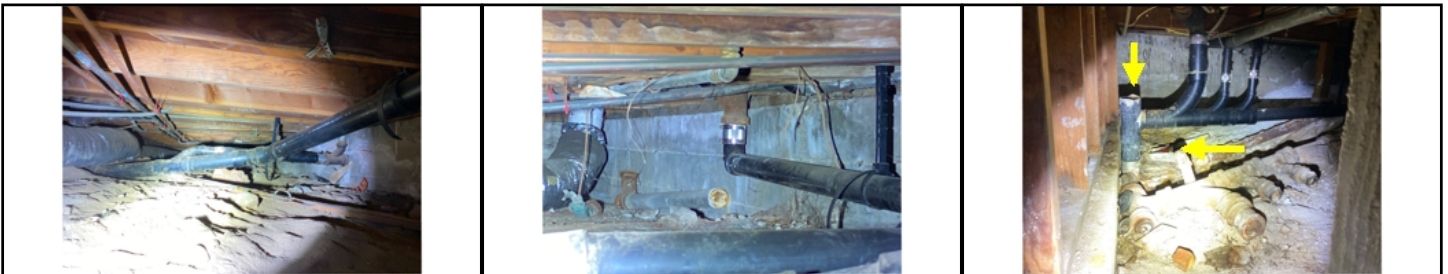
Visibly leaking plumbing - recommend immediate evaluation by a licensed plumber to prevent unwanted moisture in crawl space
