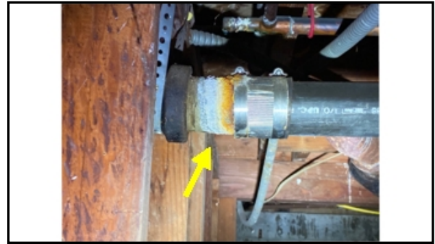
Corrosion present in areas - needs to be serviced
