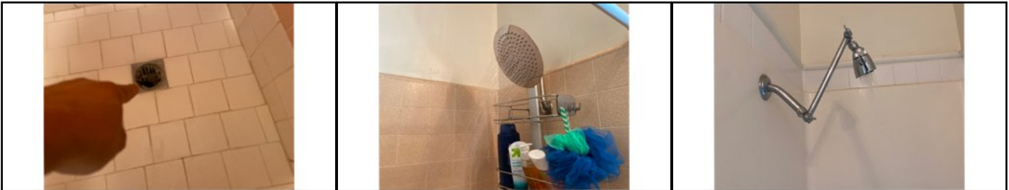
Drain cover is damage - needs to be serviced-711
