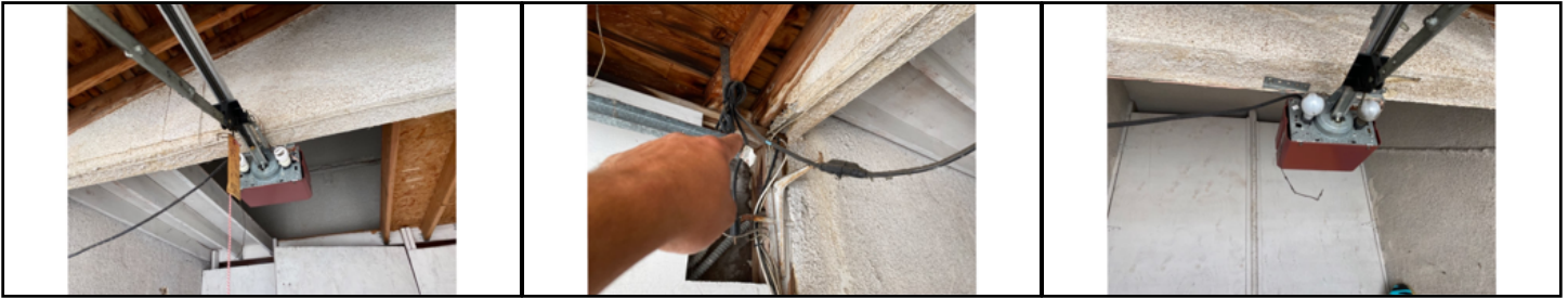
Operates with an extension cord as permanent wiring - recommend contacting a licensed electrical contractor to install a proper outlet near the opener
