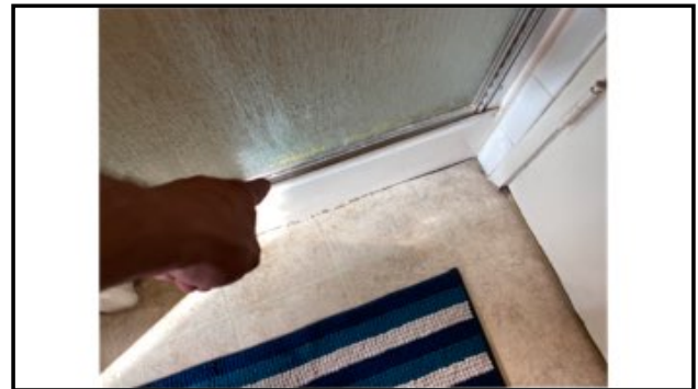
Bottom sweep/seal is missing - needs to be serviced- both units
