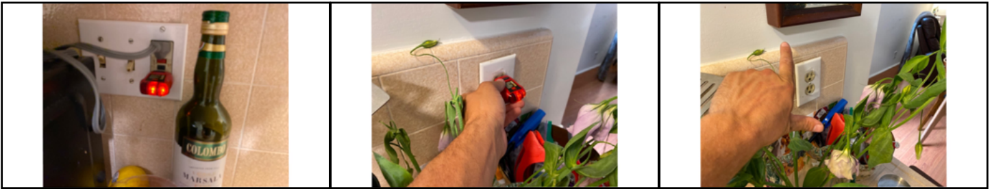
Loose outlets - needs to be serviced
