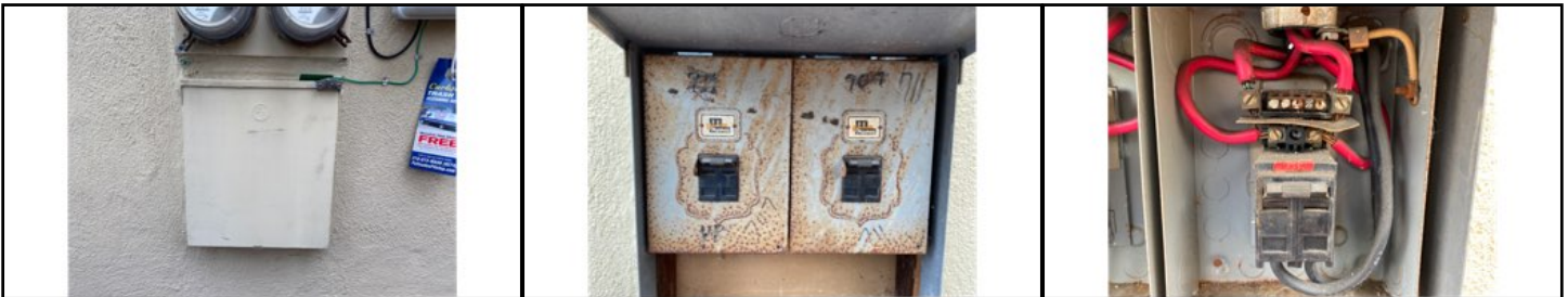
Heavy rusting or rust damage present - needs to be serviced
