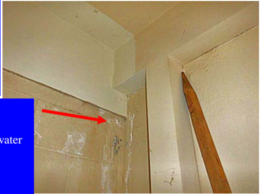
The rear patio N-wall is prone to water infiltration
