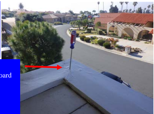
The living room deck surface has developed a few splits at the N-drain area
