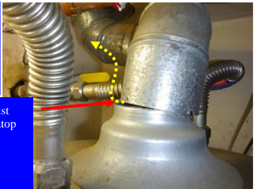
The water heater TPR valve may not use a flexible connector
