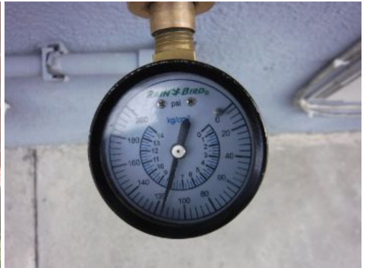
Foundations and Floors Main Water Shut Off/Water Pressure
