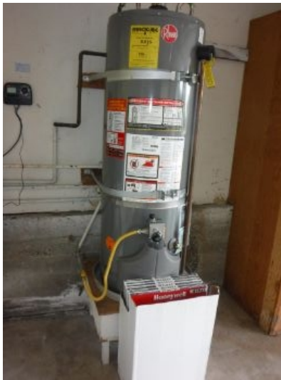
Water Heater Water Heater Condition
