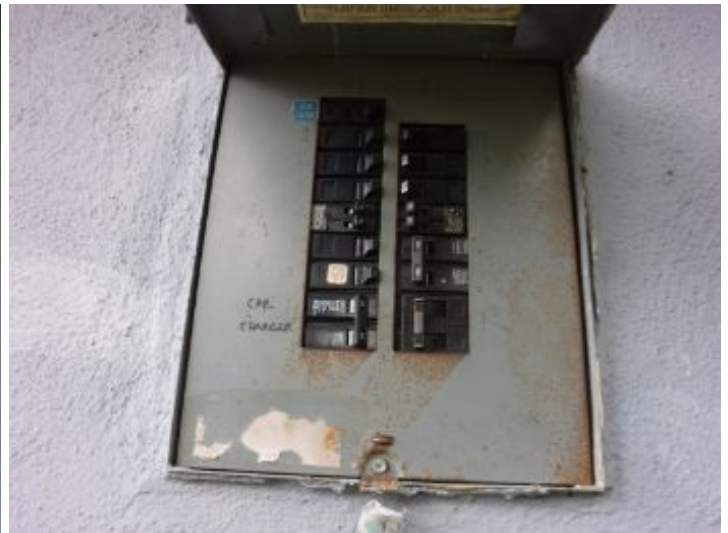
Electrical Electrical Panel
