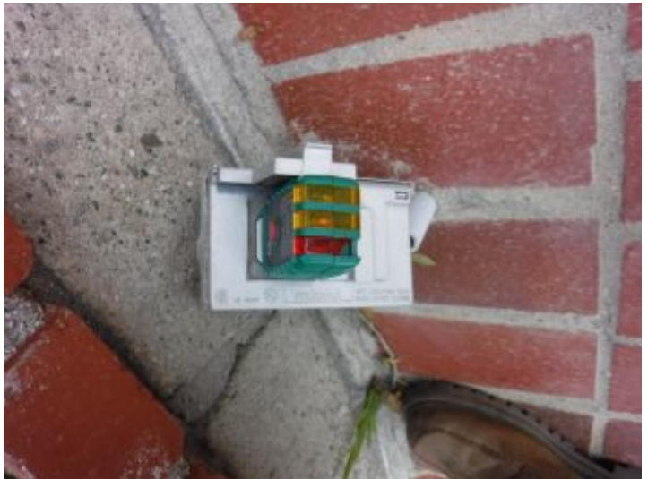
Foundations and Floors Grounds Electrical
