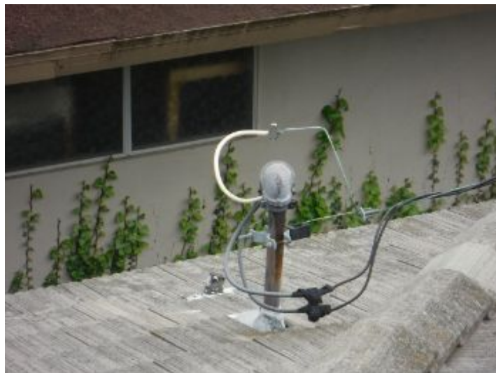
Electrical Cable Feeds
