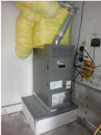
Heat/AC Heater/Ductwork Condition
