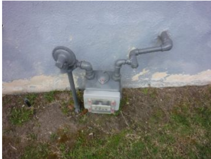
Foundations and Floors Main Gas Valve Condition
