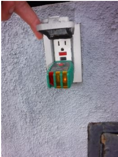
Foundations and Floors Grounds Electrical
