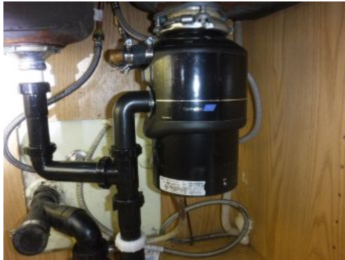
Kitchen Garbage Disposal
