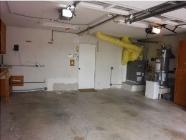
Garage Floor Condition
