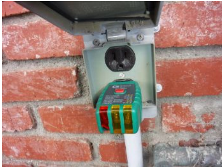
Foundations and Floors Grounds Electrical
