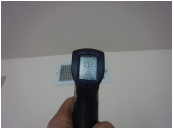
Heat/AC Heater/Ductwork Condition
