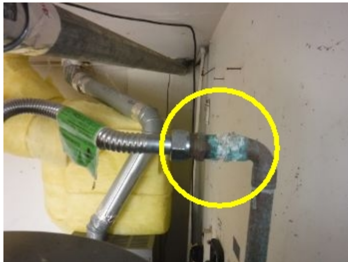
Water Heater Plumbing
