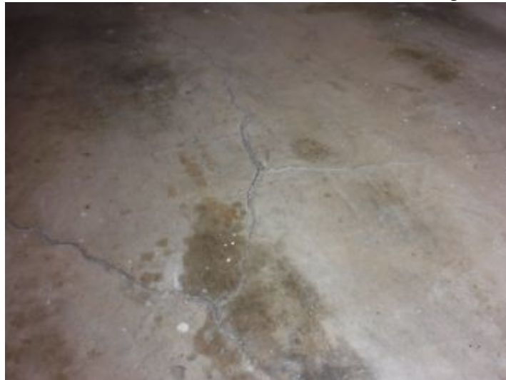
Garage Floor Condition
