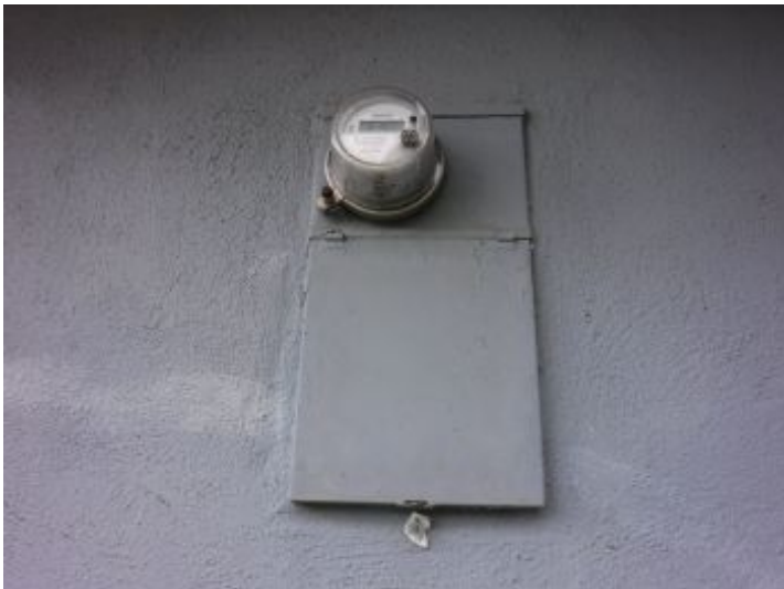
Electrical Electrical Panel
