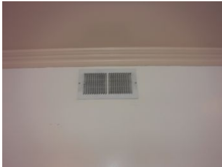
Heat/AC Heater/Ductwork Condition
