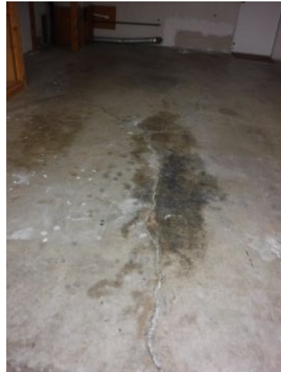
Garage Floor Condition
