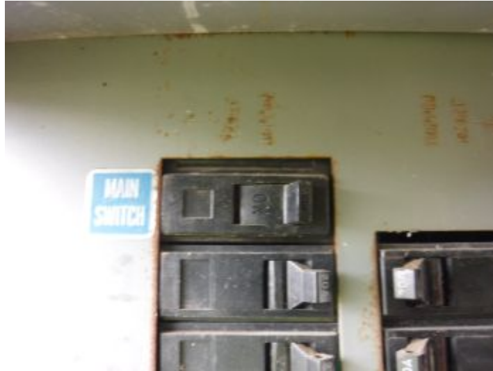
Electrical Main Amp Breaker
