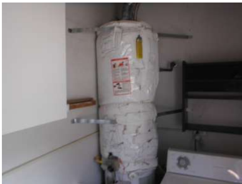
12. ● Water heater thermal blanket covers ID & safety placard.. ⑤ - See example at photo page)
