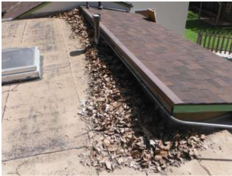
10. ● Debris covers portions of roof. Not fully visible. ⑨ See example at photo page)
