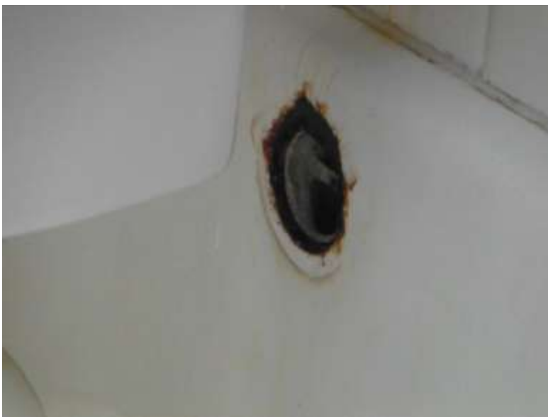
17. ● Tub overflow cover missing ④③: @ hall bathroom - See example at photo page)
