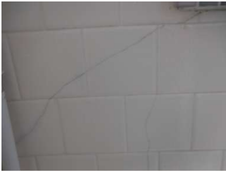
16. ● Cracked tiles found both sides of window ②⑦: in hall bathroom shower enclosure - See example at photo page)
