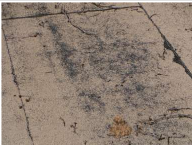
9. ● Roof is weathered and deteriorated. @@ garage & bonus room - See example at photo page) X 2
