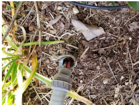
Recommend repairing elec. Conduit in garden area
