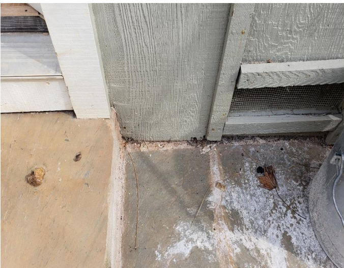
3A - Damaged siding and trim.
