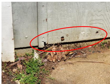
Dry rot on garage siding and trim
