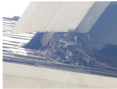
Upper gutter full of debris
