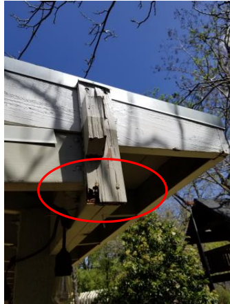
Dry rot at patio cover trim
