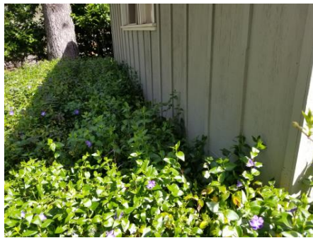
Recommend trimming vegetation
