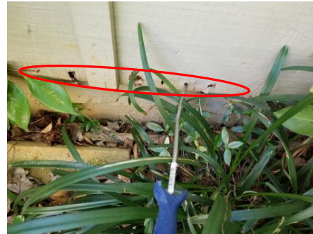
Dry rot at bottom of siding
