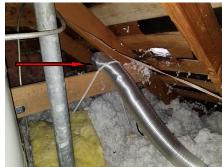
Vent pipe not directed outside
