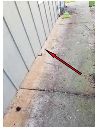
Siding too close to concrete
