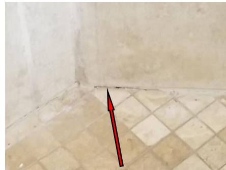
Shower tile needs re grouting in master bath
