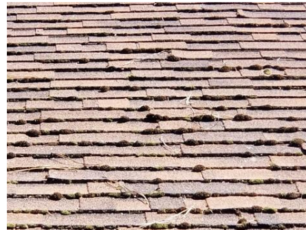
Moss build up on garage
