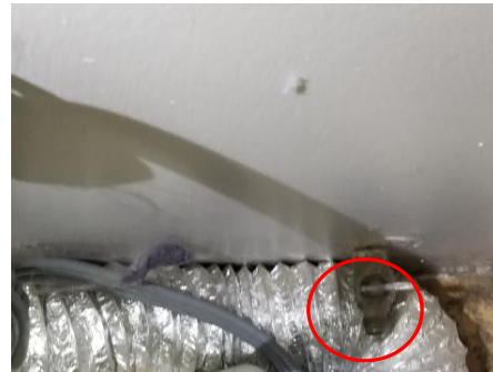
Safety Issue: Gas valve needs cap
