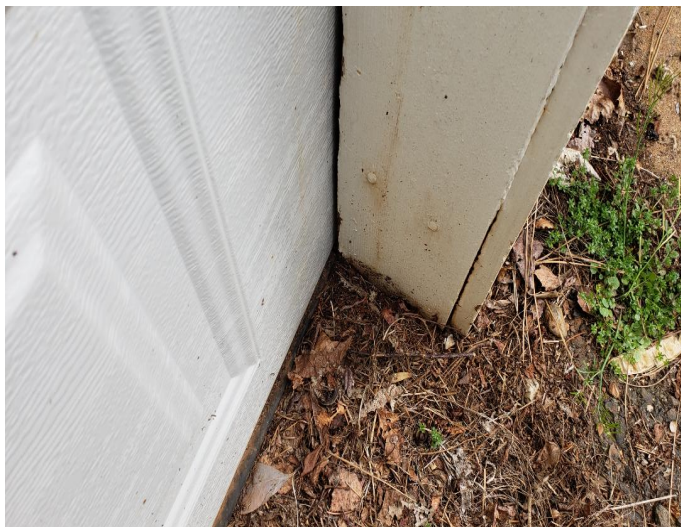
3D - Damaged garage door jambs.
