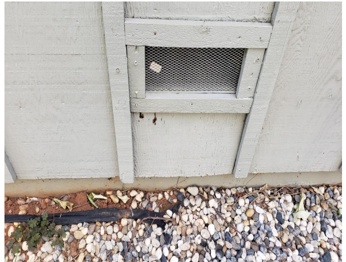
3A - Damaged siding.
