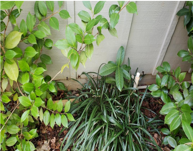
3A - Damaged siding and trim.
