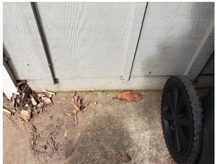
3A - Damaged siding and trim.
