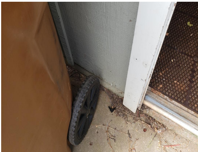
3A - Damaged siding.
