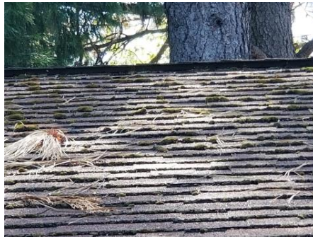
Moss build up on guest home roof
