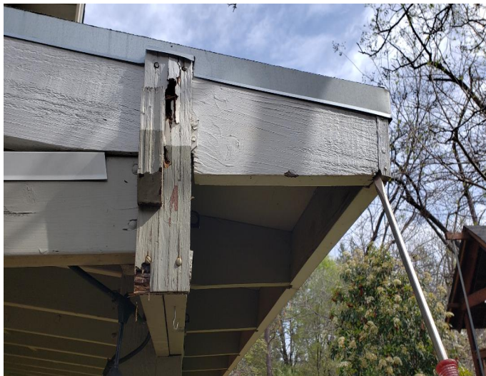
3B - Damaged patio joist and trim.
