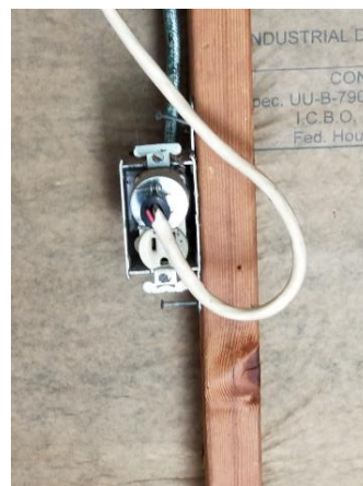
Missing outlet cover in garage
