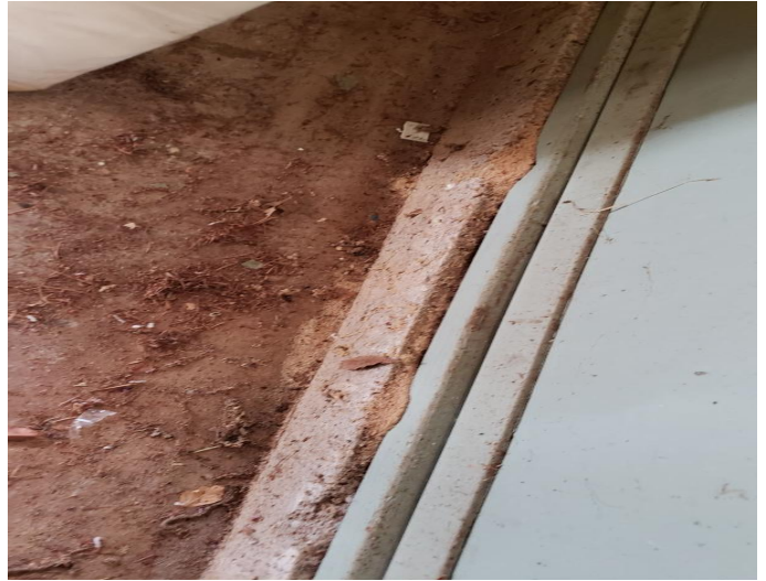
3E - Carpenter ants in the garage.
