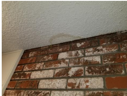
Ceiling stain upstairs in hall
