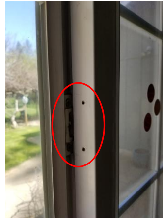
Window lock missing in guest home
