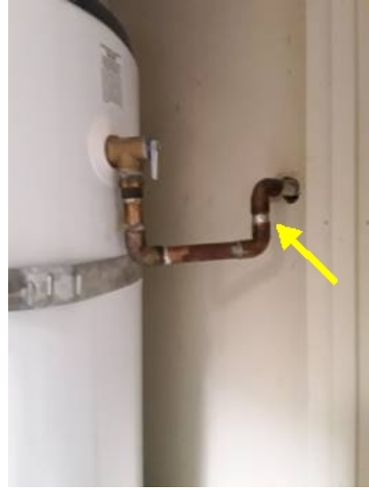
The discharge pipe from the pressure relief valve has been incorrectly plumbed uphill. This is not permissible and the discharge pipe should be correctly plumbed.
