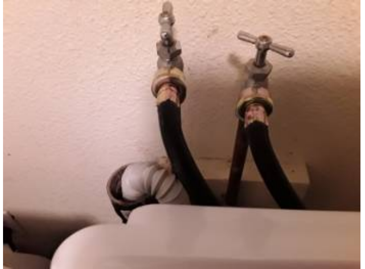
The water supply to washing machines is commonly left on, and over time, the rubber hoses that are commonly used to supply water can become stressed and burst. For this reason we recommend replacing all rubber supply hoses with metal-braided ones that are more resilient.
