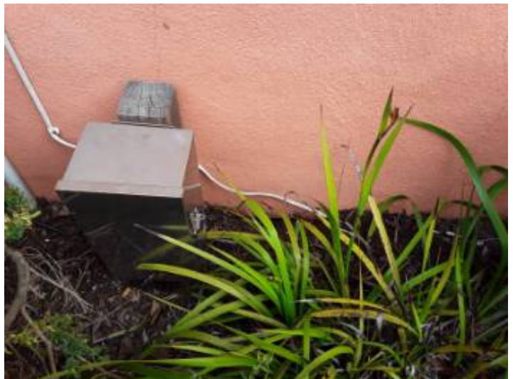
The soil is too high against the home at various areas around the home which should be serviced.
