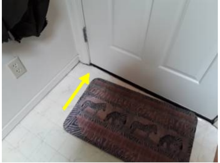
The floor is moisture damaged at the exterior doors and should be evaluated by a termite inspector.
