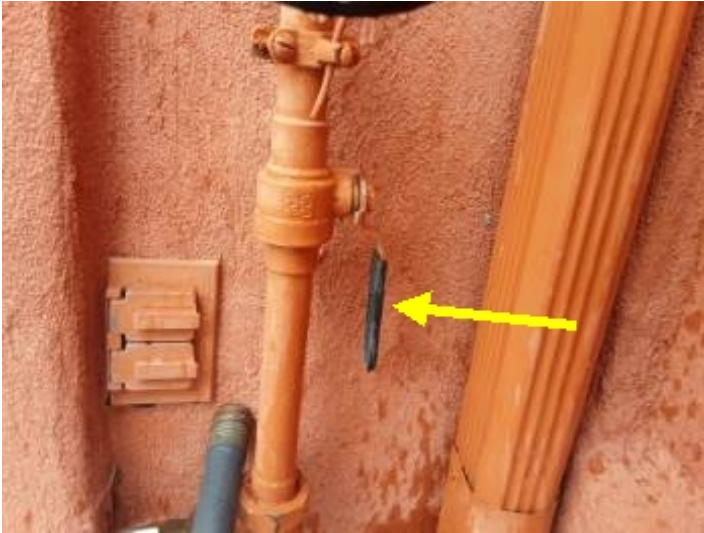
The main water shut-off valve is located at the left side of the house.
