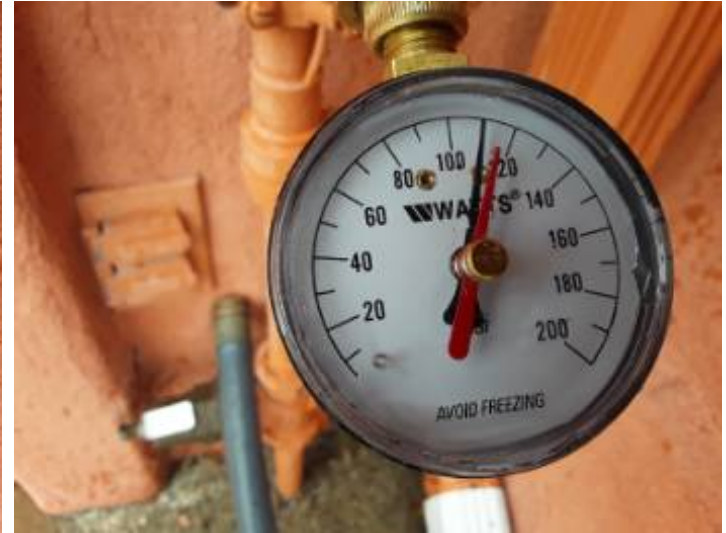
The pressure inside the residence is above 80 PSI and will stress components of the system. A licensed plumber should reduce the pressure at the regulator to sixty pounds per square inch, which is optimum. However, the regulator may have failed and would need to be replaced.
