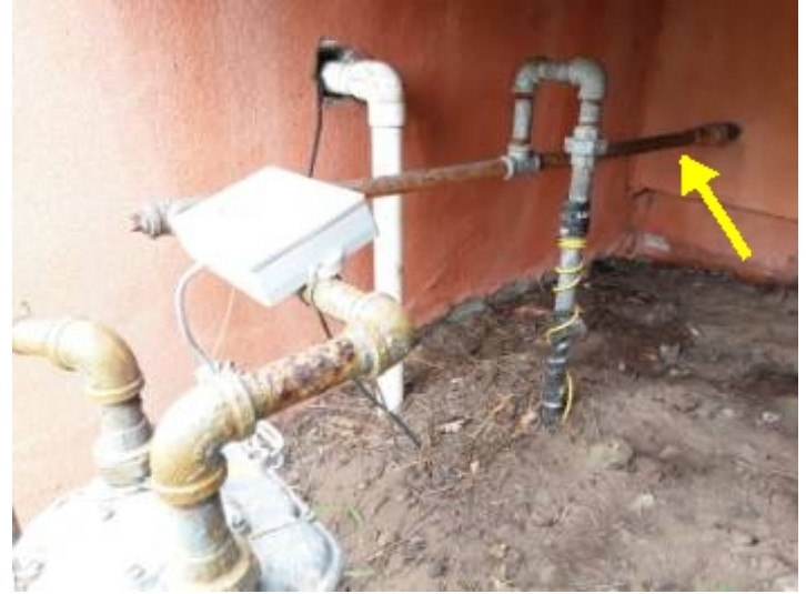
The gas lines at the meter are rusted and should be painted to prevent further corrosion.
