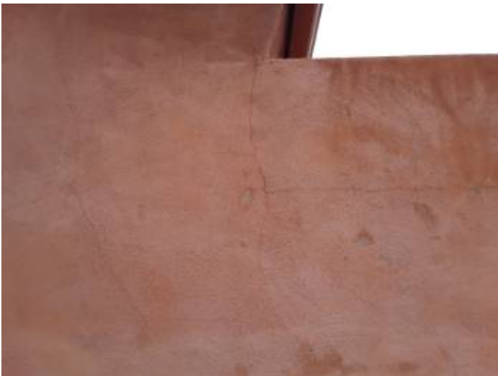
The spider-like cracks in the smooth stucco, or which is sometimes referred to as being a steel-trowel finish, are commonplace and not indicative of structural damage. However, you could have a specialist confirm this.
