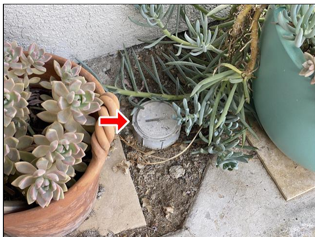
5.6 Item 1(Picture) Plumbing System
