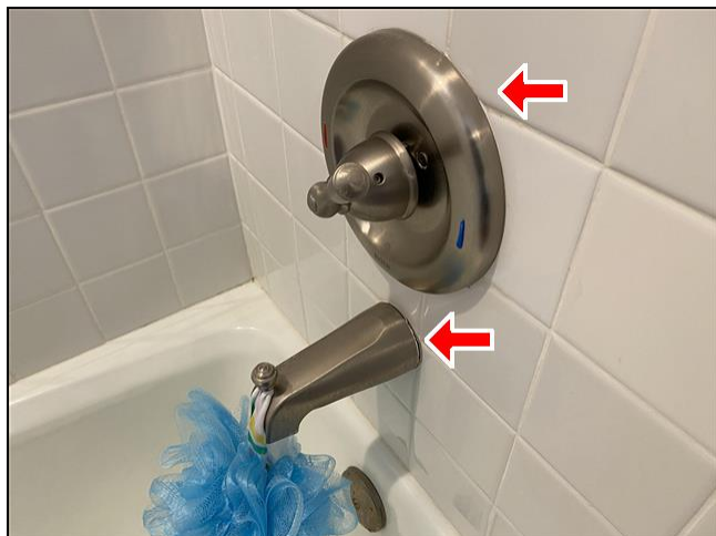
5.1 Item 1(Picture) Plumbing System
