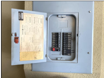
6.5 Item 1(Picture) Electrical System
