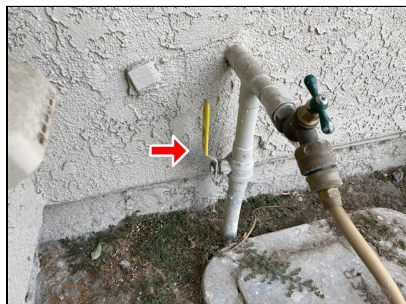
5.4 Item 1(Picture) Plumbing System
