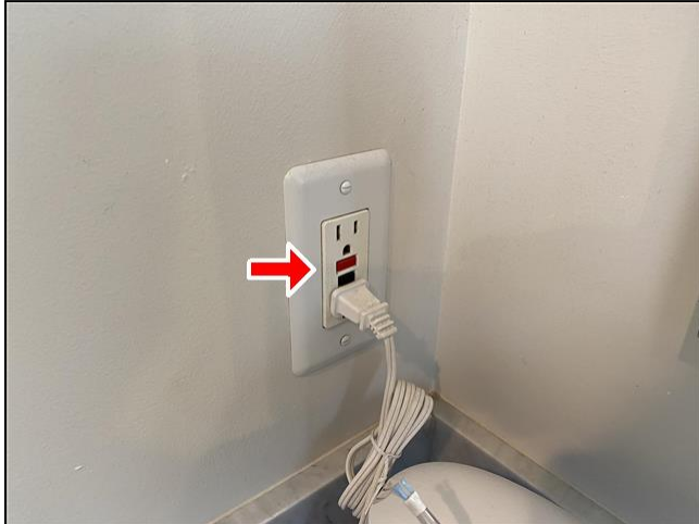
6.2 Item 1(Picture) Electrical System
