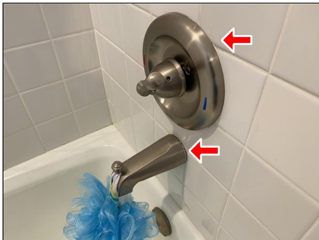
Item 7 - Item 1(Picture) Plumbing System
