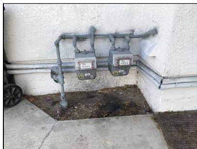
5.5 Item 1(Picture) Plumbing System
