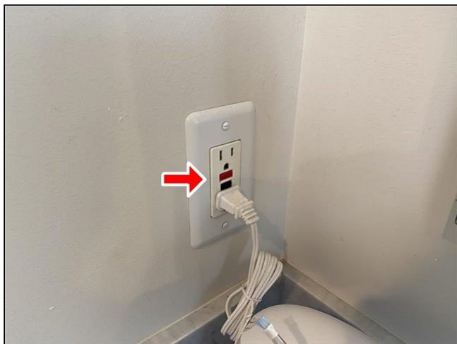
Item 8 - Item 1(Picture) Electrical System
