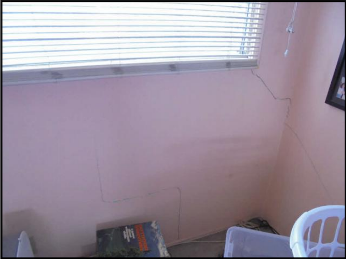
Interior settlement cracks
