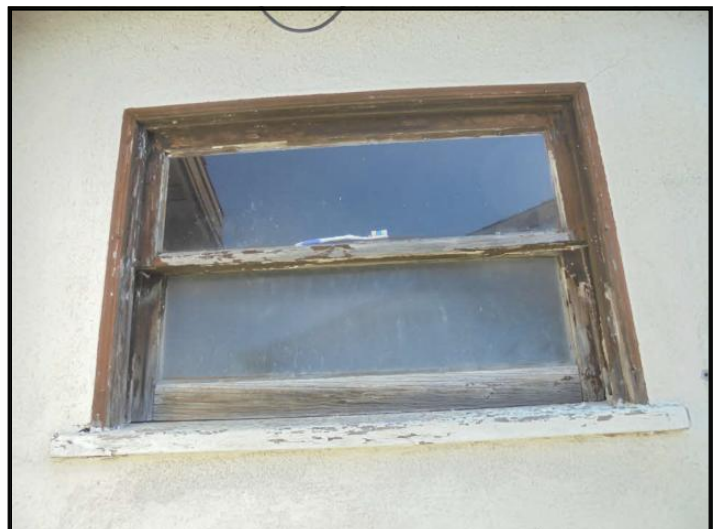
Peeling paint on exterior window trim
