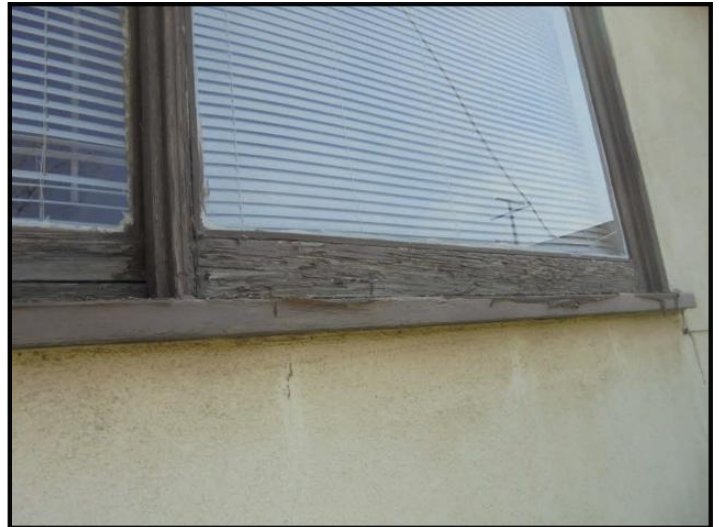
Peeling paint on exterior window trim
