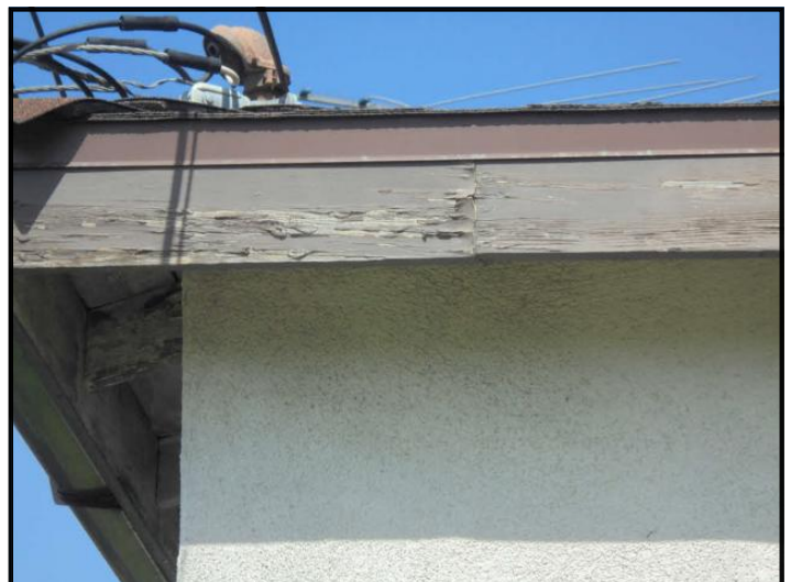
Peeling paint on exterior eaves
