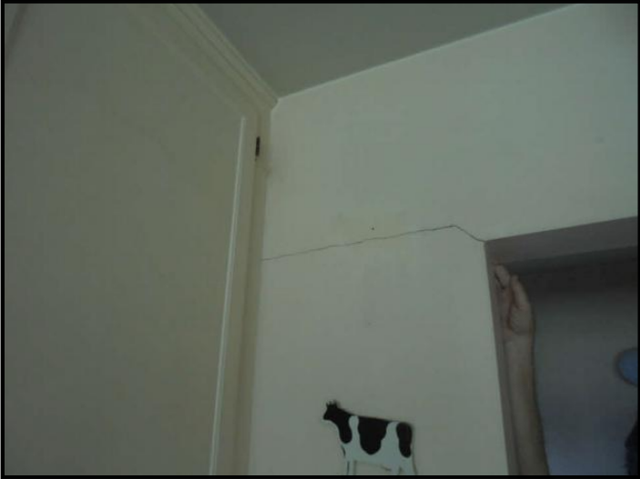
Interior settlement cracks
