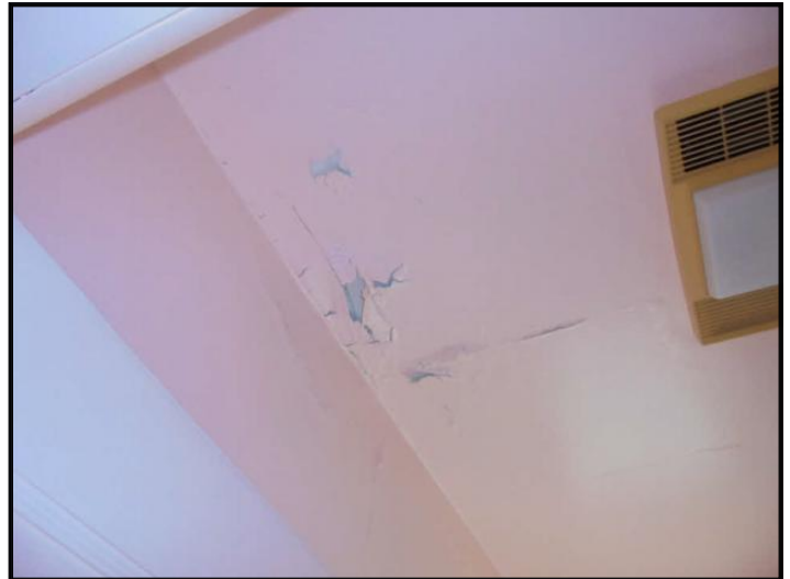
Peeling paint on interior walls
