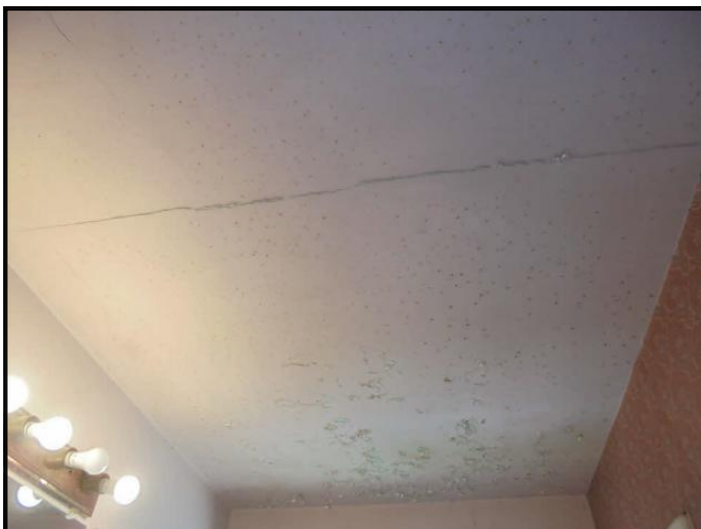
Peeling paint on bathroom ceiling
