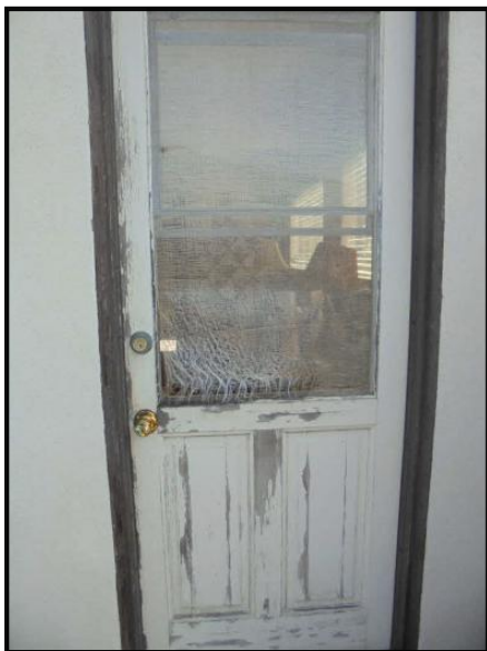
Peeling paint on exterior door
