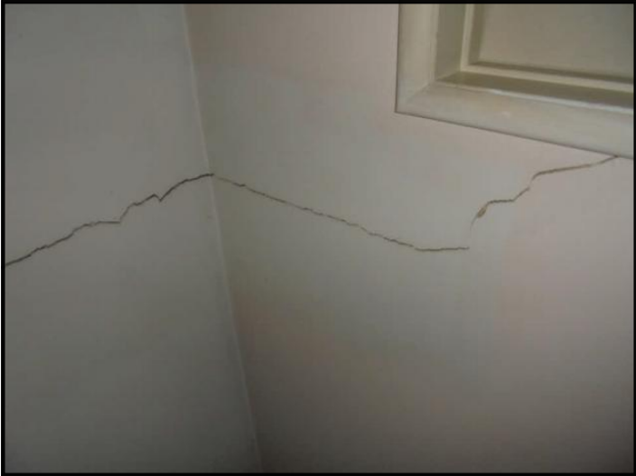
Interior settlement cracks
