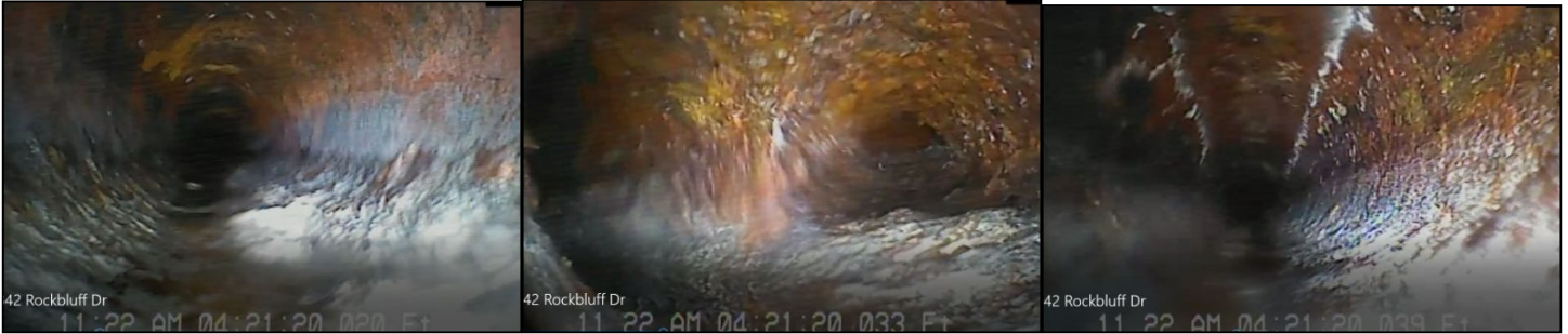
Condition of sewer line at 20 feet. Condition of sewer line at 33 feet. Condition of sewer line at 39 feet.
