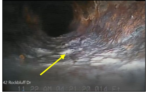
Sewage present at 14 feet.
