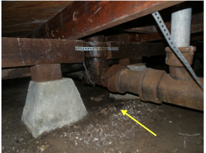
There is a leak beneath the hallway bathroom which should be repaired
