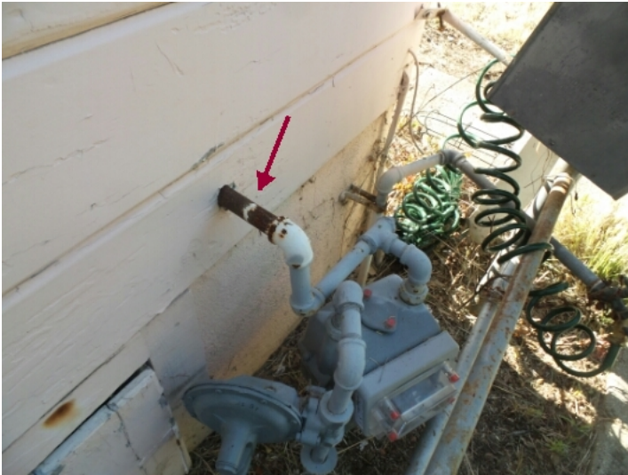
Some of the gas lines at the meter are rusted and should be painted to prevent further corrosion.
