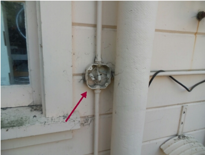
There is one or more open junction boxes that should be sealed.
