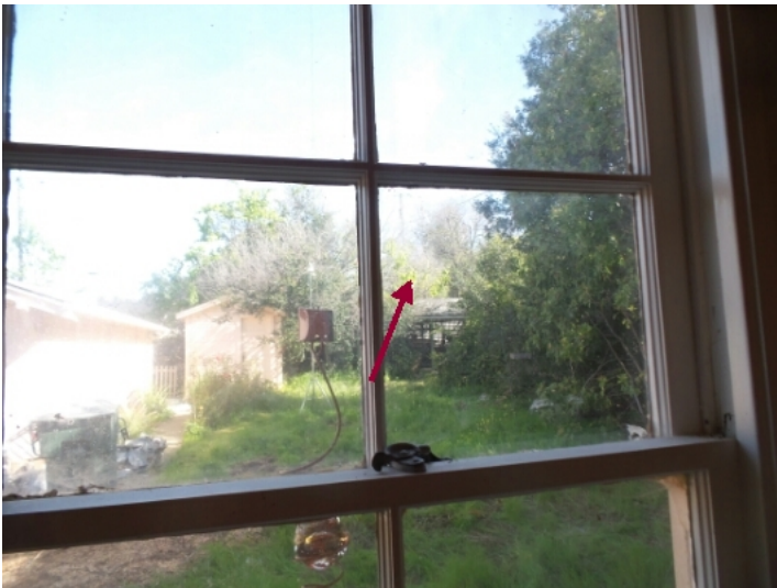
A window pane is cracked or broken and should be replaced.
