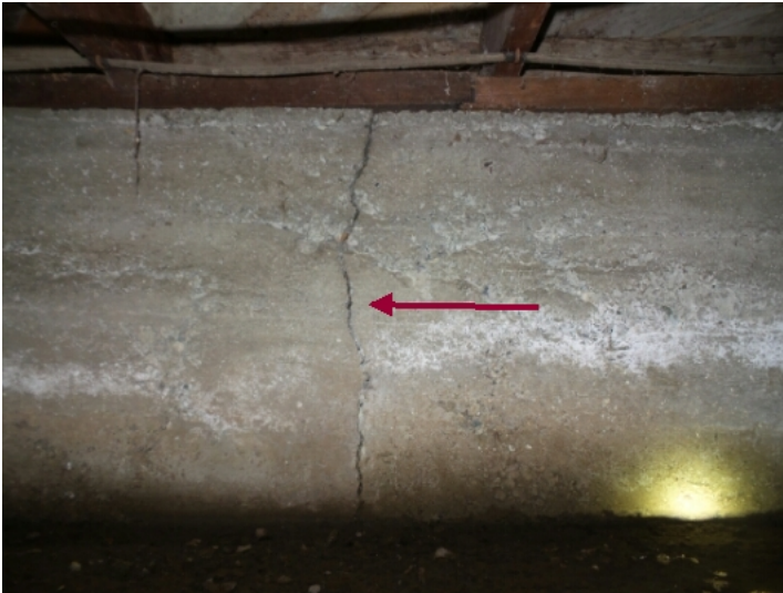
There are atypical cracks in the foundation walls that should be evaluated by a specialist.
