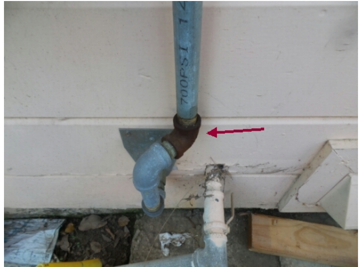
Rusted gas lines
