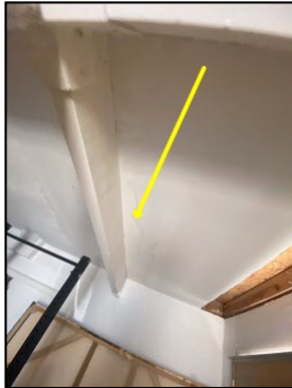
Stains present - tested dry at time of inspection - monitor for possible moisture intrusion
