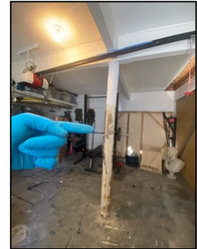
Ceiling support Beam seems to be deteriorating needs to be serviced and further evaluated by a licensed contractor
