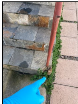
Damaged steps - unsafe - needs to be serviced
