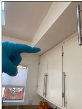
Loose cabinet - needs to be serviced - potential detach and fall hazard
