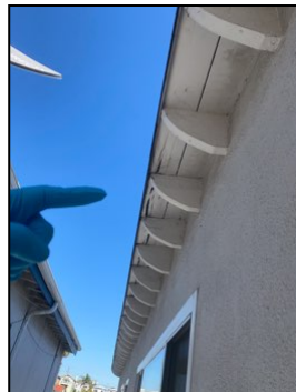
Deteriorated in areas - needs to be serviced - consult the termite report
