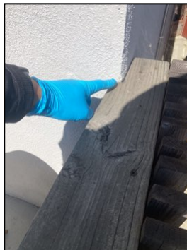
Railing not properly fastened - safety hazard - needs to be serviced
