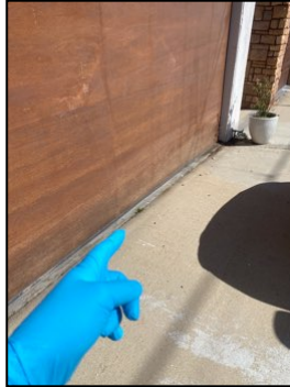
Driveway slopes towards garage - potential for water intrusion - needs to be serviced
