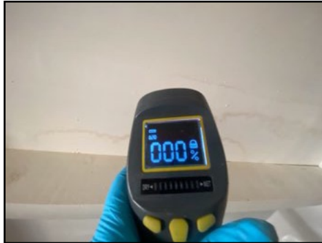
Stains present - tested dry at time of inspection - monitor for possible moisture intrusion
