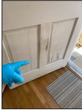
Moisture damage- needs to be serviced
