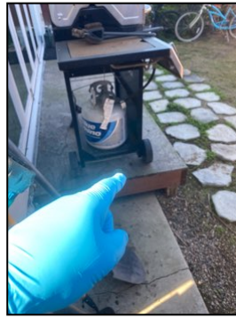
Irregular installation/patching/workmanship - needs to be serviced
