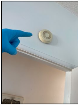
Did not operate - needs to be serviced or replaced
