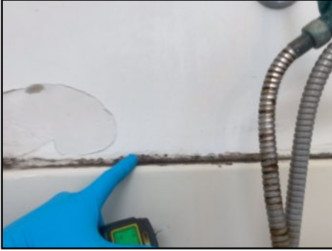
Microbial growth/irregular staining present - further evaluation is recommended
