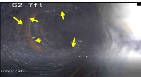
Offset & root intrusion present at 62.7 feet
