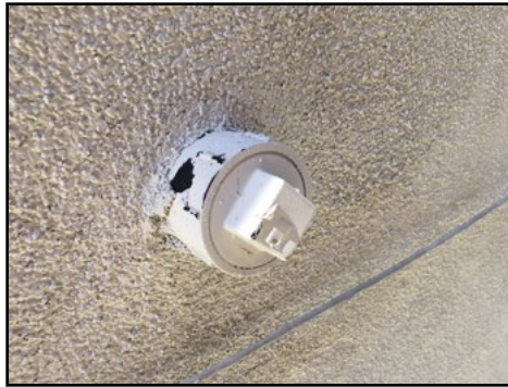
Clean out used for inspection
