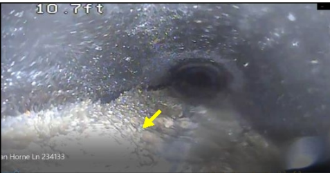
Sewer line sludge observed at 10.7 feet
