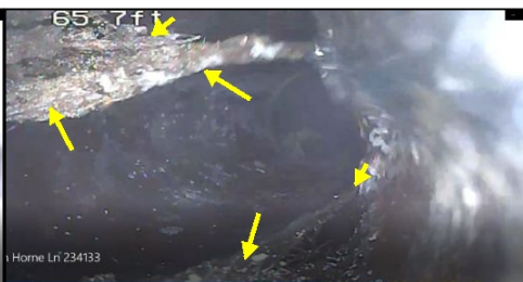
Root intrusion present at 65.7 feet
