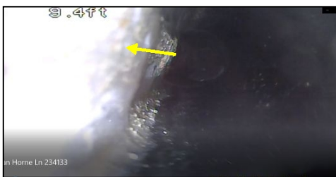
Sewer line sludge observed at 9.4 feet
