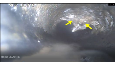
Sewer line sludge build up present at 42.0 feet
