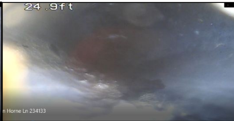
Condition of sewer line at 24.9 feet
