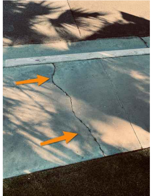
This moderate crack was at the city street and may be maintained by the city.
