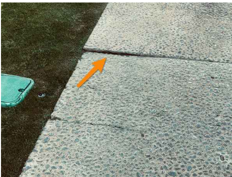
Where is approximately 1/2 inch, potential trip hazard.
