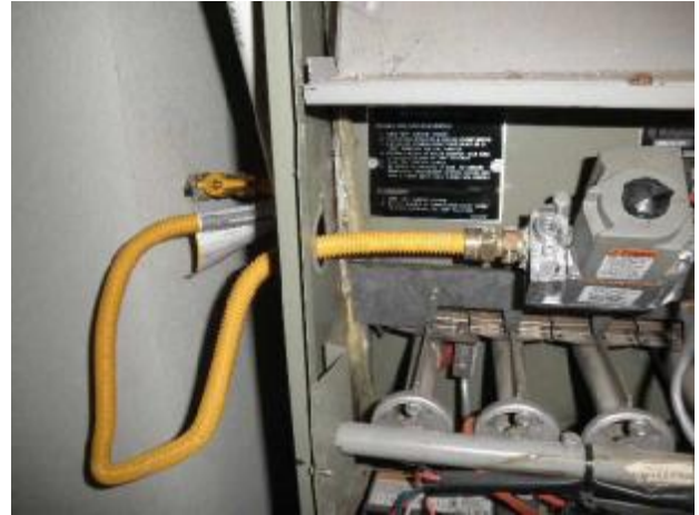
Flexible gas line penetrates the housing at the furnace.
