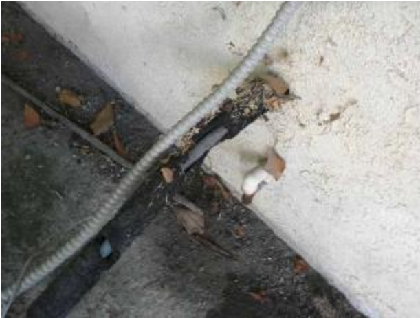
Damage to the insulation at the low pressure refrigerant lines.
