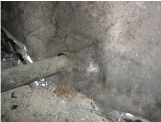
Caulking needed at the gas starter pipe inside the firebox.
