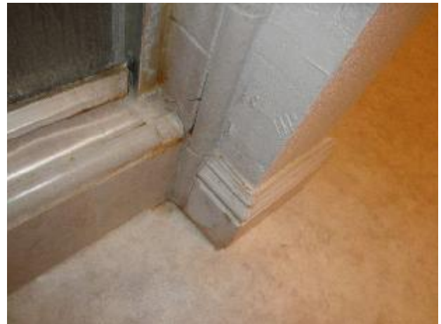
Evidence of leaks at both sides of the shower door in the hall bathroom.
