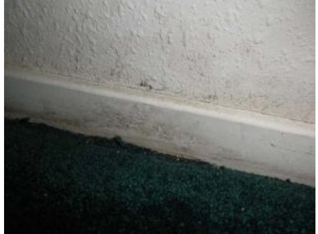
Black mildew like substance at the base of the wall in the SE bedroom closet.
