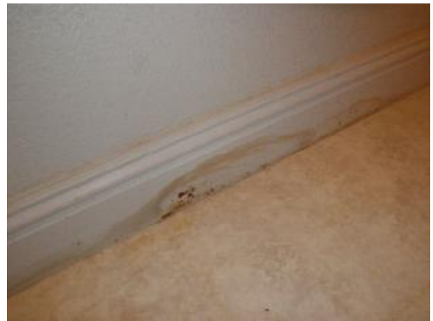
Water stain at the base of the hall bathroom wall behind the shower.
