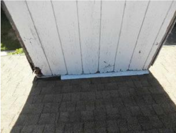
No cricket flashing behind the chimney enclosure.
