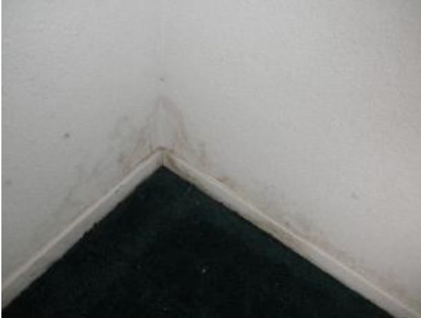
Water stain at the base of the wall in the SE bedroom closet.
