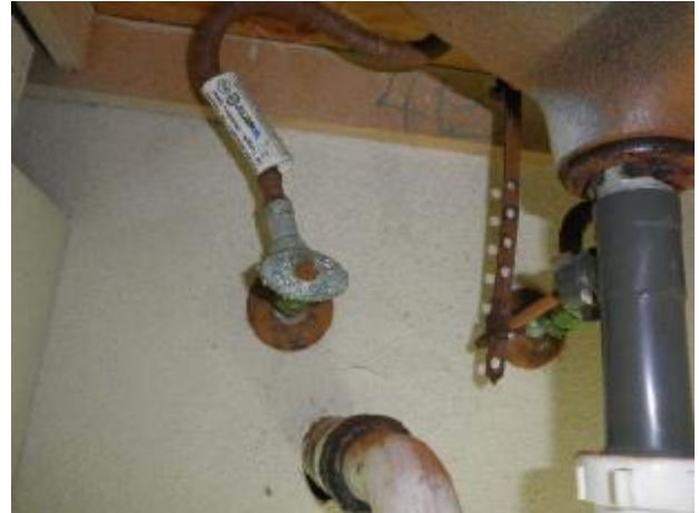
Rust damage to the angle stop valves and drain line connection at the hall bathroom sink.
