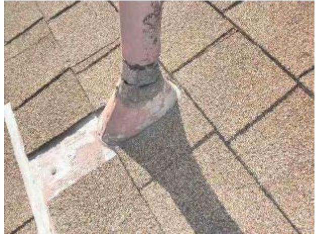
The flashings need to be resealed.
