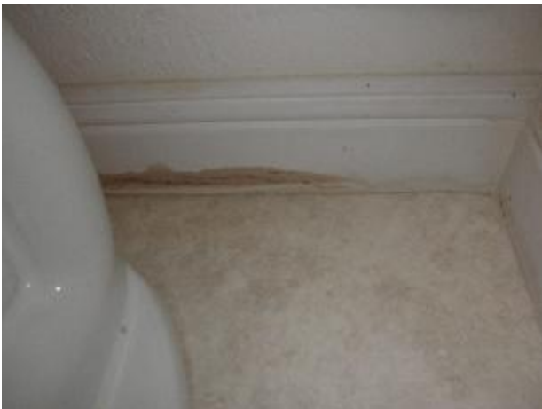
Water stain at the baseboard behind the toilet.
