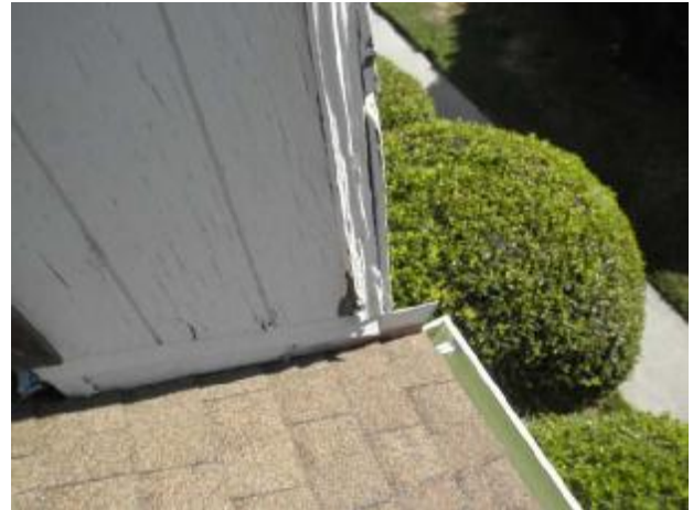
Moisture damage to the wood siding and trim at the chimney enclosure.
