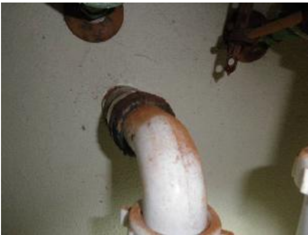
Rust damage to the angle stop valves and drain line connection at the hall bathroom sink.
