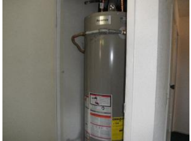
Improper straps at the water heater.
