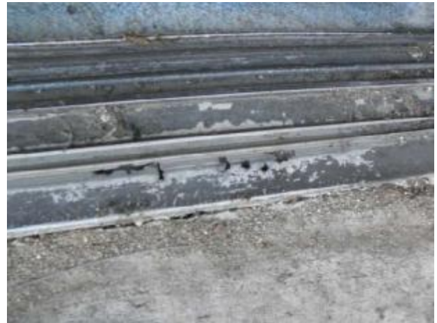
Damage/holes to the metal track for the sliding glass door.
