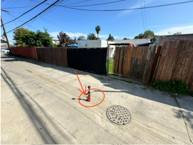
Connection to city sewer under tool.
