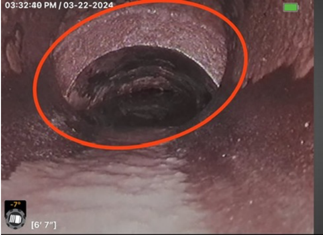
Location of offset/shifted clay pipe 3.2' deep.
