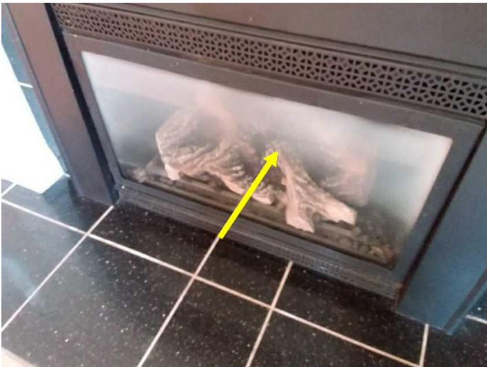
The fireplace glass is functional, however does not have a protective screen, which is required by current standards and should be installed for optimal safety.
