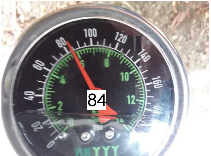
The pressure inside the residence exceeds 80psi, which is too strong and will stress components of the system, and a regulator should be installed. Most regulators come factory pre-set at 60psi.
