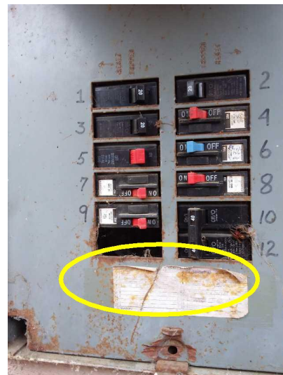
Various circuits are not labeled or legible, which is recommended.
