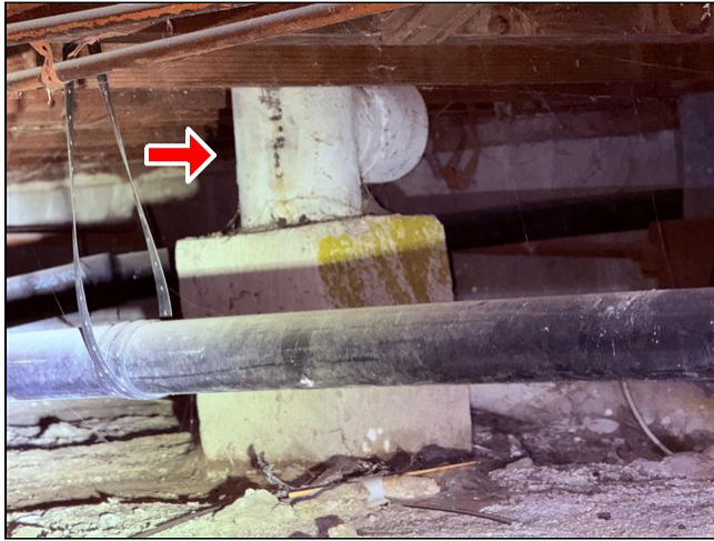
4.3 Item 1 (Picture) Heating/Central Air
