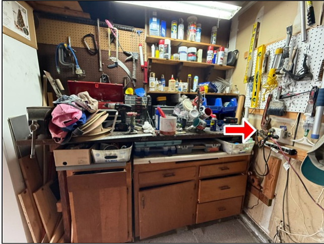
Item 17 - Item 1 (Picture) Electrical System
