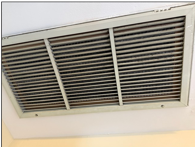
4.5 Item 1 (Picture) Heating/Central Air
