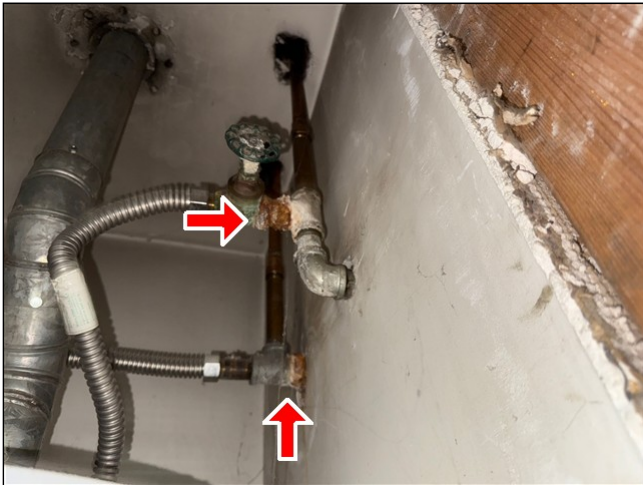
Item 6 - Item 1 (Picture) Plumbing System
