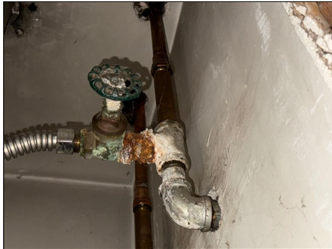
Item 6 - Item 2 (Picture) Plumbing System
