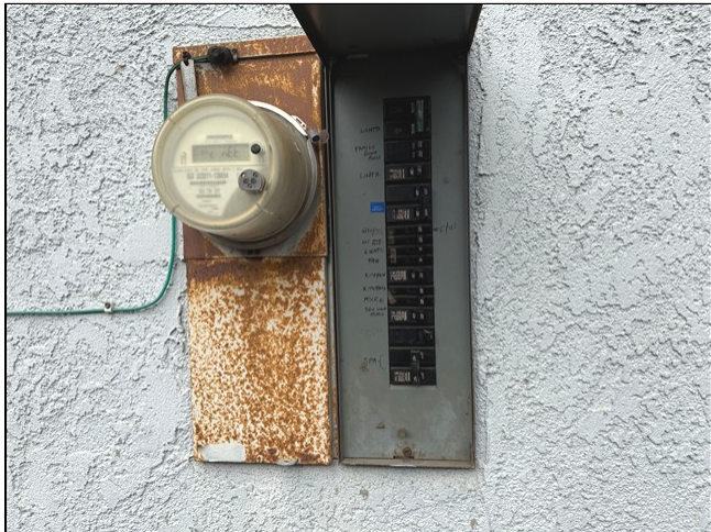
6.0 Item 1 (Picture) Electrical System
