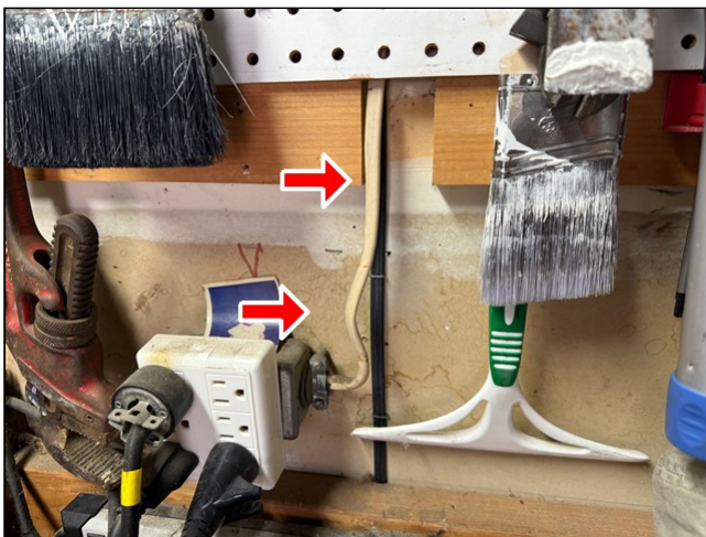
Item 14 - Item 1 (Picture) Electrical System
