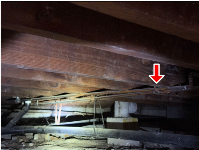
Item 8 - Item 1 (Picture) Plumbing System
