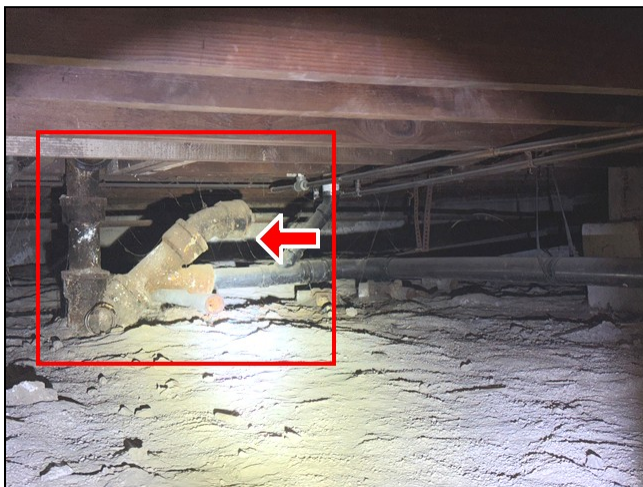
5.0 Item 2 (Picture) Plumbing System
