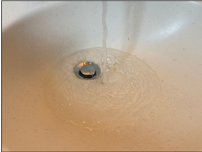
5.1 Item 3 (Picture) Plumbing System
