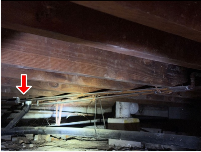
Item 9 - Item 1 (Picture) Plumbing System
