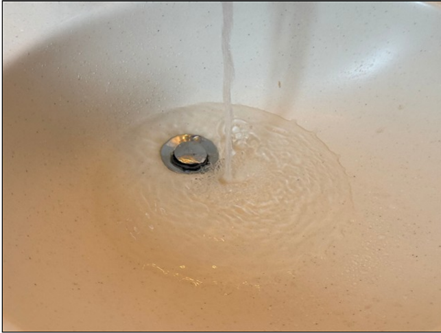
Item 7 - Item 1 (Picture) Plumbing System
