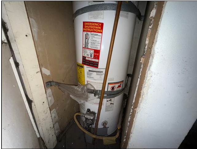
5.2 Item 2 (Picture) Plumbing System
