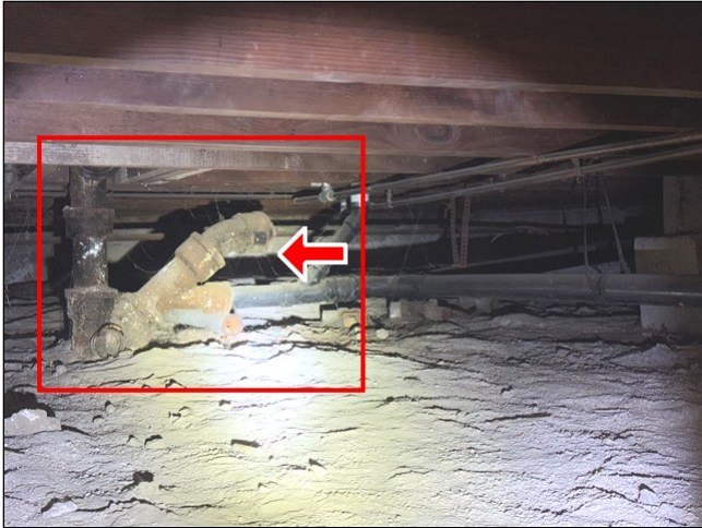
Item 5 - Item 1 (Picture) Plumbing System
