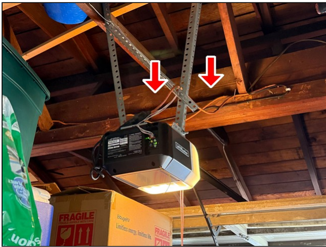
Item 15 - Item 1 (Picture) Electrical System
