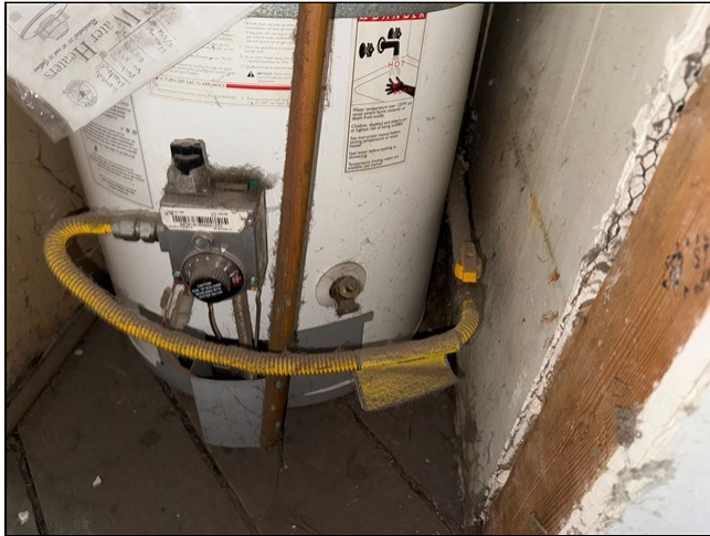
5.4 Item 1 (Picture) Plumbing System
