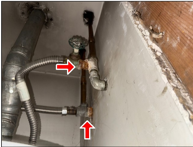
5.1 Item 1 (Picture) Plumbing System
