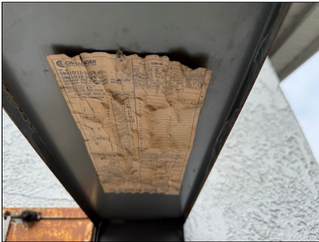
Item 13 - Item 3 (Picture) Electrical System
