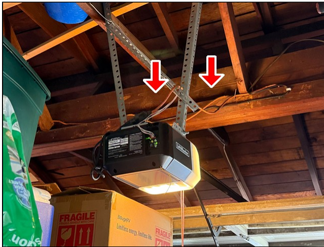
6.1 Item 3 (Picture) Electrical System
