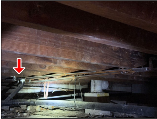
5.1 Item 5 (Picture) Plumbing System
