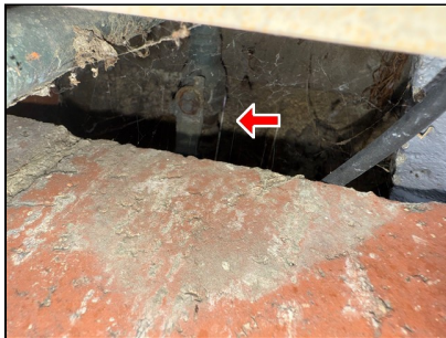
5.6 Item 1 (Picture) Plumbing System
