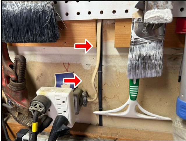
6.1 Item 1 (Picture) Electrical System
