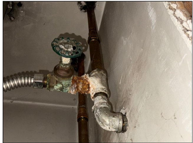
5.1 Item 2 (Picture) Plumbing System
