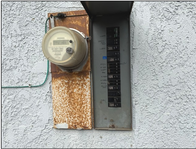
Item 13 - Item 1 (Picture) Electrical System
