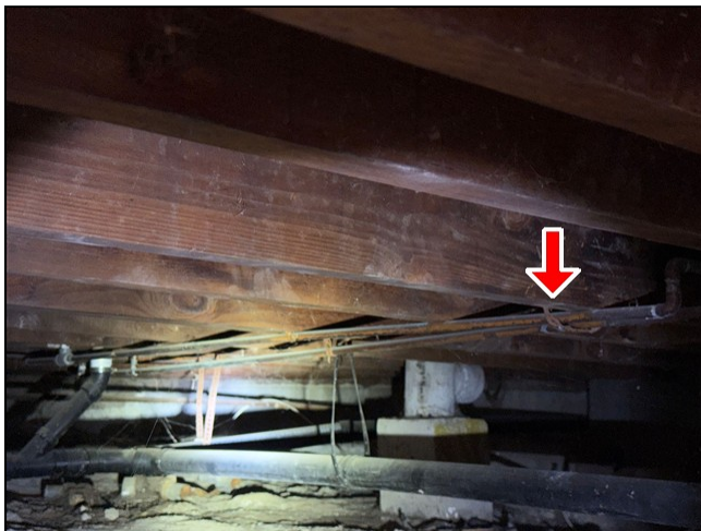
5.1 Item 4 (Picture) Plumbing System
