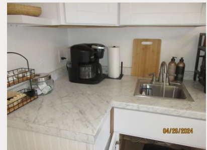
Missing at bar sink
