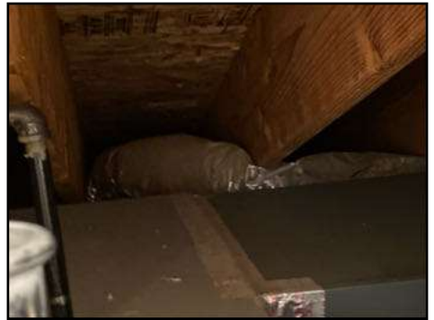
Compressed/squashed ductwork - needs to be serviced
