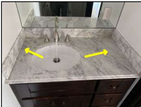
Gap at back splash to counter top joint - needs to be sealed to prevent unwanted moisture entering the cabinet
