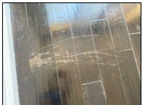
Worn/stained heavily in areas - recommend servicing
