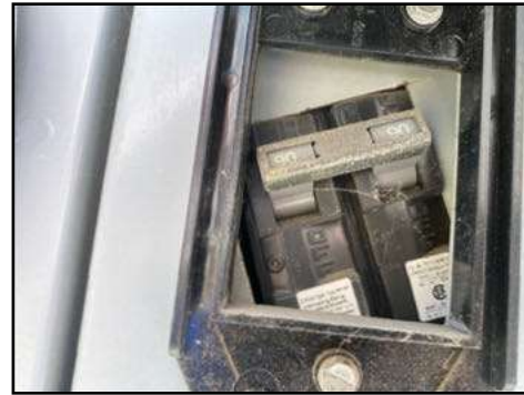
90 amp - this is considered to be low capacity by today's standards - recommend upgrading service
