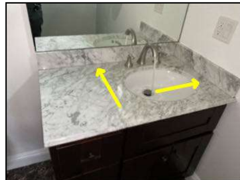
Gap at back splash to counter top joint - needs to be sealed to prevent unwanted moisture entering the cabinet
