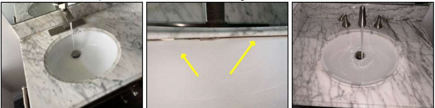
Gaps/deteriorated sealant present between sink and counter top - potential for leakage - recommend sealant maintenance to prevent unwanted moisture entering the cabinet
