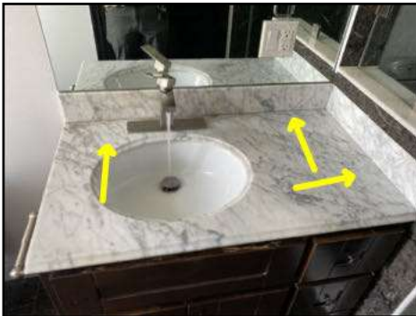
Gap at back splash to counter top joint - needs to be sealed to prevent unwanted moisture entering the cabinet
