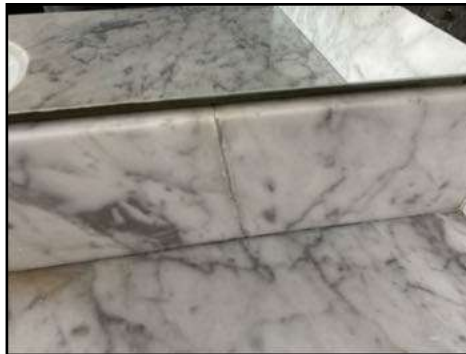
Cracked materials - recommend servicing
