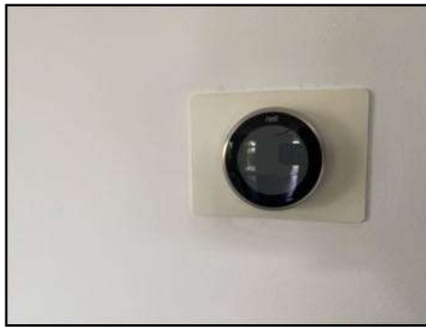
Not operating - needs to be serviced
