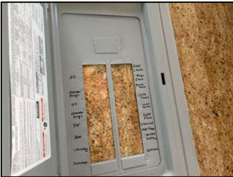
Labels are present on panel cover - the inspector does not confirm accuracy of labels
