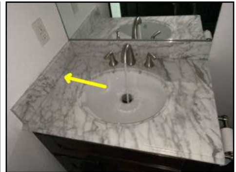
Gap at back splash to counter top joint - needs to be sealed to prevent unwanted moisture entering the cabinet
