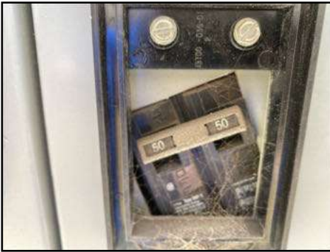
50 amp - this is considered to be low capacity by today's standards - recommend upgrading service
