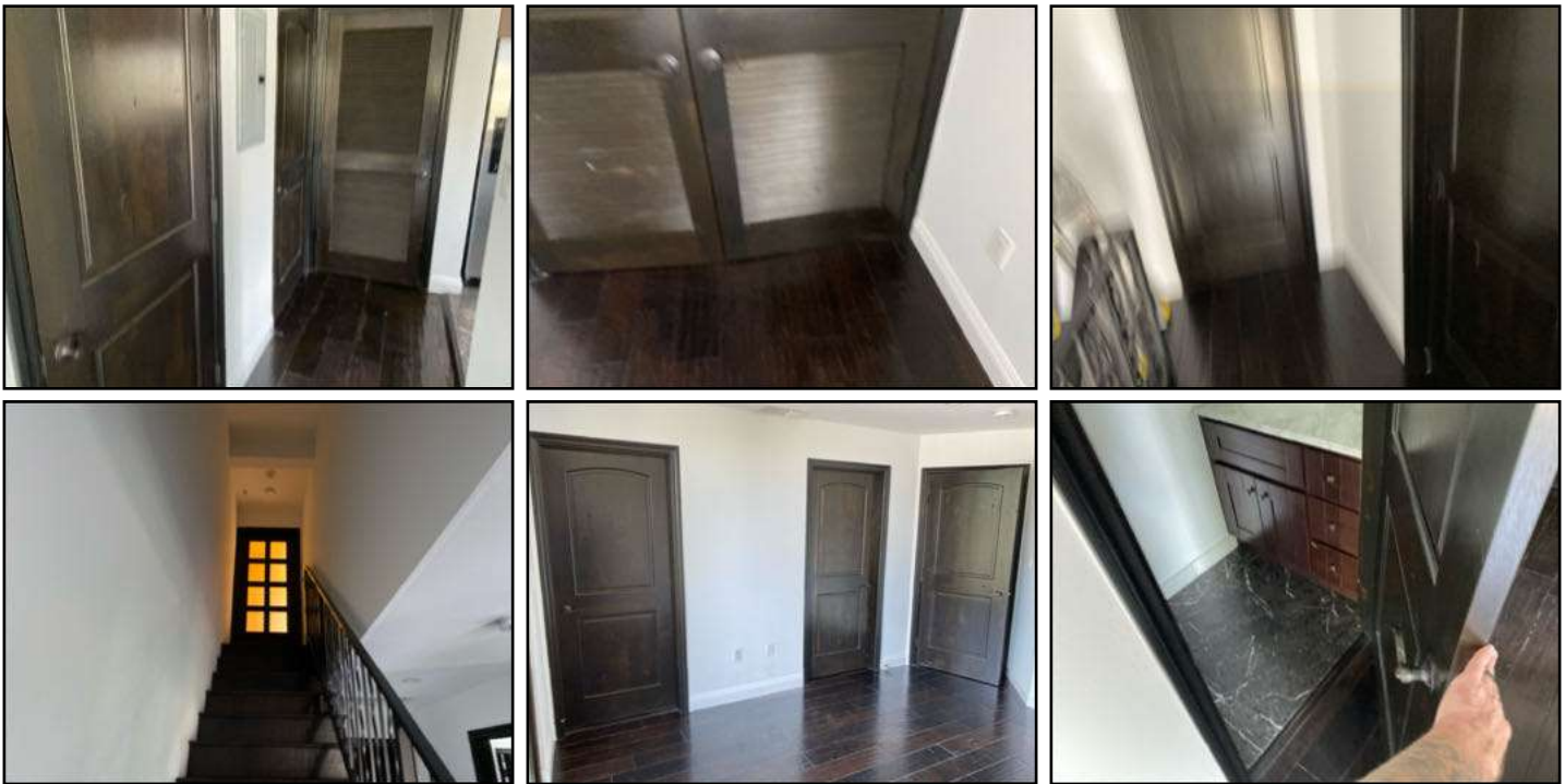
Door opens into hallway - may be problematic during emergency egress situation
