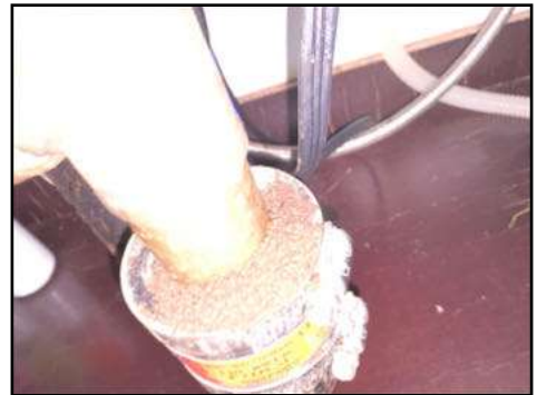
Corrosion is present at plumbing areas - this is a sign of slow leaking and should be further evaluated by a plumber
