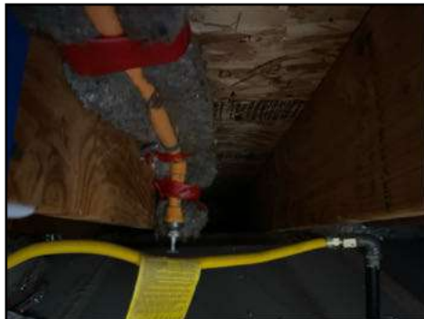
Fire sprinkler piping present and is beyond the scope of this inspection - not inspected/evaluated
