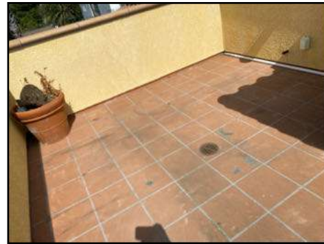
Stained and worn - will likely require re-waterproofing in the near future
