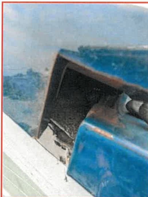
Popped Slid Rake Tile Exposing Capsheet Underlayment And Wood Rot Plywood
