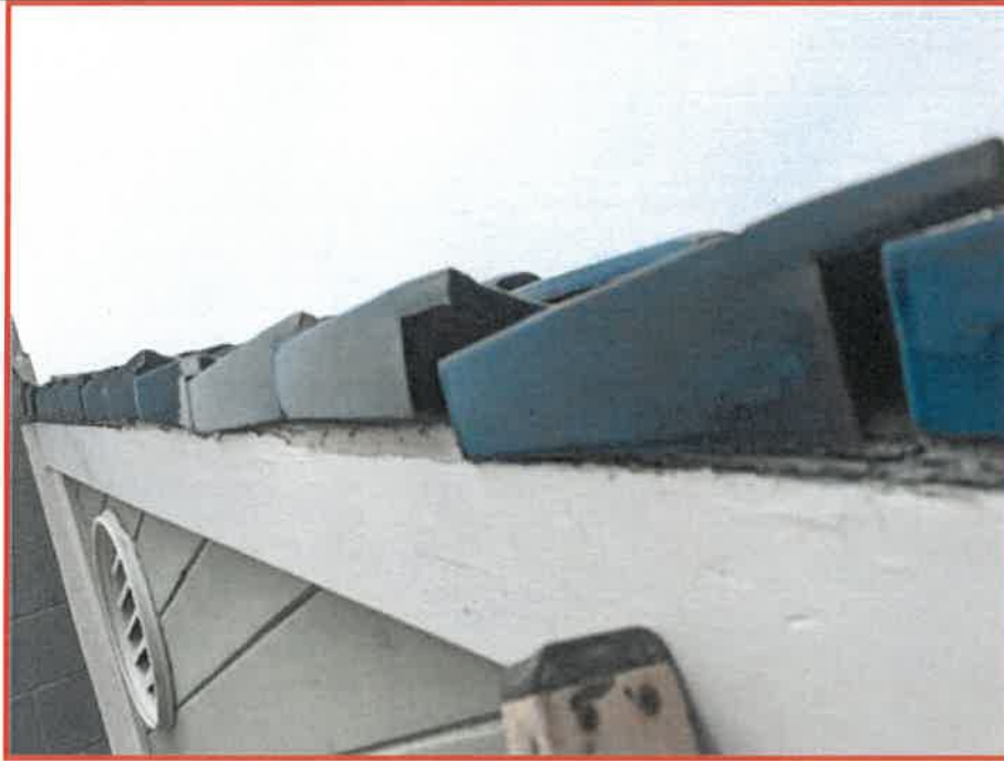
Slid Rake Tiles And Wood Rot At Fascia Board
