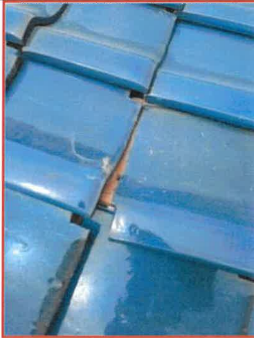
Slid Tile With Missing Nail
