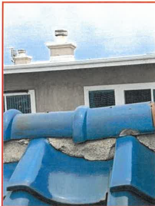
Popped Nails On Ridge Cap Tiles
