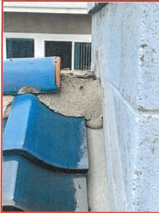
Missing Ridge Cap Tile
