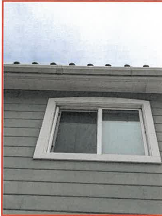
Wood Rot Shiplap And Fascia Board
