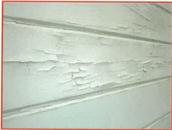
Example of Deteriorating Wood Siding
