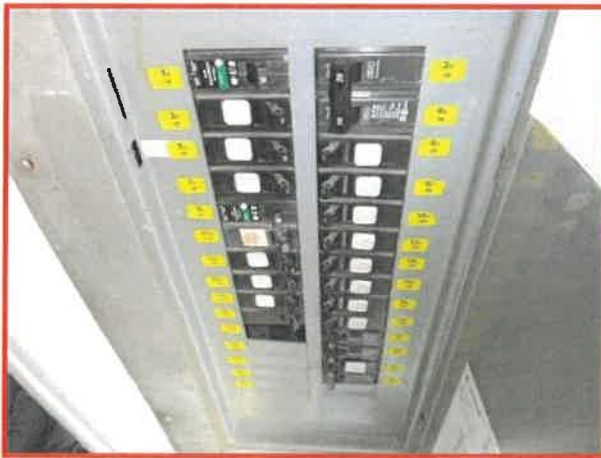
Sub Panel with Open Knockout
