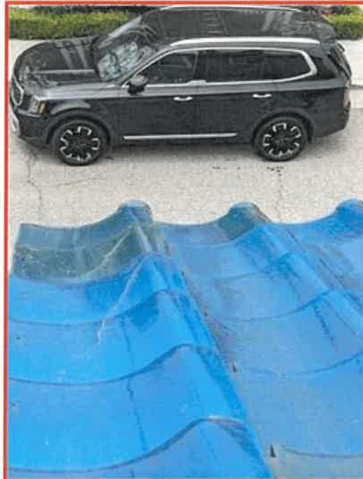
Shifted And Cracked Tile
