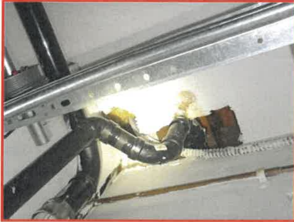
Breach in Fire Barrier in Garage
