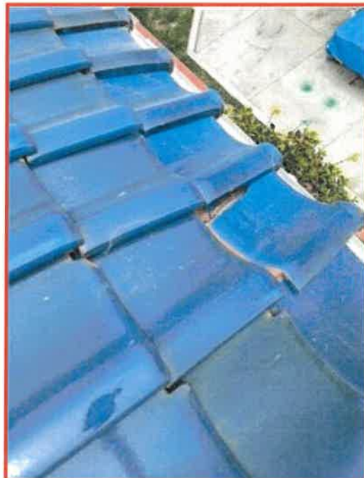
Broken / Slid Tile
