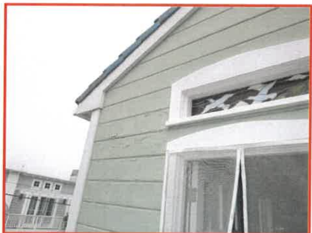
Example of Deteriorating Wood Siding
