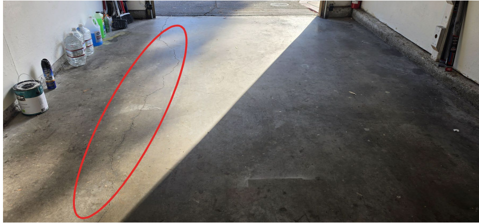
Red outline marks the hairline crack in the garage slab.
