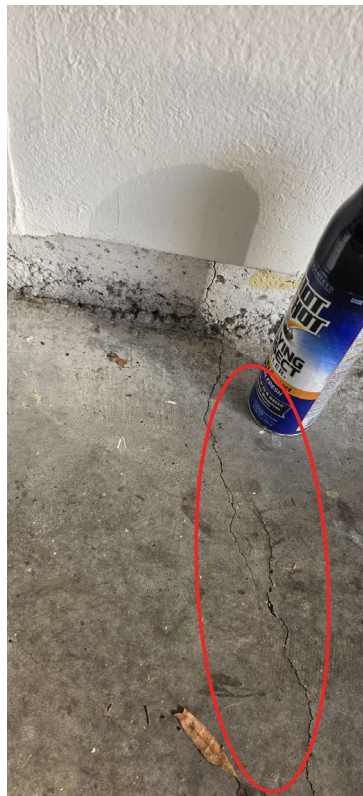
Red outline marks the hairline crack extending from the base of the garage side wall.
