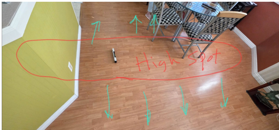
Red outline marks the raised high spot in the dining area floor; teal arrows indicate the direction of floor slope away from the high spot.
