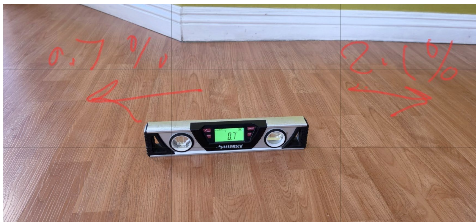
Digital level readings of approximately 0.7% on one side of the high spot and 2.1% on the opposite side; red arrows indicate the direction of slope.
