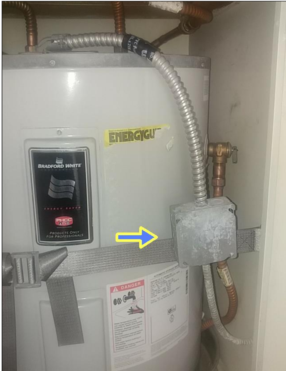
1.2 Item 3(Picture) Electrical connection should be serviced.
