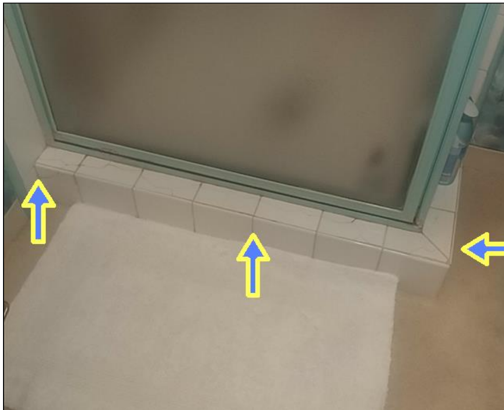
8.1.A Item 1(Picture) The shower stall floor tiles are cracked in several areas and should be serviced.
