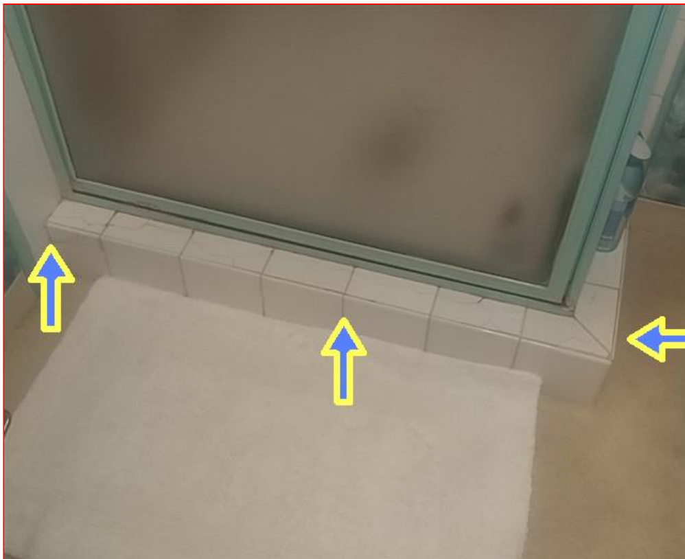
8.1.A Item 1(Picture) The shower stall floor tiles are cracked in several areas and should be serviced.
