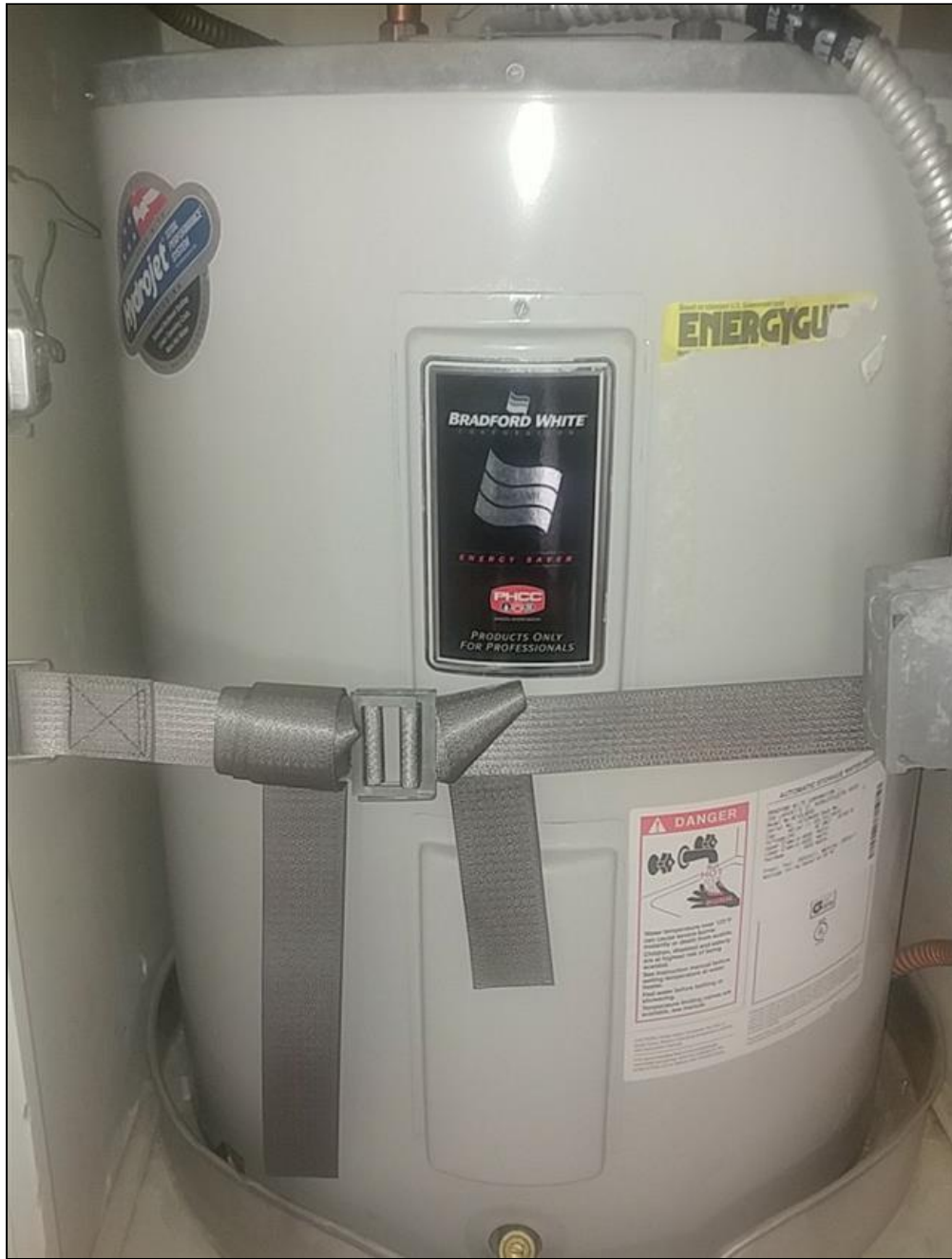
1.2 Item 2(Picture) Water heater is not properly strapped and should be serviced.
