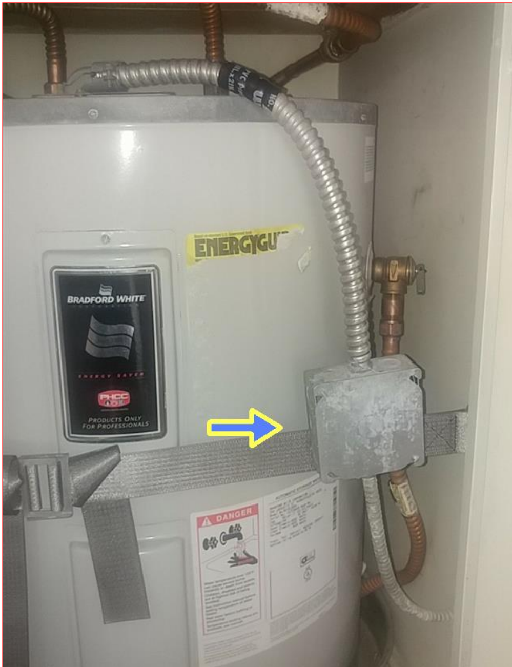
1.2 Item 3(Picture) Electrical connection should be serviced.
