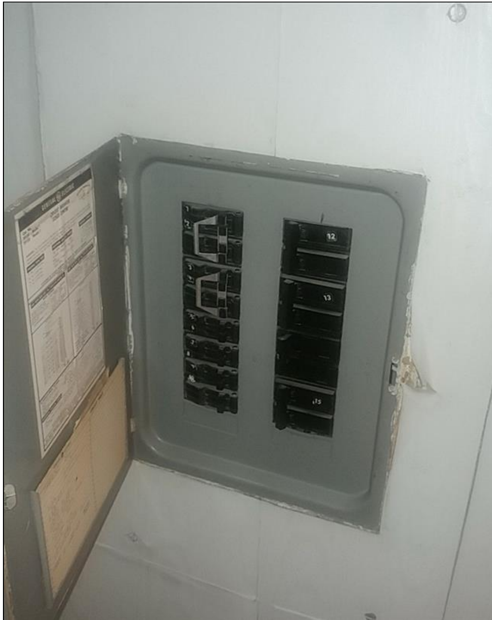
2.2 Item 1(Picture) Sub-Panel in the hallway.
