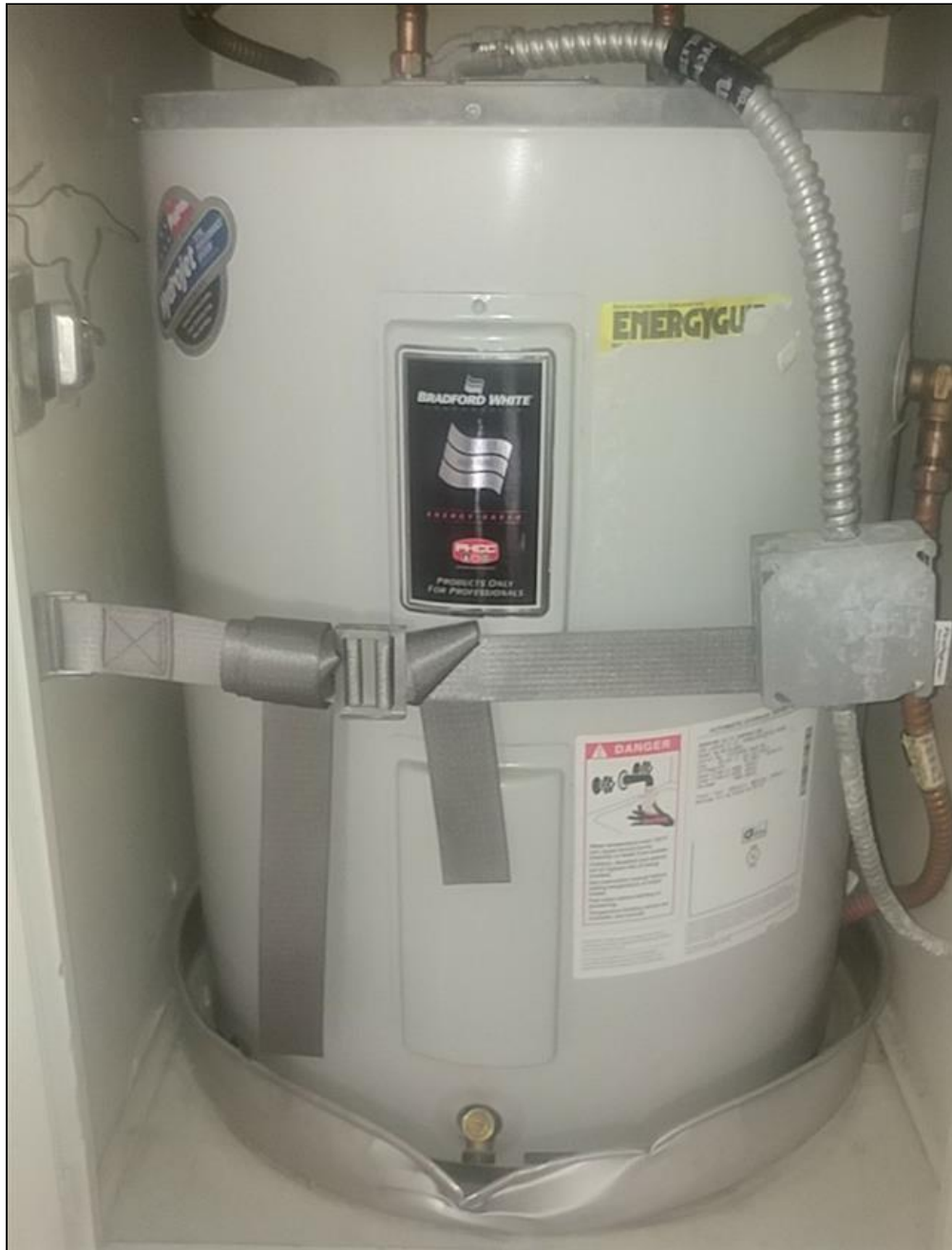
1.2 Item 1(Picture) Water Heater in the hallway is C years old and 40 gallons
