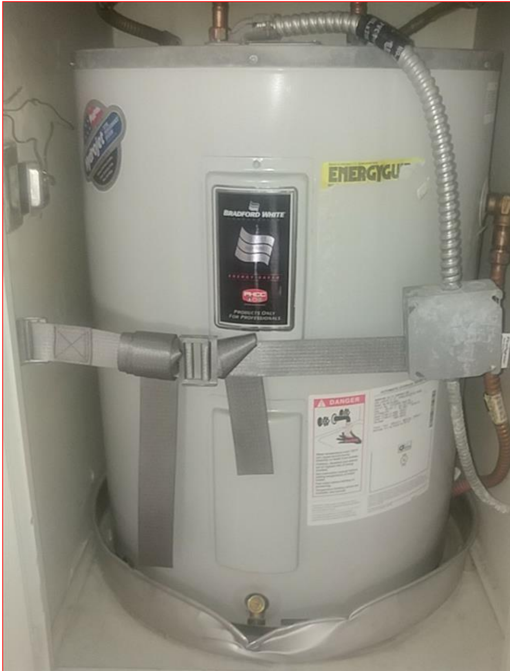
1.2 Item 1(Picture) Water Heater in the hallway is C years old and 40 gallons
