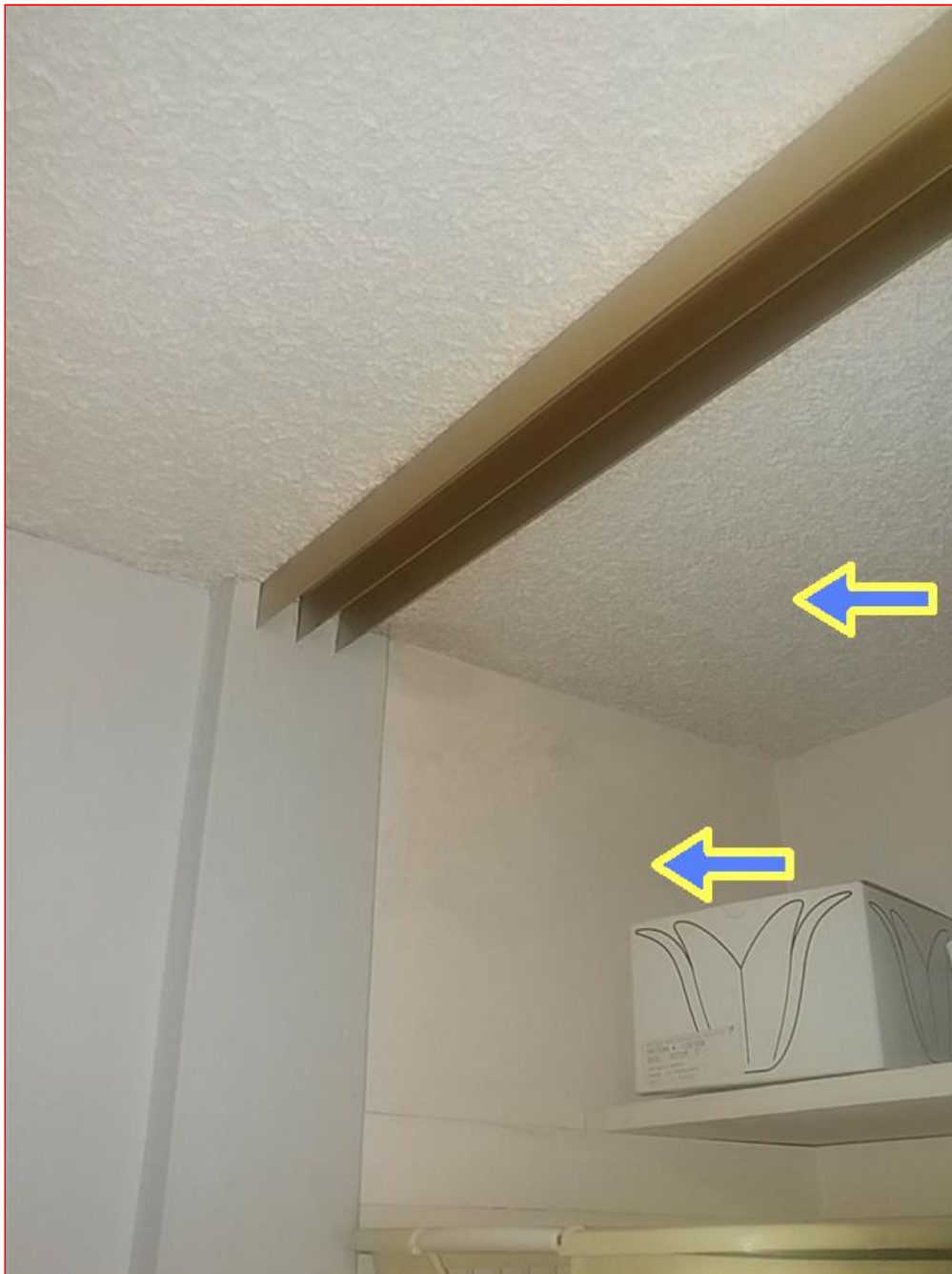
7.3.A Item 1(Picture) There is a moisture stain on the closet ceiling that should be serviced.
