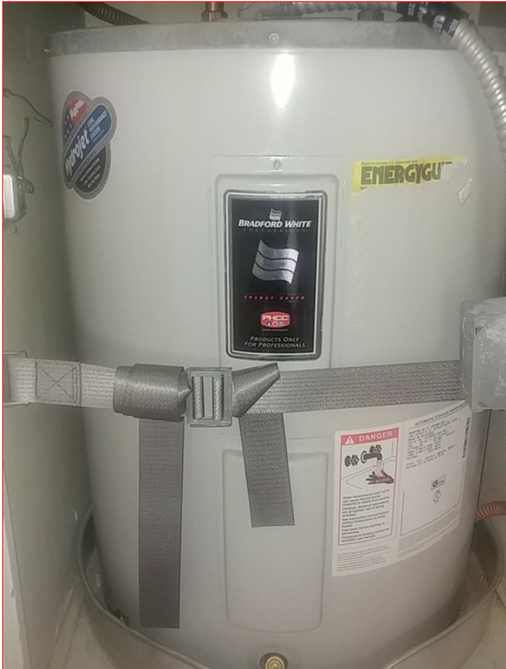
1.2 Item 2(Picture) Water heater is not properly strapped and should be serviced.
