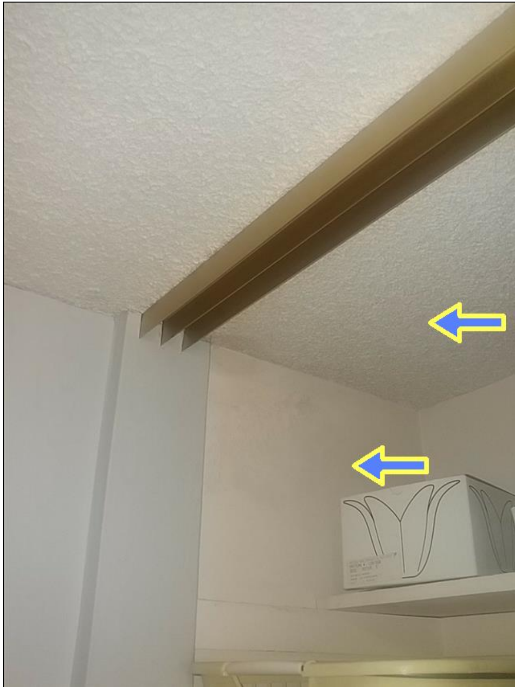
7.3.A Item 1(Picture) There is a moisture stain on the closet ceiling that should be serviced.
