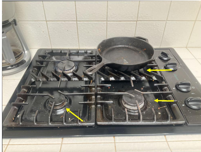
Burner(s) on the gas cook top do not respond or need to be serviced.
