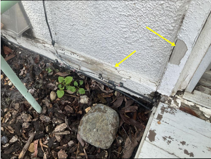
The stucco has been applied over a wood substrate is peeling in places, as a result of inadequate bonding or preparation.
