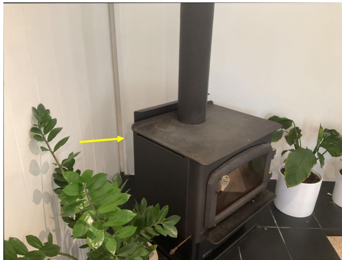
The wood burning stove does not have proper clearance to combustibles. Clearances are determined by the manufacture. Refer to original manufacture installation requirements. We recommend further evaluation by a qualified licensed specialist and serviced as required.
