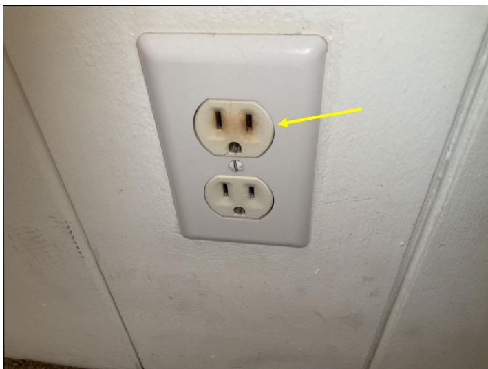
One or more outlets is damaged or has a scorch mark on it, and should be evaluated and serviced by a licensed electrical contractor.
