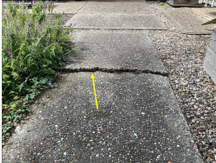
There are several offsets in the walkways that could prove to be trip-hazards.
