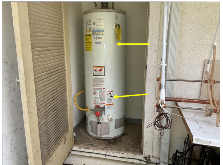
The water heater is not correctly secured, and needs to be seismically strapped and braced in accordance with local standards.
