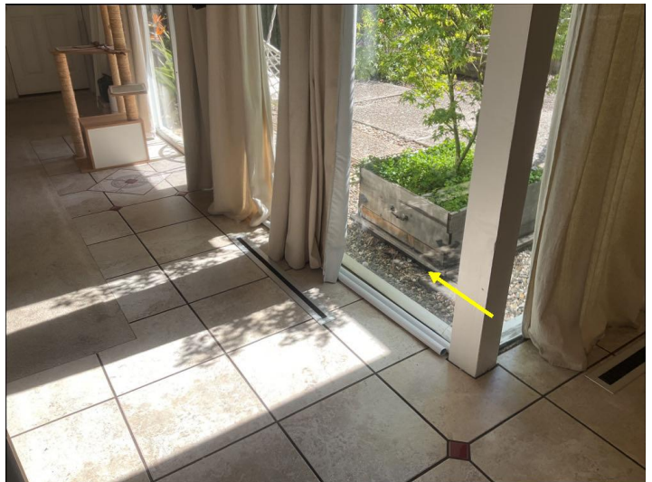
There's one or more windows installed within 18 inches of the finished floor that could not be identified as tempered glass. Current standards require such windows to be tempered or safety glass. We recommend further evaluation by a glass specialist. Often a film can be added that would hold the glass together in case of breakage.
