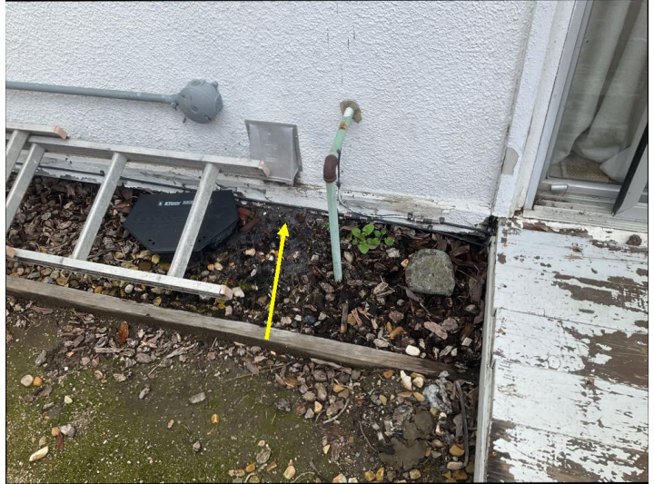
The soil is too high against the home at various areas around the home which should be serviced. Siding clearance should be maintained 2" to hard surfaces, and 4" to soils.
