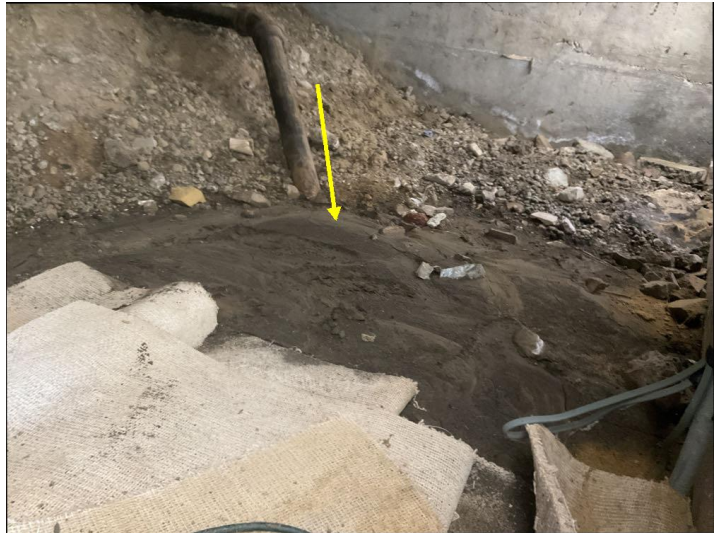
The soils within the crawlspace are moist, which appear to have resulted from recent rains. This can contribute to differential settling, and facilitate the growth of a variety of molds and fungi that can produce unhealthy conditions. The crawlspace should be carefully monitored to insure there is adequate ventilation and that it dries out in an appropriate manner and time.
