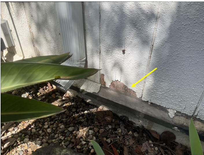
The stucco has been applied over a wood substrate is peeling in places, as a result of inadequate bonding or preparation.
