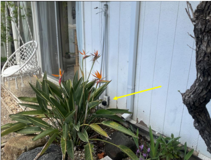
An outlet at the front does not function and should be evaluated and serviced by a licensed electrical contractor.
