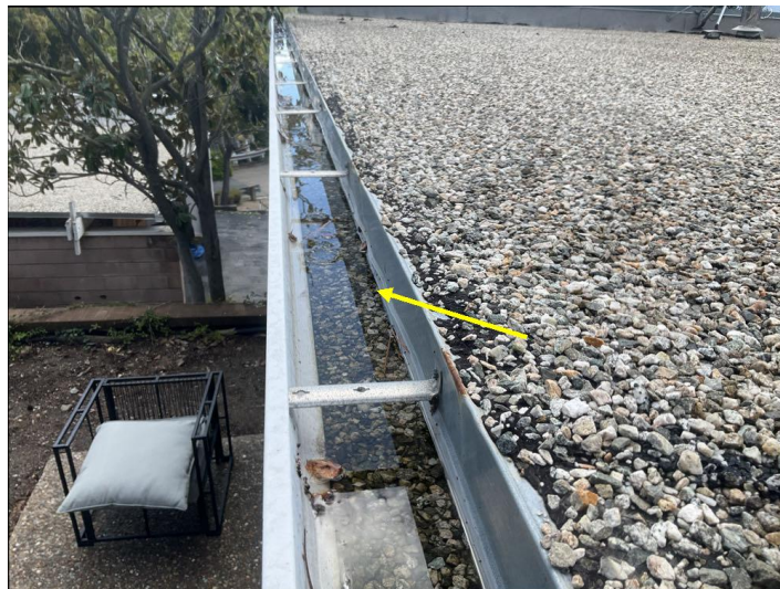
The gutters need to be serviced as well as being cleaned such as securing them or sealing separated seams.
