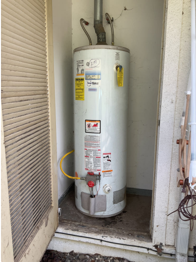
Hot water is provided by a 50 gallon gas water heater that is located in the exterior closet.
