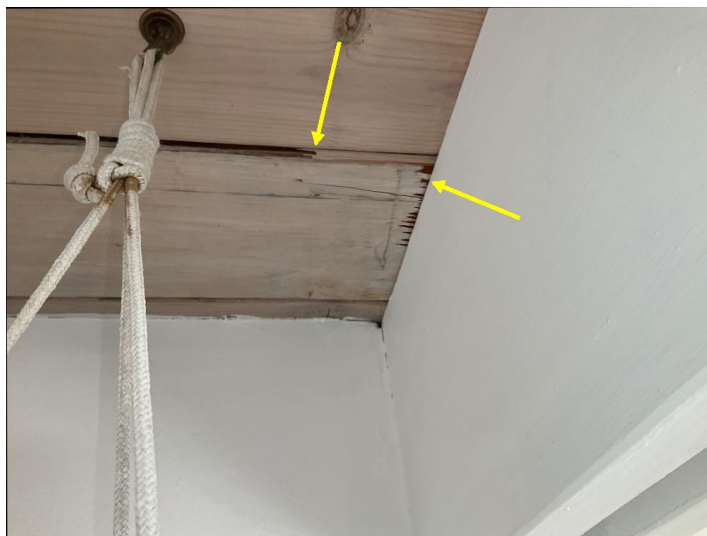
There is a moisture stain/damaged on the ceiling that should be explained or explored further. The area is currently dry after recent storms.
