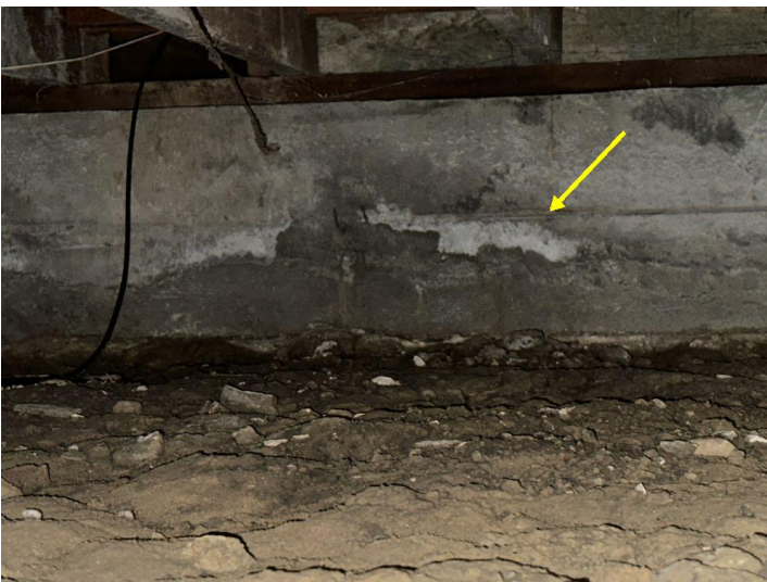
Moisture has entered the crawlspace, as is evident by salt crystal formations around the base of the stem walls. However, this is a common phenomenon that does not necessarily indicate a chronic or serious problem. The soils are currently dry, but it would be prudent to monitor this area.
