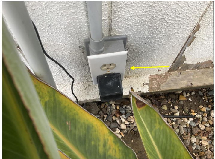
Some of the exterior electrical outlets do not have a weather rated cover or the cover is damaged and should be serviced.
