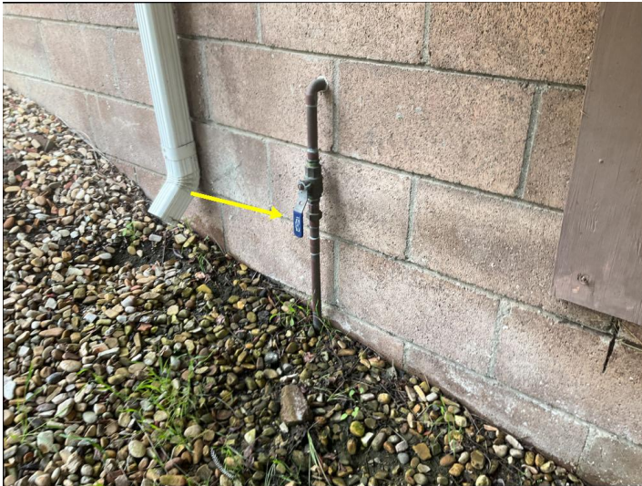
Main water shutoff
