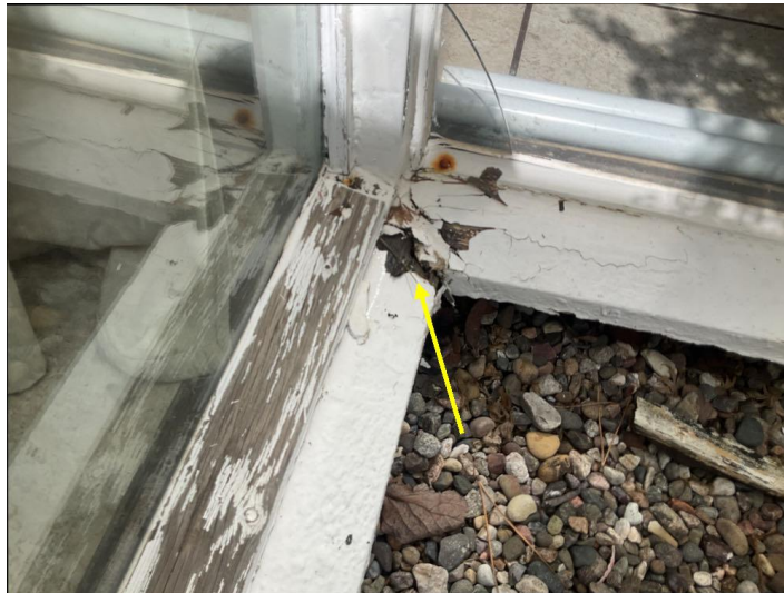
There is damage to the wood trim that should be evaluated by a termite inspector.
