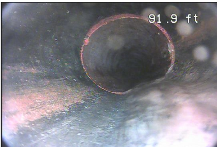
ABS to Clay pipe connection
