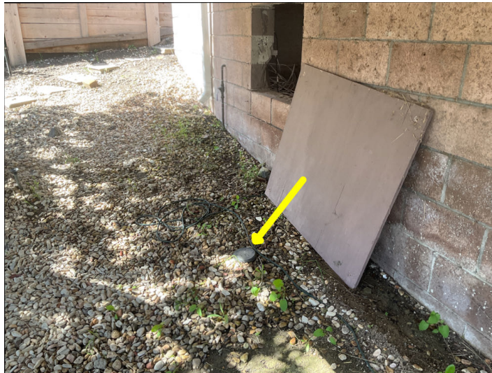
A clean-out is located at the front.
