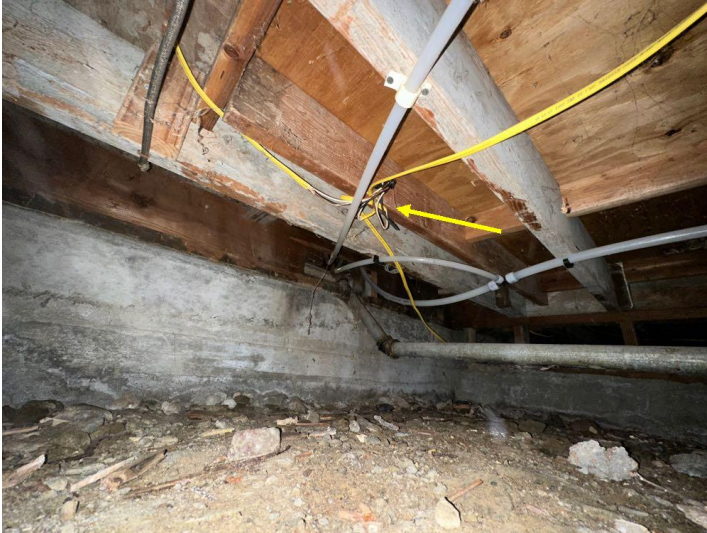
An electrical connection within the crawlspace have been incorrectly made outside of junction boxes. All such connections should be made within junction boxes in order to contain any arcing or sparking that could occur.
