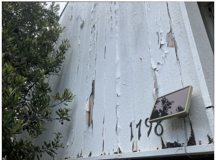
The siding needs typical maintenance such as sealing and painting. This should include caulking and filling gaps or openings such as small cracks or openings at hose bibs, and sealing with a proper primersealer, then one or two finish coats.
