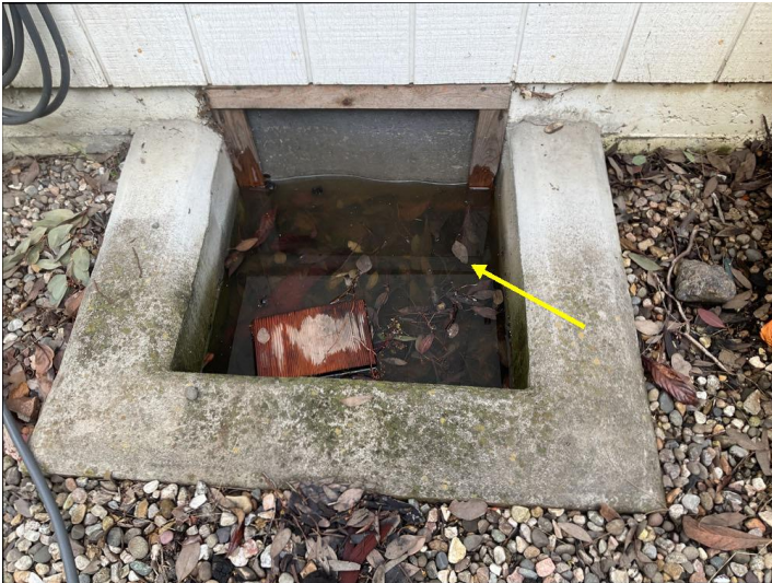
We cannot access all areas of the foundation crawlspace, due to the obstruction of ducts pipes or conduit and or limited space. We were able to inspect or view about 80%. The Area under the office is under water and was not evaluated.
