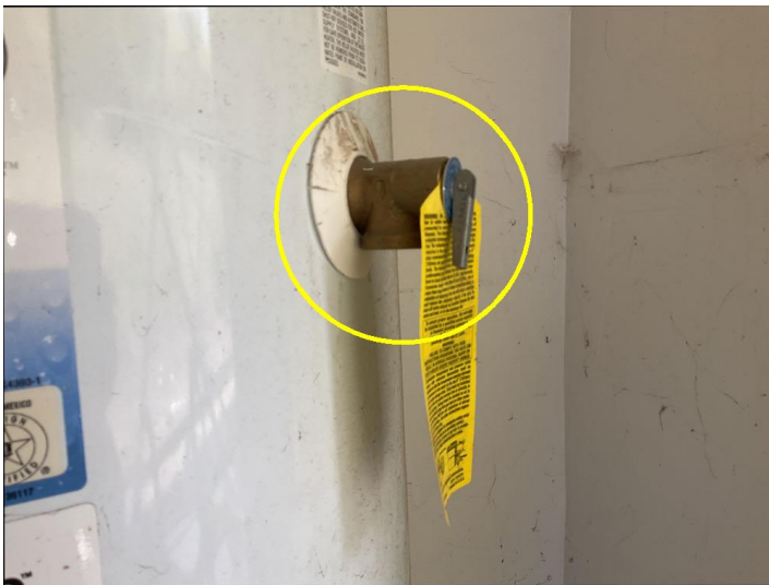
The pressure relief valve on the water heater does not have a discharge pipe. One should be installed to terminate no more than 24 inches above grade and no closer than 6 inches to it and be directed down towards the ground.
