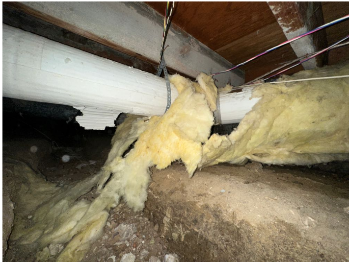
The ducts are rigid metal type that are mostly insulated with fiberglass. Some insulation is missing and should be serviced for more efficiency.
