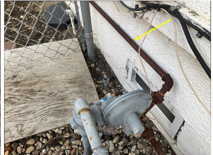
Some gas lines are rusted and should be painted to prevent further corrosion.
