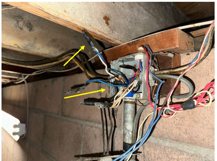
Electrical conduits within the crawlspace were not professionally installed and include detached electrical junction boxes, loose or unsecured vinyl conduit, or conduit without restraint clamps, et cetera, which should be evaluated serviced by a licensed electrician.
