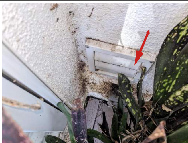
No air flow at dryer termination while dryer was operating
