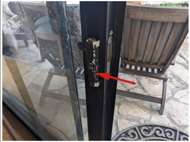
Sliding doors difficult to open, door handle broken
