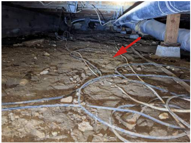
Moist soil under master bedroom area
