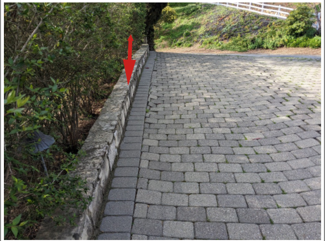
Side retaining wall is leaning and appears to have moved
