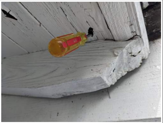
Wood damage roof eaves, roof leaks
