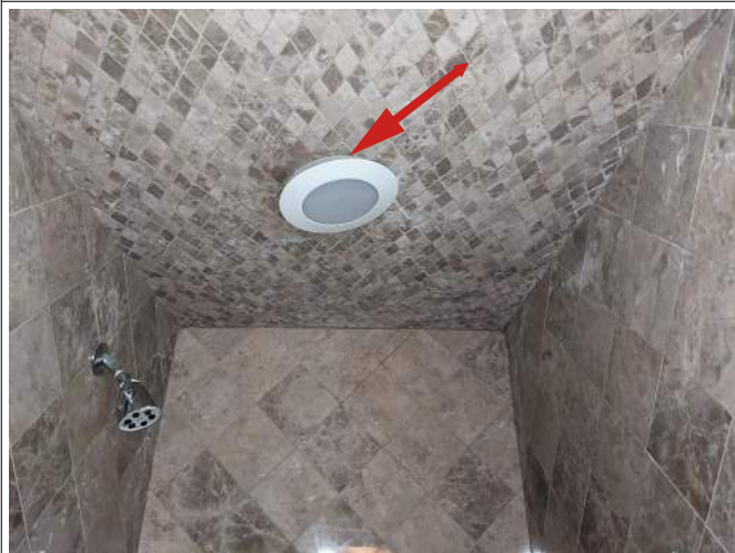
Light in shower inoperable
