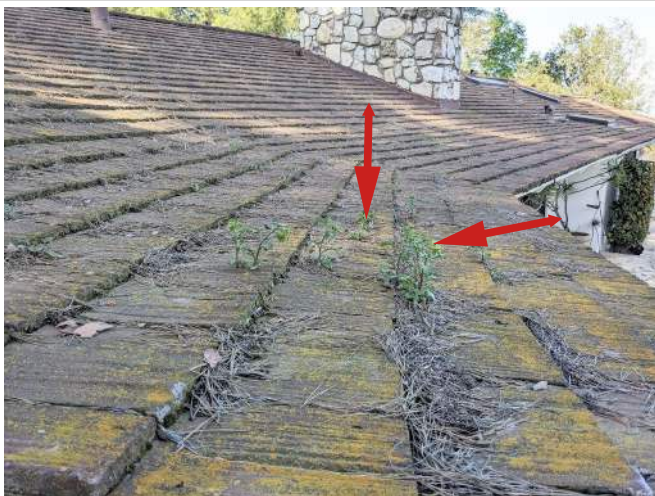
Roof slope too low, debris and weeds growing on roof
