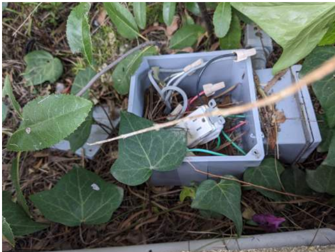
Missing cover at electrical box alongside driveway
