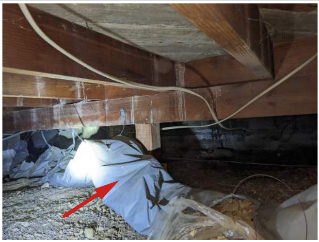
Damaged abandoned ducting under house
