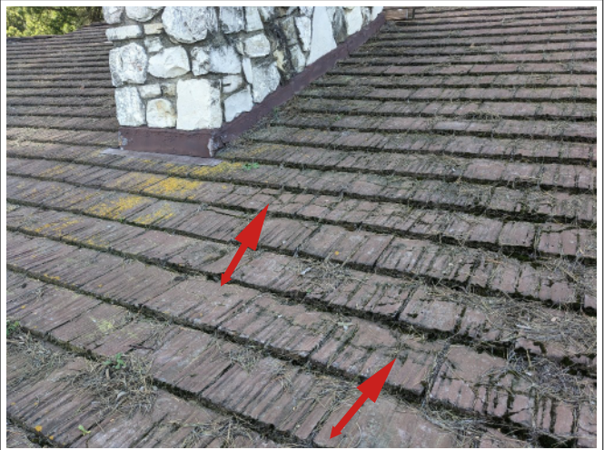
Cracked and damaged tiles
