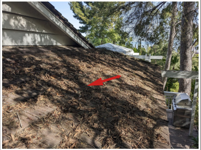
Tree leaf debris on roof
