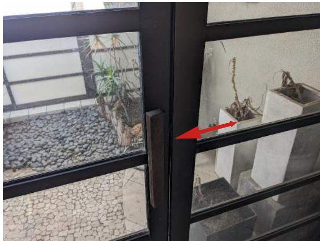
Master bathroom door miss aligned and not latching
