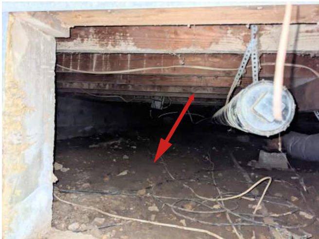
Moist/damp soil under master bedroom area, source not determined
