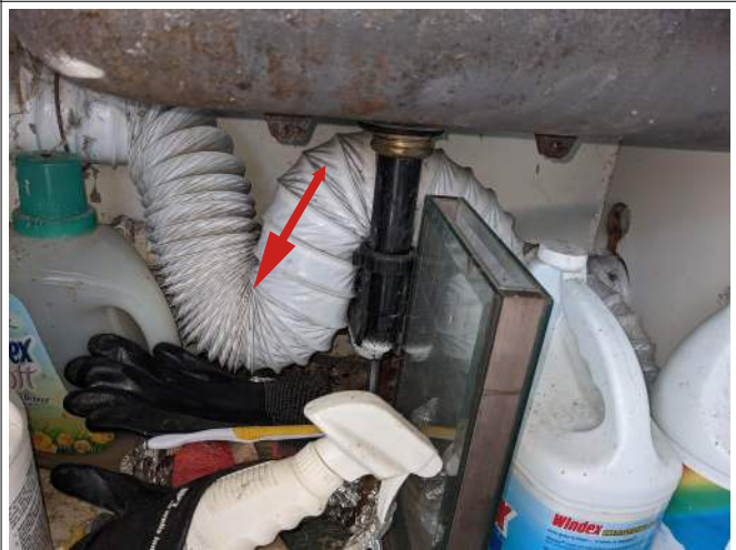
Laundry dryer vent improper and clogged
