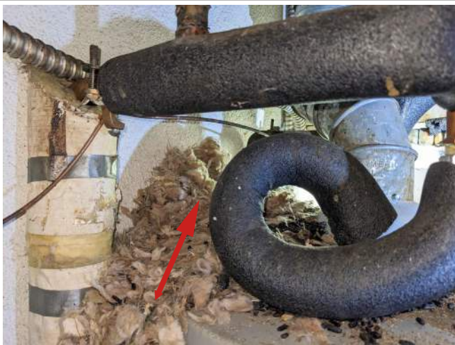
Rat nesting insulation on top of water heater
