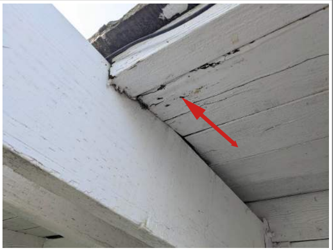
Wood damage rear eaves
