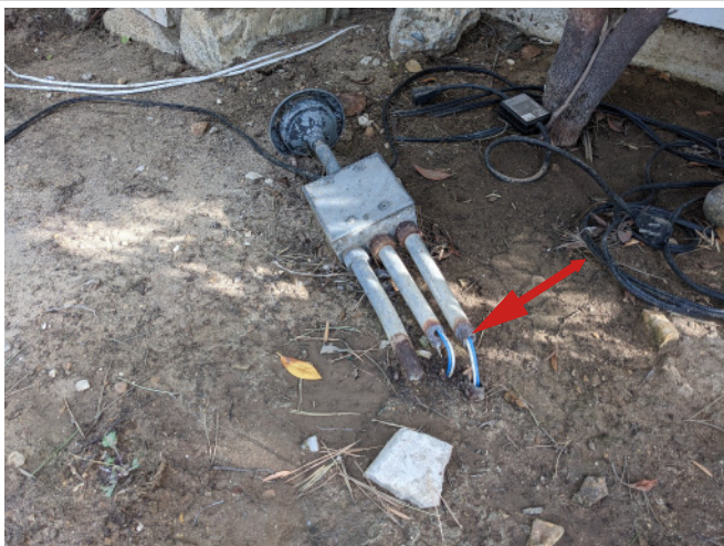
Damaged landscape lighting
