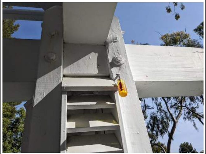
Wood damage at deck cover structure
