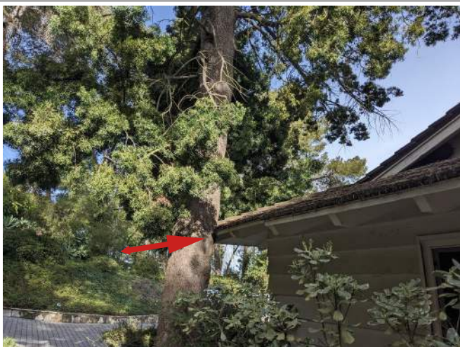
Tree touching garage roof
