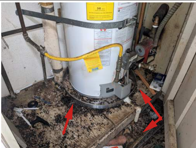
Rat droppings around rear water heater
