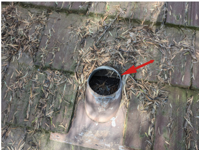
Roof vent flashing cover missing
