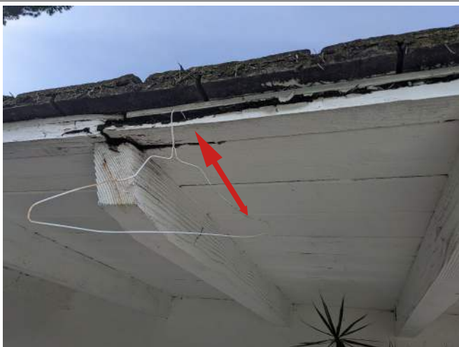
Wood damage rear eaves, roof slope too low
