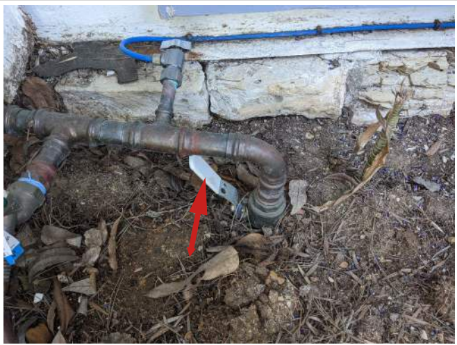
Main plumbing water shut off valve buried in soil
