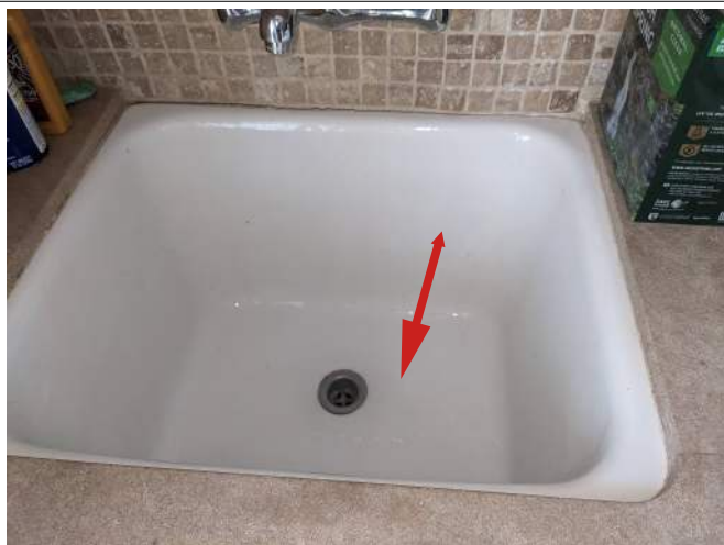
Laundry sink slow draining
