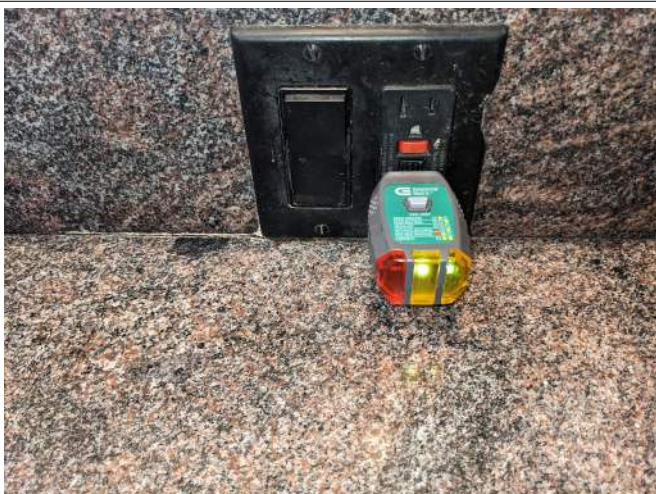
GFCI inoperable in kitchen
