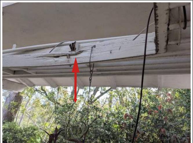
Wood damage outside kitchen window
