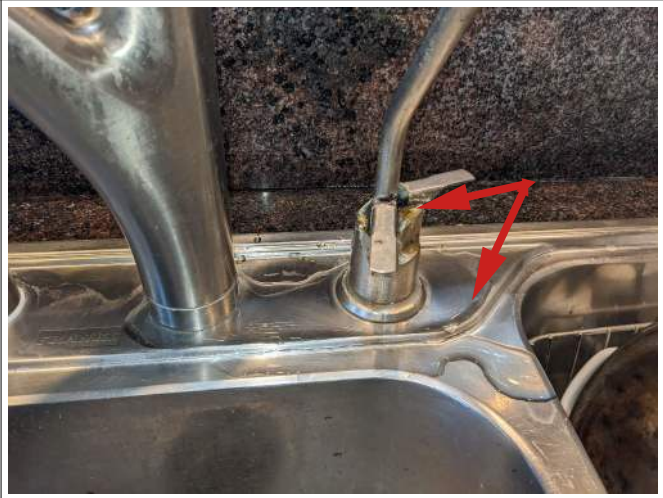
Water dispenser faucet leaking
