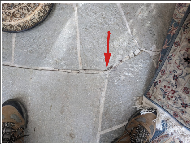
Cracks in rear office floor tile joints
