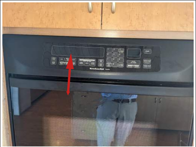
Over power shut off, circuit breaker improper size
