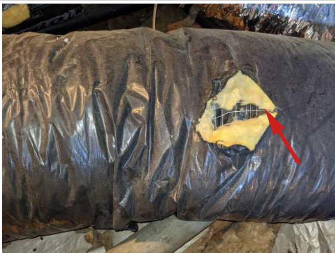
Damaged duct in main attic
