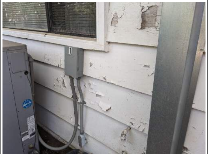
Wood siding paint finish peeling
