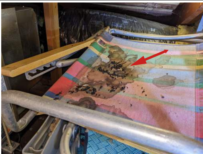
Rat droppings and urine stains in garage attic
