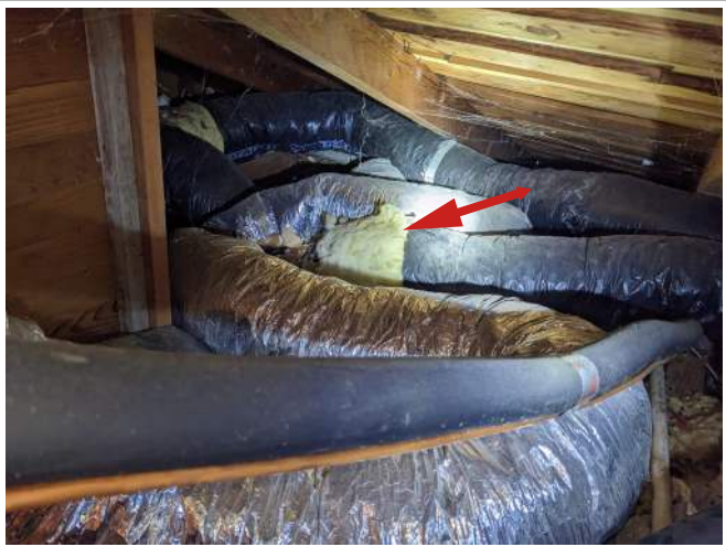
Air leaking from ducting in main attic
