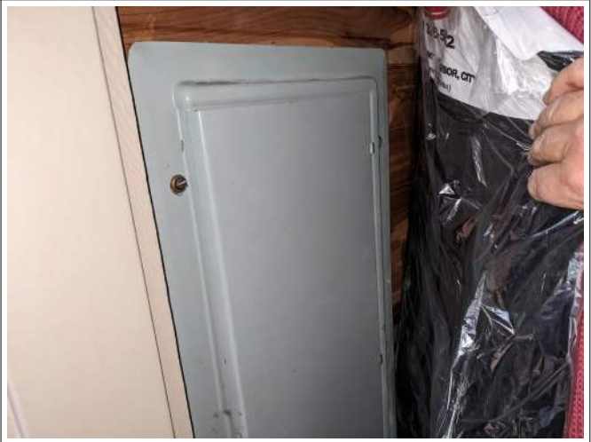
Improper electrical panel in clothes closet
