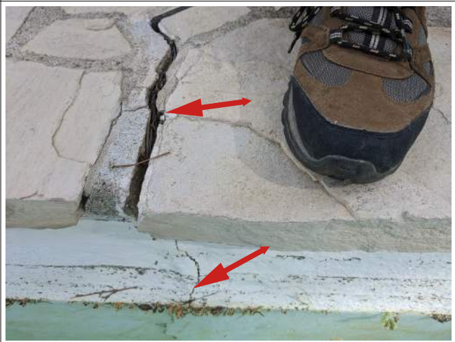
large cracks through bond beam and into pool
