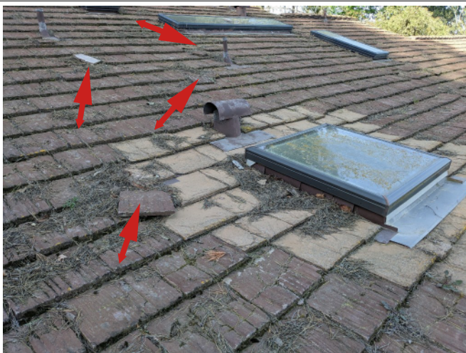
Lots of broken tiles
