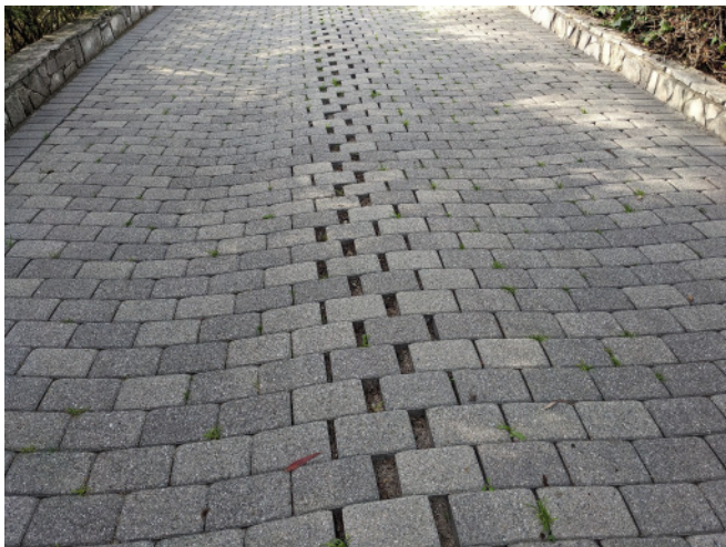
Gaps in driveway pavers due to settlement and movement
