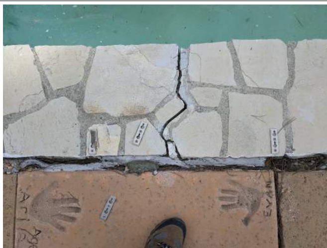
Pool patio separations, large cracks through bond beam and into pool
