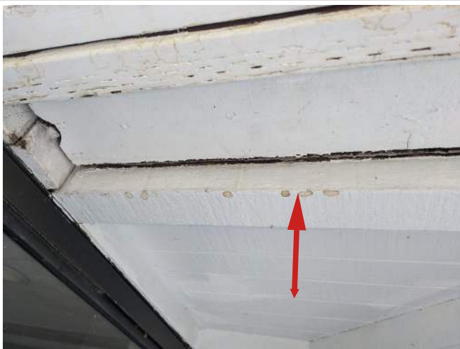
Water drips from roof leaks
