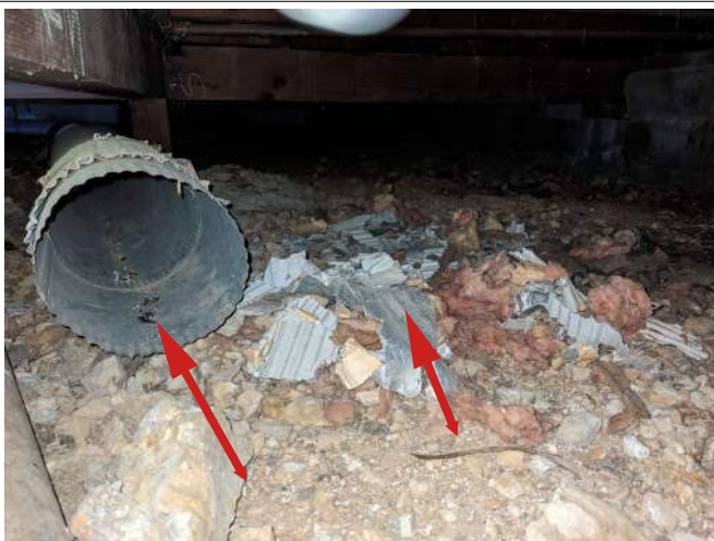
Old ducting under houses, asbestos insulation
