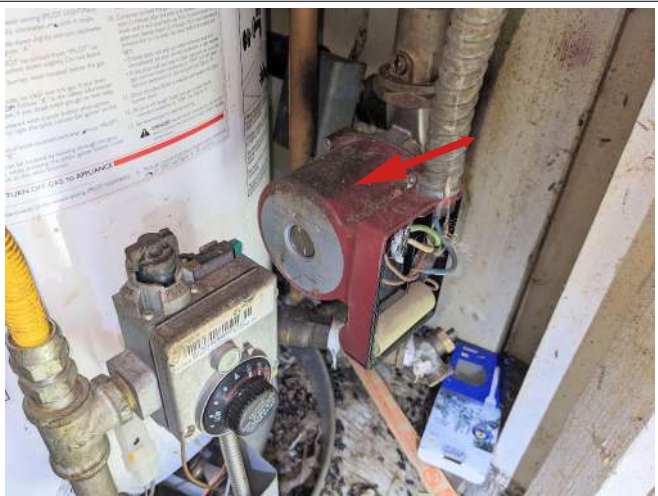
Water heater recirculation pump inoperable
