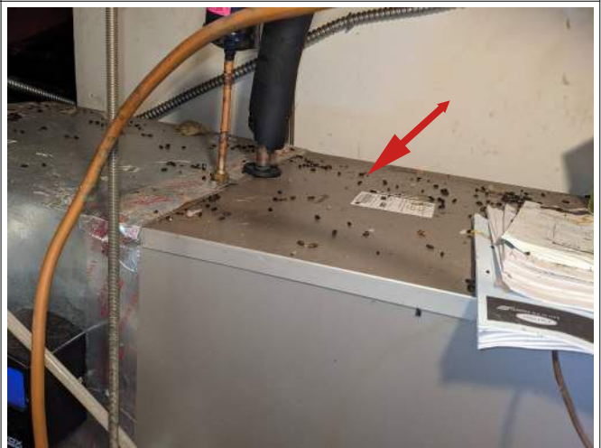
Rat dropping on and around furnace in garage attic
