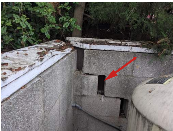
Pool equipment wall movement
