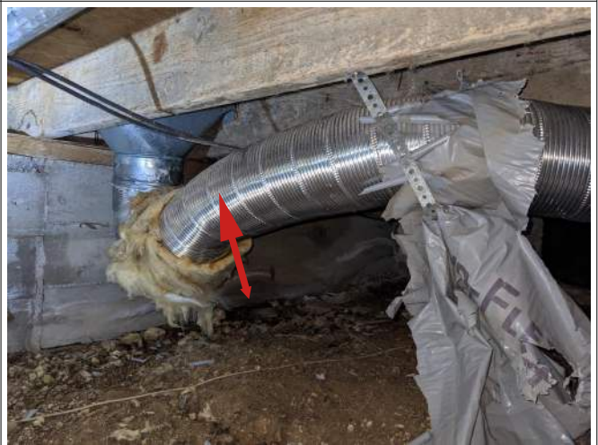
Damaged/abandoned ducting under master bedroom
