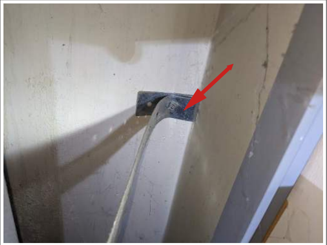
Hallway water heater strapping improperly secured
