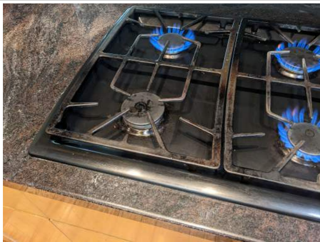
Burner ignitor inoperable
