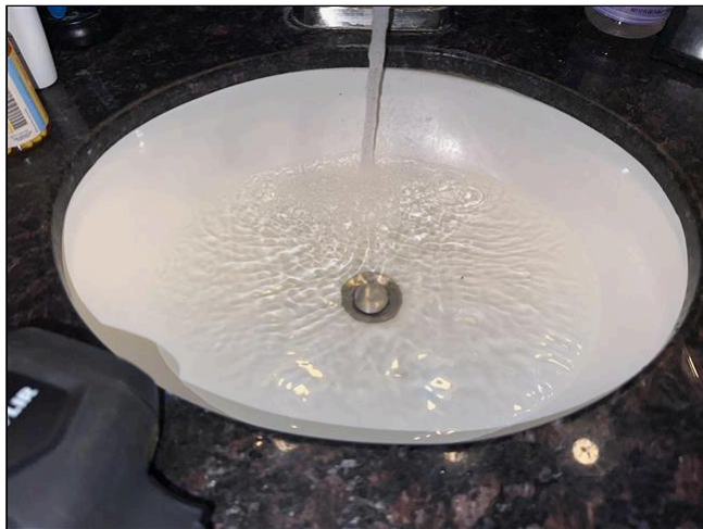
Item 1 - Item 1(Picture) Plumbing System
