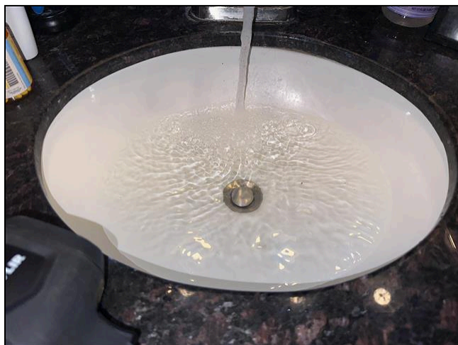
5.0 Item 1(Picture) Plumbing System
