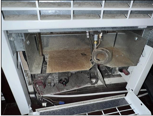
4.0 Item 2(Picture) Heating/Central Air
