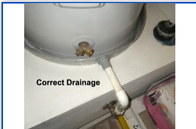
2.1 Water heater drip pan exampe
