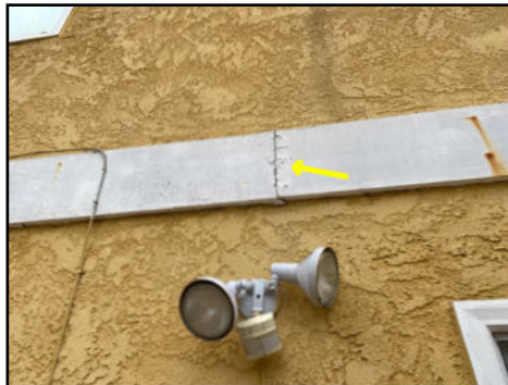
Deteriorated wood - needs to be serviced - consult termite report
