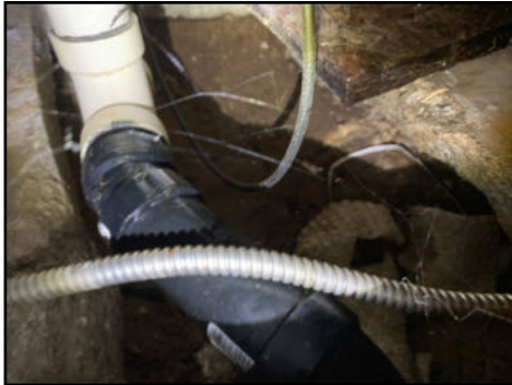
Visible leaking under spa tub. recommend licensed plumbing contractor for further evaluation and repair
