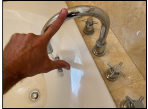
Loose fixture(s) - needs to be serviced
