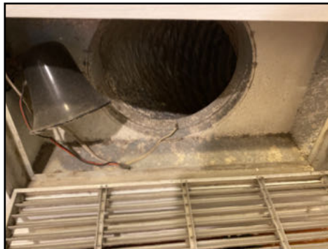
Missing filter - needs to be serviced
