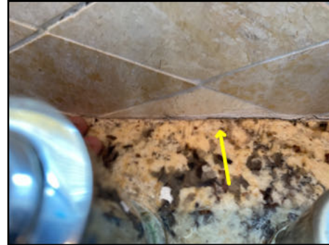
Gap at backsplash to countertop joint - needs to be serviced
