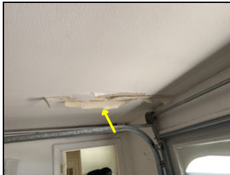
Heavy blistering - needs to be evaluated/serviced
