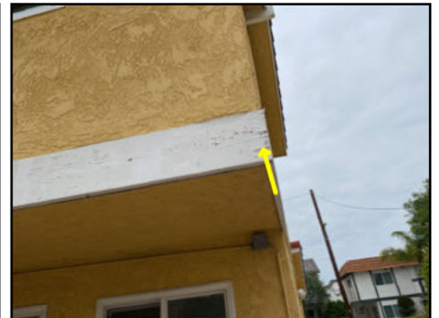
Weathering, cracking and staining present - typical for age and weather exposure - recommend maintenance
