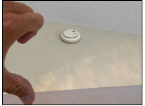
Did not operate - needs to be serviced or replaced
