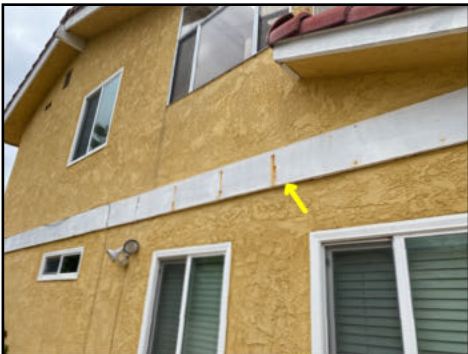
Recommend general trim maintenance and sealing any holes/gaps
