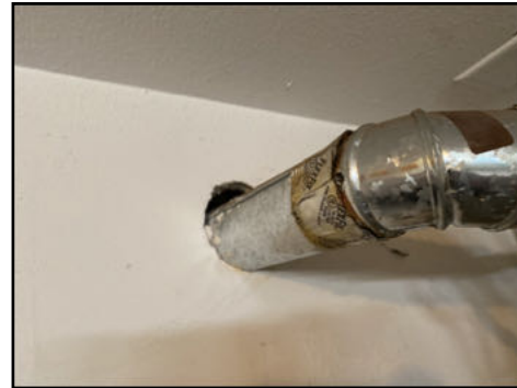
Vent too close to combustibles - needs to be serviced
