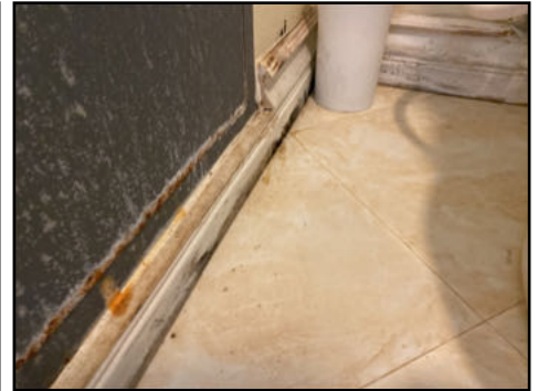
Stains at base - moisture present when tested with moisture meter - needs to be serviced/further evaluated
