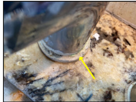
Corrosion present at fixture(s) - signs of wear
