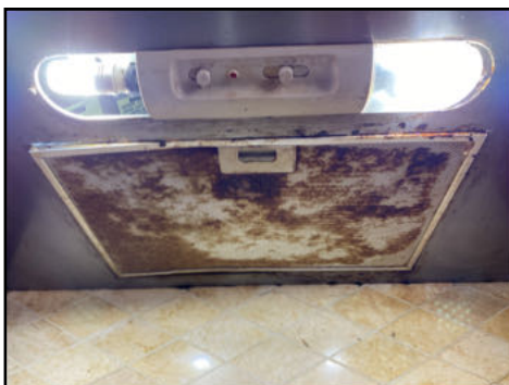
Greasy/dirty unit - recommend cleaning
