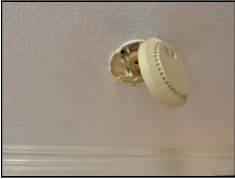
Did not operate - needs to be serviced or replaced
