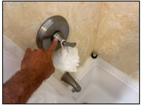
Tub fixture difficult to operate - needs to be serviced
