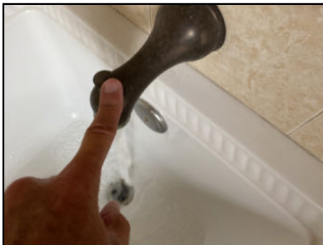
Tub to shower diverter not operating properly - needs to be serviced
