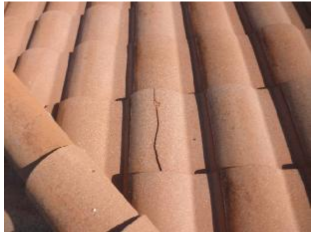
Cracked roof tile at the east facing slope.
