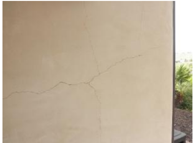
Example of the excessive surface cracking at parts of the plaster walls.
