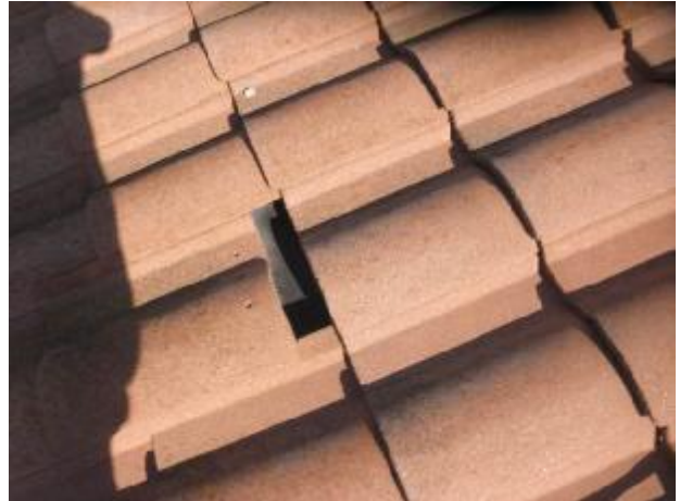
Displaced roof tile at the west facing slope.
