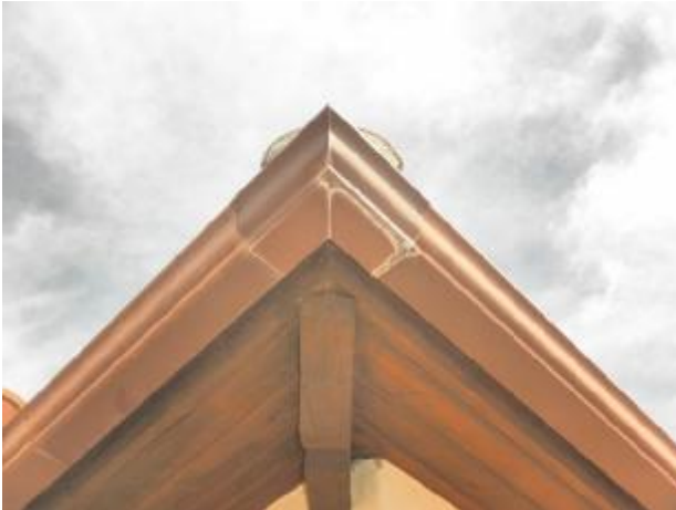
Some of the gutter seams are leaking.
