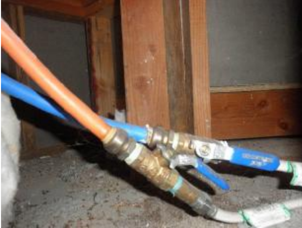
Example of the Kitec plumbing water lines at the master bath hydrotherapy tub.
