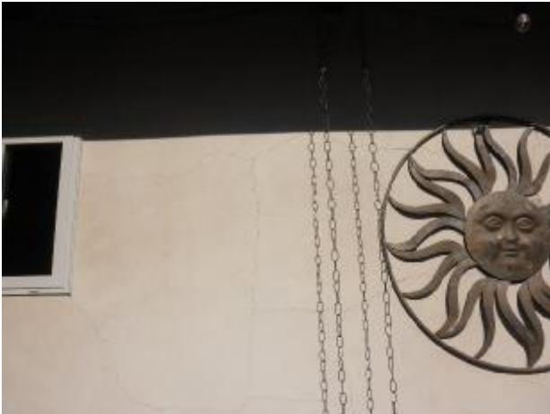
Example of the excessive surface cracking at parts of the plaster walls.
