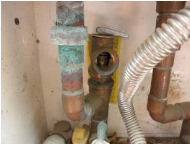
Missing discharge pipe for the TPR valve on the pool house water heater.
