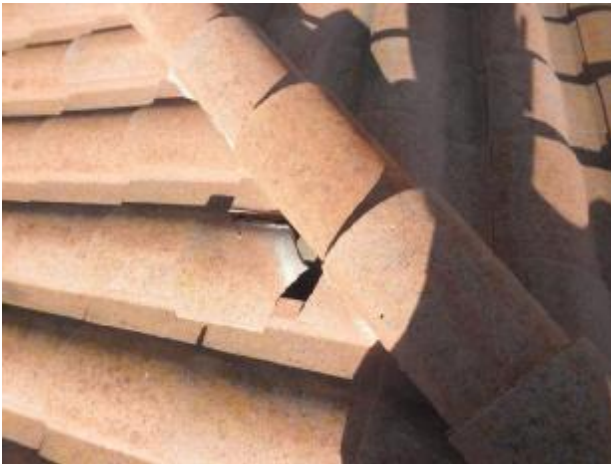
Cracks and displaced roof tile at the NW slope.
