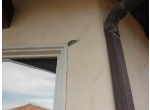
Damage to the stucco above the family room window.
