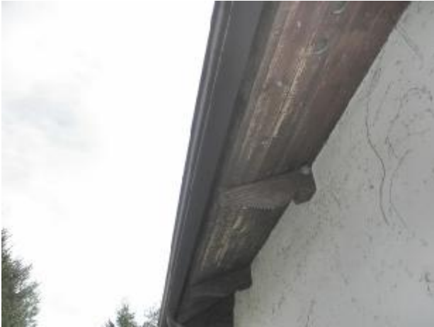
The soffit at the NE eave needs to be refinished.
