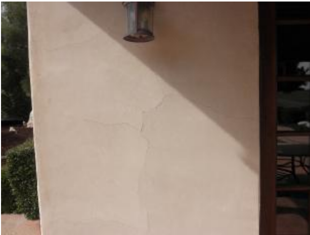
Example of the excessive surface cracking at parts of the plaster walls.
