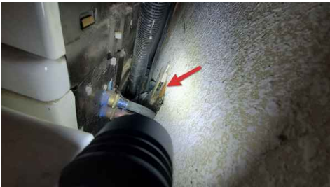
This is the fire wall and it needs to be complete.
