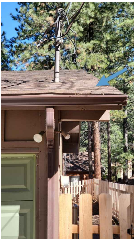
Looks to be a failure of the fascia and roof deck
