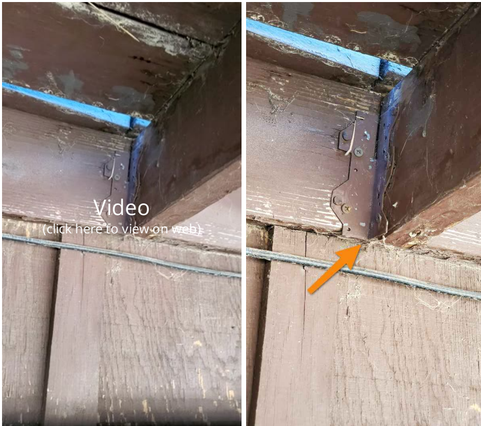
wrong type of hanger for purpose.
