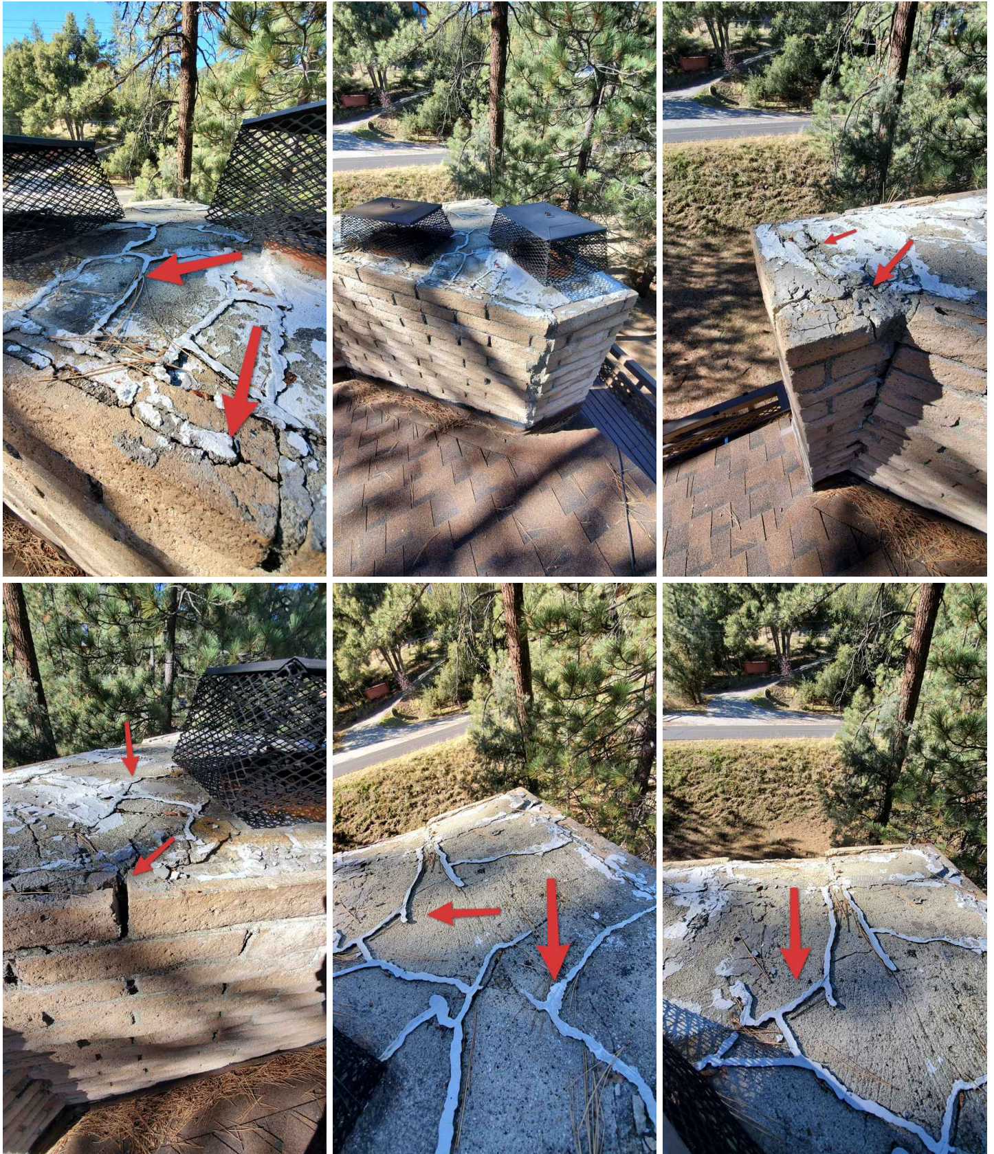
Failed caulking, inappropriate repair
