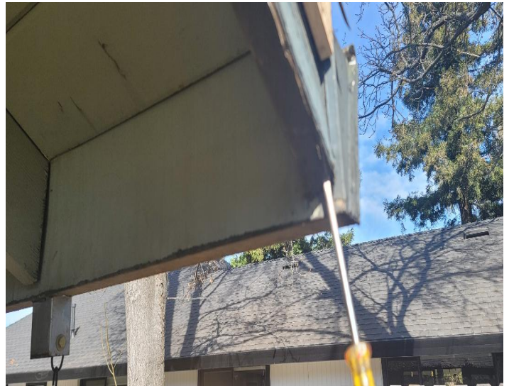
3B - Damaged barge rafter at the left rear corner.
