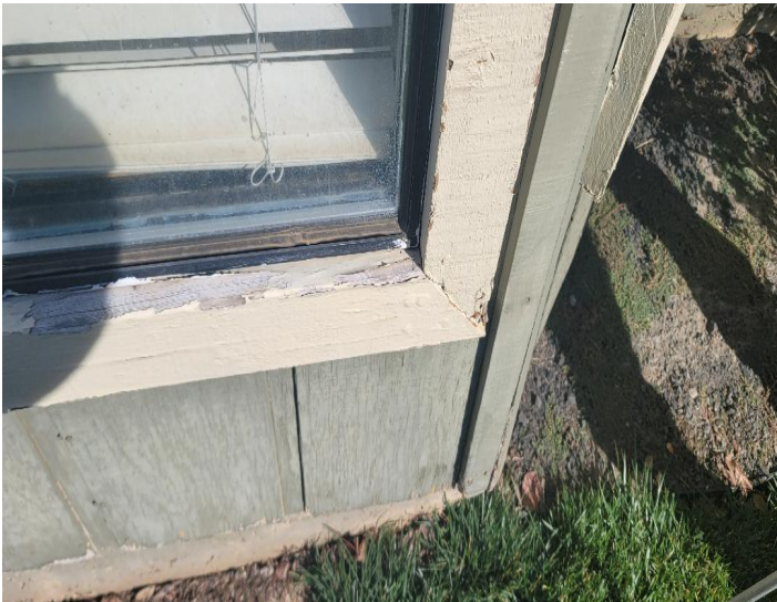
3A - Damaged window trim.
