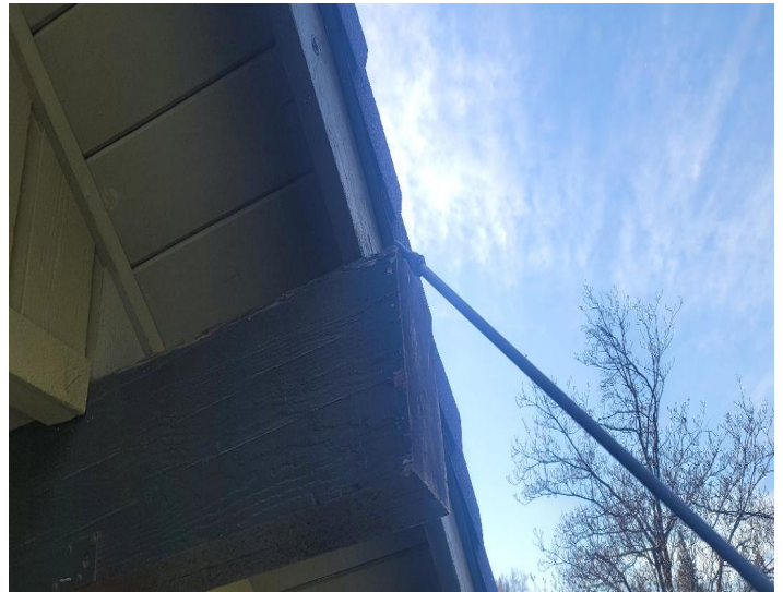
3B - Damaged top of the support beam at the front of the structure.
