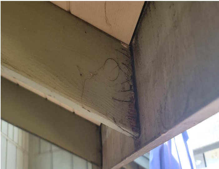
3B - Damaged rafter tail at the left side of the structure.
