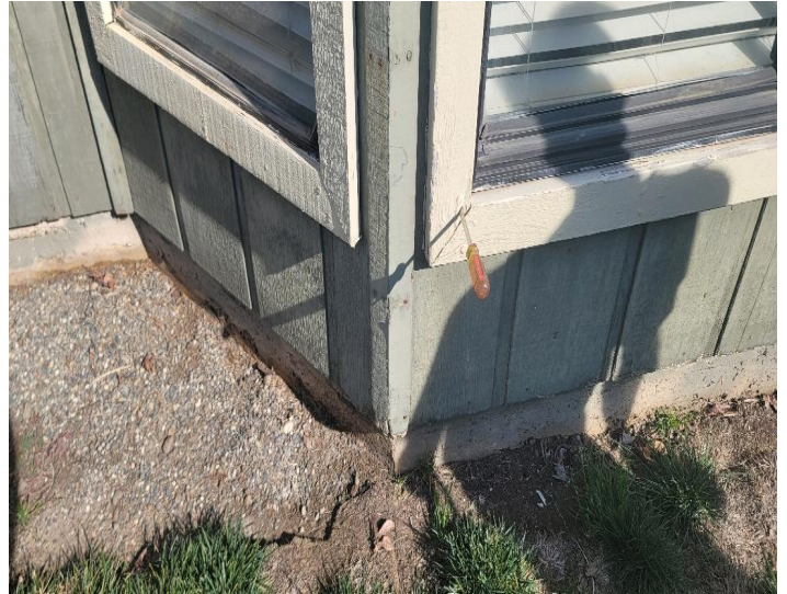
3A - Damaged window trim.
