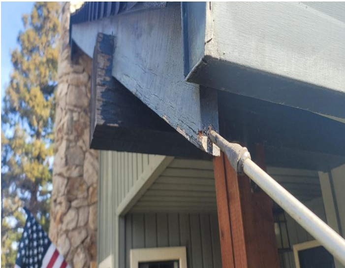
3B - Damaged barge rafter at the front of the structure.
