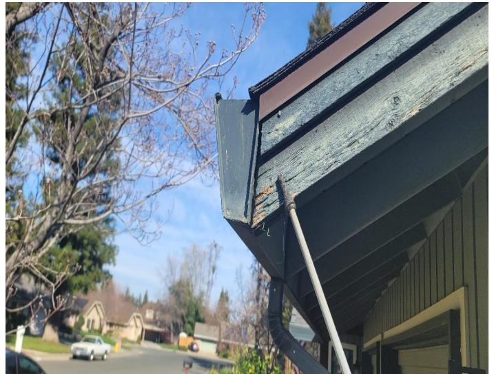
3B - Damaged barge rafter.
