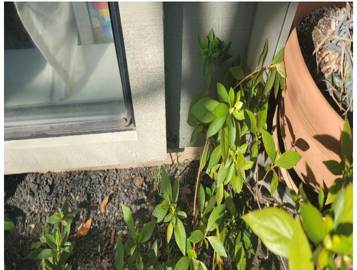
3A - Damaged siding.
