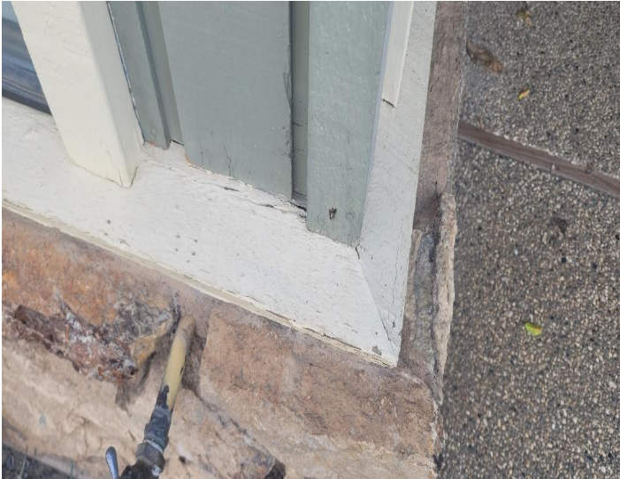
3A - Damaged corner trim.
