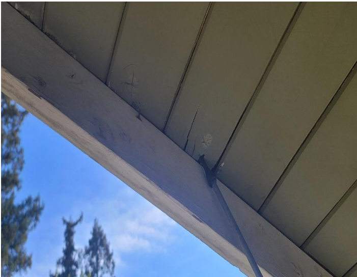
3B - Damaged roof sheathing on the rear patio roof.
