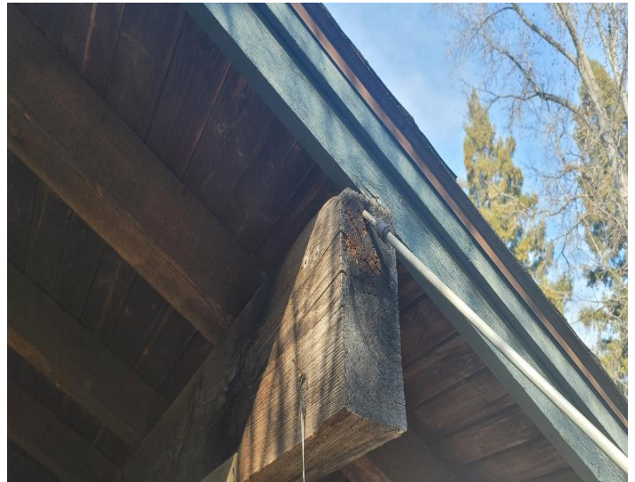
3B - Damaged roof beam end at the rear patio roof.
