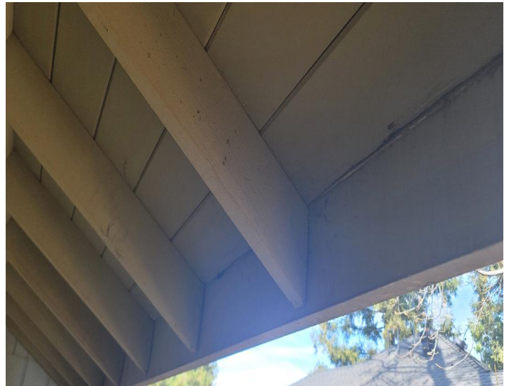
3B - Damaged roof sheathing at the left side of the structure.
