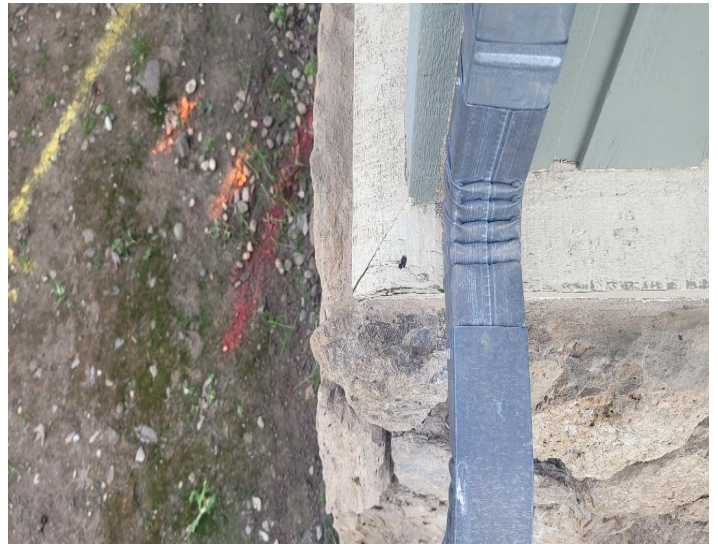
3A - Damaged water table trim.
