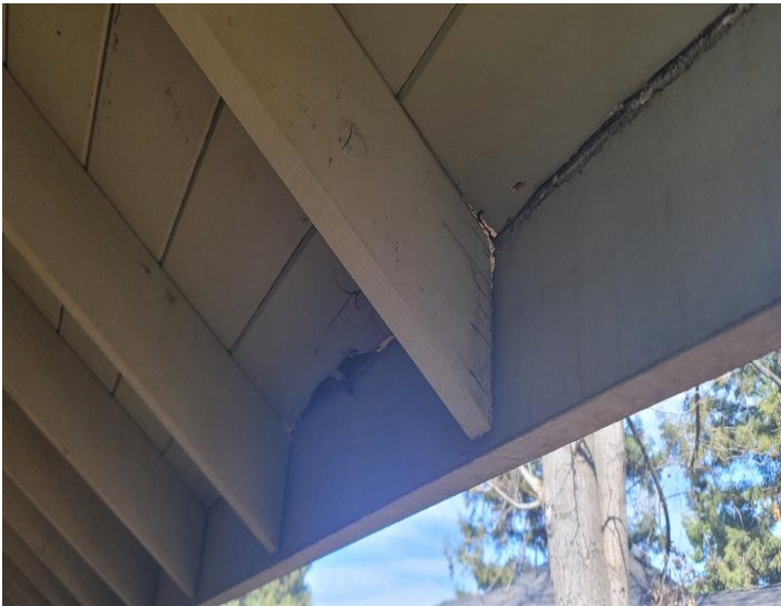
3B - Damaged roof sheathing at the left side of the structure.
