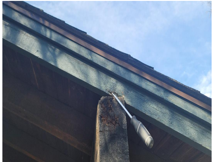
3B - Damaged barge rafter at the rear patio roof.
