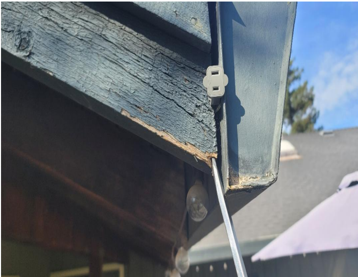
3B - Damaged barge rafter at the rear patio roof.
