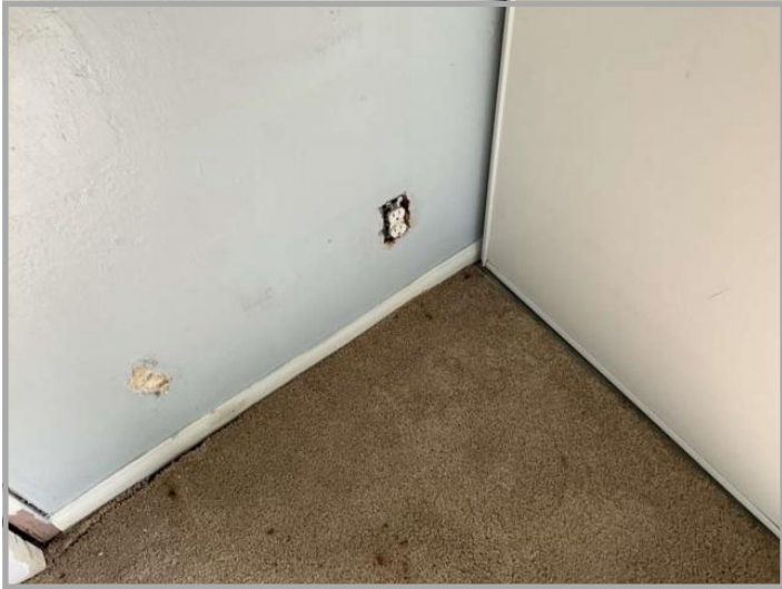
Missing Outlet Cover at Basement
