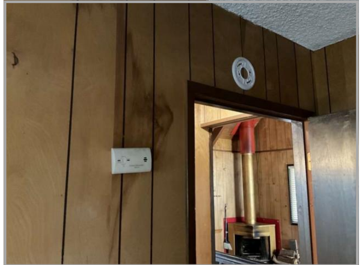
Missing Bedroom Smoke Detector
