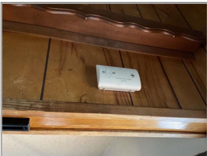
Carbon Monoxide Detector at Main Level
