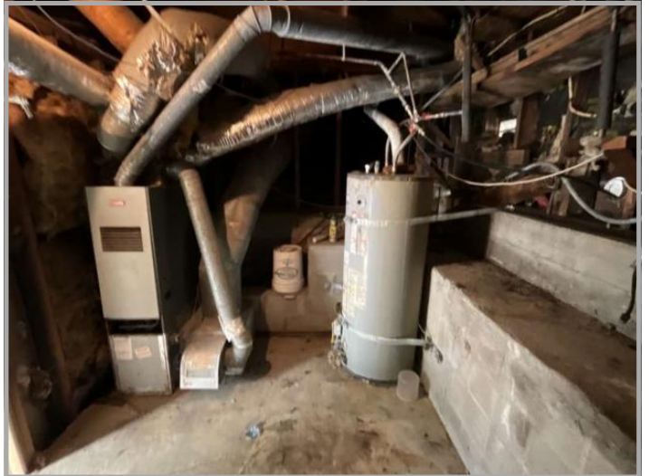
Water Heater- Legally Strapped
