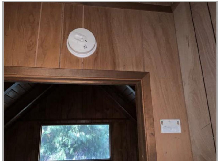
Smoke Detector at Upper Bedroom, Missing Carbon Monoxide Detector at Upper Level
