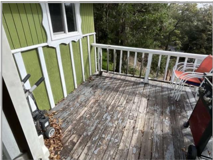
Decking Paint Peeling
