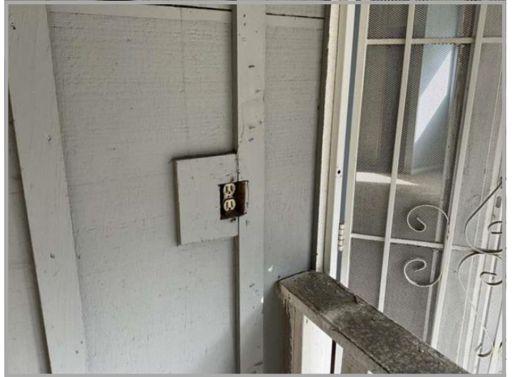
Missing Outlet Cover at Exterior Right Side
