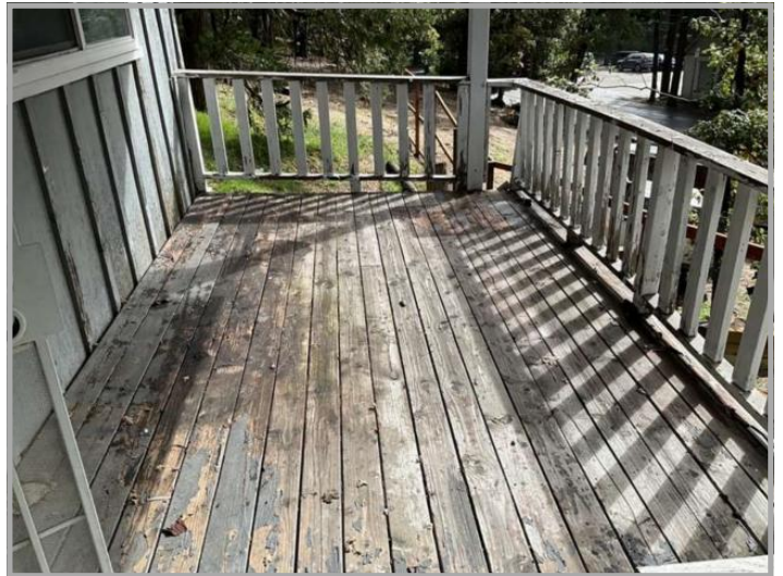
Decking Paint peeling
