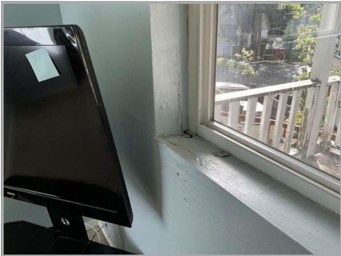
Water Damage Evidence at Basement
