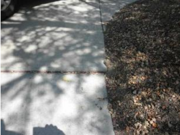
Tripping hazard at the uplifted concrete driveway.
