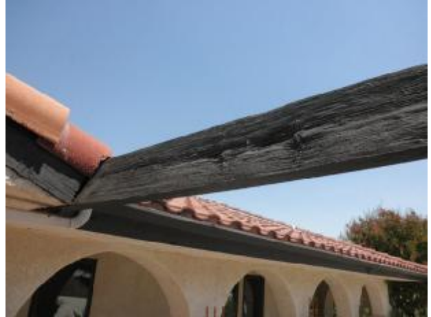
Moisture damage at the fascia board.
