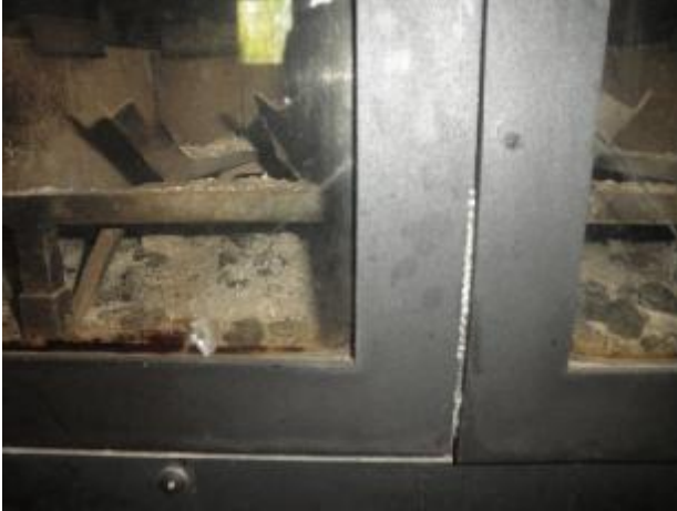
Cracks in the glass doors at the living room fireplace.
