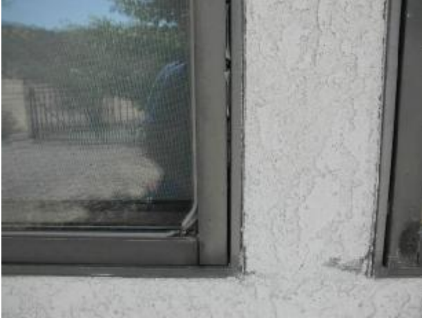
Loose/damaged weather stripping at the garage window.
