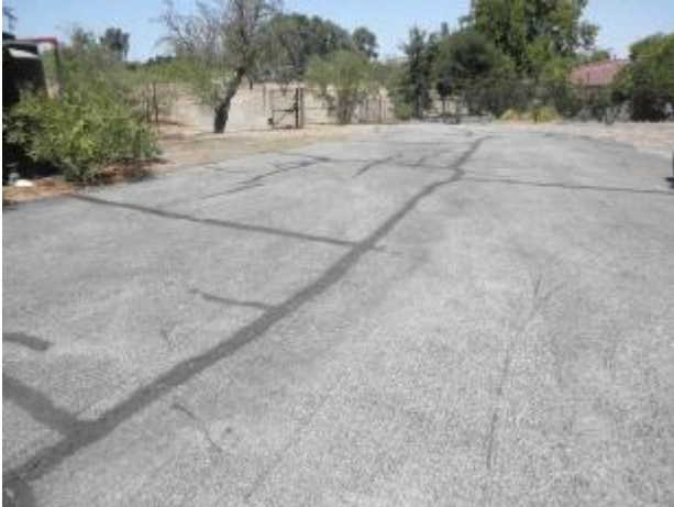
The asphalt portion of the driveway needs maintenance sealing.
