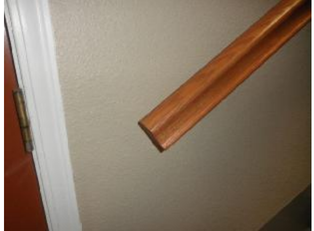
Handrails at the family room do not return to the wall.
