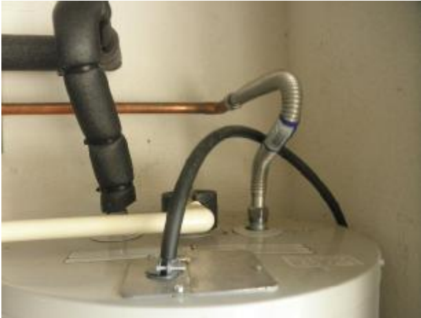
Exposed wiring at the Bradford White water heater.
