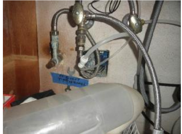
Open junction box below the kitchen sink.
