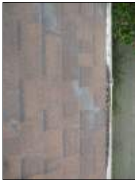
Missing/damaged shingles/tiles in areas - needs to be serviced
