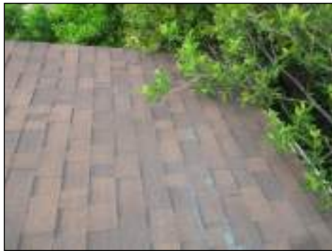
Tree branches rub roof - needs to be cut back
