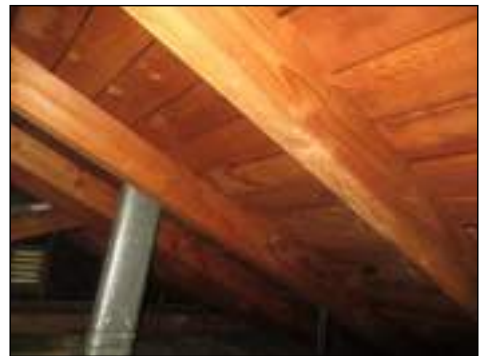
Large stains present on wood members of structure - needs to be serviced and further evaluated for possible leak
