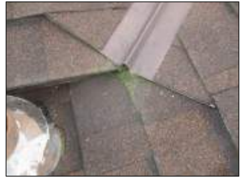
Moss growth present in areas - sign of moisture accumulation and lack of sunlight for drying - recommend servicing as part of seasonal maintenance
