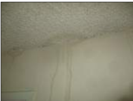
Stains/blistered areas - tested dry with moisture meter/thermal Imaging device at time of inspection - monitor area for moisture
