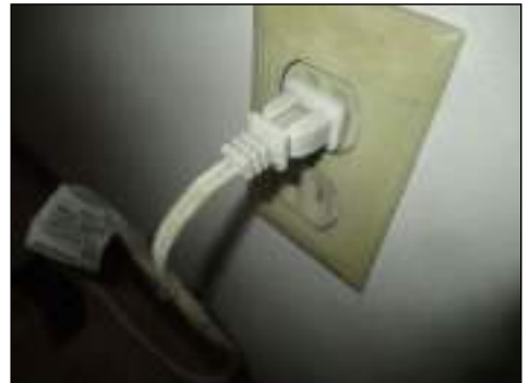
Ungrounded outlets present - typical for the age of the structure - consider upgrading electrical services
