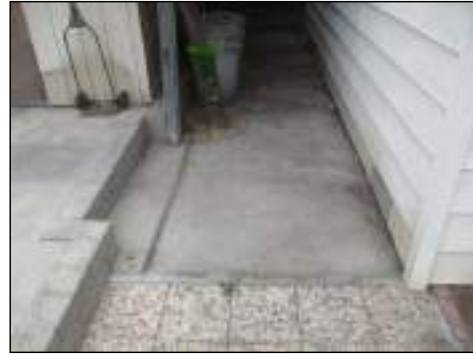
Small localized water ponding may occur in areas - monitor these areas as drains may be needed
