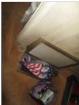
Pilot not lit could not test - needs to be serviced
