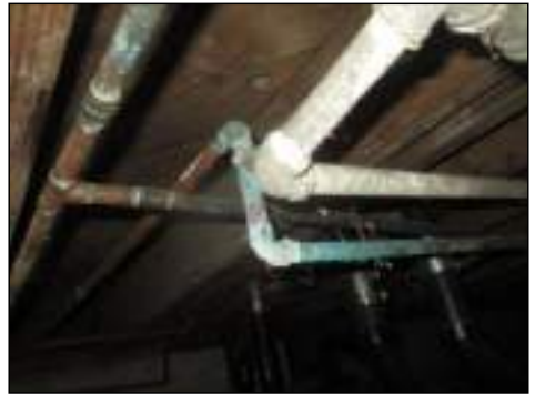
Corrosion at supply piping - recommended further evaluation by a licensed plumber
