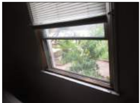
Evidence of possible moisture entry point - needs to be serviced/further evaluated
