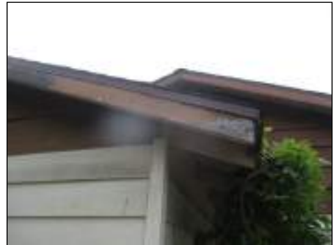
Exposed wood surfaces, wood rot & deterioration can occur - recommend servicing
