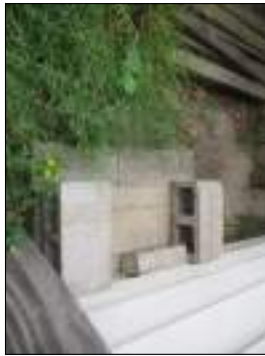
Irregular installation/workmanship - needs to be serviced
