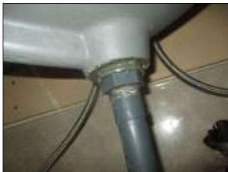
Visible leaking under sink jack and jill - recommend licensed plumbing contractor for further evaluation and repair
