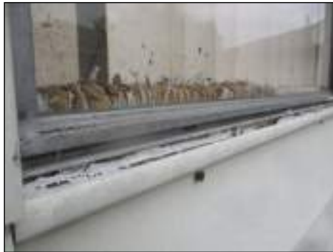
Gaps in siding at joints and around windows/doors - recommend servicing to prevent moisture entry
