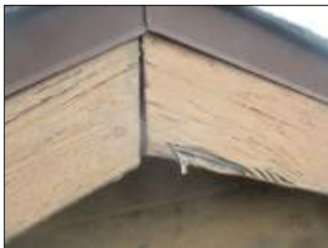
Inspector does not determine wood destroying organism presence or damage - always obtain a structural pest control inspection
