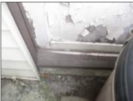
Irregular installation/materials/workmanship - needs to be serviced
