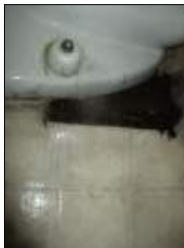
Moisture damaged at jack and Jill bathroom area - needs to be serviced
