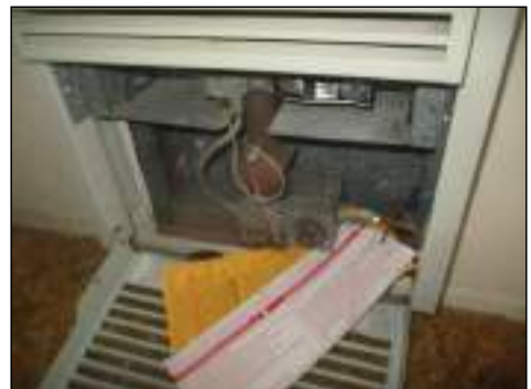
Gas heater located in a bedroom - recommend removal for safety - consult a HVAC contractor to further evaluate
