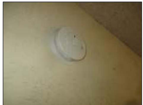
Operational at time of inspection via factory installed test button at rear and bedrooms
