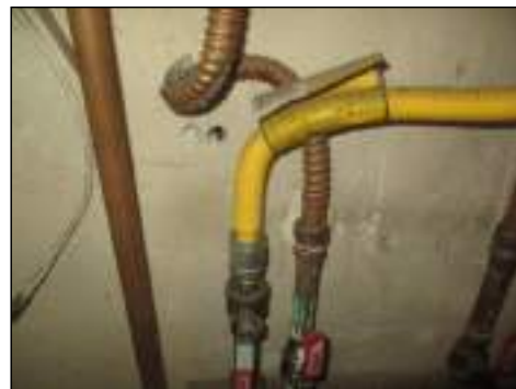
Holes present - needs to be serviced to retain integrity of fire separation
