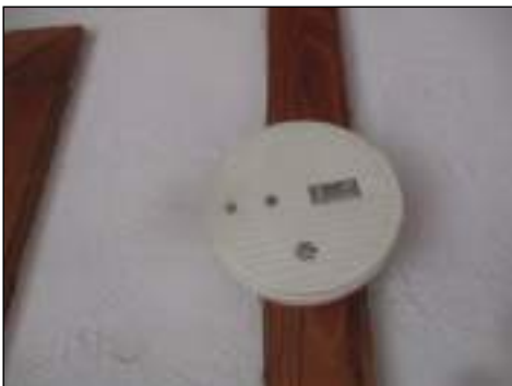
Operational at time of inspection via factory installed test button at rear and bedrooms
