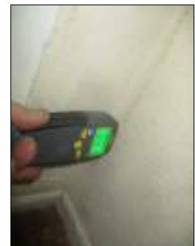
Stains/blistered areas - tested dry with moisture meter/thermal Imaging device at time of inspection - monitor area for moisture
