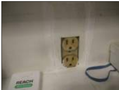
Missing/damaged outlet/switch covers - recommend installation/replacement of all covers for safety
