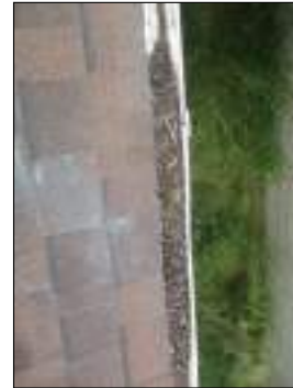
Clogged/restricted by debris in areas - recommend servicing
