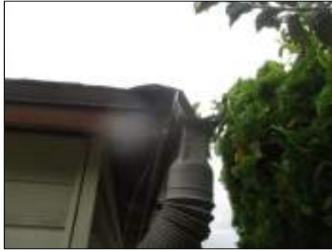
Missing gutter/downspout section(s) - needs to be serviced
