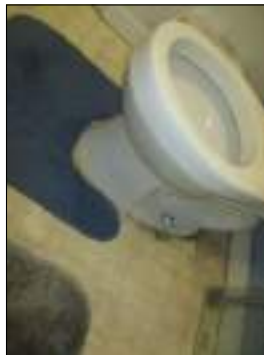
Moisture damaged at jack and Jill bathroom area - needs to be serviced
