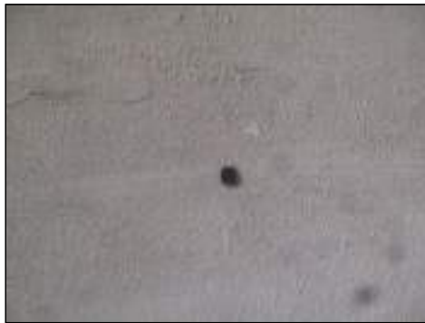
Holes present - needs to be serviced to retain integrity of fire separation
