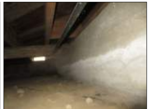
Efflorescence present - indicates past moisture accumulation - monitor for further moisture intrusion
