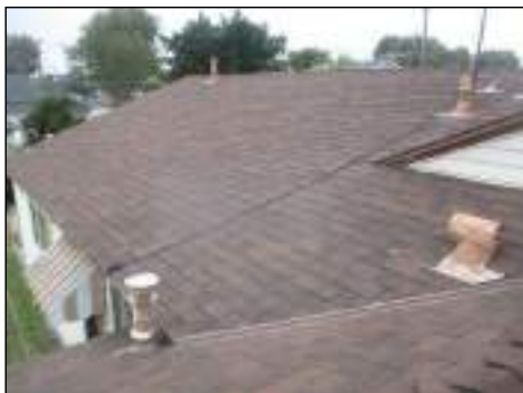
Worn and weathered materials present - typical for age and weather exposure - roof needs maintenance
