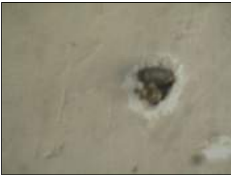
Holes present - needs to be serviced to retain integrity of fire separation
