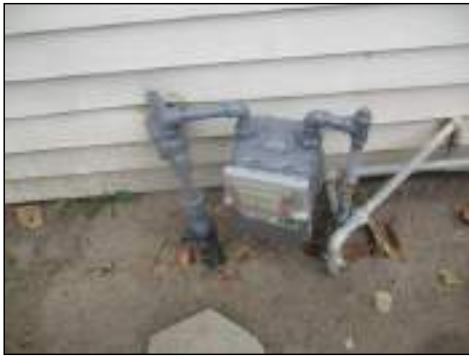
Natural gas present
