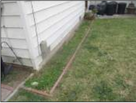
Low spots along the foundation - recommend adding additional backfill to create the proper slope away from the house to allow for effective drainage
