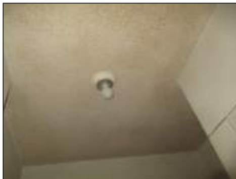
Missing at hall - needs to be installed
