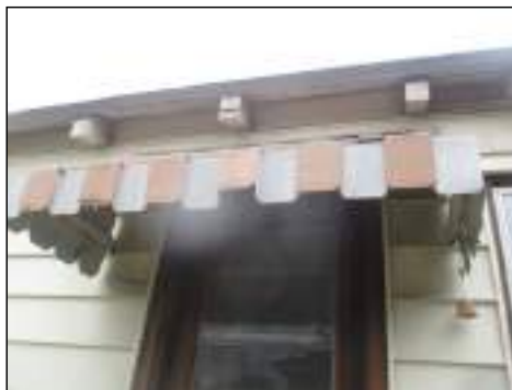
Worn/weathered/stained materials - typical for age - material in need of maintenance
