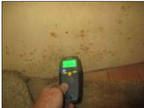
Stains/blistered areas - tested dry with moisture meter/thermal Imaging device at time of inspection - monitor area for moisture
