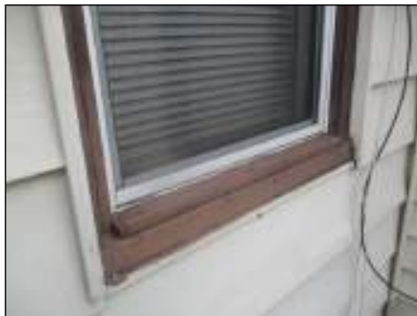
Visible gaps around window frame - recommend exterior water tight sealant to prevent moisture entering the structure
