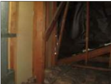
Visible daylight can be seen in areas - recommend contractor to evaluate and seal any holes/gaps
