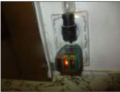
A representative number of receptacles and switches were tested and found to be operational at time of inspection
