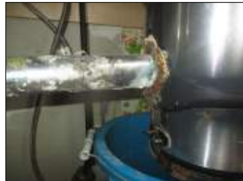
Heavily damaged - needs to be serviced
