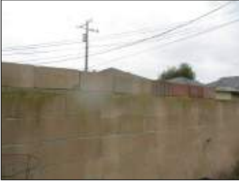
Loose/missing top caps/materials - recommend servicing
