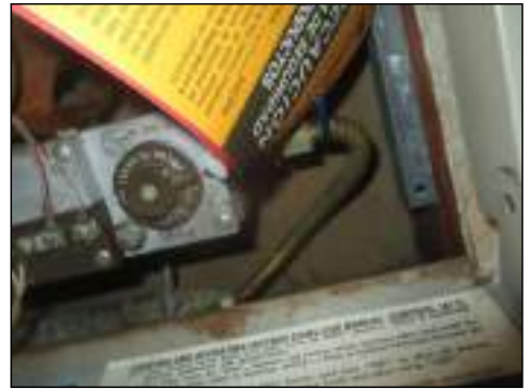
Old brass type gas line present - recommend immediate upgrade
