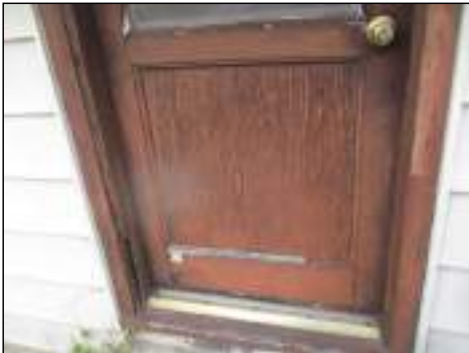
Heavily damaged/deteriorated/peeling - needs to be serviced
