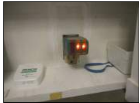
Loose/worn outlets/switches - typical for age consider upgrading
