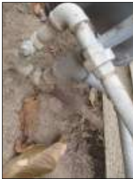
Minor rusting - typical for age - recommend rust treatment
