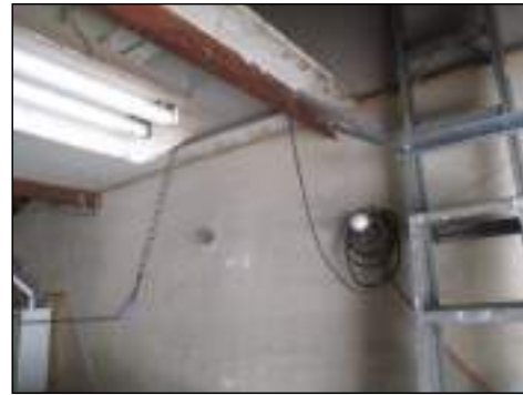
Using extension cord for power - this is not a recommended installation a more permanent installation should be done by a licensed electrician
