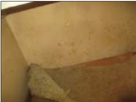
Stains/blistered areas - tested dry with moisture meter/thermal Imaging device at time of inspection - monitor area for moisture
