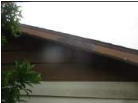
Heavily damaged/deteriorated/peeling - needs to be serviced
