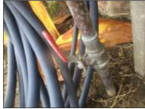
Main valve appears to have normal wear at the time of inspection - no major visible defects
