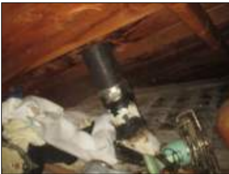
Large stains present on wood members of structure - needs to be serviced and further evaluated for possible leak
