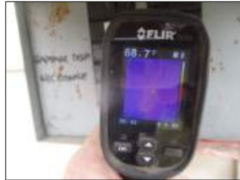
Thermal Image View - Normal temperature readings with no visible signs of overheating at time of inspection
