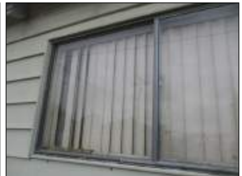
Missing screens - screens are recommended at all openable windows
