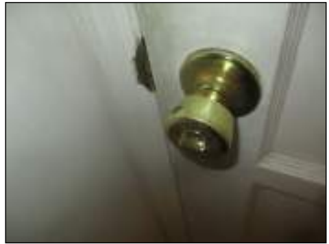
Did not latch properly/sticks at jamb hall bathroom area - recommend servicing
