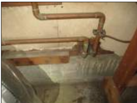
Holes present - needs to be serviced to retain integrity of fire separation
