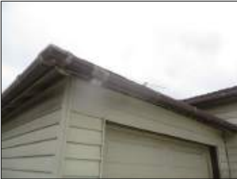
Plastic gutters present - subject to sun damage - recommend cleaning and routine maintenance on gutter system to maintain life expectancy
