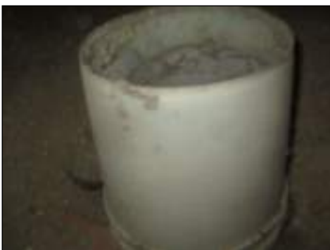
Bathroom or other exhaust fan duct appears to terminate in attic, have duct routed to exterior to minimize moisture
