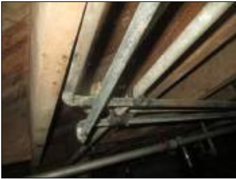
Copper to galvanized plumbing missing proper insulation – needs to be serviced by licensed plumber
