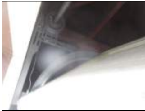
Did not operate properly - needs to be serviced/further evaluated
