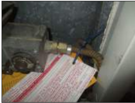
Old brass type gas line present - recommend immediate upgrade
