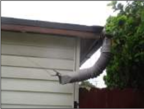
Missing gutter/downspout section(s) - needs to be serviced
