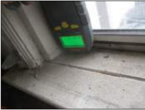
Stains/blisters at sill - tested dry for moisture at the time of the inspection - monitor the areas for moisture intrusion
