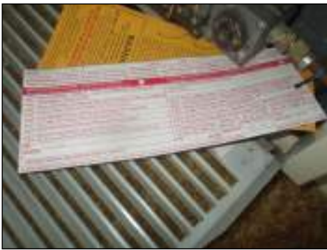
Red-tagged by gas company - needs to be serviced/evaluated by HVAC contractor
