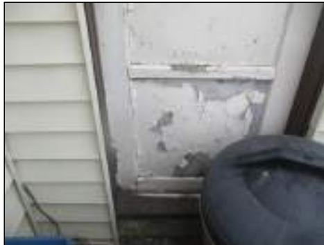
Heavily damaged/deteriorated/peeling - needs to be serviced
