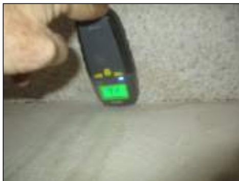
Stains/blistered areas - tested dry with moisture meter/thermal Imaging device at time of inspection - monitor area for moisture
