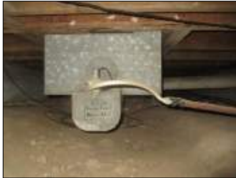
Aluminum gas line is present - immediate upgrade to appropriate flexible gas line is recommended
