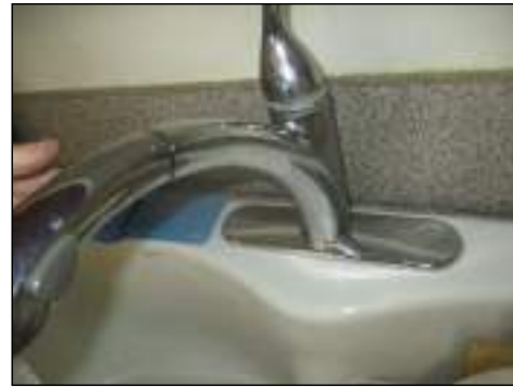
Fixture seized/stuck in position - not functional - recommend service
