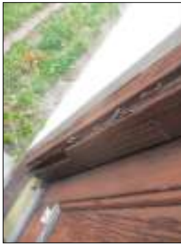
Visible gaps around the door frame - missing weather stripping or damaged - recommend exterior water tight service to prevent possible moisture intrusion
