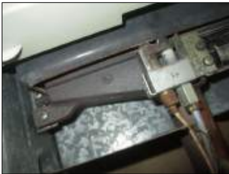
Pilot not lit could not test - needs to be serviced
