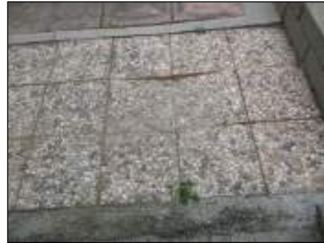
Walkway displacement/uplifted/uneven areas - potential trip hazard - needs to be serviced
