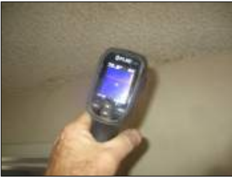
Stains/blistered areas - tested dry with moisture meter/thermal imaging device at time of inspection - monitor area for moisture
