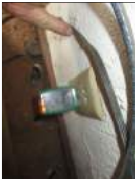
A representative number of receptacles and switches were tested and found to be operational at time of inspection
