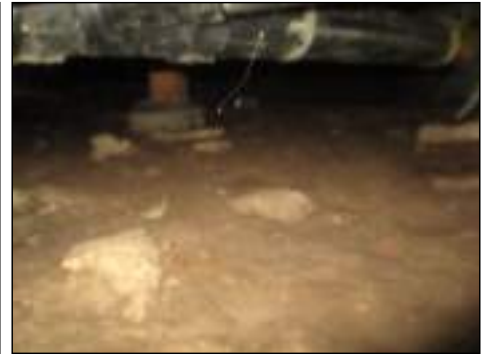
Moisture present under structure at rear addition area - needs to be serviced
