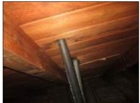
Large stains present on wood members of structure - needs to be serviced and further evaluated for possible leak
