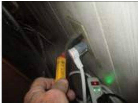
Worn/loose outlets/switches - typical for age consider upgrading
