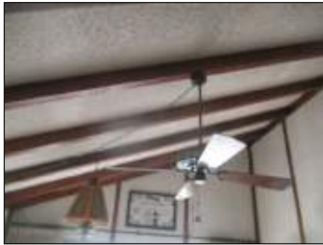
Improper electrical installation - needs to be serviced/further evaluated
