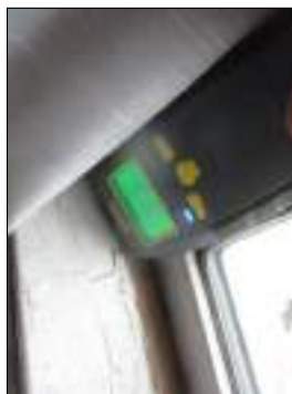
Stains/blisters at sill - tested dry for moisture at the time of the inspection - monitor the areas for moisture intrusion
