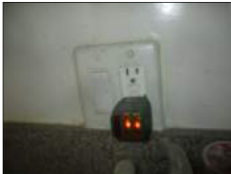
A representative number of receptacles and switches were tested and found to be operational at time of inspection
