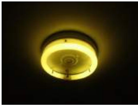
Missing fixture globes or covers
