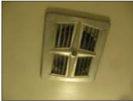
Exhaust fan did not operate at hall - needs to be serviced
