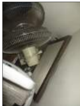
Floor heater is very old/worn - these types of heating systems are considered out dated - consider upgrading the heating system for this structure
