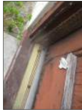
Visible gaps around the door frame - missing weather stripping or damaged - recommend exterior water tight service to prevent possible moisture intrusion
