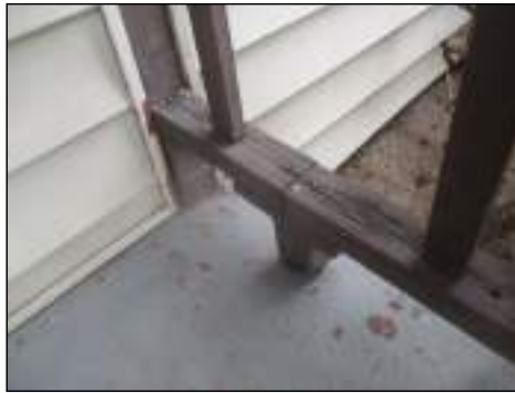
Deteriorated wood - needs to be serviced - consult termite report
