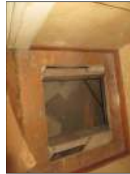
Irregular installation/workmanship - needs to be serviced
