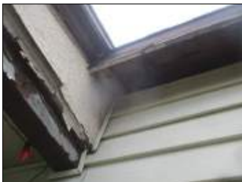
Water stains at fascia/eaves may indicate roof leakage - recommend further evaluation
