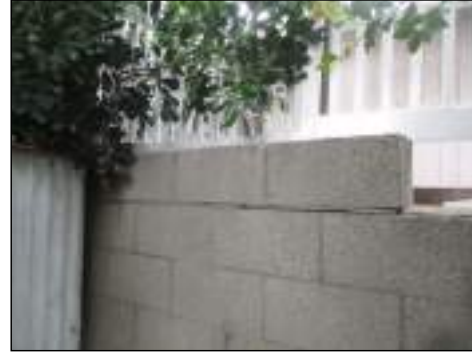
Small cracking/chipping - did not affect the performance of the fence - monitor for further cracking and repair as needed
