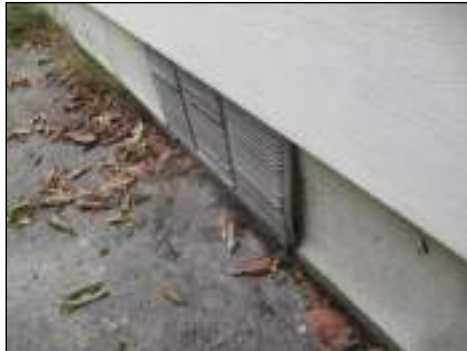
Loose screens - recommend maintenance and repairs to prevent pest intrusion
