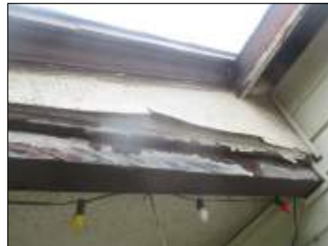
Heavily damaged/deteriorated/peeling - needs to be serviced
