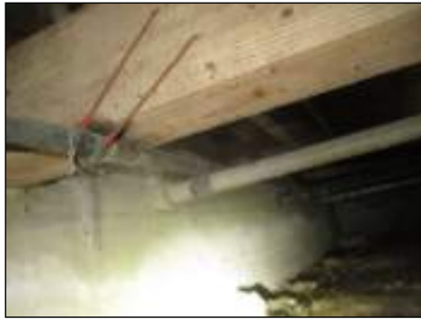
Copper to galvanized plumbing missing proper insulation – needs to be serviced by licensed plumber
