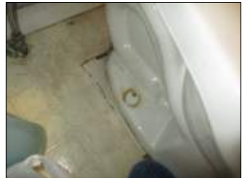
Moisture damaged at jack and Jill bathroom area - needs to be serviced
