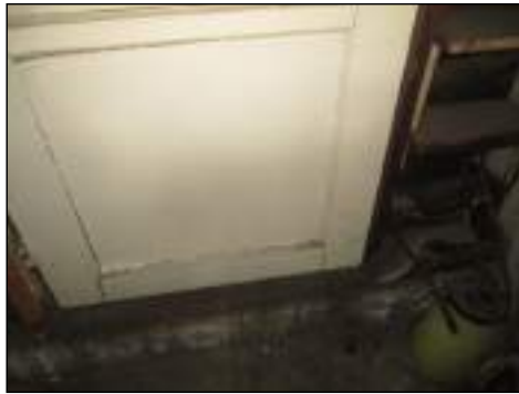
Evidence of moisture entering - needs to be serviced
