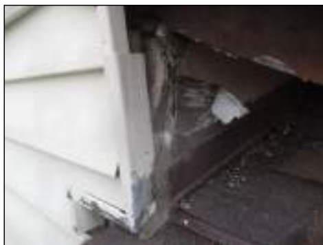
Gaps in siding at joints and around windows/doors - recommend servicing to prevent moisture entry
