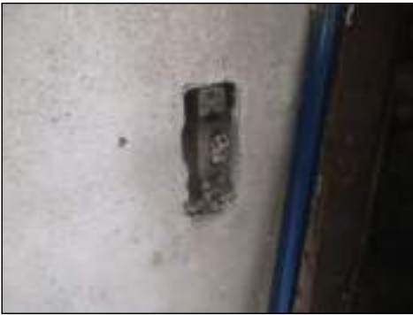
Missing/damaged outlet/switch cover - recommend installation of all covers for safety
