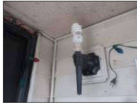
Missing fixture globe(s)
