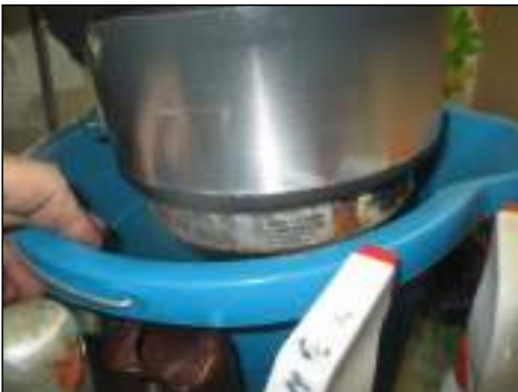
Evidence of leakage observed under sink - needs to be serviced - hidden defects may exist
