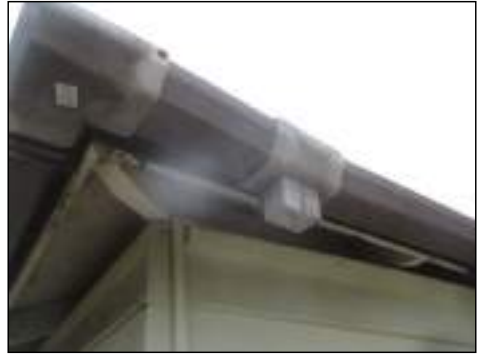
Missing gutter/downspout section(s) - needs to be serviced
