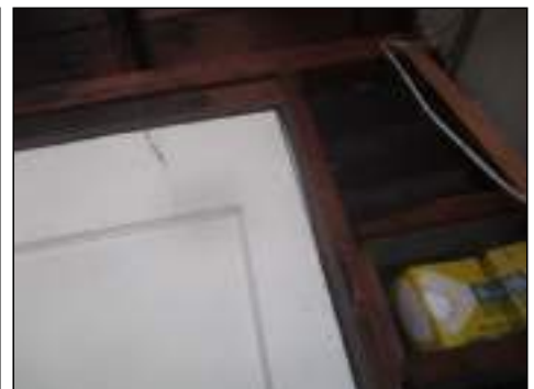
Sticks at jamb - needs to be serviced
