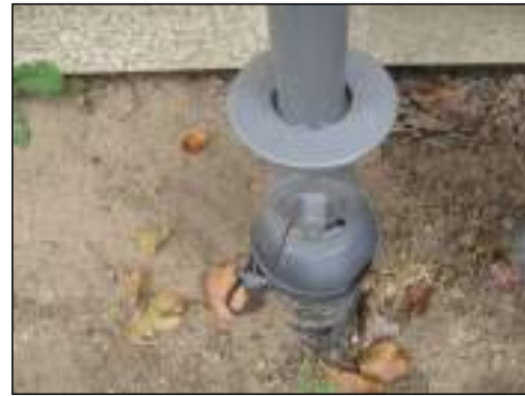
Valve has normal wear for age at the time of inspection - no major visible defects
