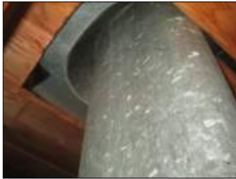
Heat exhaust vent does not have proper clearance from combustibles - needs to be serviced
