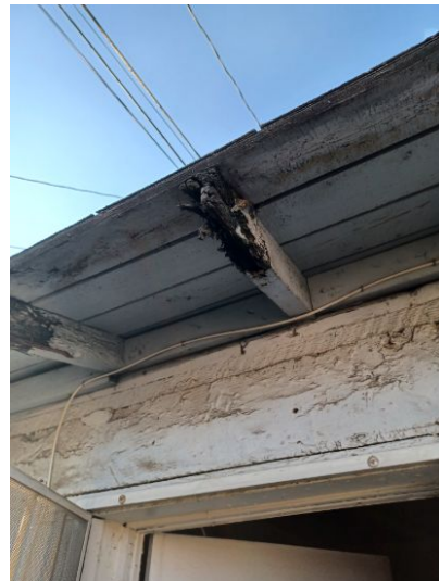
The rafter tails are deteriorated. (Back House)
