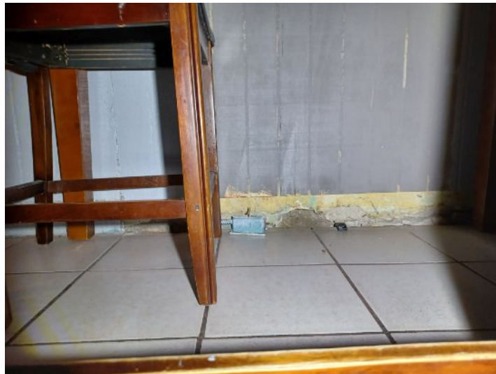
The baseboard is missing. front
