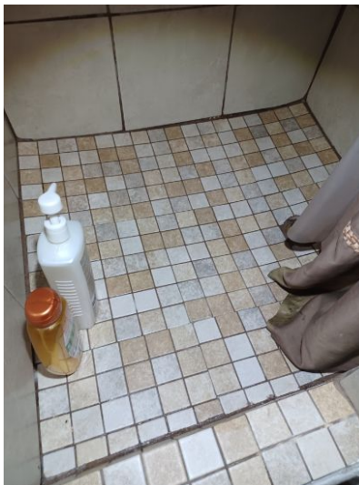
Shower pan installed poorly.
