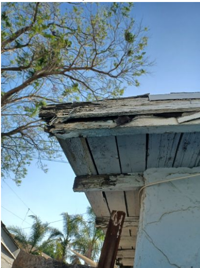
The fascia is damaged. (Back House)
