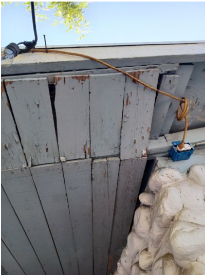
The surfaces are weathered and have peeling paint.
