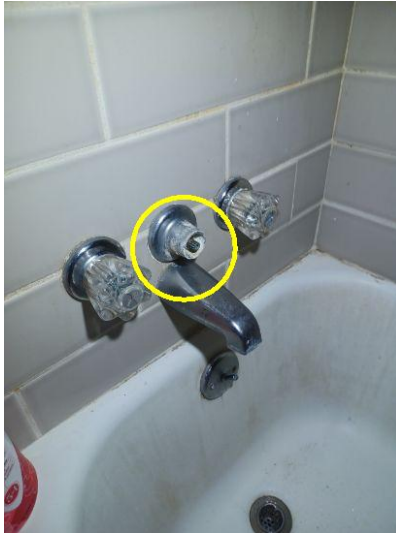
Handle is missing to one faucet
