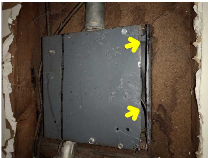
The exterior cover for the main electrical panel is damaged, and should be replaced by a qualified tradesperson.
