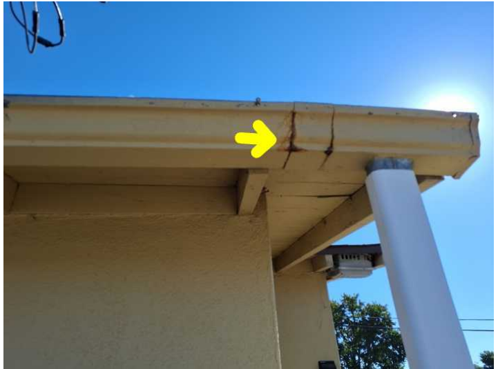
The gutters need to be serviced, such as reconnecting, sealing separated seams, cleaning, or making sure they are secure.
