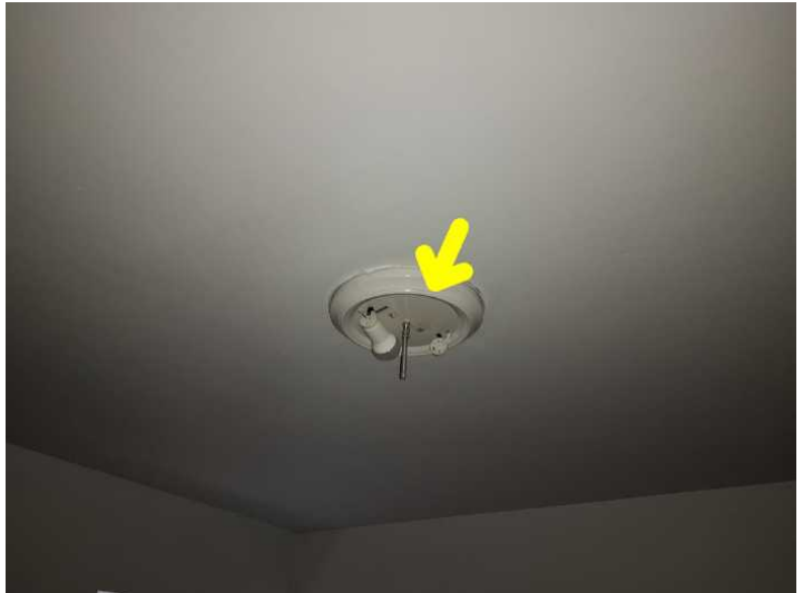
A light cover or globe is missing and should be installed.
