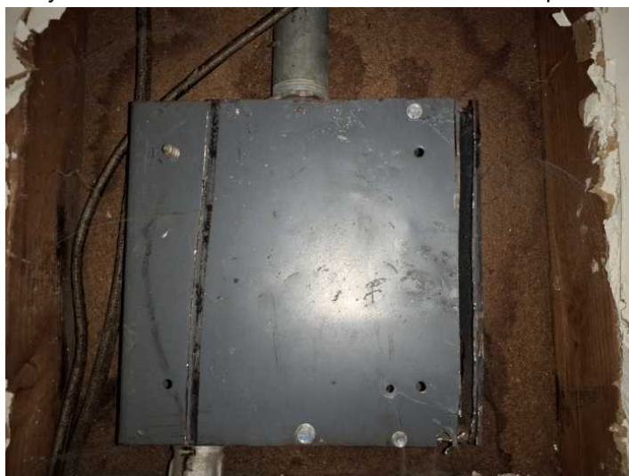
The panel does not have a main disconnect, which is required by current standards. We recommend an evaluation by a qualified electrical contractor and service as necessary,
