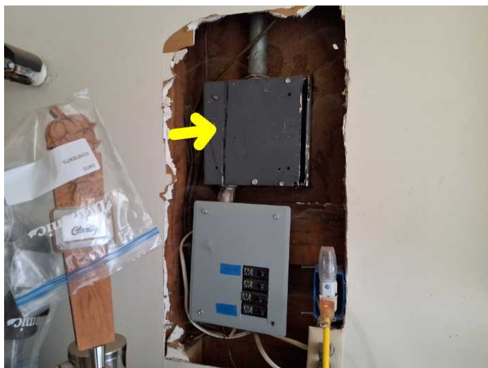
The residence is served by a main electrical panel located within the laundry room.
