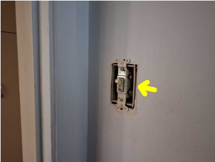
One or more light switch covers are missing and should be installed.
