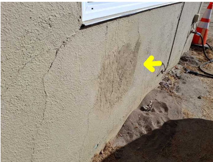
There are stucco patches or repairs that should be explained by the sellers.
