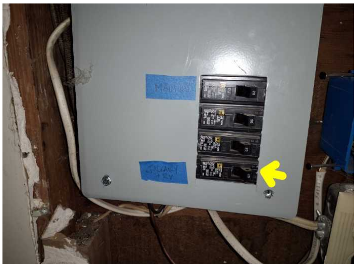
One or more of the breakers do not properly fit within the buss bar. Because of this the breaker is loose, which can cause arcing and should be evaluated and serviced by a qualified electrical contractor.
