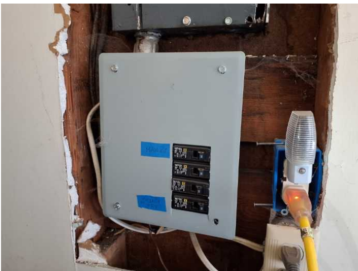
The sub panel is located adjacent to the main panel.
