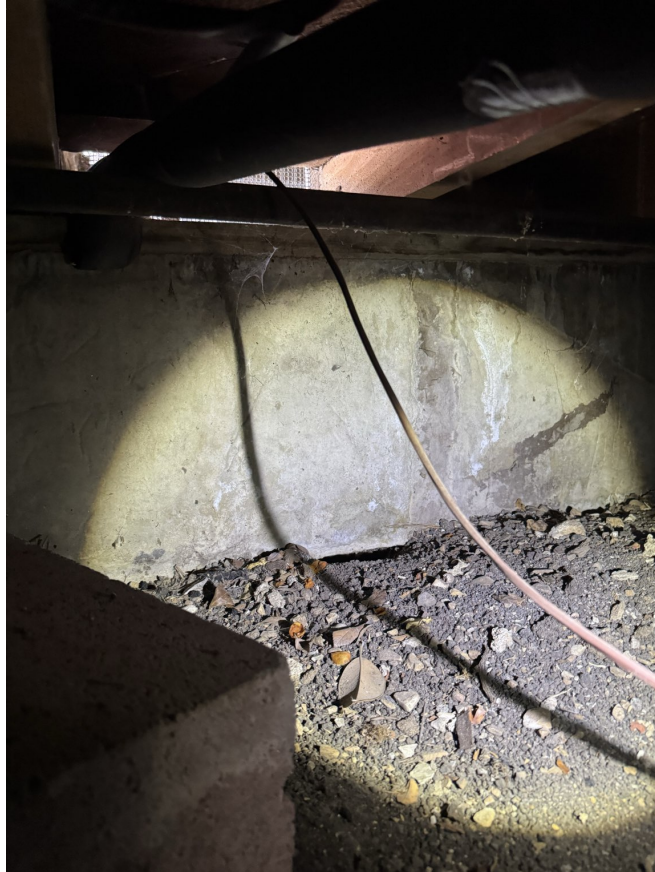
Exposed soil under foundation beam
