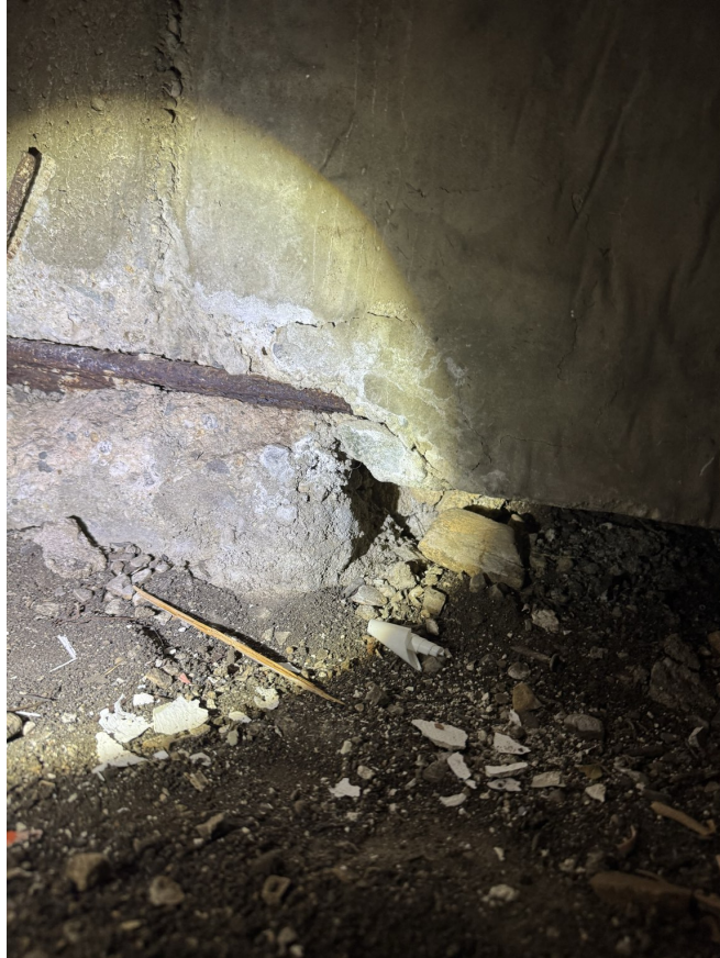
Exposed rusted rebar
