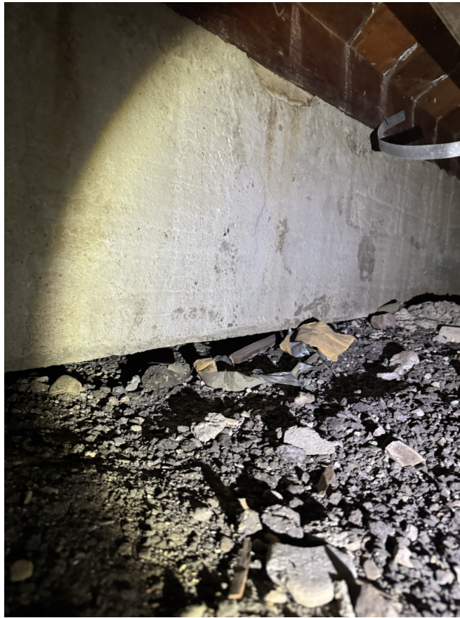
Exposed soil under foundation beam
