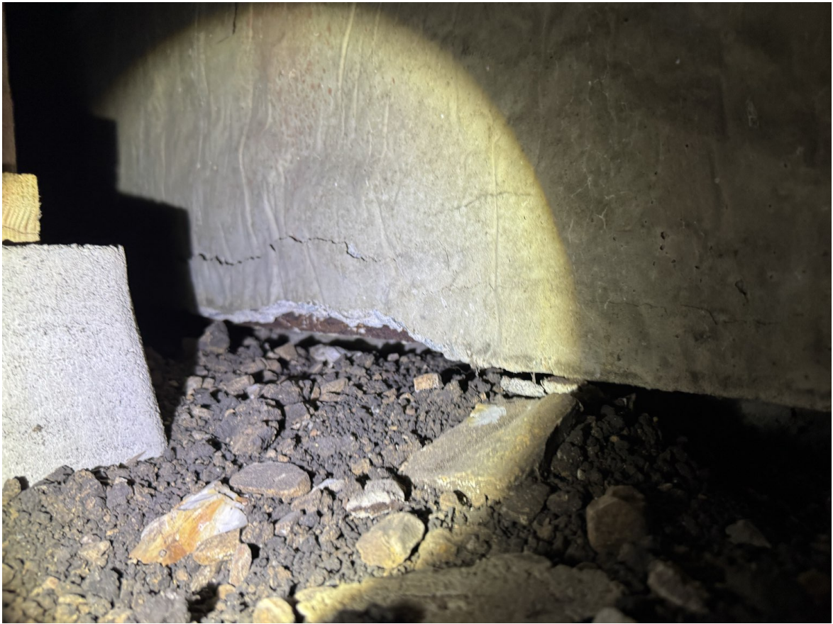
Exposed soil under foundation beam and exposed rebar
