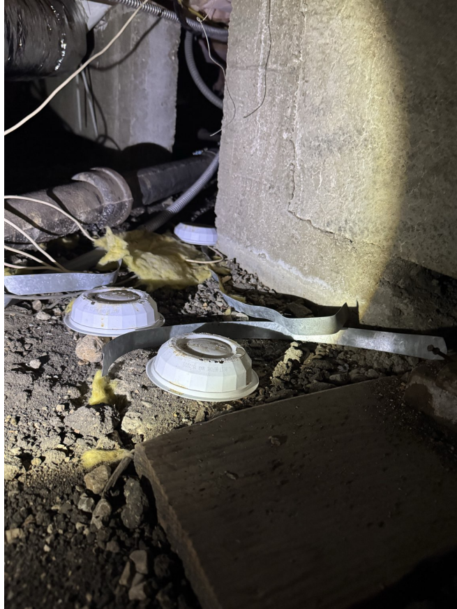
Debris in crawlspace
