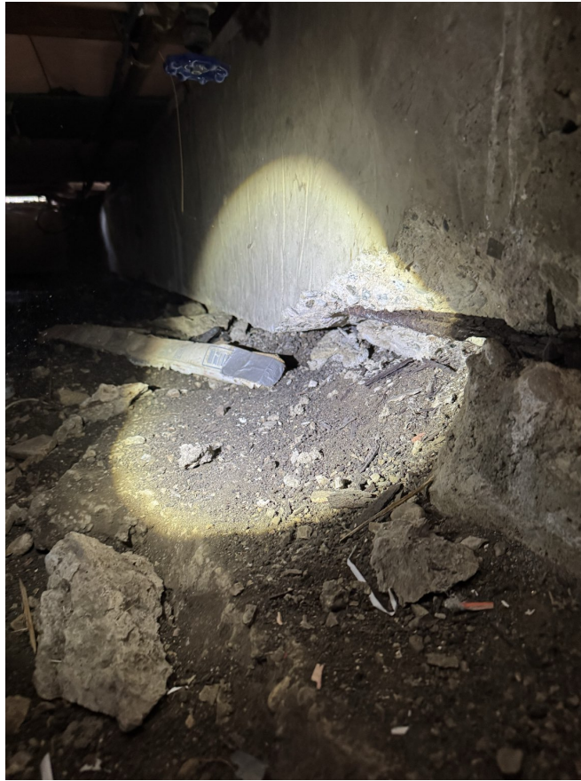
Exposed rusted rebar
