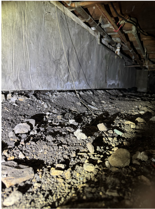
Exposed soil under foundation beam
