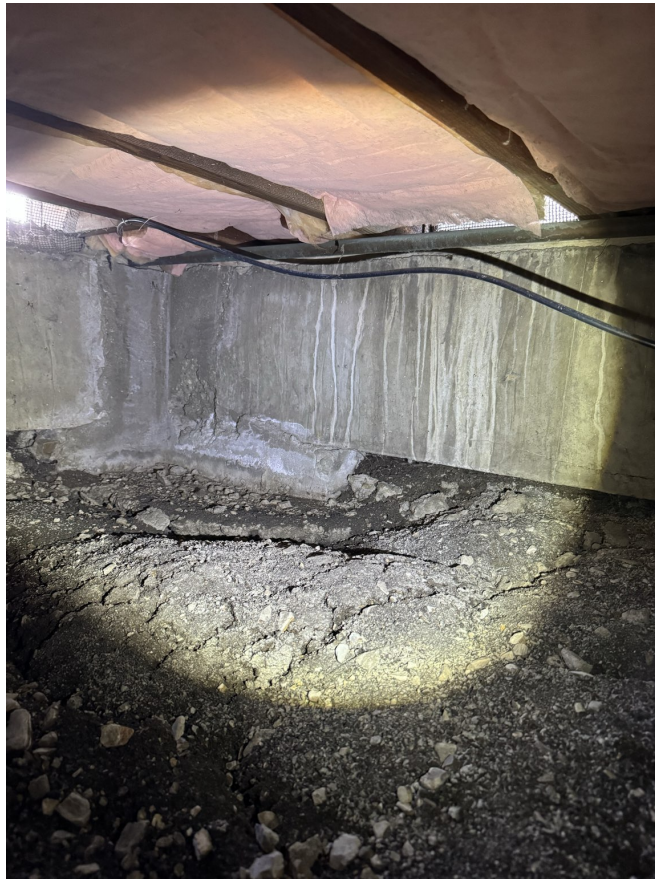
Exposed soil under foundation beam
