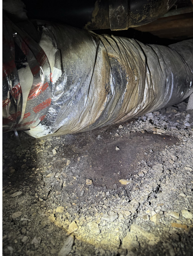
Evidence of server leak
