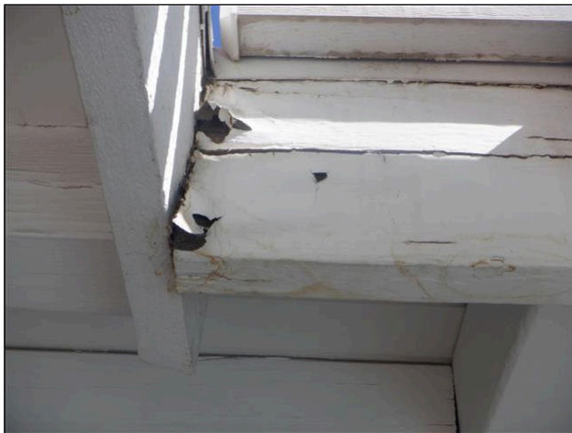
2.4 Item 2(Picture) Damaged Wood
