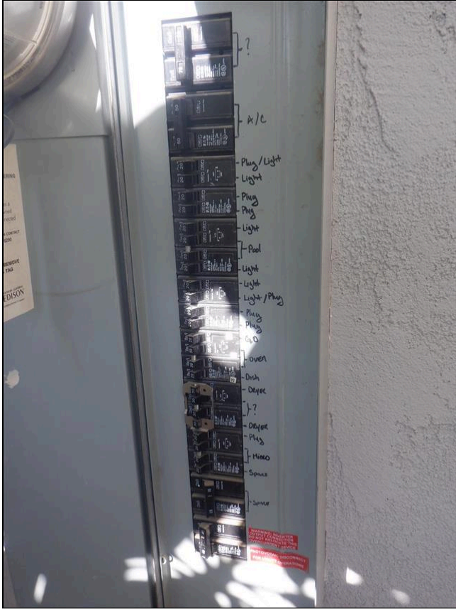
9.1 Item 3(Picture) Electrical Panel Distribution
