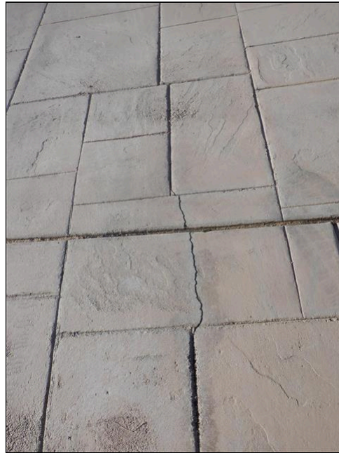
2.3 Item 2(Picture) Driveway Cracks
