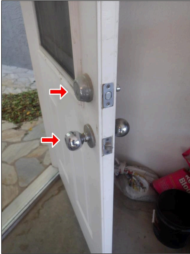
3.6 Item 5(Picture) Locks Not Functioning
