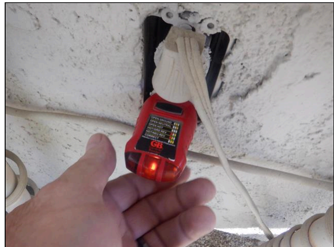
2.6 Item 2(Picture) Outlet No GFCI Protection
