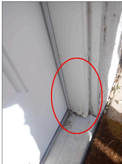
3.6 Item 4(Picture) Failing Trim Paint
