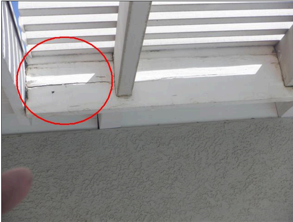
2.4 Item 1(Picture) Damaged Wood
