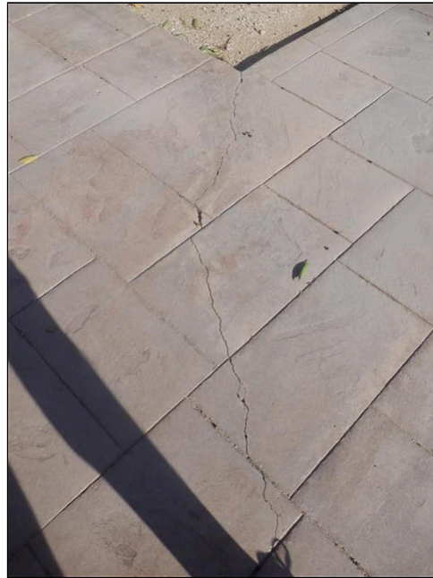
2.3 Item 6(Picture) Driveway Cracks
