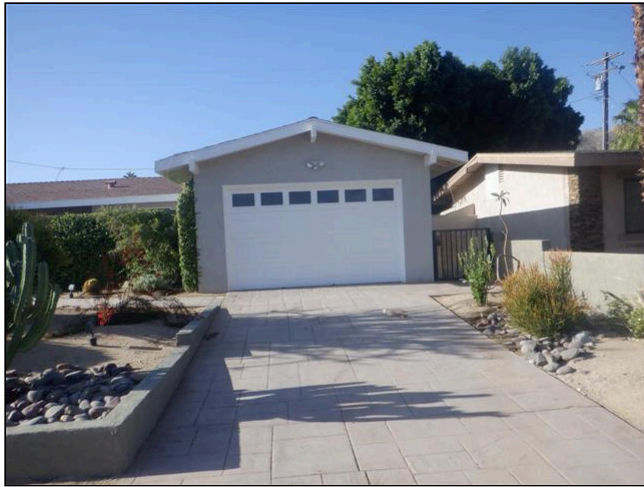
2.3 Item 1(Picture) Driveway Cracks
