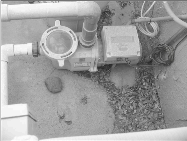
11.28 Item 1(Picture) :Pool Pump No GFCI Protection
