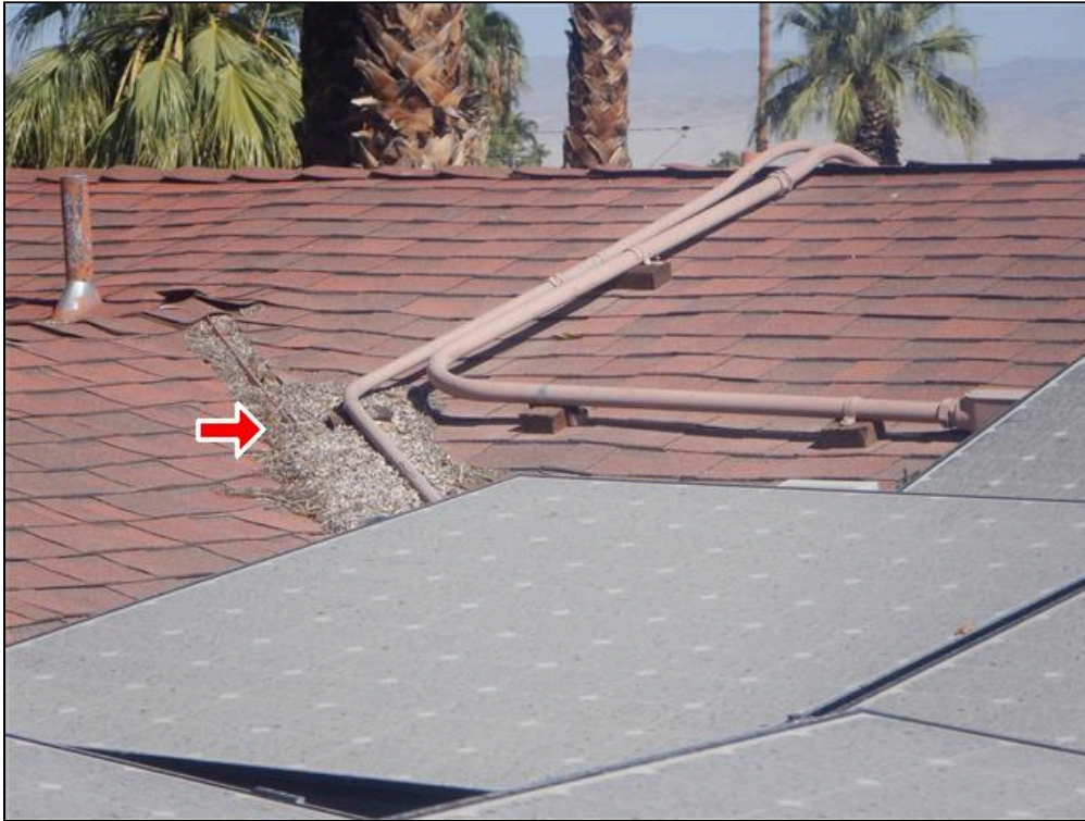
1.6 Item 3(Picture) Roof Debris
