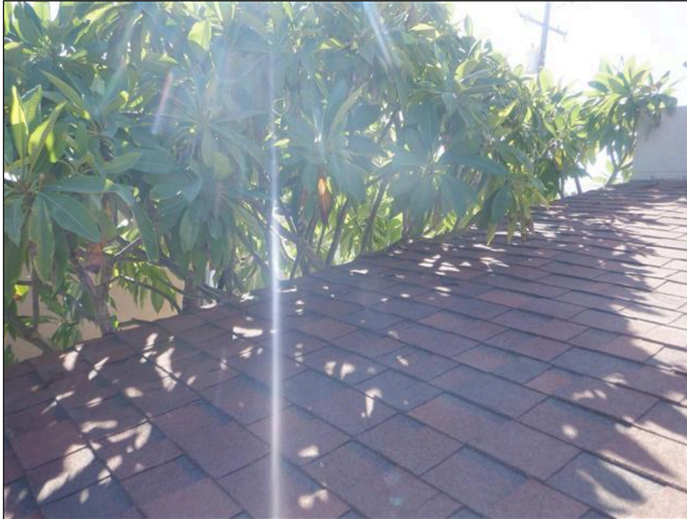
1.6 Item 1(Picture) Roof Tree Contact
