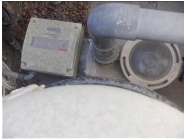
11.18 Item 1(Picture) Pool Pump
