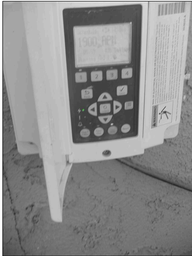
11.29 Item 1(Picture) Pump Controls
