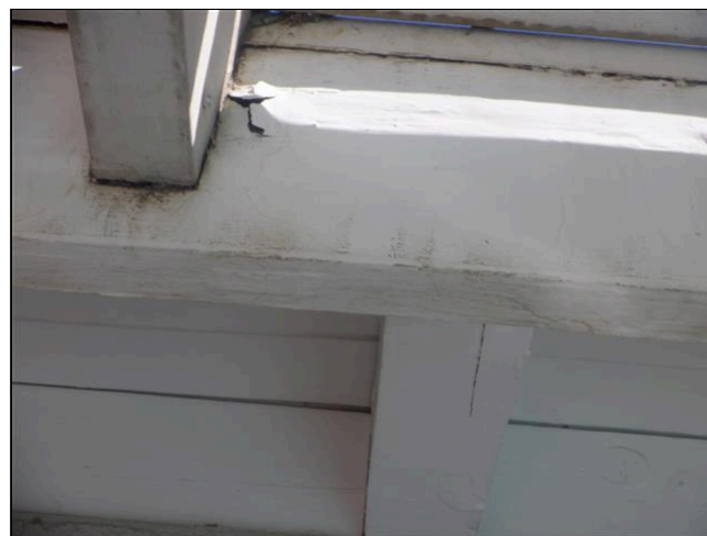
2.4 Item 3(Picture) Damaged Wood
