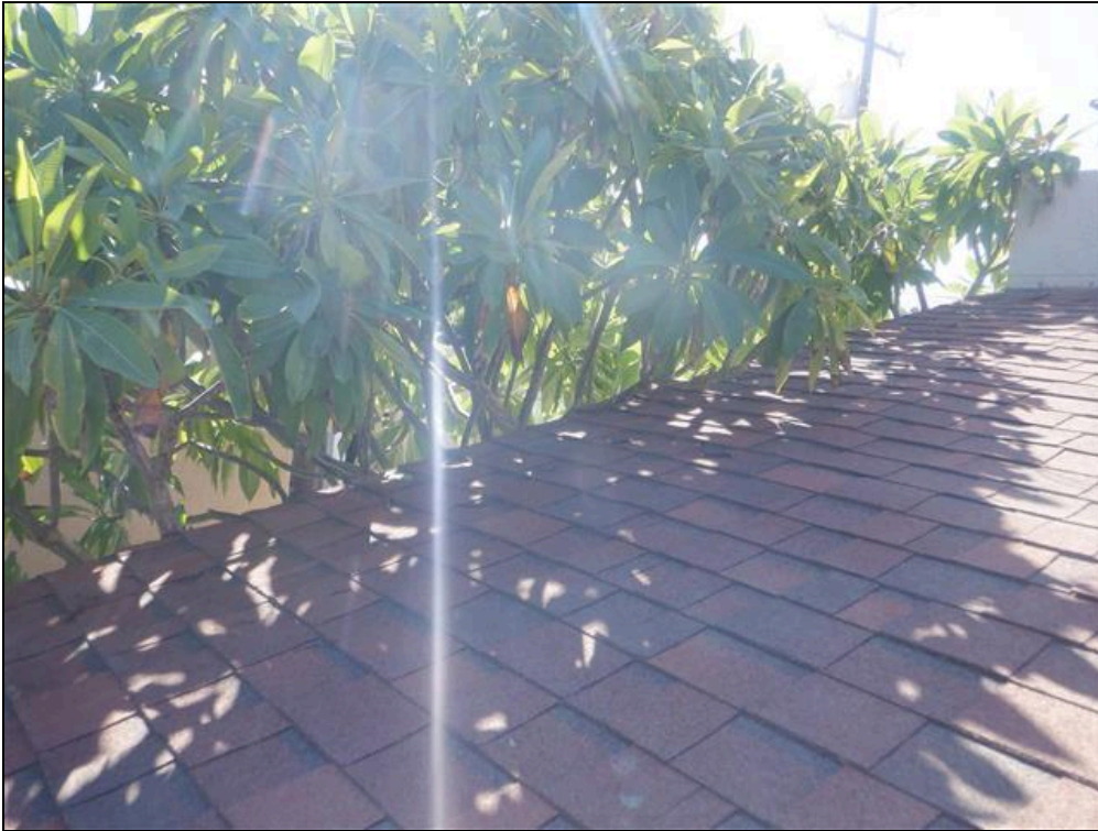
1.6 Item 1(Picture) Roof Tree Contact
