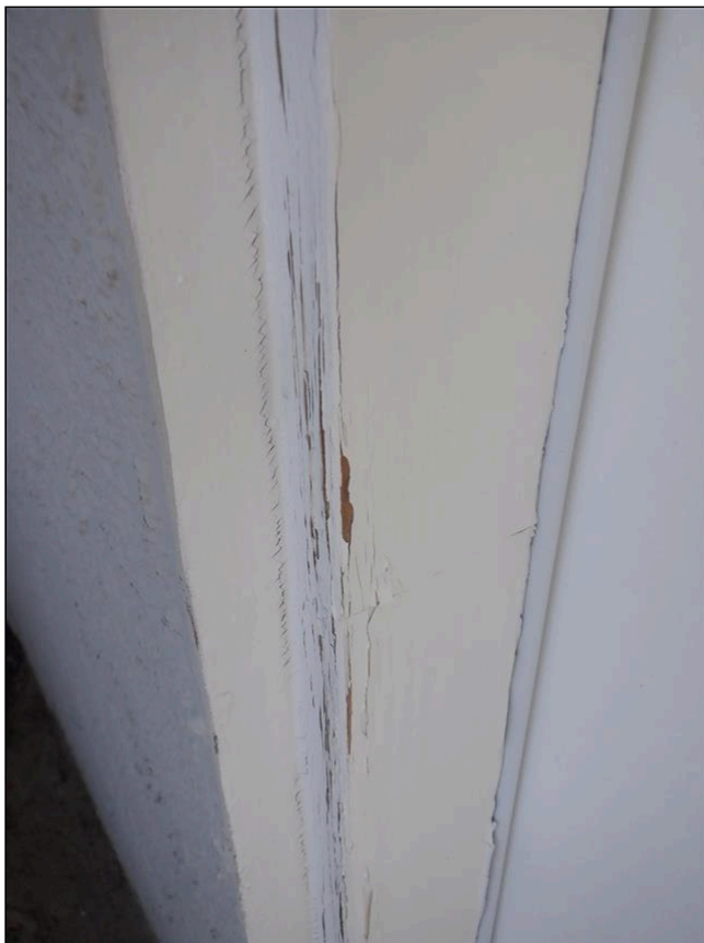
3.6 Item 3(Picture) Failing Trim Paint
