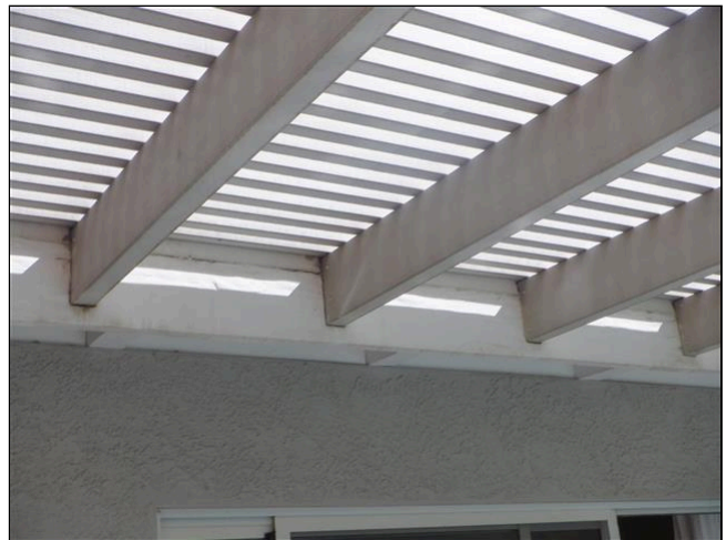
2.4 Item 6(Picture) Failing Paint
