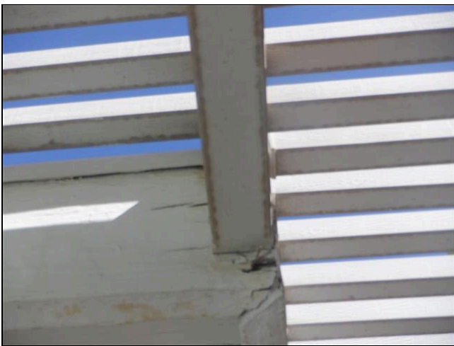
2.4 Item 5(Picture) Failing Paint
