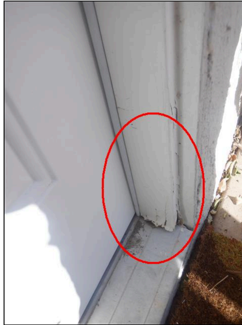
3.6 Item 4(Picture) Failing Trim Paint
