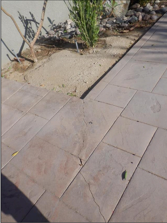
2.3 Item 5(Picture) Driveway Cracks
