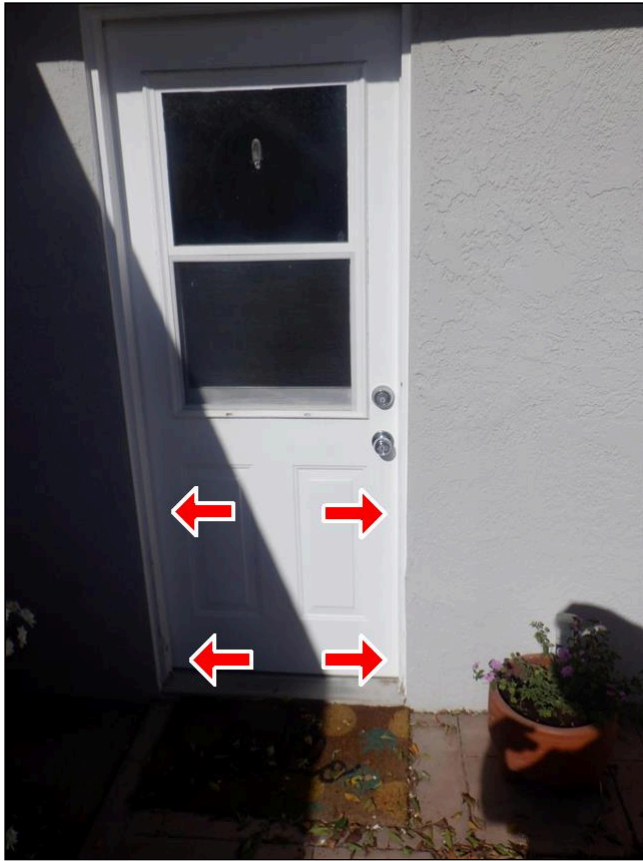
3.6 Item 1(Picture) Failing Trim Paint
