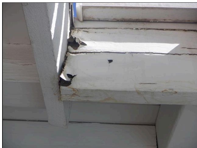
2.4 Item 2(Picture) Damaged Wood
