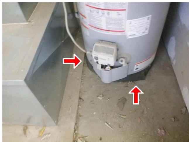
8.2 Item 5(Picture) Water Heater Missing Catch Pan
