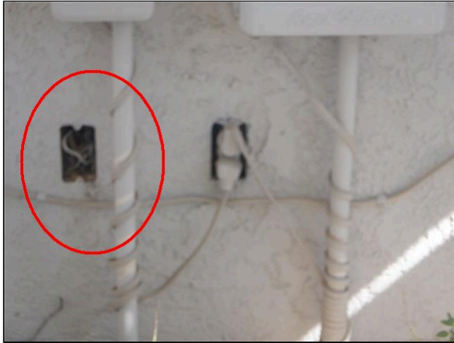
2.12 Item 1(Picture) Missing Cable Box Cover
