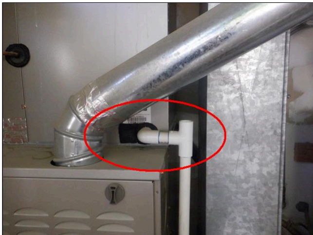
10.0 Item 4(Picture) Heating Unit Missing Condensate Safety Switch
