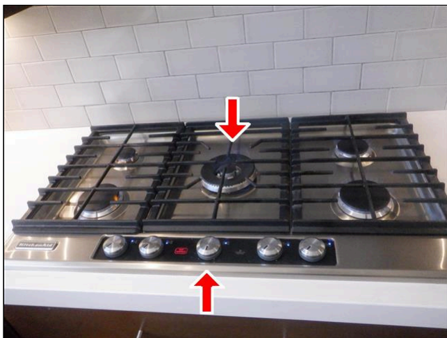
4.9 Item 1(Picture) Center Burner/Igniter
