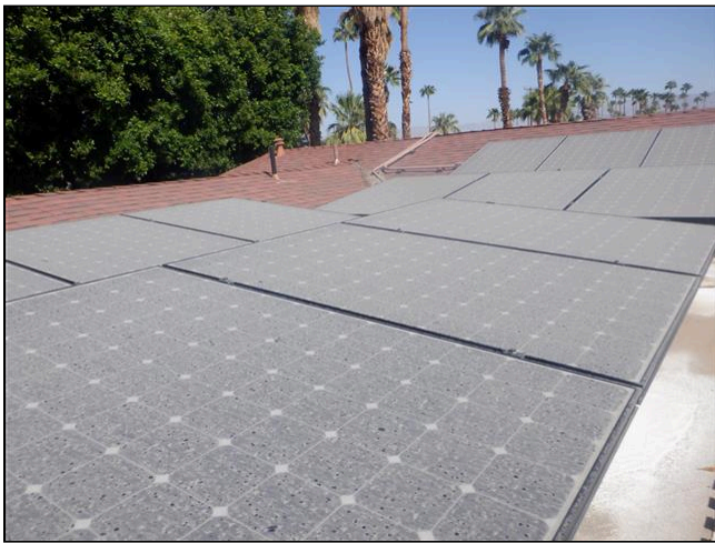
1.8 Item 1(Picture) Solar Panels
