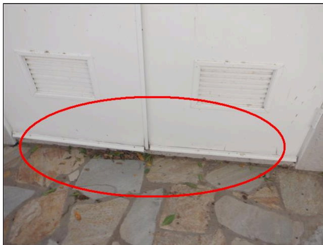
2.1 Item 2(Picture) Utility Room Doors Weathered
