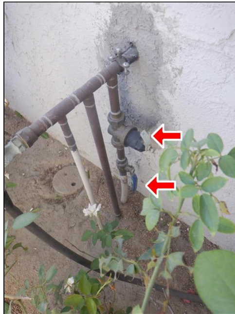
8.5 Item 1(Picture) Main Water Shut Off/Regulator
