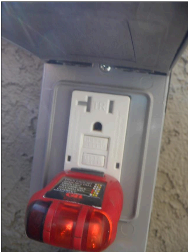
11.17 Item 1(Picture) Pool Light GFCI
