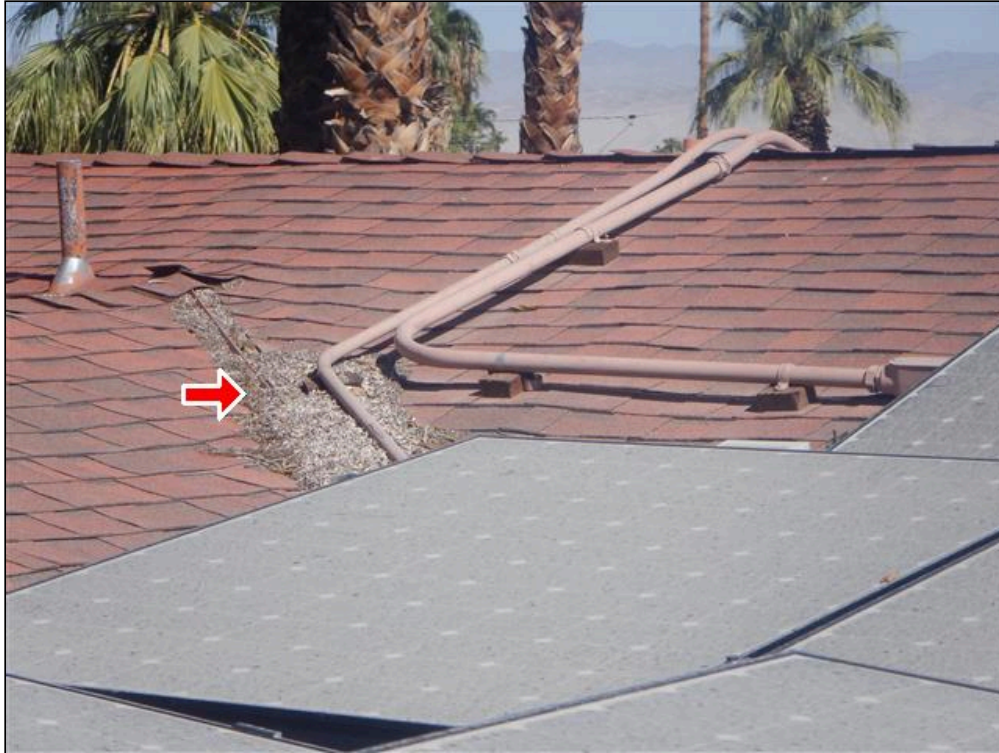
1.6 Item 3(Picture) Roof Debris
