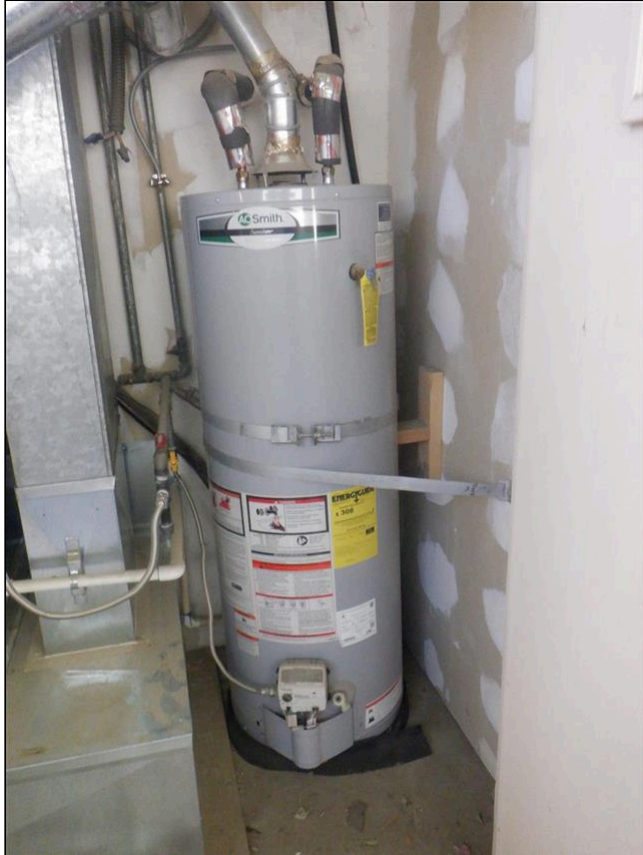
8.2 Item 1(Picture) Water Heater
