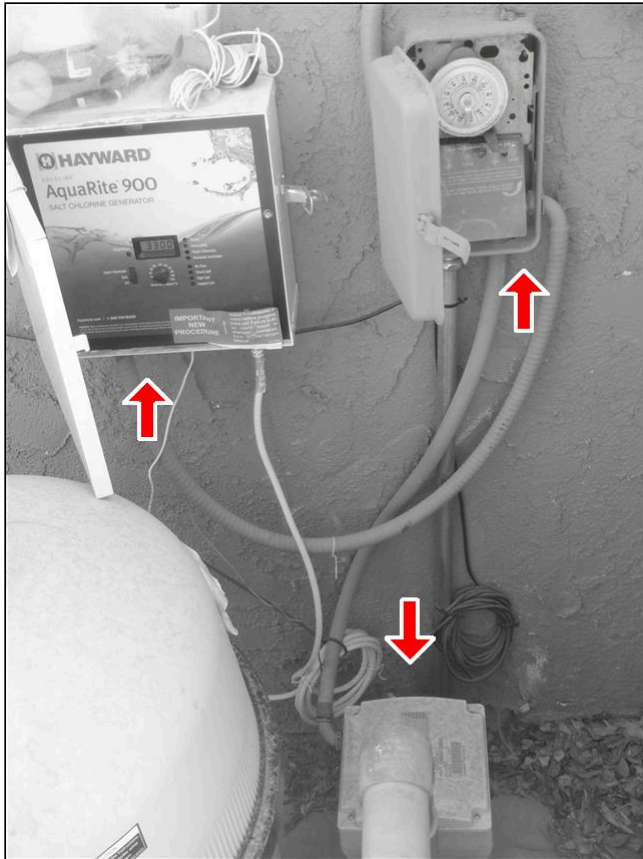
11.27 Item 1(Picture) Pool Equipment No Bond Wire Present
