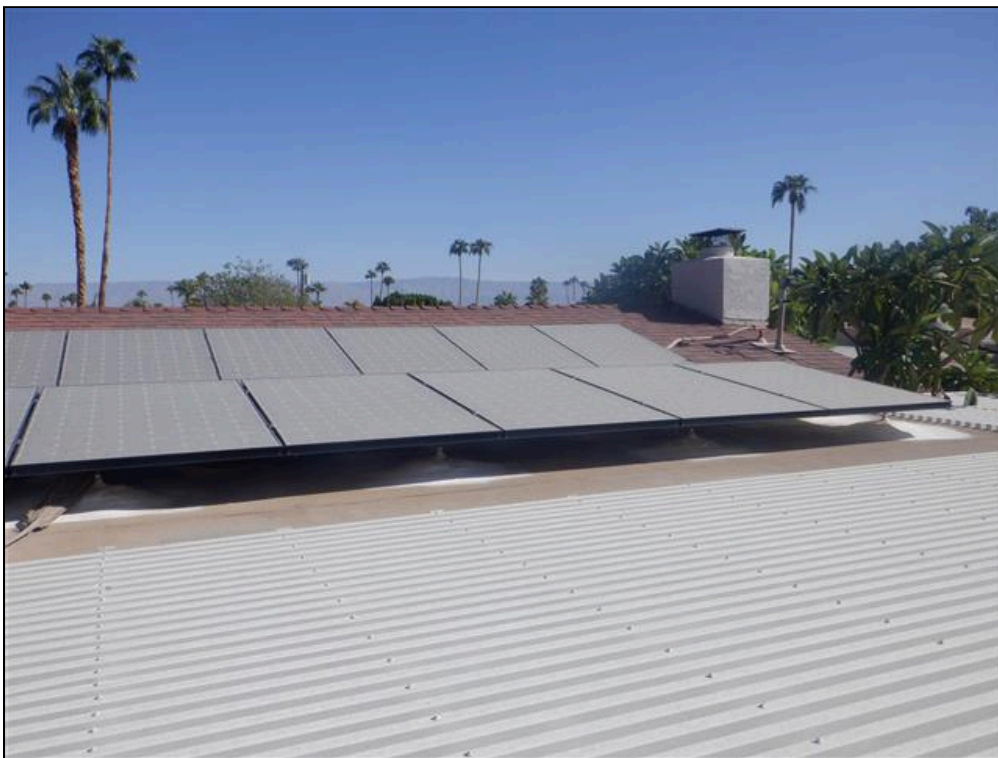
1.8 Item 2(Picture) Solar Panels
