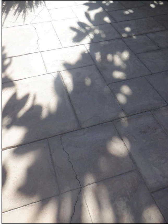
2.3 Item 9(Picture) Patio Cracks
