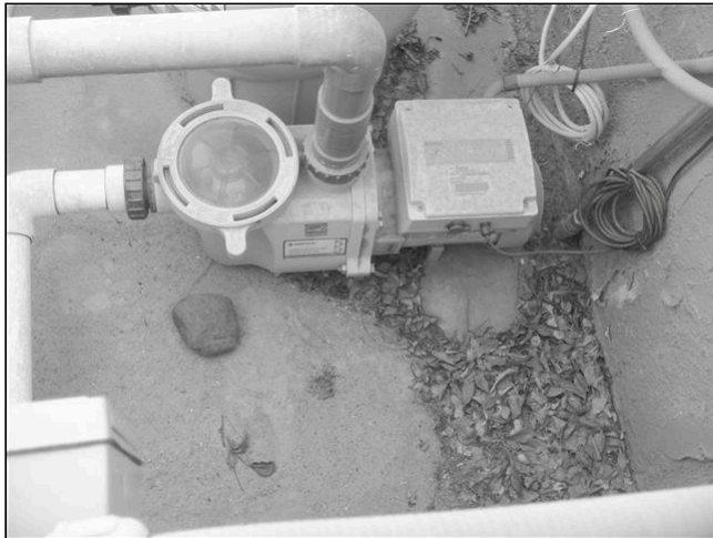
11.28 Item 1(Picture) :Pool Pump No GFCI Protection
