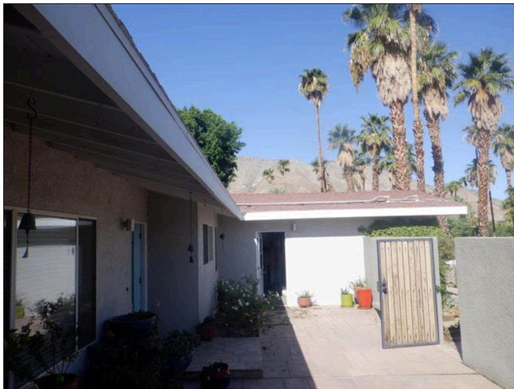
2.3 Item 11(Picture) Rain Gutters Needed
