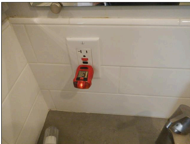
6.5.A Item 1(Picture) GFCI Not Functioning Properly
