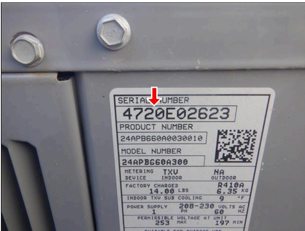
10.6 Item 2(Picture) Cooling Unit
