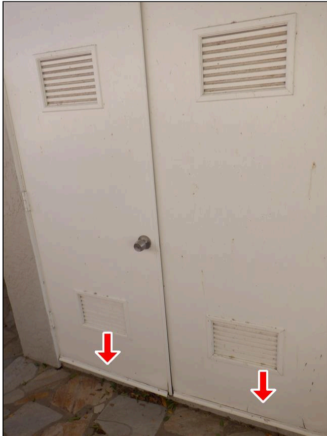
2.1 Item 1(Picture) Utility Room Doors Weathered
