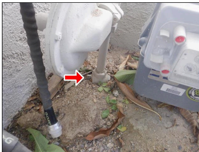
8.6 Item 1(Picture) Main Gas Shut Off
