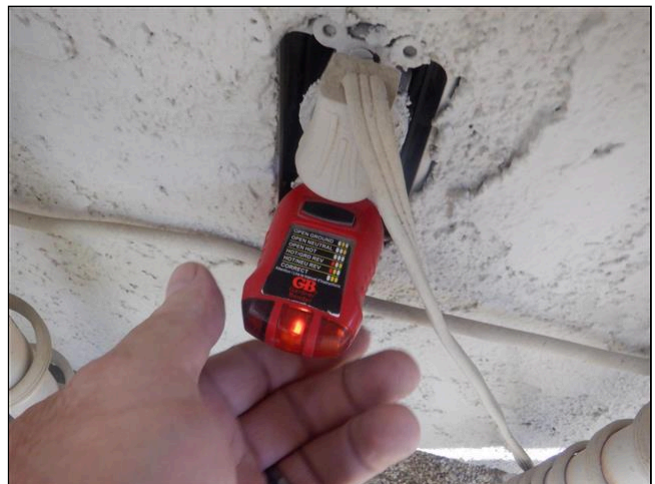
2.6 Item 2(Picture) Outlet No GFCI Protection
