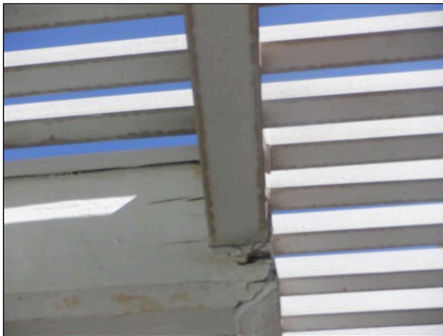
2.4 Item 5(Picture) Failing Paint
