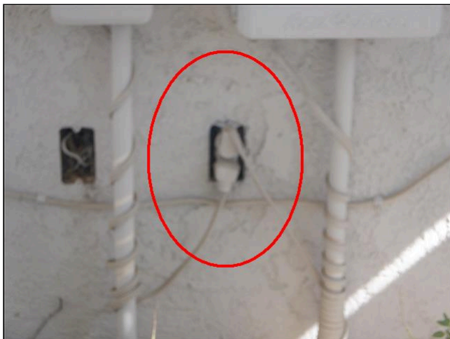
2.6 Item 1(Picture) Outlet No GFCI Protection
