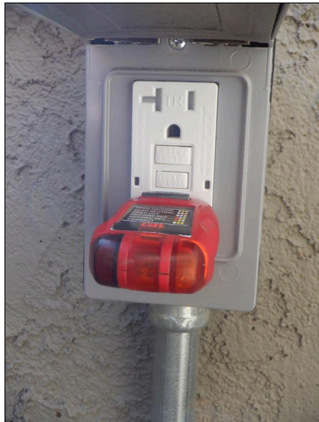
11.17 Item 2(Picture) Pool Light GFCI Functioning Properly
