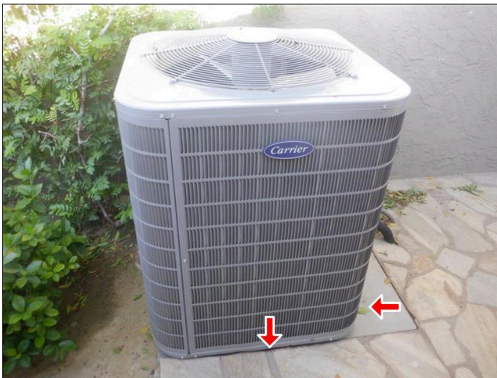
10.6 Item 1(Picture) Cooling Unit Not Secured
