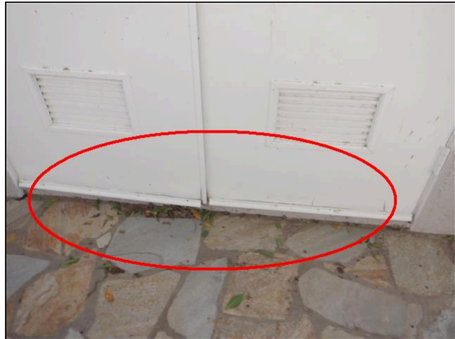
2.1 Item 2(Picture) Utility Room Doors Weathered
