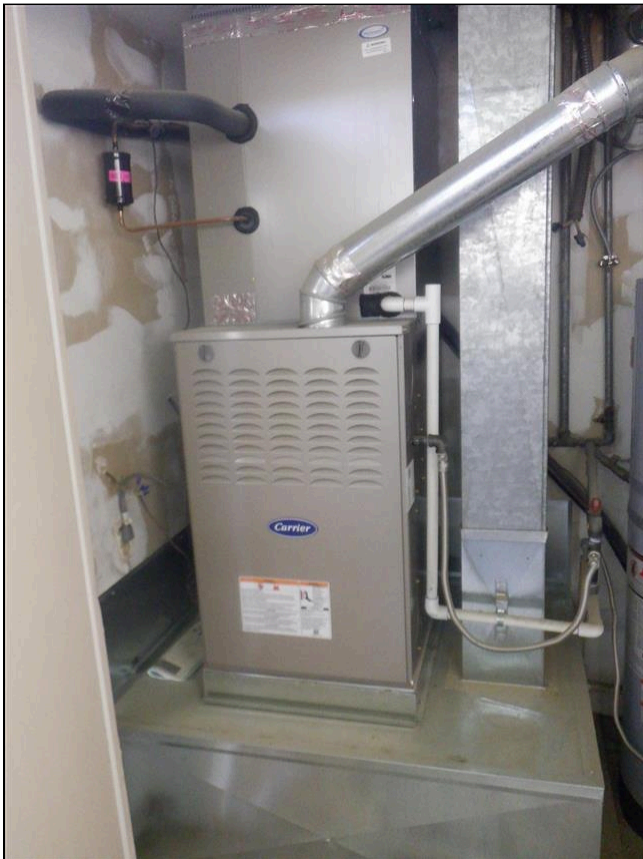
10.0 Item 1(Picture) Heating Unit
