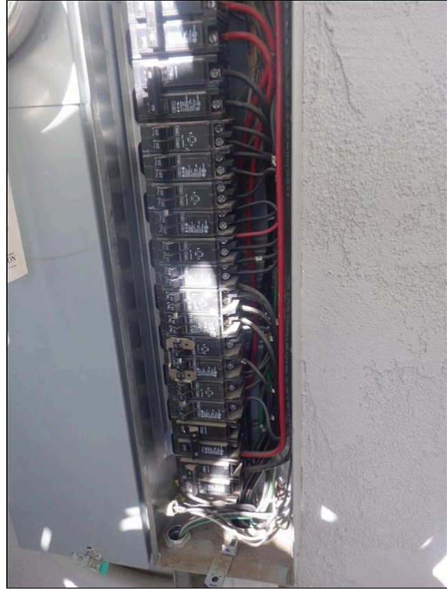
9.1 Item 4(Picture) Electrical Panel Breakers/ Conductors
