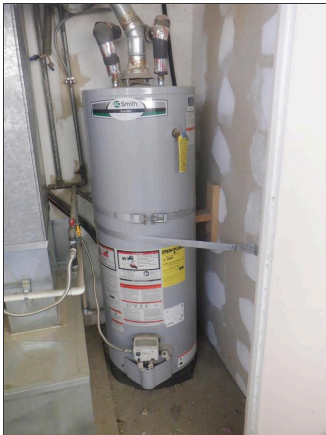
8.4 Item 1(Picture) Water Heater One Seismic Strap Only
