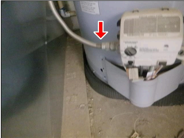
8.2 Item 3(Picture) Water Heater Fuel Line Missing Sediment Trap
