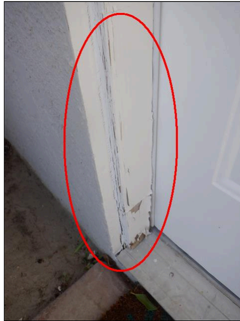
3.6 Item 2(Picture) Failing Trim Paint
