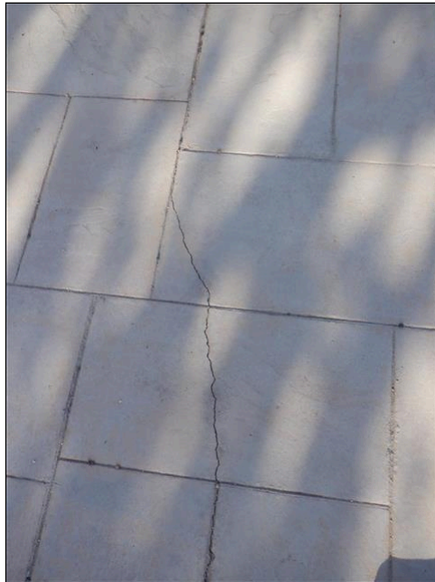
2.3 Item 4(Picture) Driveway Cracks
