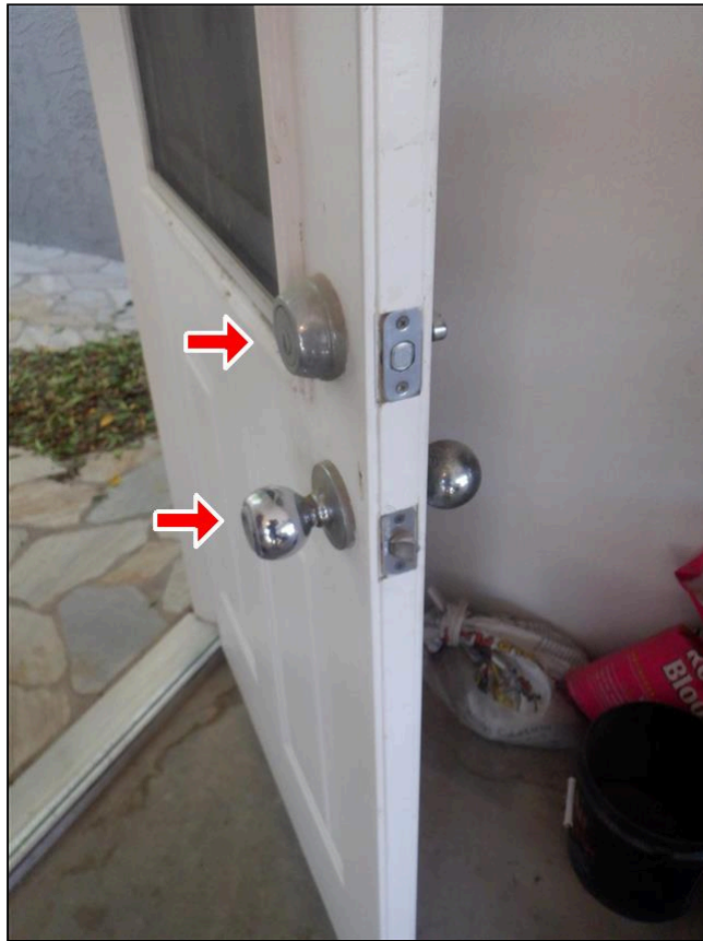
3.6 Item 5(Picture) Locks Not Functioning
