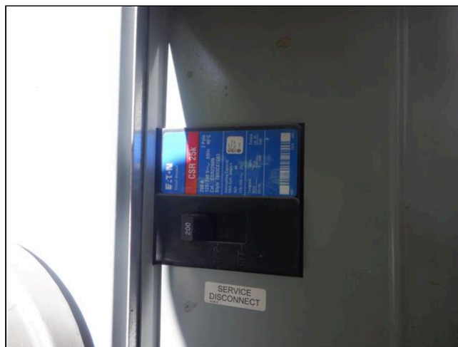
9.1 Item 2(Picture) Electrical Panel Disconnect 200 Amp
