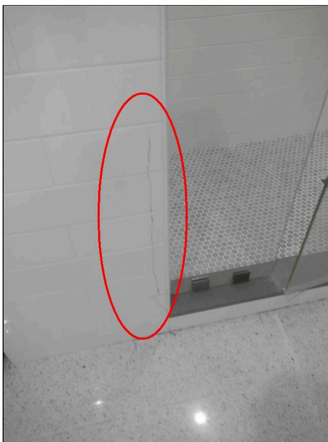
6.10.A Item 1(Picture) Damaged Tiles
