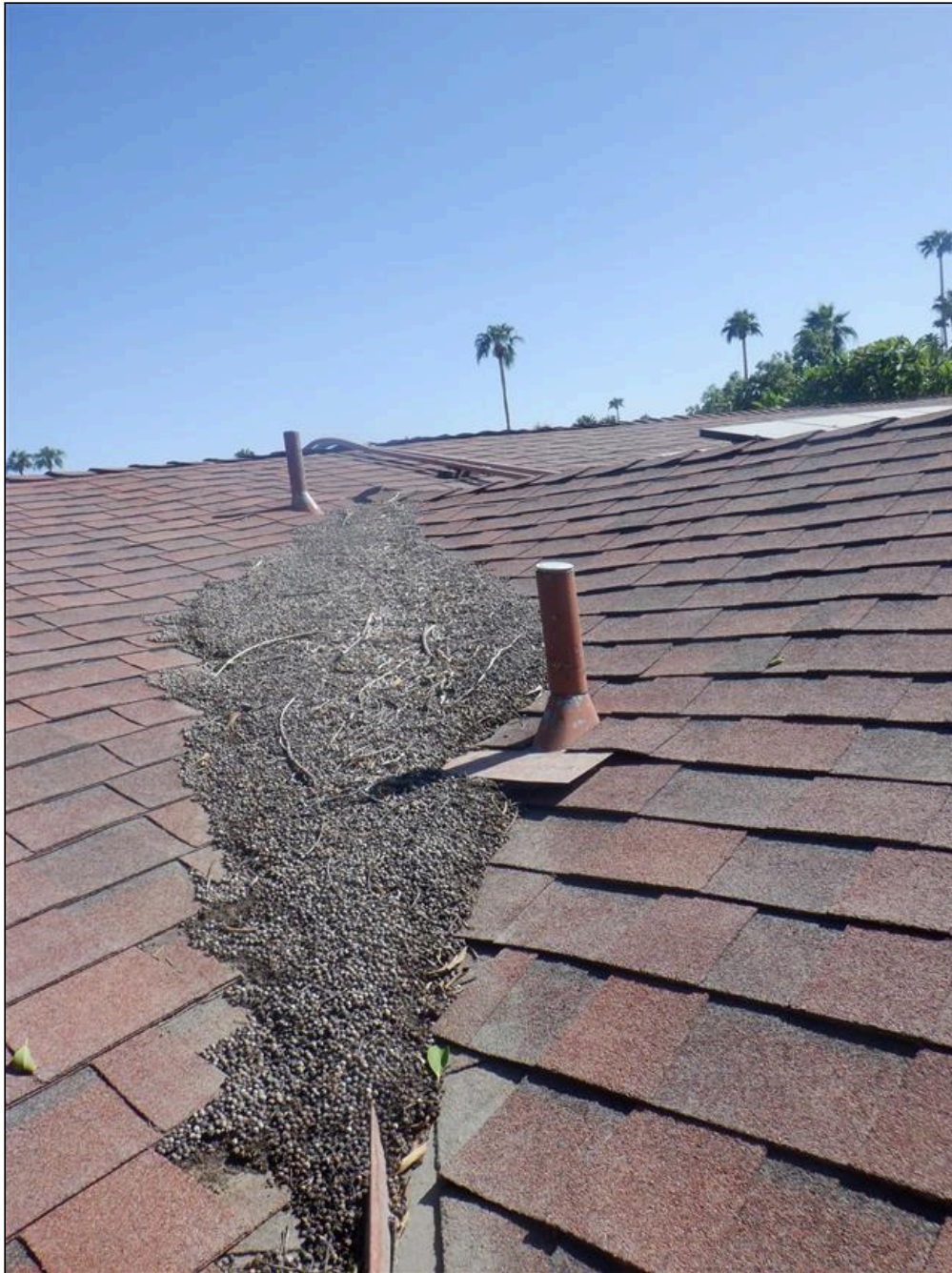
1.6 Item 2(Picture) Roof Debris
