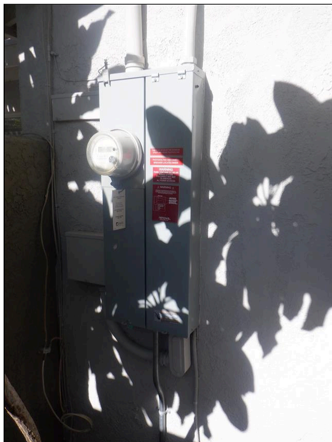
9.1 Item 1(Picture) Electrical Panel
