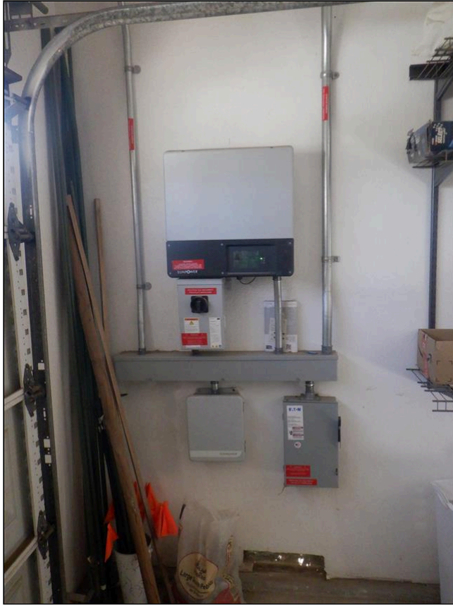
1.8 Item 3(Picture) Solar Equipment
