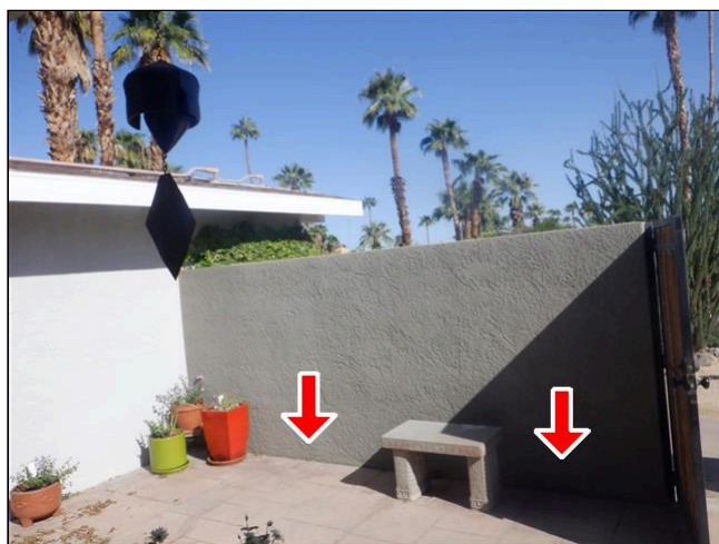
2.3 Item 12(Picture) Weep Holes Needed
