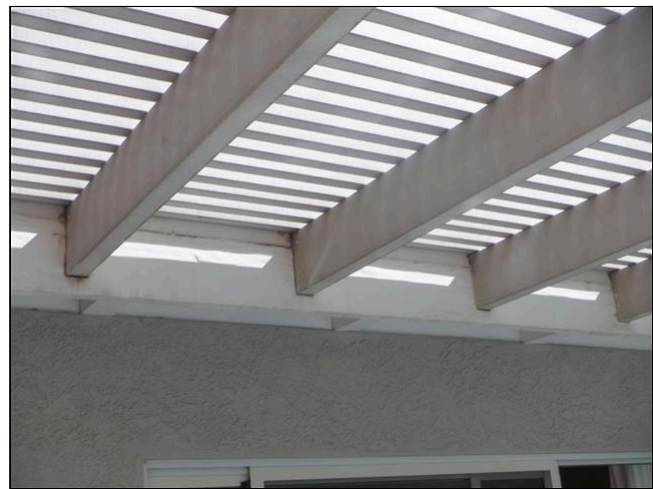
2.4 Item 6(Picture) Failing Paint
