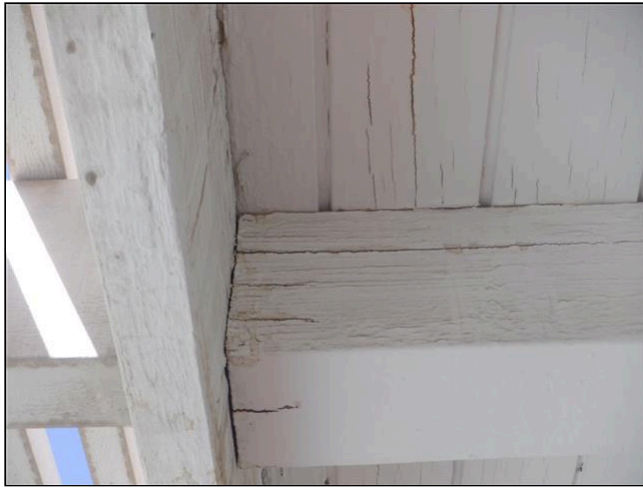
2.4 Item 4(Picture) Failing Paint
