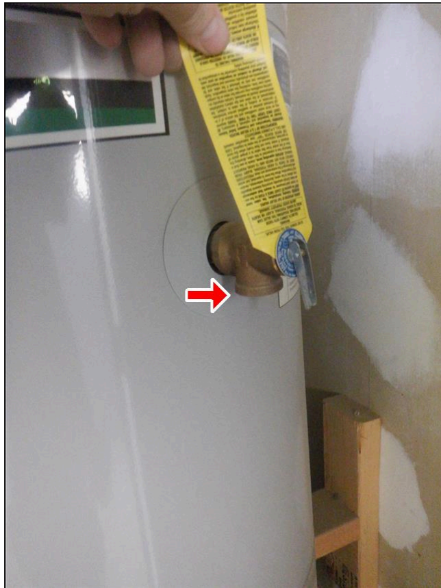
8.3 Item 1(Picture) Water Heater Missing TPR Valve Piping
