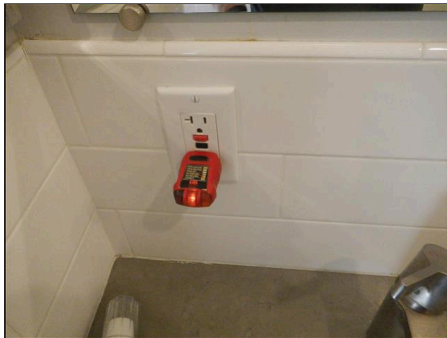
6.5.A Item 1(Picture) GFCI Not Functioning Properly
