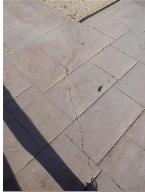
2.3 Item 6(Picture) Driveway Cracks
