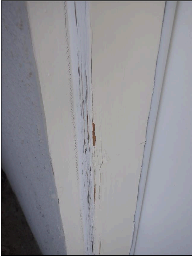
3.6 Item 3(Picture) Failing Trim Paint
