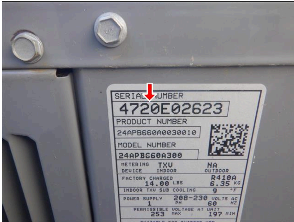
10.6 Item 2(Picture) Cooling Unit
