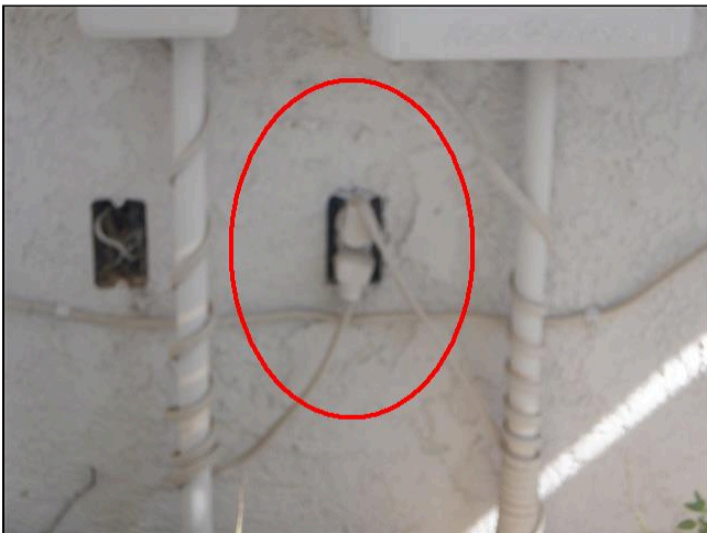
2.6 Item 1(Picture) Outlet No GFCI Protection
