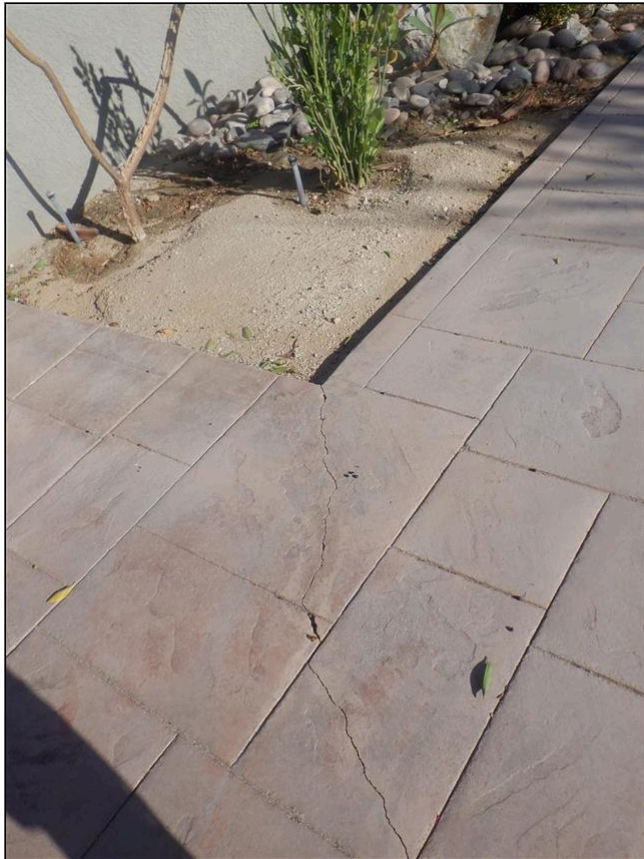
2.3 Item 5(Picture) Driveway Cracks
