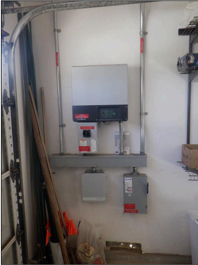
1.8 Item 3(Picture) Solar Equipment
