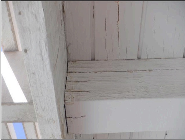
2.4 Item 4(Picture) Failing Paint
