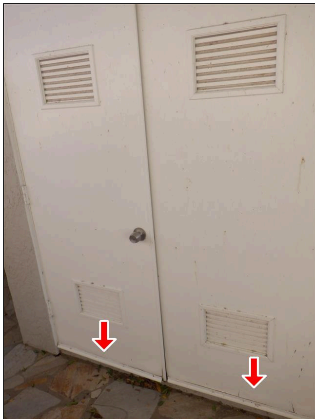
2.1 Item 1(Picture) Utility Room Doors Weathered
