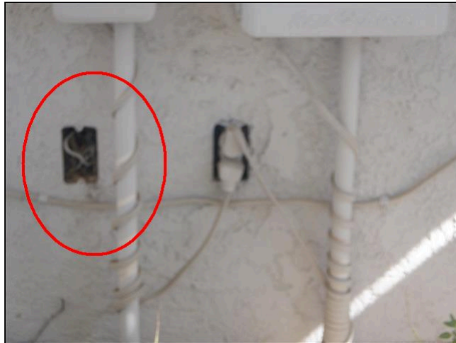
2.12 Item 1(Picture) Missing Cable Box Cover
