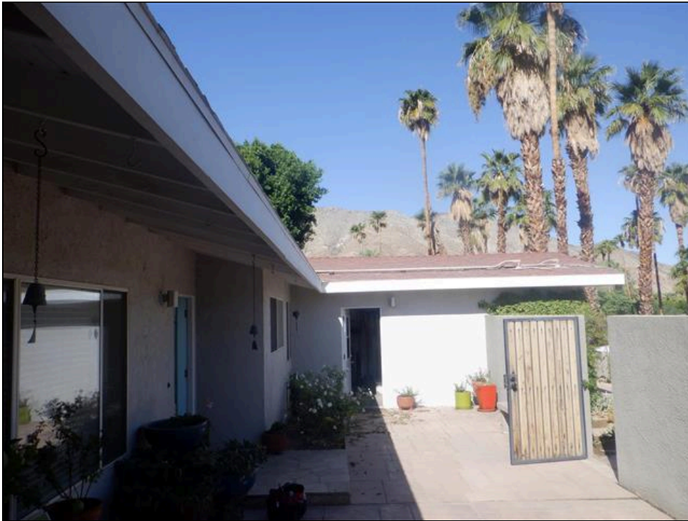
2.3 Item 11(Picture) Rain Gutters Needed
