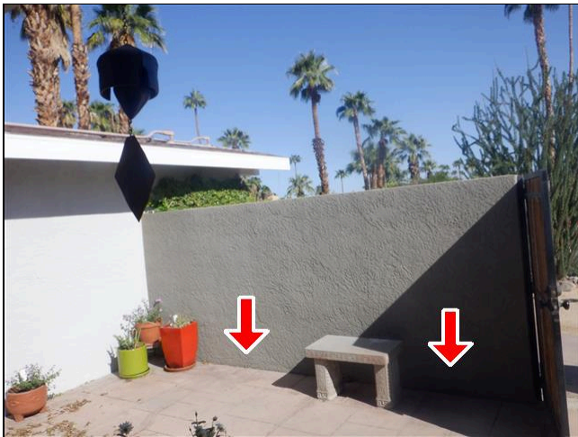
2.3 Item 12(Picture) Weep Holes Needed
