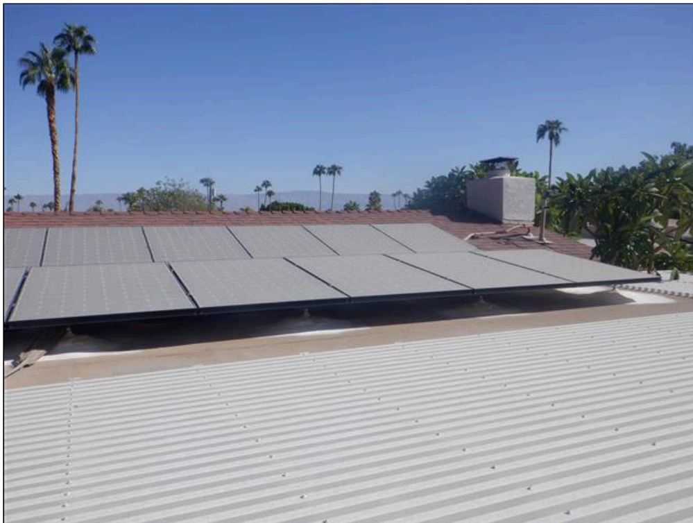
1.8 Item 2(Picture) Solar Panels
