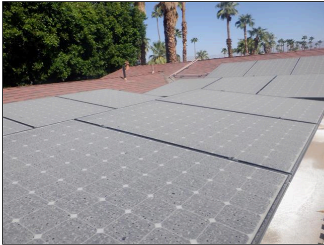
1.8 Item 1(Picture) Solar Panels
