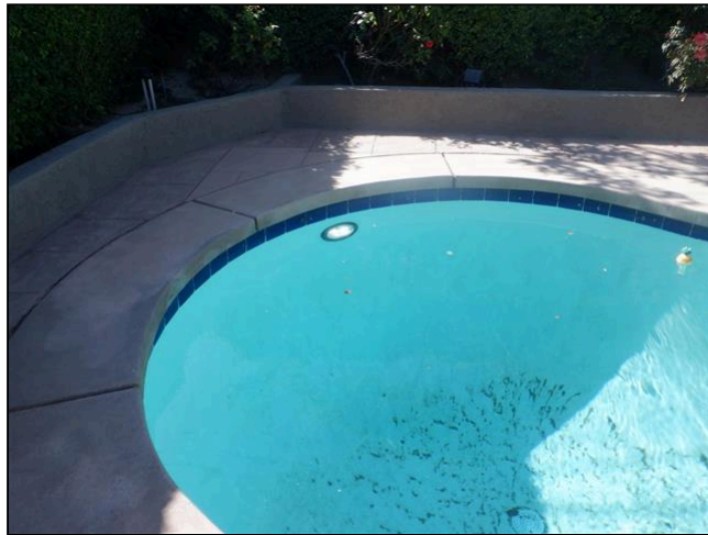
11.16 Item 1(Picture) Pool Light
