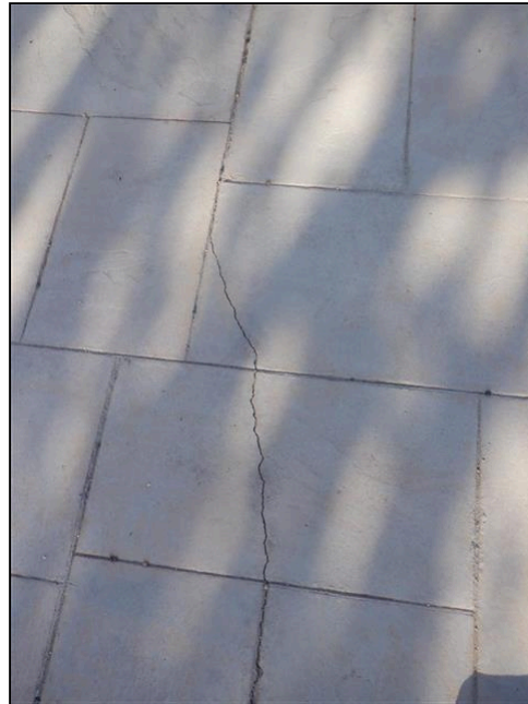
2.3 Item 4(Picture) Driveway Cracks
