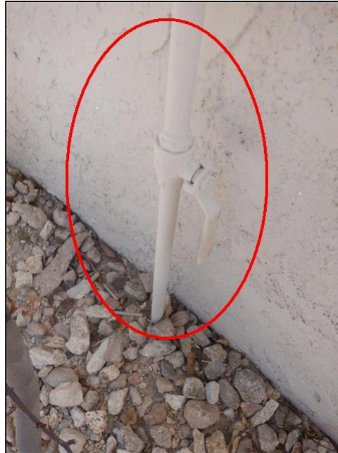
11.13 Item 2(Picture) Auto Fill Supply Missing Backflow Preventer
