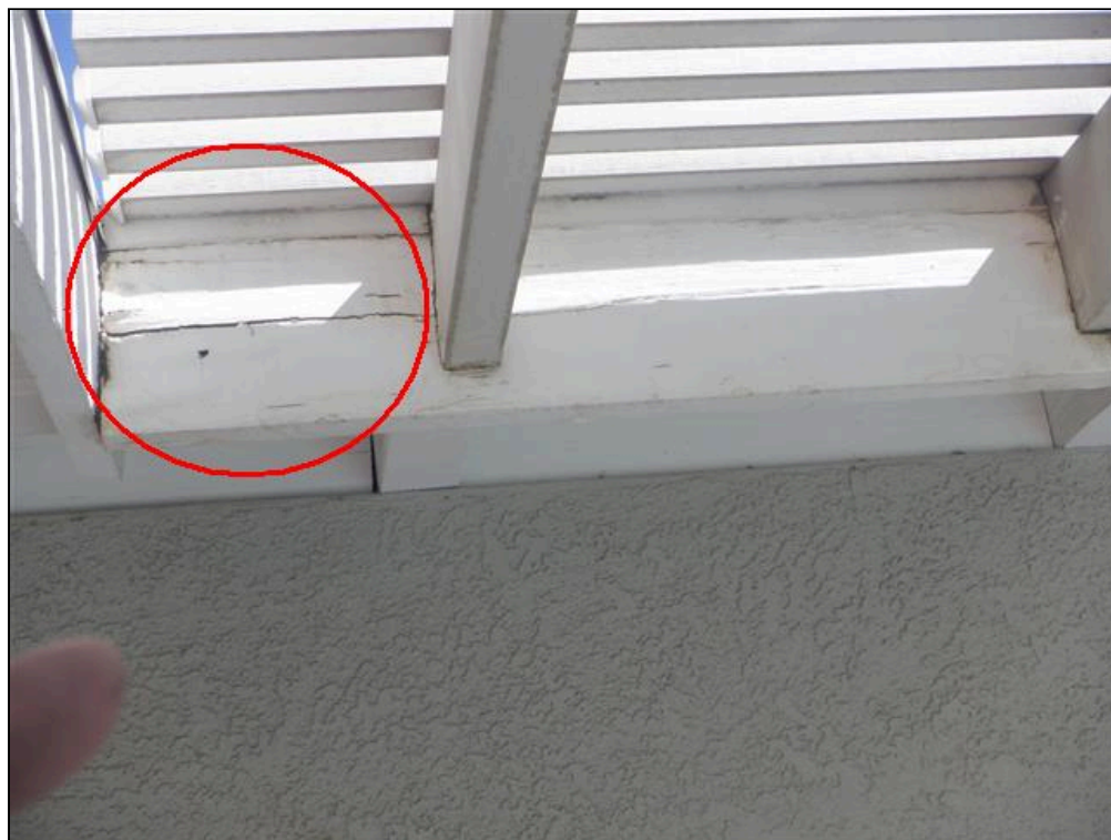
2.4 Item 1(Picture) Damaged Wood
