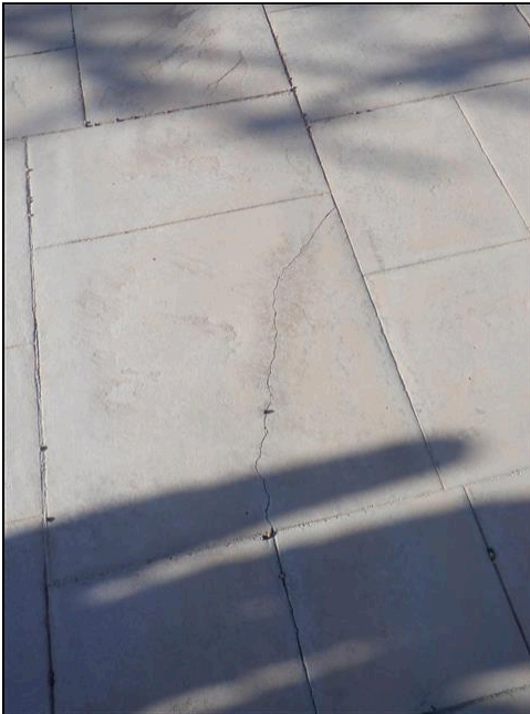
2.3 Item 3(Picture) Driveway Cracks
