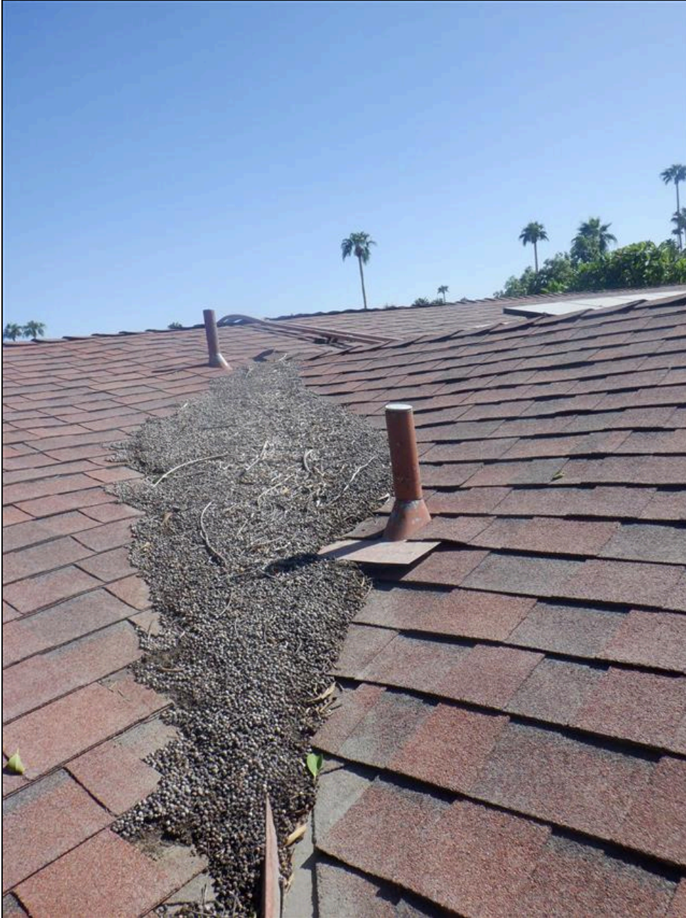
1.6 Item 2(Picture) Roof Debris
