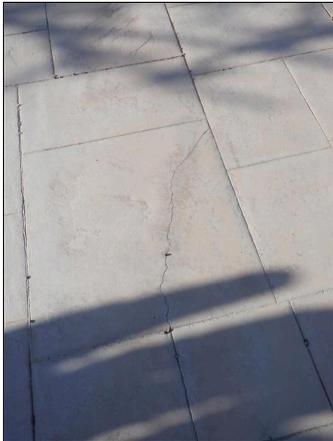
2.3 Item 3(Picture) Driveway Cracks
