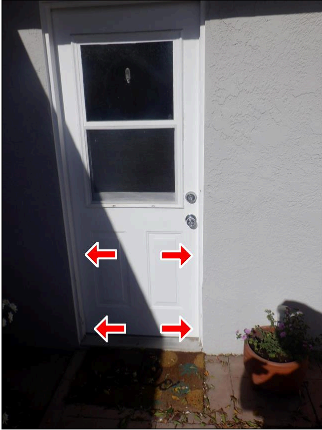
3.6 Item 1(Picture) Failing Trim Paint
