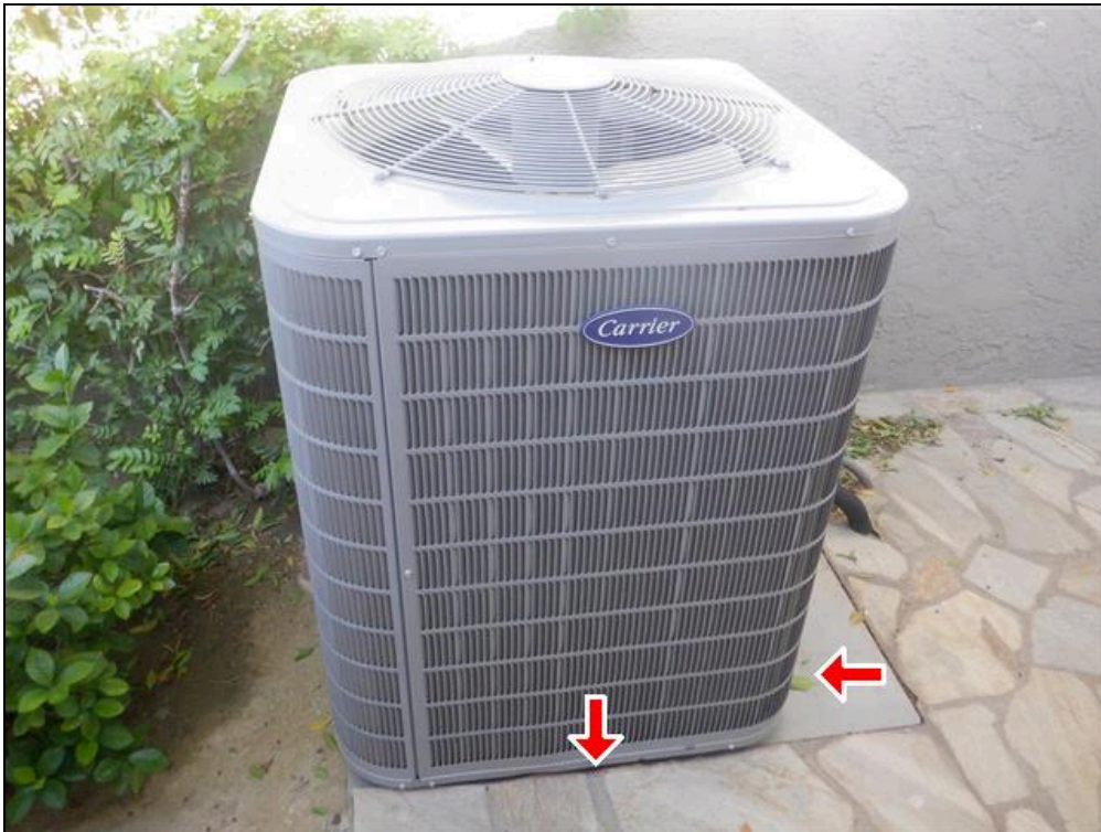
10.6 Item 1(Picture) Cooling Unit Not Secured
