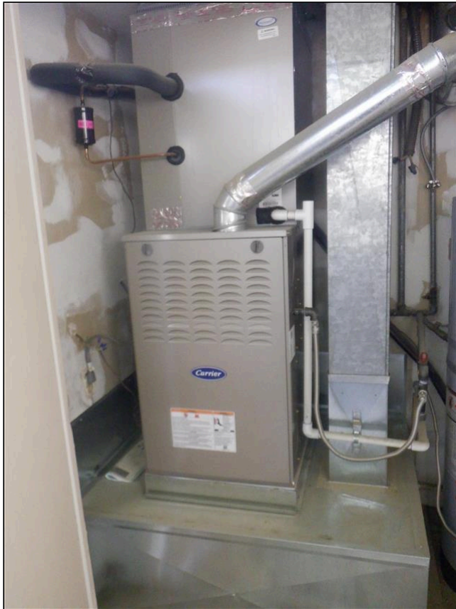
10.0 Item 1(Picture) Heating Unit
