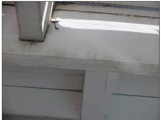
2.4 Item 3(Picture) Damaged Wood
