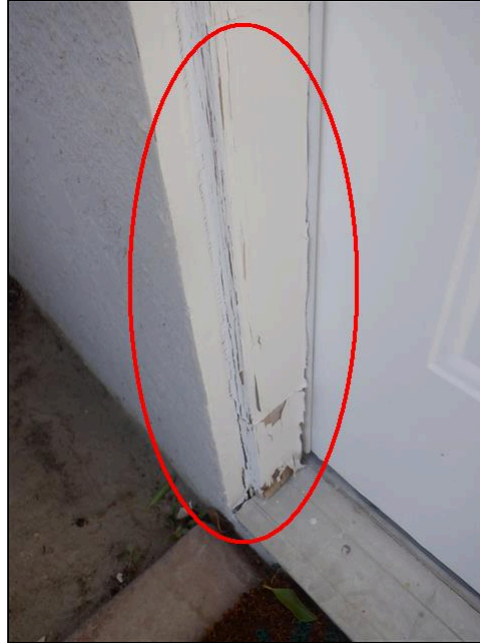
3.6 Item 2(Picture) Failing Trim Paint
