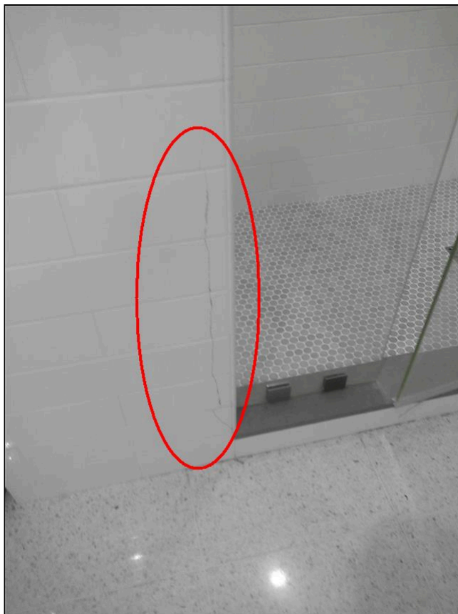
6.10.A Item 1(Picture) Damaged Tiles
