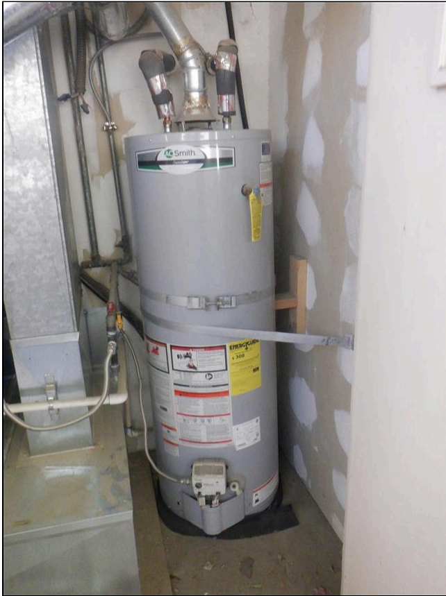
8.2 Item 1(Picture) Water Heater
