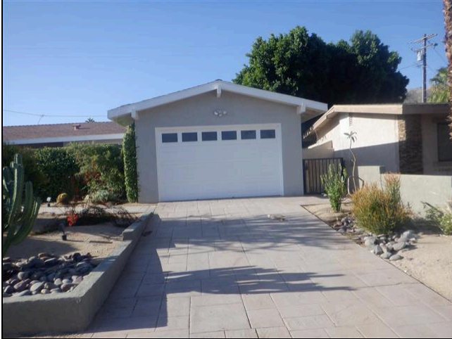
2.3 Item 1(Picture) Driveway Cracks
