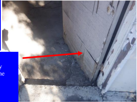
The garage shows significant offsets due to site conditions as illustrated by the floor cracks, tipped N-wall, etc.
