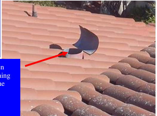
...the living room chimney flashing shows crude repairs...
