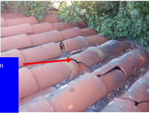
...and tile damage was noted...
