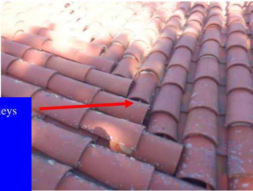
The home's roof contains moss that some insurance companies require be removed...
