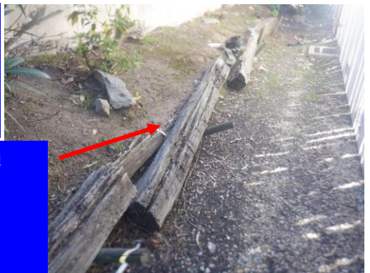
The S-property fencing is atop a buckled retaining wall...
