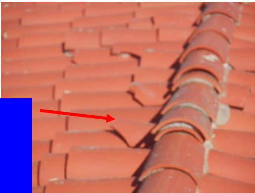
...the skylight's sloped side curb flashing pans terminate below tiles...
