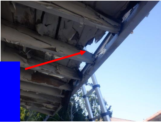
The garage roof has rotted through...
