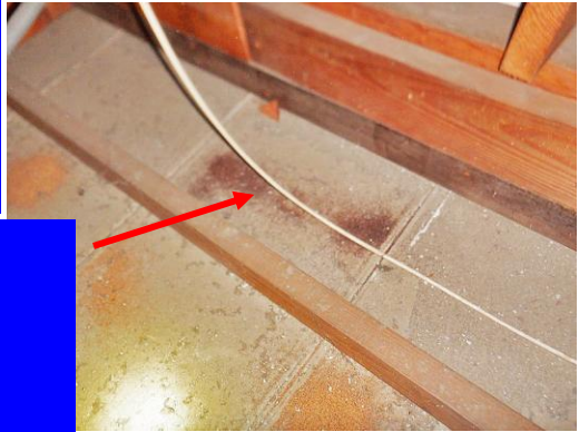
The attic also has termite droppings...
