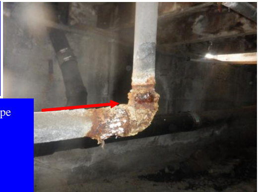
The original galvanized water supply piping shows extensive corrosion and leaks at the living room crawl space...
