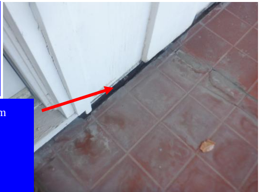
...while the entry stoop has split...
