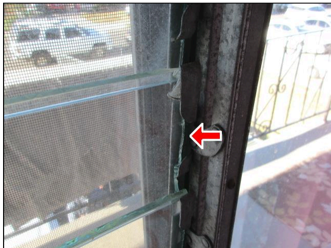
Chipped Glass, Unit D Living Room
