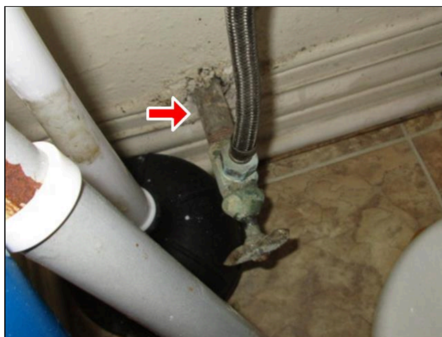
Old Galvanized Steel Piping In Use
