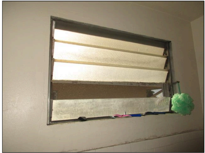
Missing Panel, Unit D Bath
