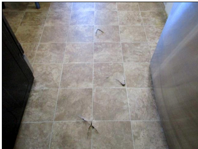
Damaged Floor, Unit C Kitchen
