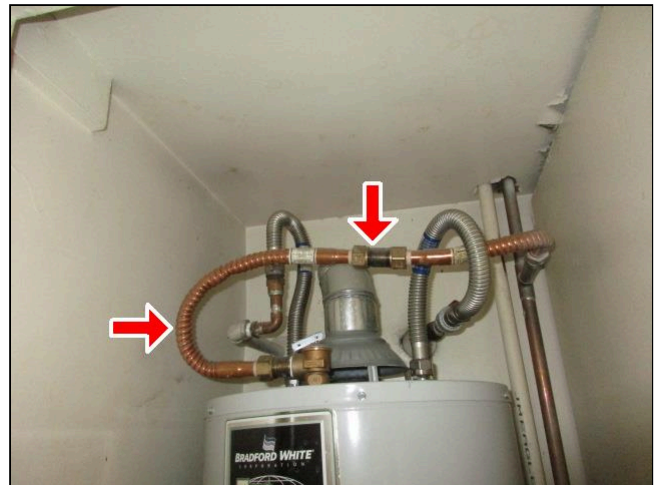
Piping Incorrectly Installed Upward, Unit A
