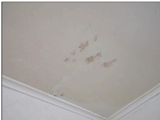
Suspected Mold/Fungus/Mildew, Unit B Bath
