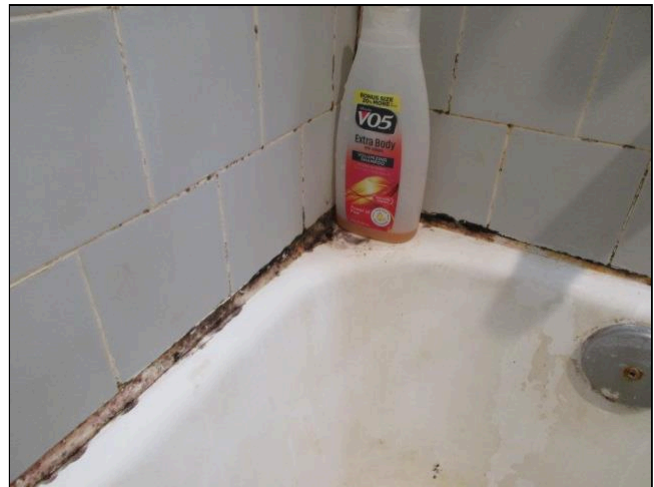
Suspected Mold/Fungus/Mildew, Unit B Bath
