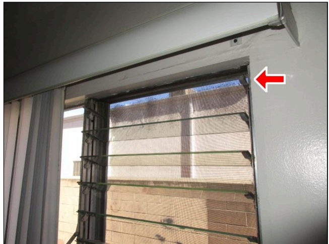
Missing Panel, Unit A
