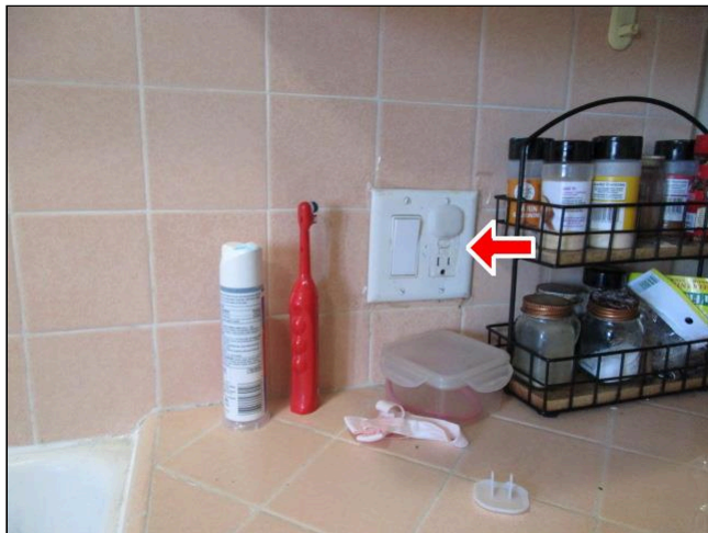
GFCI Outlet Not Operational
