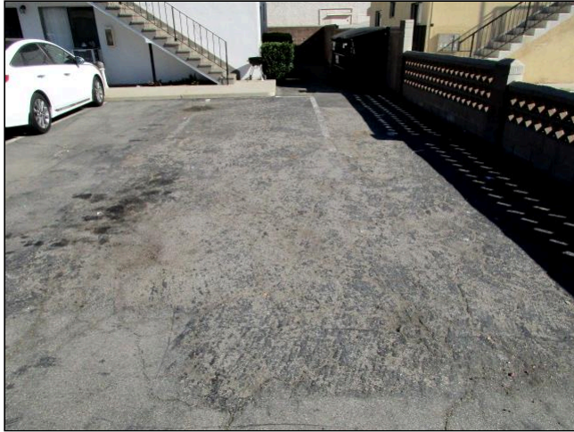
Worn, Deteriorated Drive
