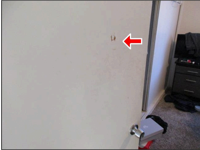
Damaged Door, Unit D
