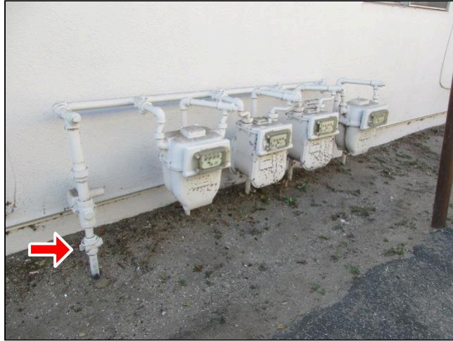
Main Gas Shut Off Valve
