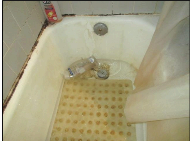
Slow Draining Tub, Unit B
