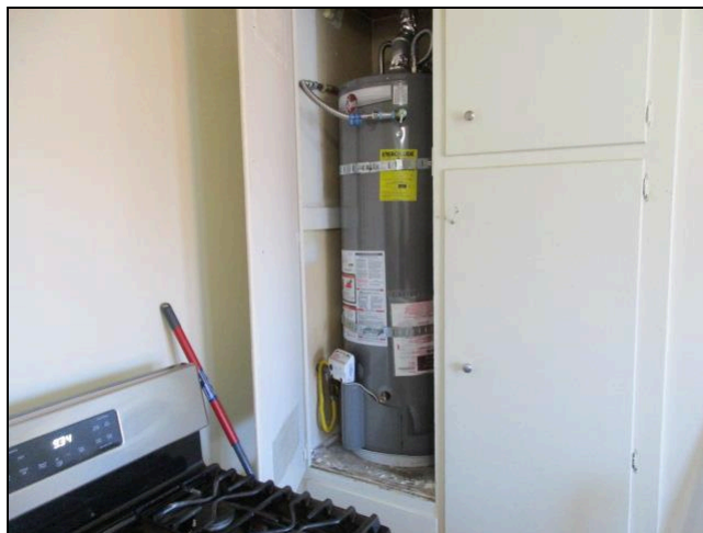
Water Heater, Unit C
