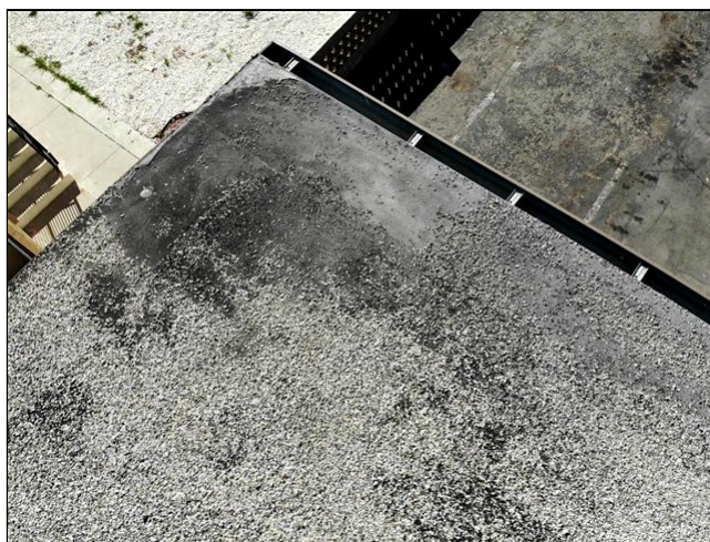
Missing Ballast, Cracked Roofing
