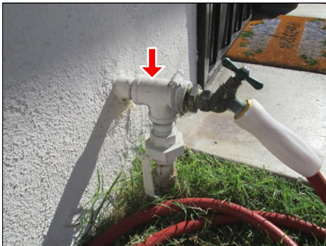
Old Galvanized Steel Piping In Use
