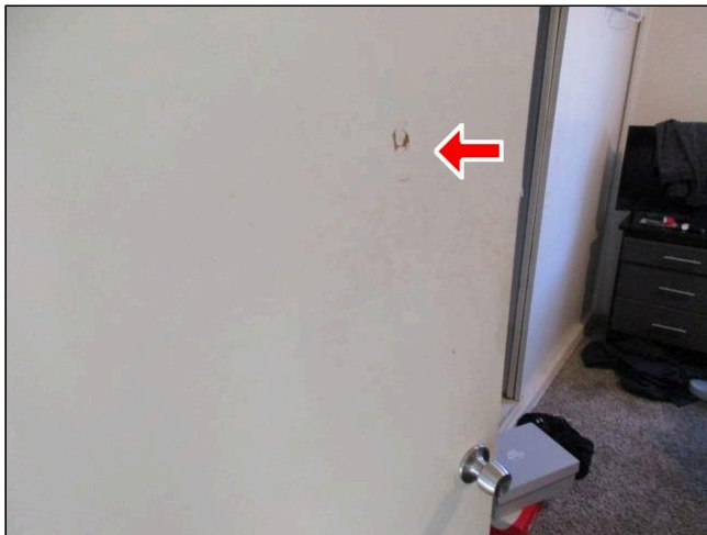
Damaged Door, Unit D
