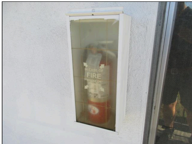
Extinguisher Certifications Expired
