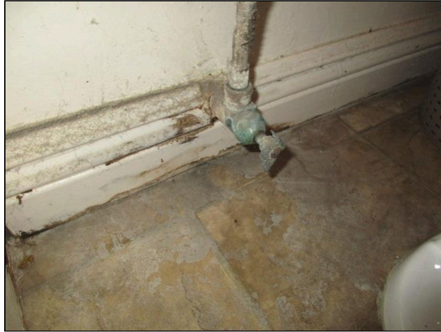
Stained, Damaged Baseboards
