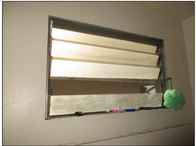
Missing Panel, Unit D Bath
