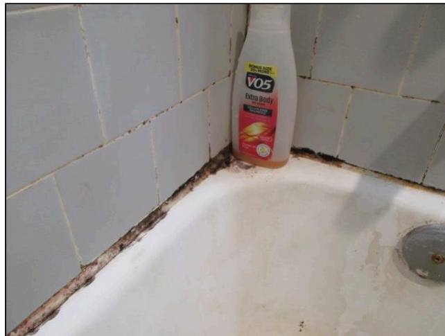
Suspected Mold/Fungus/Mildew, Unit B Bath
