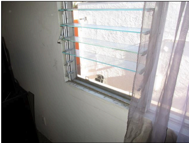
Missing Panels, Unit D Rear Bedroom
