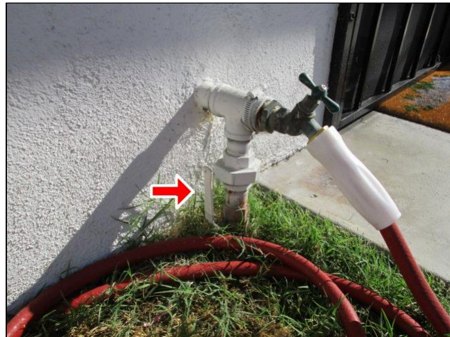
Water Shut Off Valve
