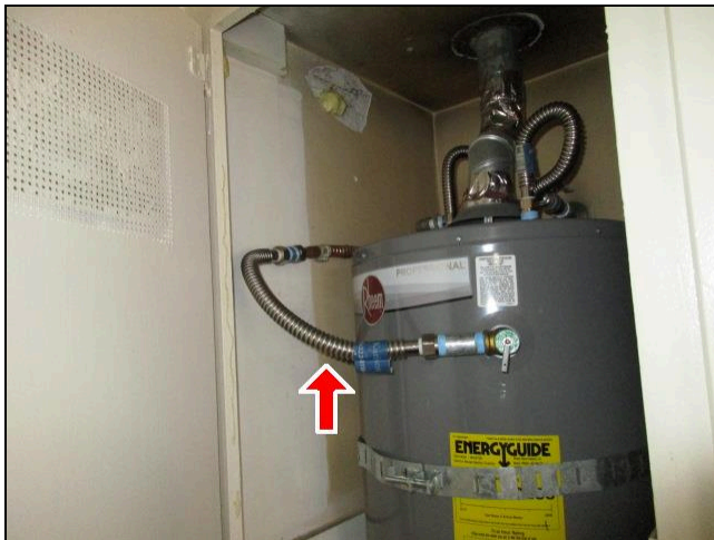
Piping Incorrectly Installed Upward, Unit C
