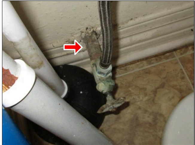
Old Galvanized Steel Piping In Use
