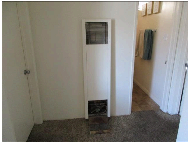
Old Water Heater Shut Off, Unit A
