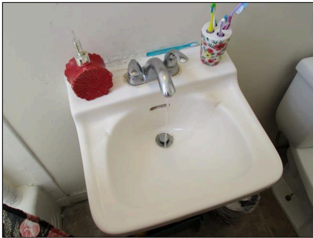
Loose Sink, Unit D
