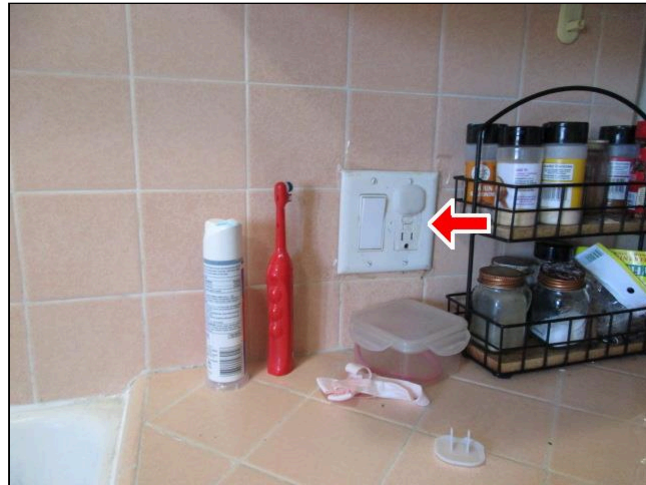
GFCI Outlet Not Operational
