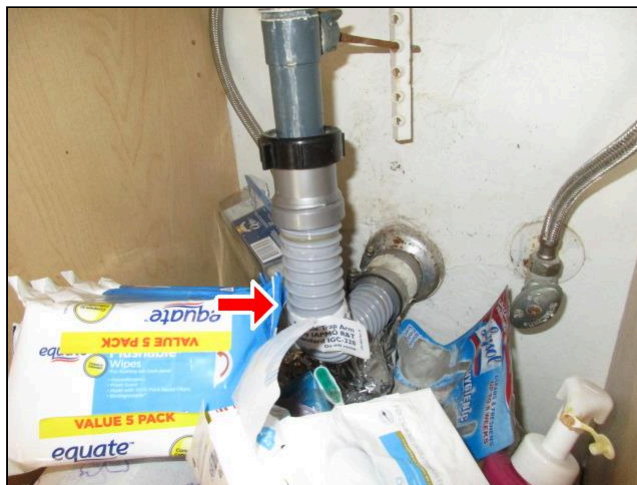
Improper Drain Repair
