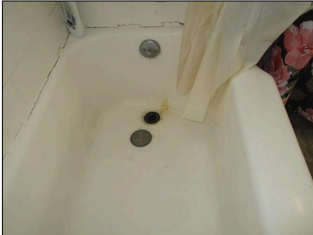
Slow Draining Tub, Unit D
