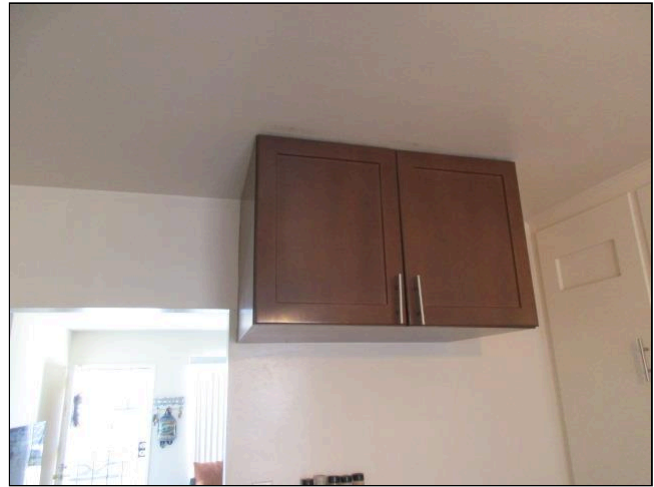
Gravity Vent Covered, Unit A
