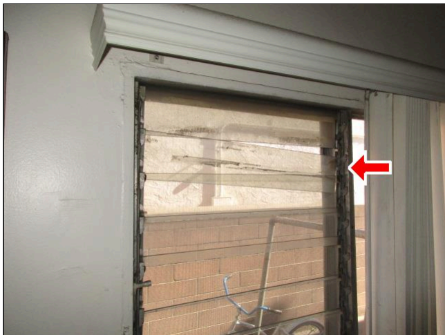
Loose Panel, Unit B Kitchen
