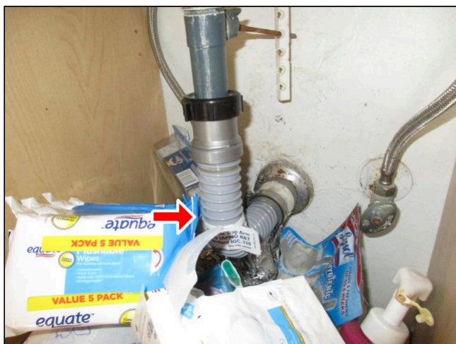
Improper Drain Repair
