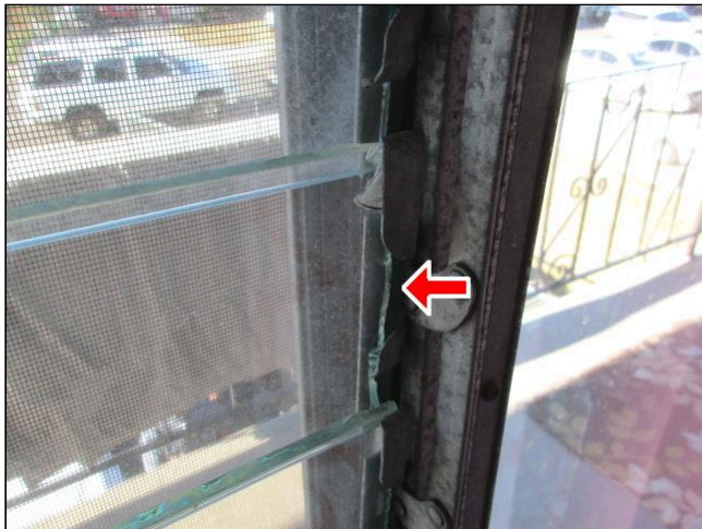
Chipped Glass, Unit D Living Room
