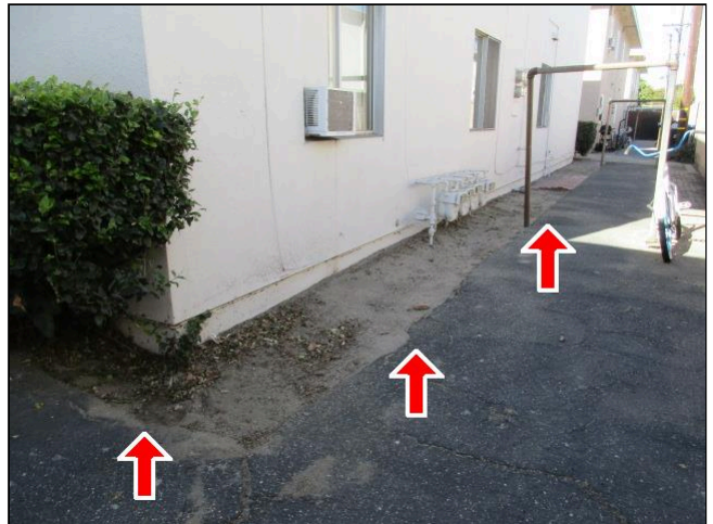
Poor Drainage Possible
