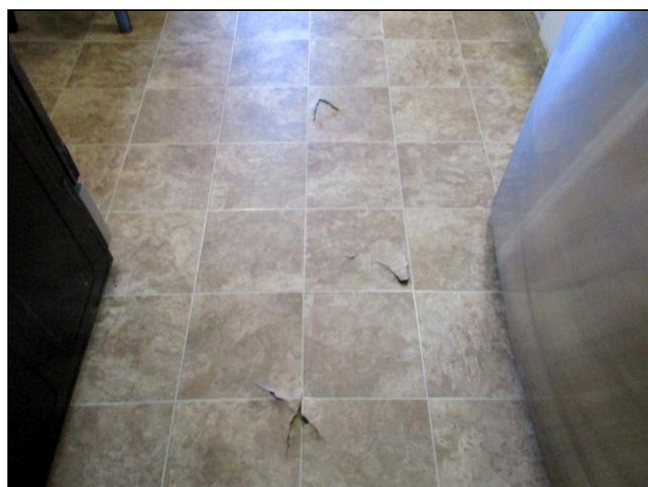
Damaged Floor, Unit C Kitchen
