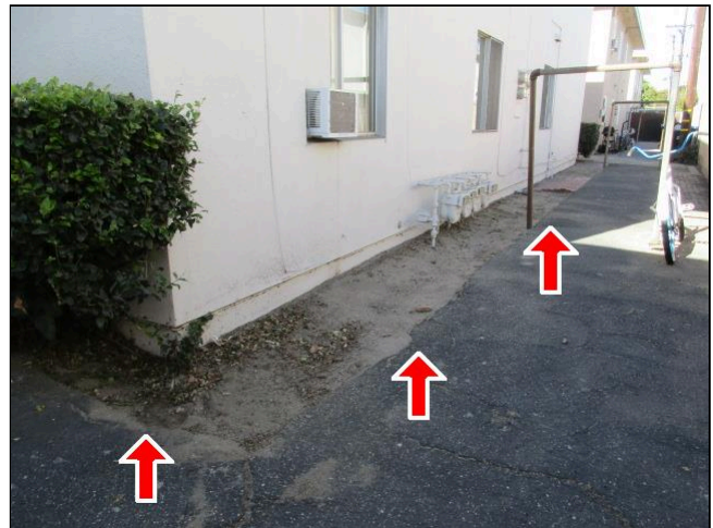
Poor Drainage Possible
