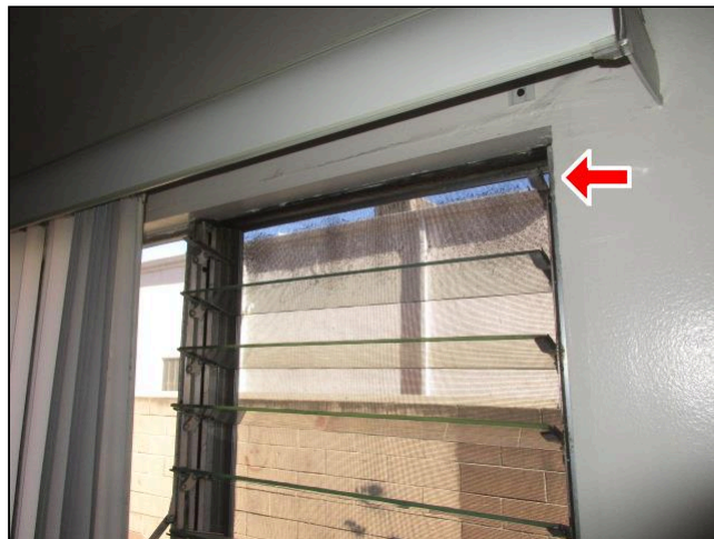
Missing Panel, Unit A
