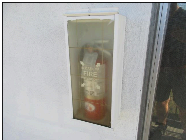
Extinguisher Certifications Expired
