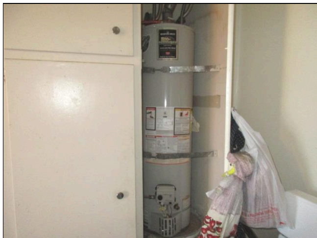
Water Heater, Unit D
