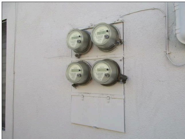
Electrical Disconnect Location
