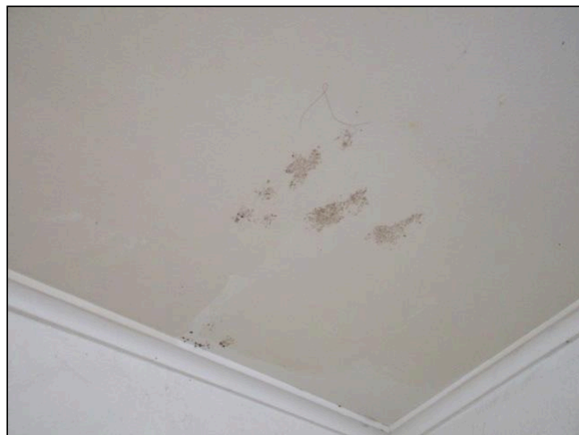
Suspected Mold/Fungus/Mildew, Unit B Bath
