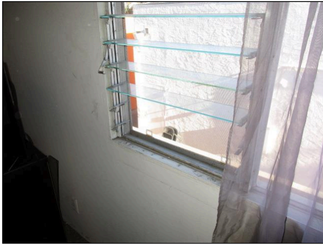
Missing Panels, Unit D Rear Bedroom
