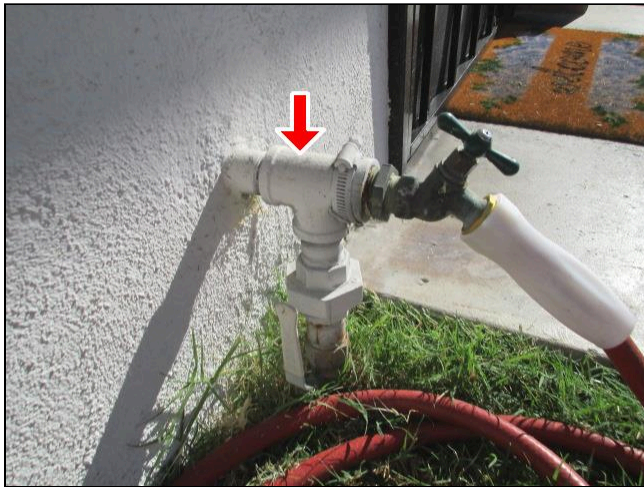
Old Galvanized Steel Piping In Use
