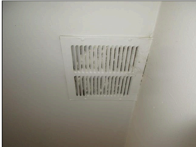
Gravity Vent Covered, Unit D
