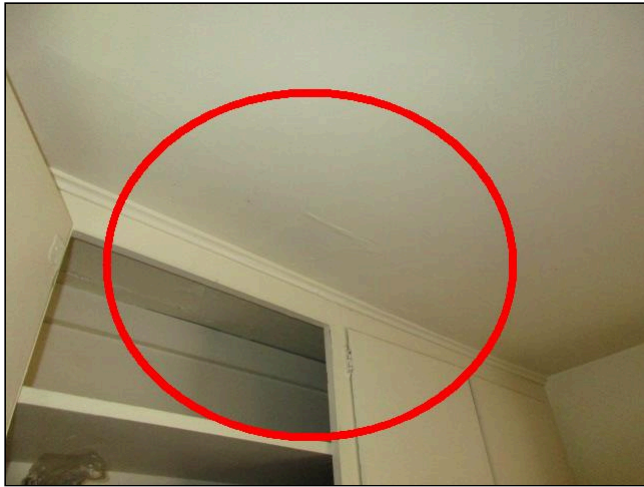
Damaged Ceiling, Unit B
