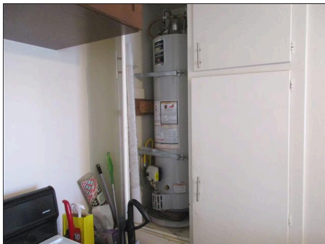
Water Heater, Unit A
