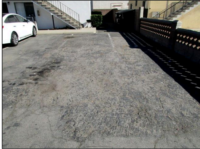
Worn, Deteriorated Drive
