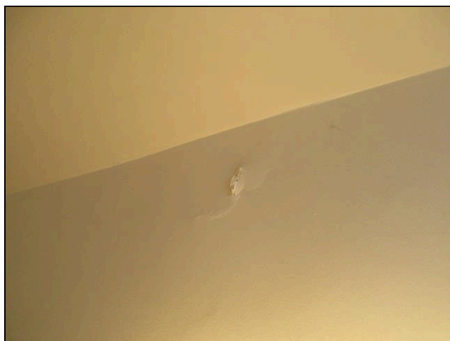
Damaged Wall, Unit A
