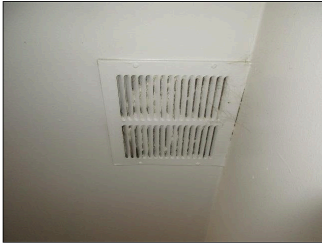
Gravity Vent Covered, Unit D
