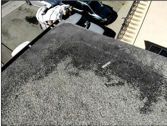
Missing Ballast, Cracked Roofing
