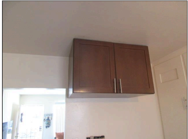
Gravity Vent Covered, Unit A
