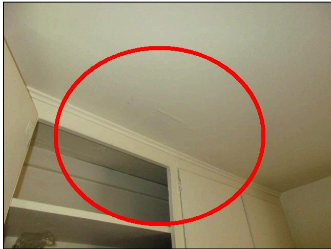
Damaged Ceiling, Unit B
