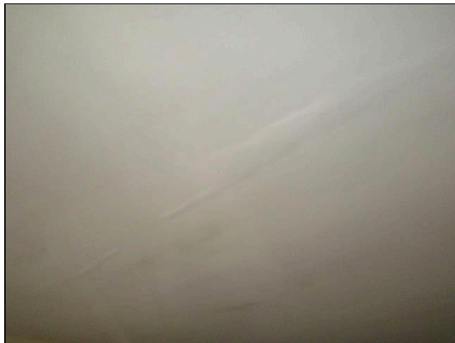
Damaged Ceiling, Unit D
