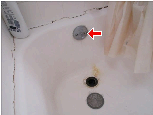
Stopper Not Operational, Unit D
