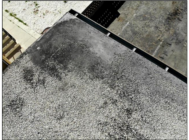
Missing Ballast, Cracked Roofing
