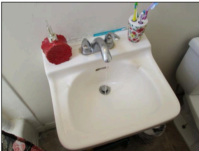
Loose Sink, Unit D
