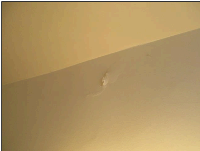
Damaged Wall, Unit A
