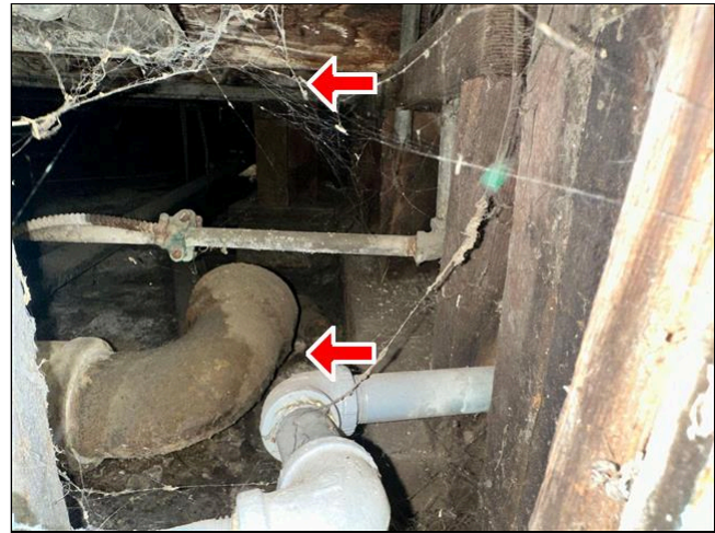
Item 21 - Item 2 (Picture) Plumbing System
