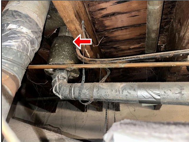
5.2 Item 2 (Picture) Plumbing System
