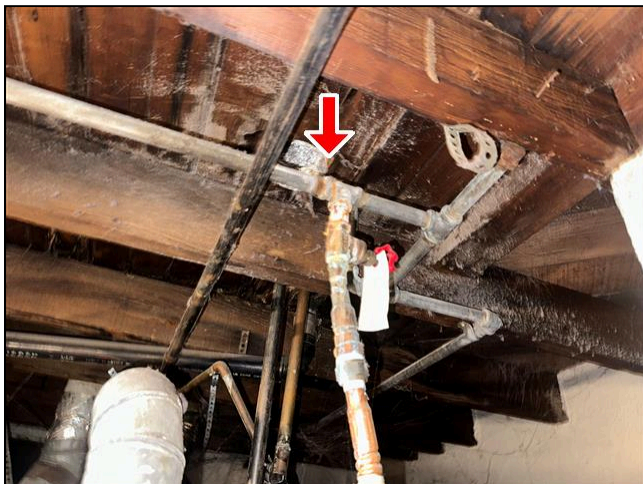
5.1 Item 2 (Picture) Plumbing System
