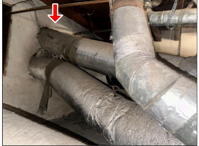
4.4 Item 2 (Picture) Heating/Central Air
