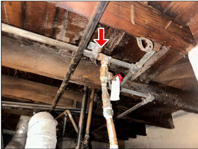
Item 24 - Item 1 (Picture) Plumbing System
