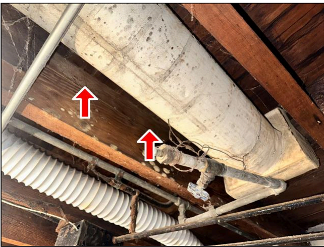
Item 19 - Item 3 (Picture) Heating/Central Air
