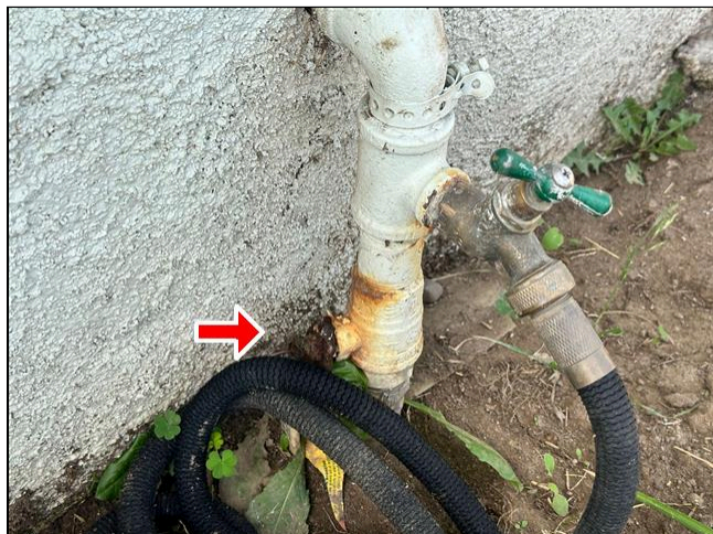
5.1 Item 3 (Picture) Plumbing System
