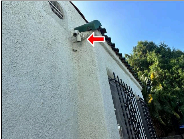
6.2 Item 2 (Picture) Electrical System
