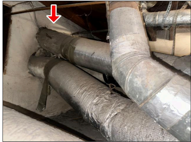
Item 19 - Item 2 (Picture) Heating/Central Air
