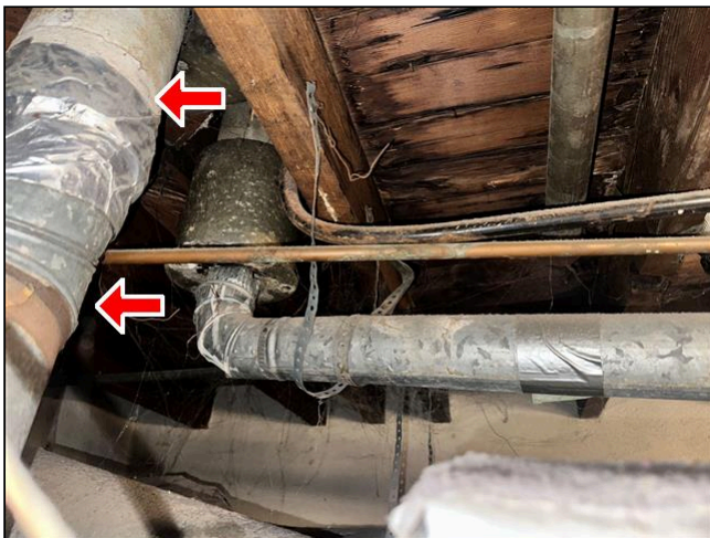
Item 17 - Item 1 (Picture) Heating/Central Air
