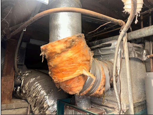
4.4 Item 1 (Picture) Heating/Central Air
