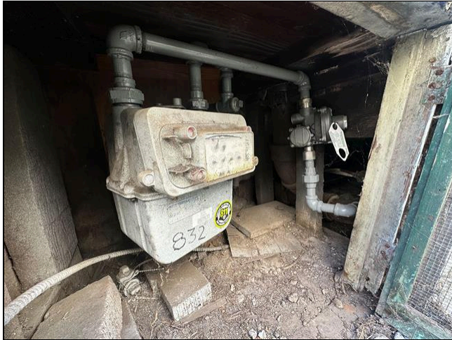
5.5 Item 1 (Picture) Plumbing System
