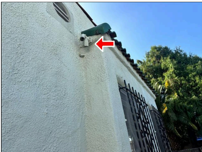
Item 27 - Item 1 (Picture) Electrical System
