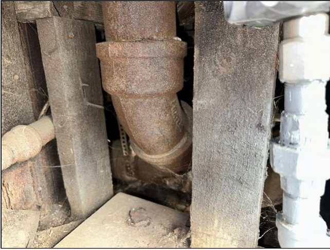
Item 20 - Item 1 (Picture) Plumbing System
