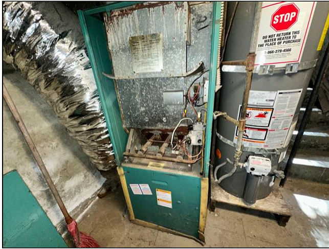
4.0 Item 1 (Picture) Heating/Central Air
