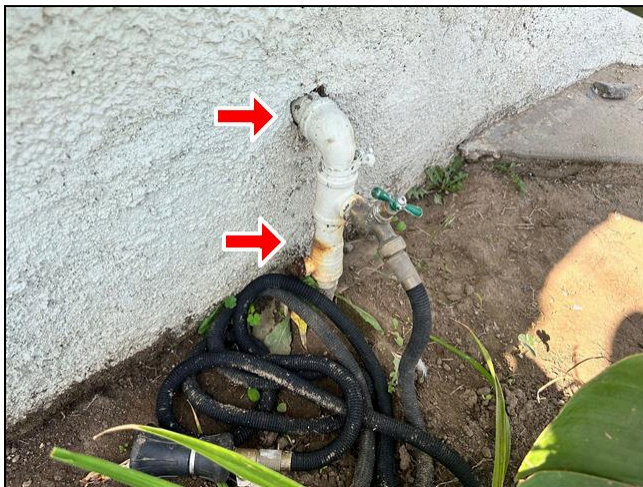
5.1 Item 1 (Picture) Plumbing System
