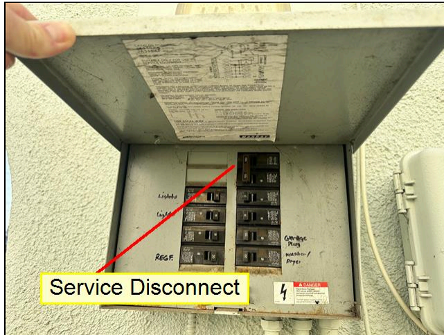
6.4 Item 1 (Picture) Electrical System
