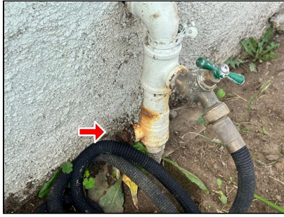
5.6 Item 1 (Picture) Plumbing System
