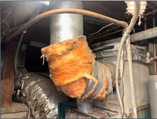
Item 19 - Item 1 (Picture) Heating/Central Air
