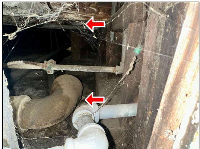
5.0 Item 3 (Picture) Plumbing System
