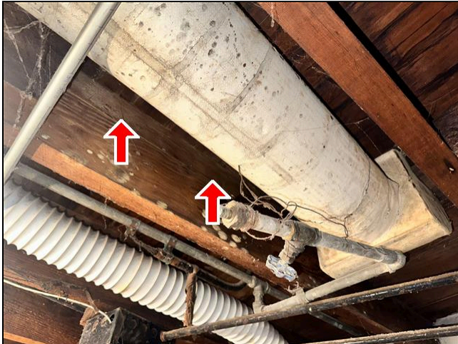
4.4 Item 3 (Picture) Heating/Central Air
