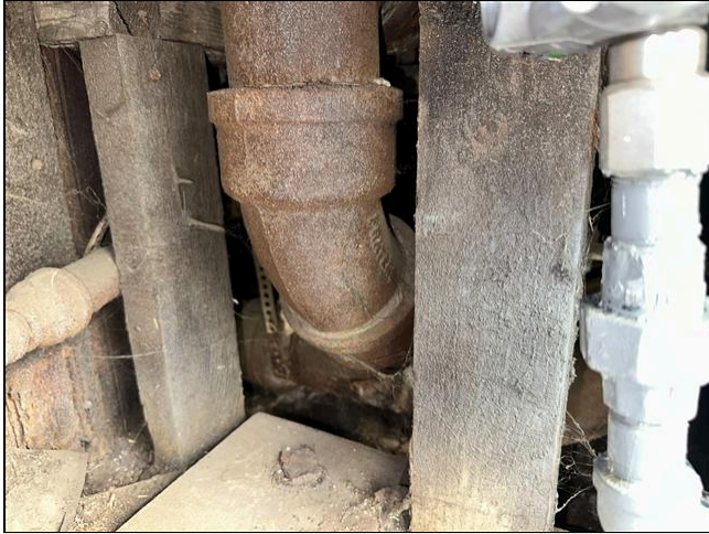
5.0 Item 1 (Picture) Plumbing System
