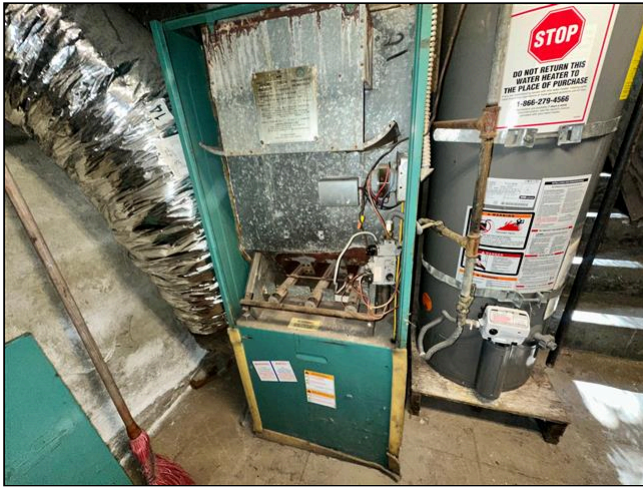
Item 16 - Item 1 (Picture) Heating/Central Air Flues and Vents (for gas heating systems)
