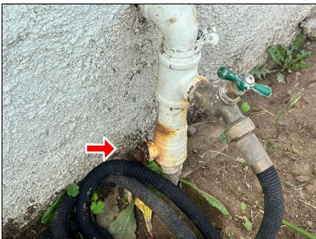
Item 25 - Item 1 (Picture) Plumbing System
