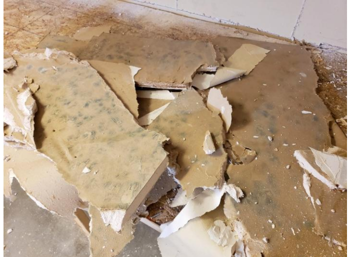
2. Mold Contaminated drywall
