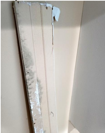
16. Mold contaminated baseboard
