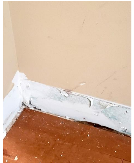
18. Fungal growth on the north wall
