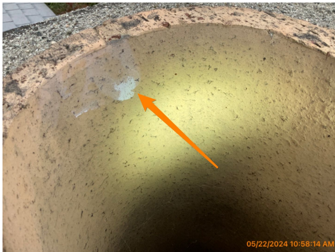
Efflorescence in flue
