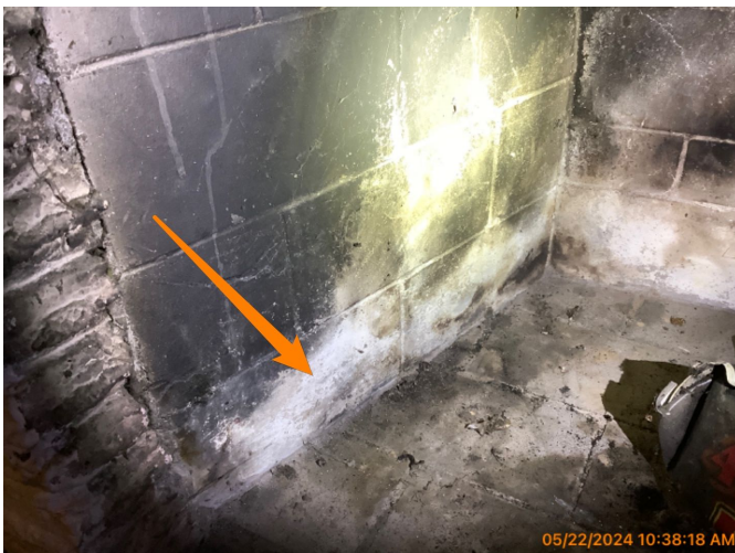
Efflorescence in firebox
