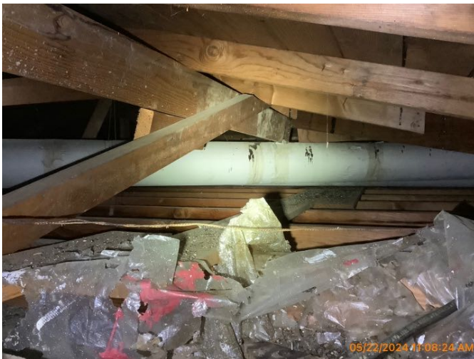
No catwalk and low clearances in attic space
