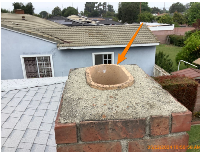
Spark arrester rain cap missing
