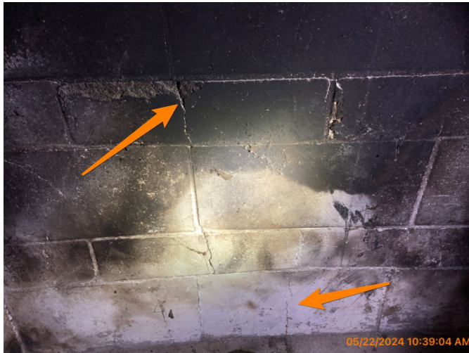
Cracks in firebox back wall
