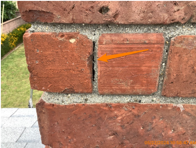
Deteriorated grout above roof
