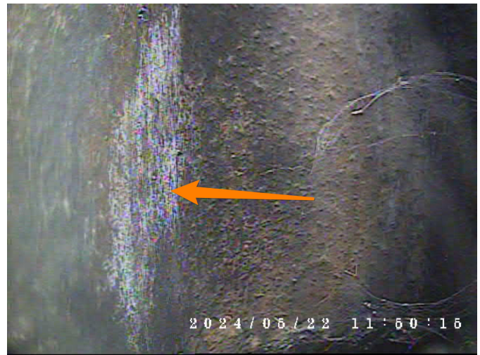
Efflorescence in flue
