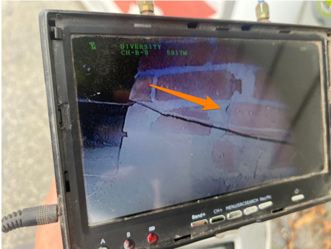
Deteriorated grout at base of chimney
