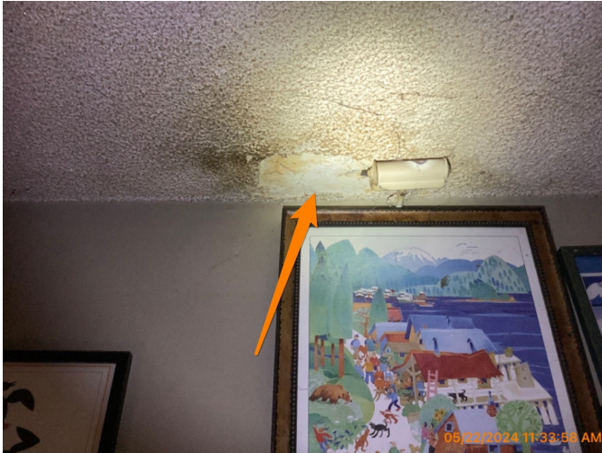
Moisture stain above firebox
