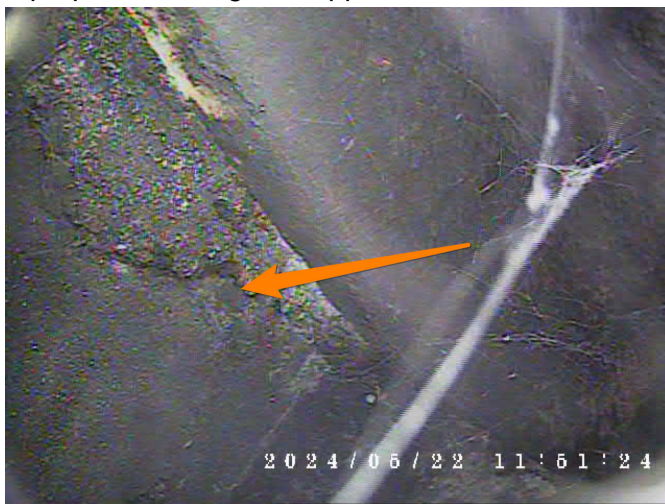
Smoke chamber surfaces worn
