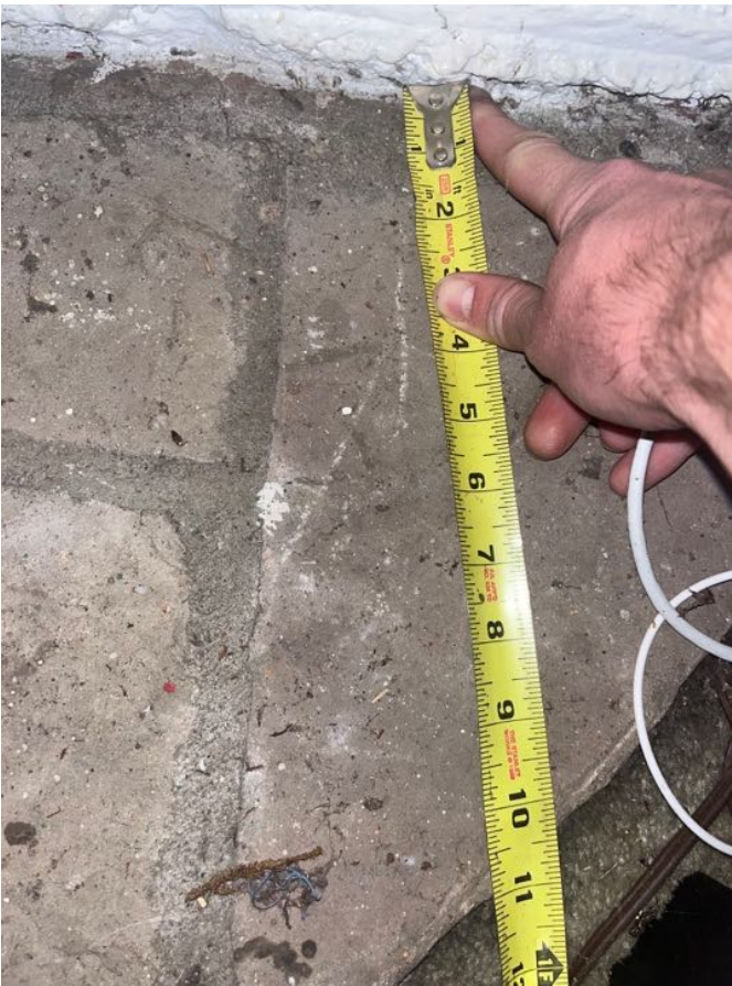
Hearth extension depth as measured 12 inches from the right of the firebox opening
