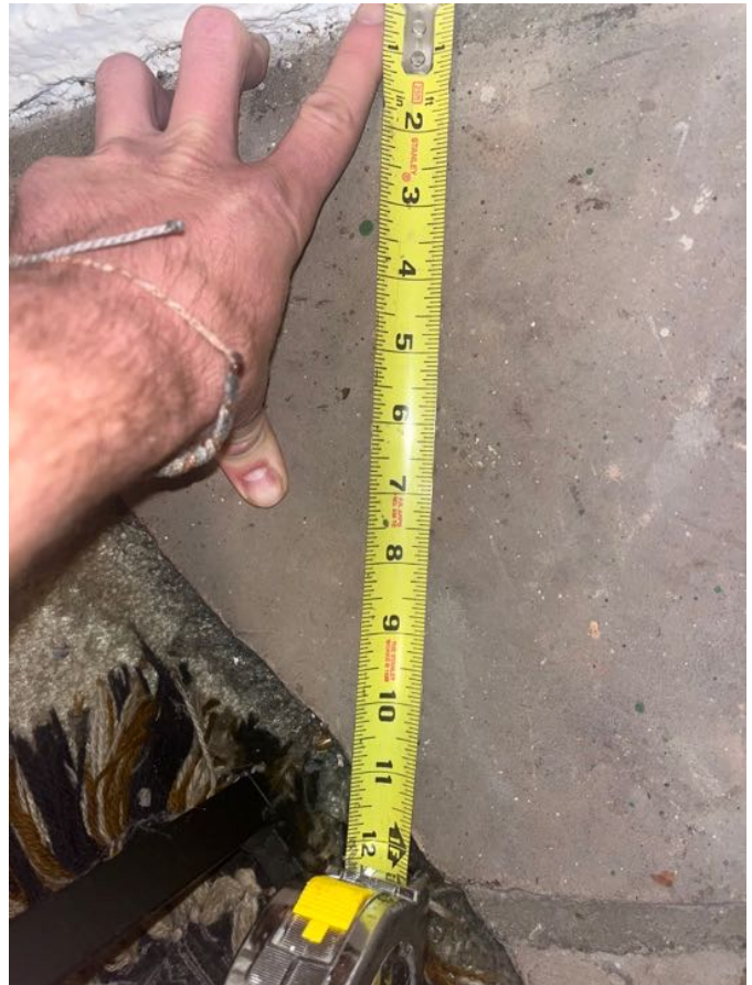
Hearth extension depth as measured 12 inches from the left of the firebox opening
