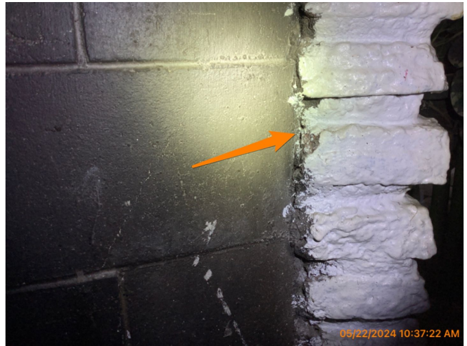
Gap in surround
