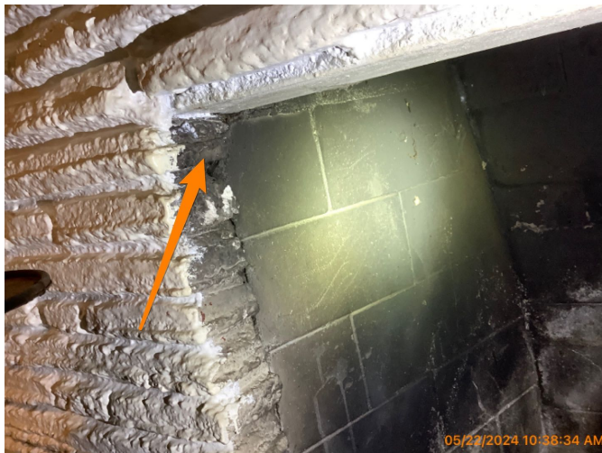
Smoke stains near outside of firebox
