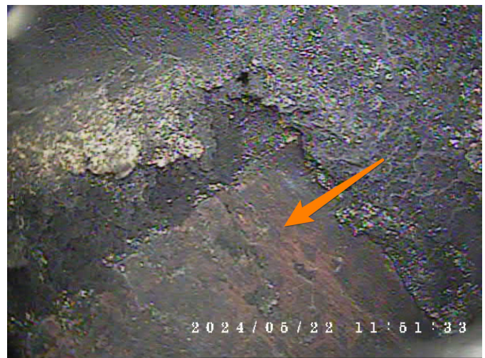
Smoke chamber surfaces worn
