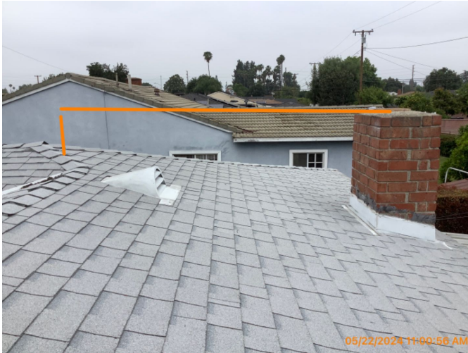
Chimney slightly too short
