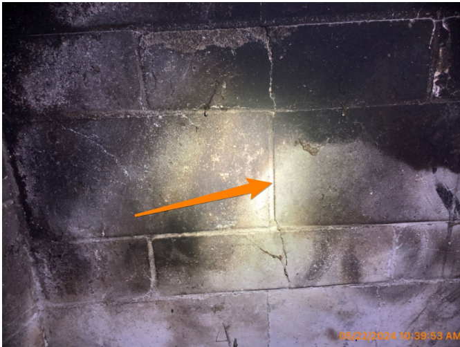
Slight gap in back wall
