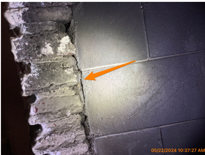
Gap in surround
