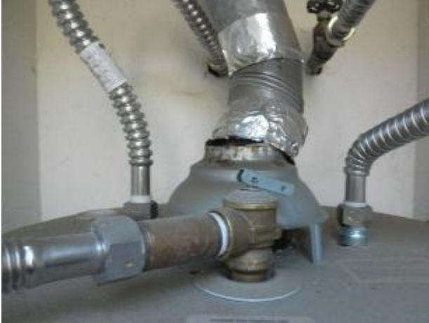
The exhaust vent has separated at the top of the water heater.
