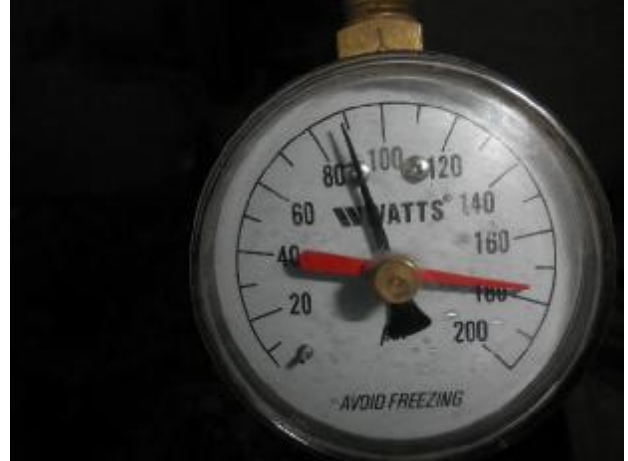
The water pressure exceeds the maximum allowable of 80 psi.
